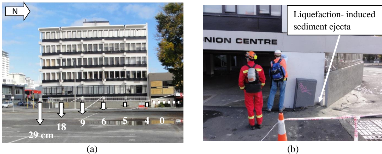
Figure 4-18. Building undergoing significant liquefaction-induced differential settlement due to part of it being founded on the liquefaction feature in this area (24 Mar 2011; -43.52878^\circ , 172.64252^\circ ).
