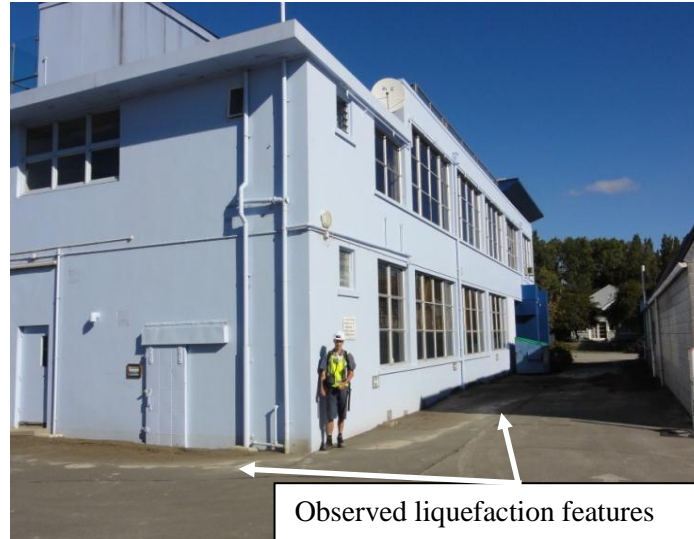
Figure 4-15. Two-story building that underwent liquefaction-induced punching movements (7 Mar 2011; -43.52506^\circ , 172.64176^\circ ).
