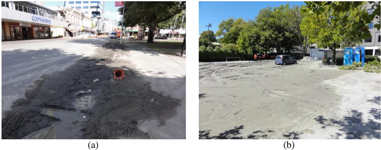
Figure 4-11. Representative areas of: (a) moderate liquefaction (7 Mar 2011; -43.52791^{\circ} , 172.63653^{\circ} ), and (b) severe liquefaction within the CBD principal liquefaction zone (4 Mar 2011; -43.52604^{\circ} , 172.63839^{\circ} ).
