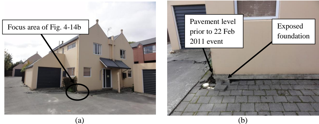
Figure 4-14. Duplex housing complex: (a) looking north at center building, and (b) close-up of ground settlement next to center building (16 Mar 2011; -43.52399^{\circ} , 172.64417^{\circ} ).
