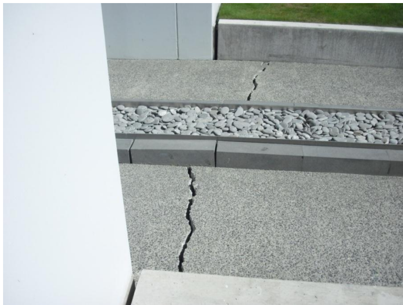
Figure 5-4. Differential settlement along concrete walkway between patios and surrounding ground north of the building. (-43.5577°, 172.7066°)
