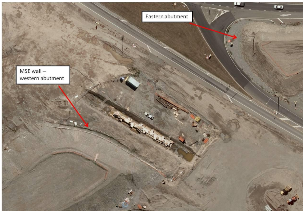
Figure 5-19. Aerial view of Curletts Rd interchange western abutment MSE wall in early stages of construction. (-43.5478°, 172.5789°)
