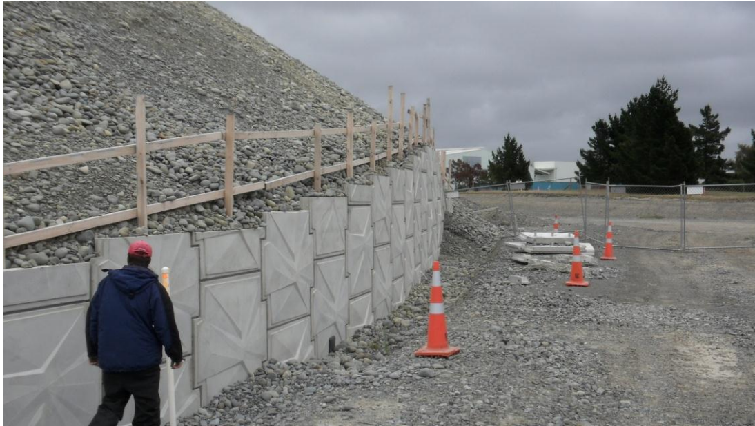
Figure 5-20. Partial construction of the MSE walls for the Curletts Rd interchange western abutment. (-43.5478°, 172.5789°)
