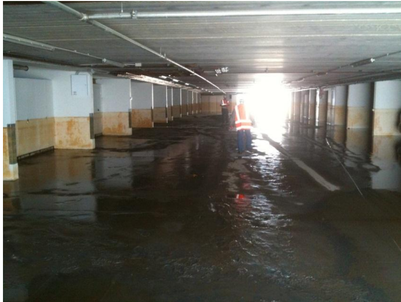
Figure 5-5. Photograph of the basement parking garage. Note the high water mark on the walls. (-43.5577°, 172.7066°)
