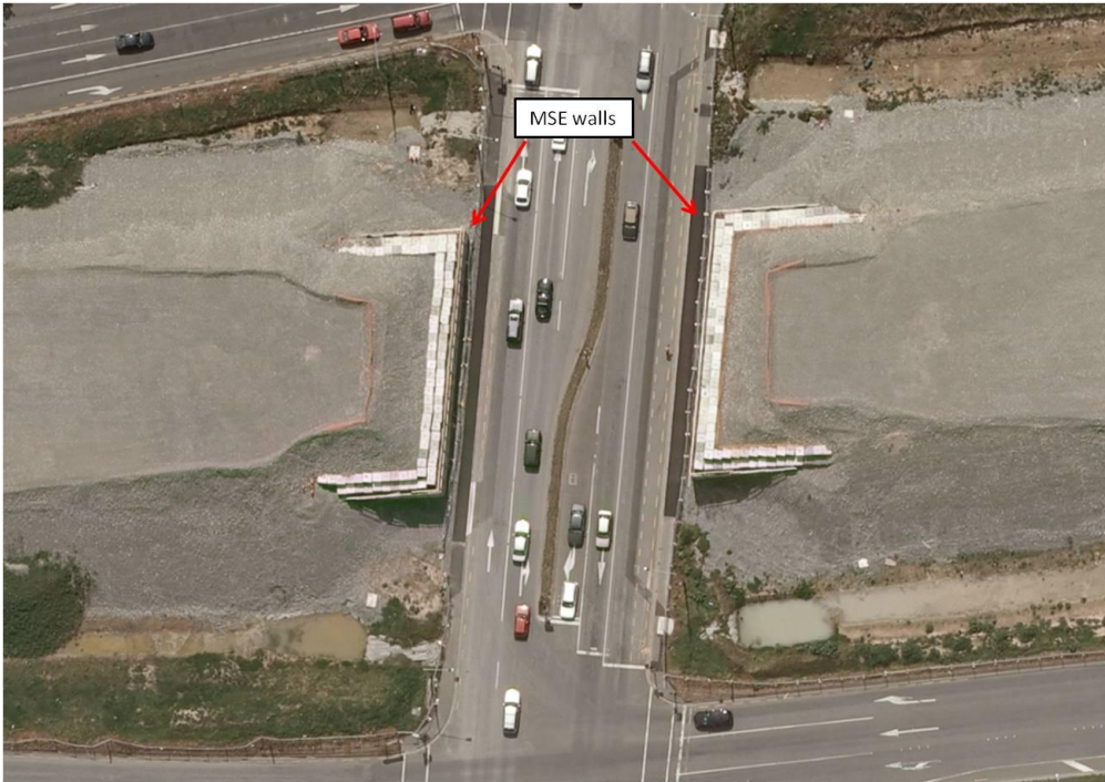
Figure 5-18. Aerial view of Barrington St interchange MSE walls in later stages of construction. (-43.5480°, 172.6101°)
