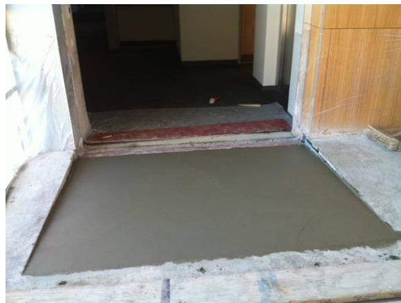
Figure 5-25. Ramp construction to mitigate differential movement between structures (position 2). (Position locations shown in Figure 5-23.)
