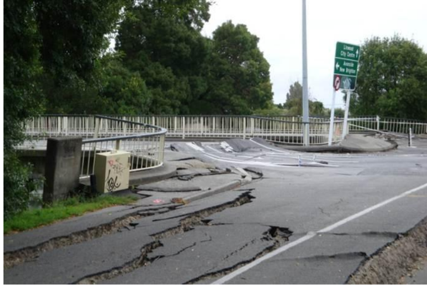
Figure 7-6. Photograph of the north approach of Fitzgerald Avenue Bridge looking toward the southwest. Note the lateral spreading cracks parallel to the river and the settlements at the abutments. (-43.5263°, 172.6506°)
