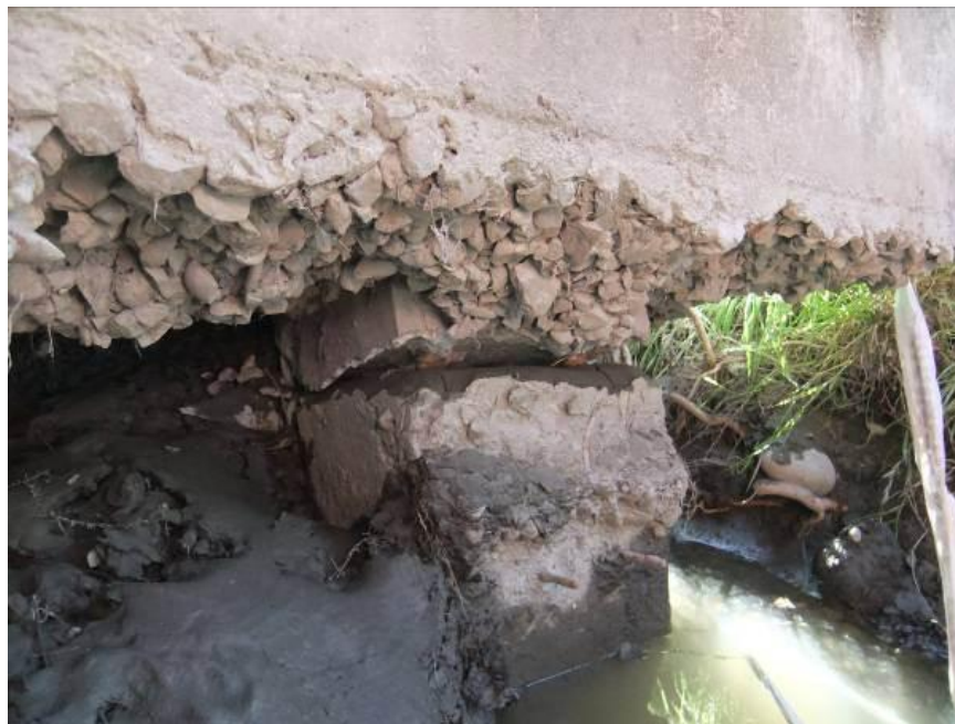
Figure 7-9. Photograph of tension failure and reinforcement elongation at north abutment of the eastern Fitzgerald Avenue Bridge. (-43.5263°, 172.6506°)
