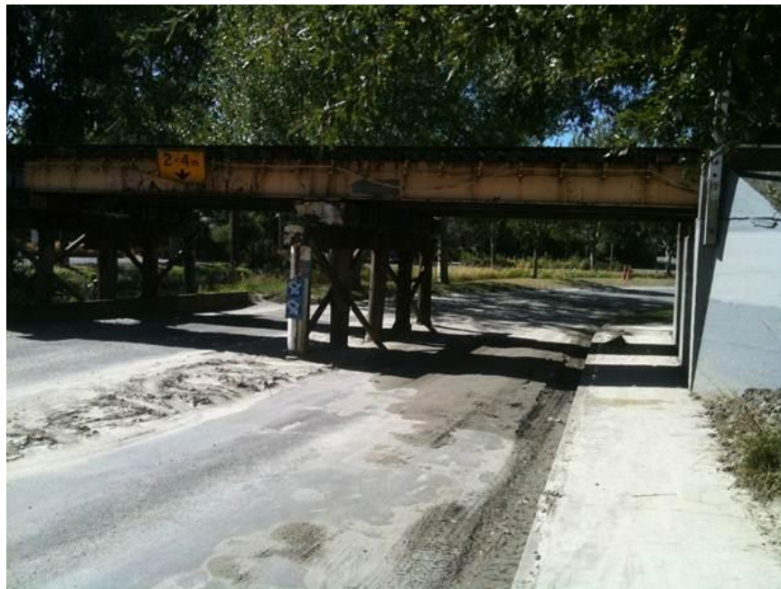
Figure 7-46. Photograph of the northeast abutment looking northwest. Note the sand deposits on the roadway and the horizontal crack at the top of the abutment. (-43.5529°, 172.6676°)
