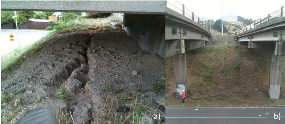
Figure 7-42. a) Transverse crack running along the crest of the slope near the southeast abutment; b) toe scarp running horizontally between the columns of the southeast abutment. (-43.5725°, 172.6947°)
