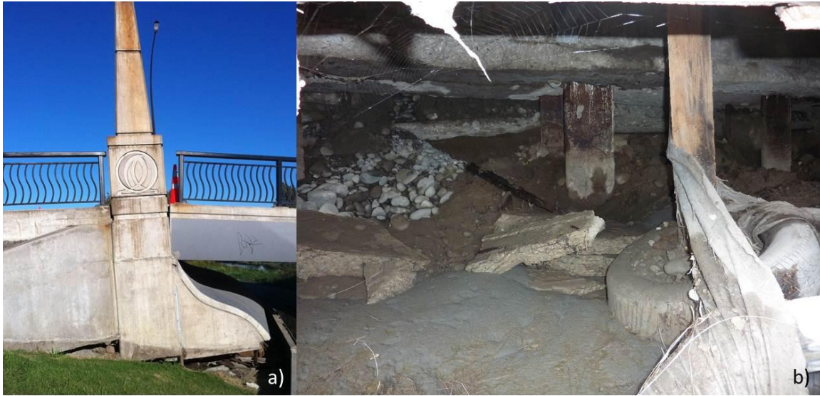
Figure 7-24. Photographs of a) the back rotation of the south abutment; b) view beneath the northern abutment of exposed piles. (-43.5009°, 172.7012°)
