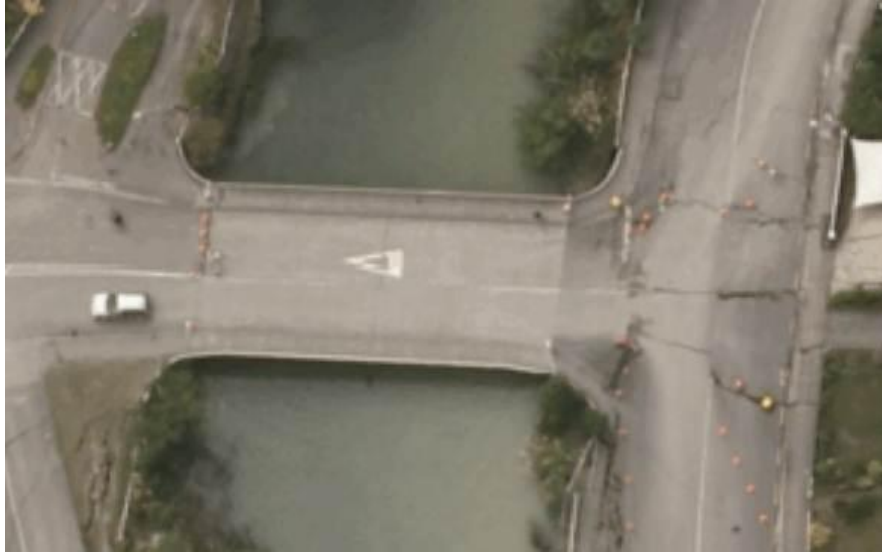
Figure 7-12. Satellite image of Swanns Road Bridge post-earthquake (LINZ 2011). (-43.5222°, 172.6601°)
