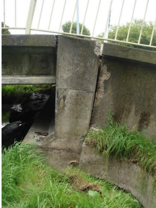
Figure 7-8. Photograph of back rotation of the north abutment of the eastern bridge on the eastern side. (-43.5263°, 172.6506°)
