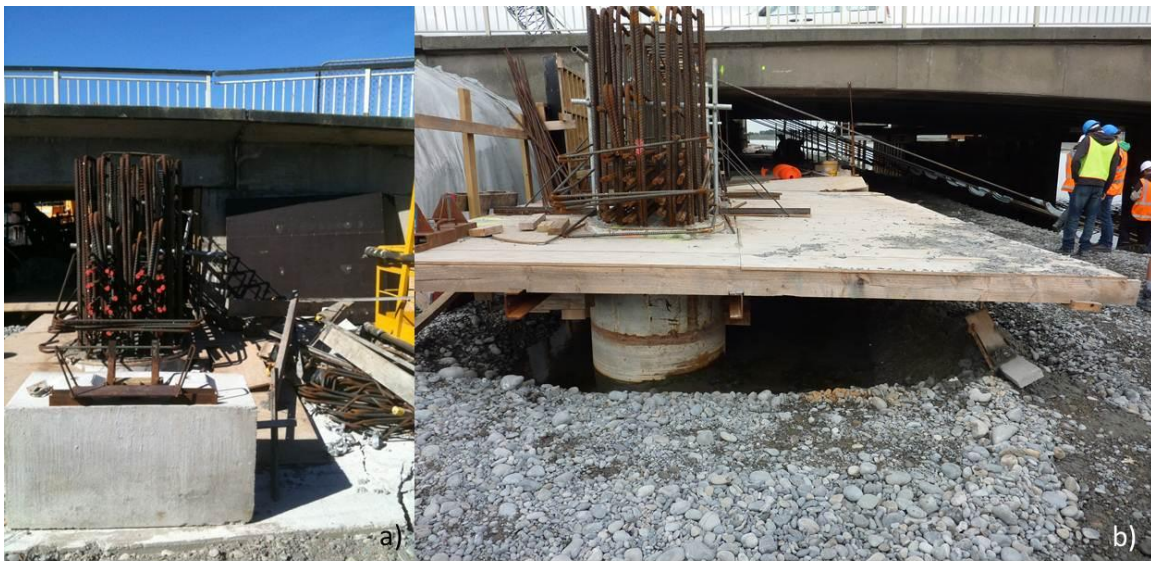
Figure 7-36. Photograph of the west abutment a) looking south showing no appreciable tilting; b) looking north with settlement of material in front of abutment indicated by the level of the wooden form work. (-43.5584°, 172.7088°)
