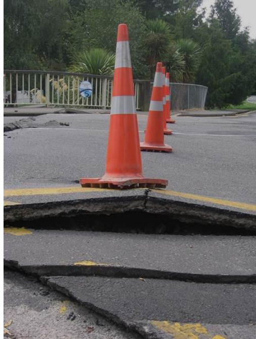
Figure 7-33. Approach damage at Malcolm Avenue Bridge (2) (Flickr 2011). (-43.565073 °, 172.639302°)
