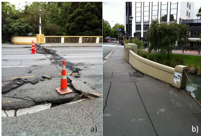
Figure 7-2. a) Damage to the western approach of Hereford Street Bridge (6) due to lateral spreading ( -43.532026^{\circ} 172.633390^{\circ} ); b) Outward rotation of wingwalls on western approach of Gloucester Street Bridge (8) due to lateral spreading ( -43.529887^{\circ} 172.633986^{\circ} ).
