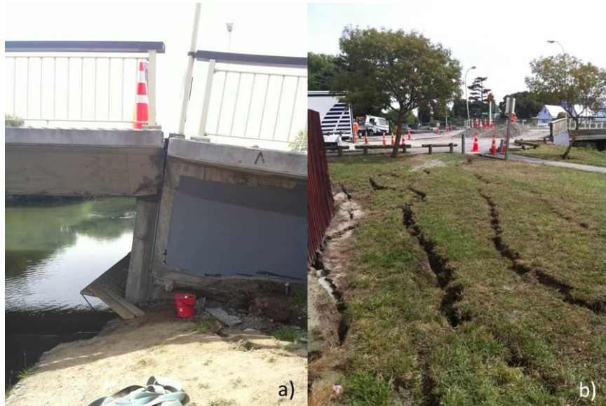
Figure 7-19. Photograph of the south abutment showing (a) back rotation of the abutment and (b) lateral spreading in the vicinity of the approach. (-43.5005°, 172.6878°)
