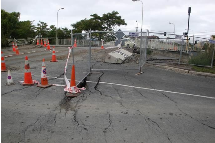
Figure 7-15. Photograph of the approach to the north abutment. Note the aggregate resurfacing and extensive pavement cracking. (-43.5216°, 172.6728°)
