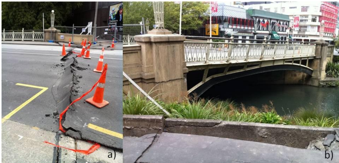
Figure 7-3. a) Moderate approach damage and settlement on northern approach of Colombo Street Bridge; b) Buckling of steel arch and handrail as a result of lateral spreading compressive forces on bridge structure. ( -43.5272^{\circ} 172.6366^{\circ} )
