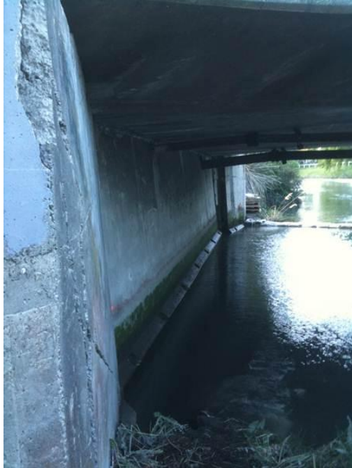
Figure 7-17. Photograph of the north abutment looking east. Note the displacement of the wingwalls on either side of the abutment. (-43.5216°, 172.6728°)
