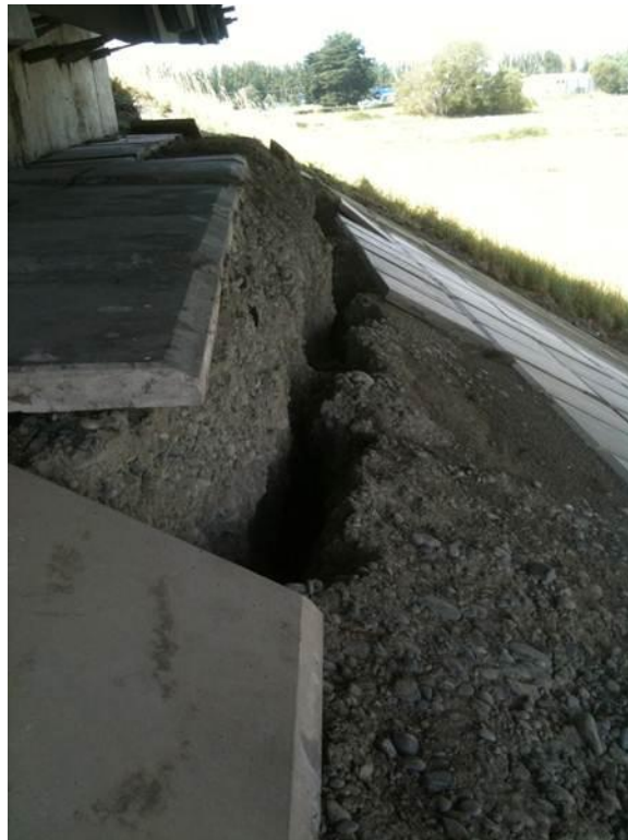
Figure 7-40. Photograph of the top of the slope at the northeast abutment looking southeast. Note the transverse crack. (-43.4298°, 172.6463°)
