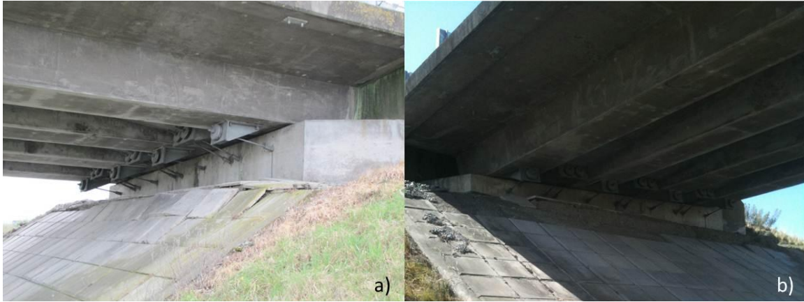
Figure 7-39. Photograph of the northeast abutment slope after the (a) Darfield event and (b) Christchurch event. (-43.4298°, 172.6463°)
