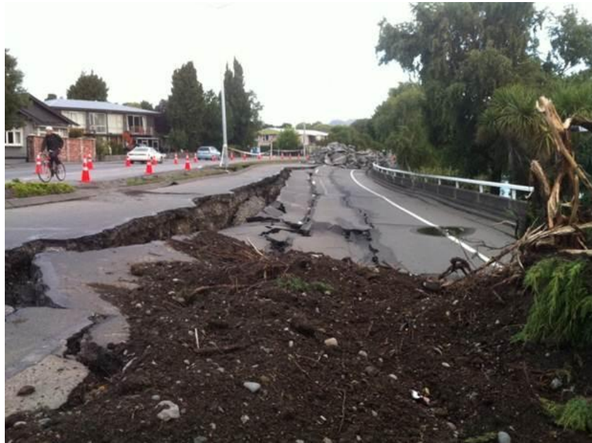
Figure 7-7. Photograph of lateral spreading damage of roadway north of Fitzgerald Avenue Bridge. (-43.524156°, 172.650891°)
