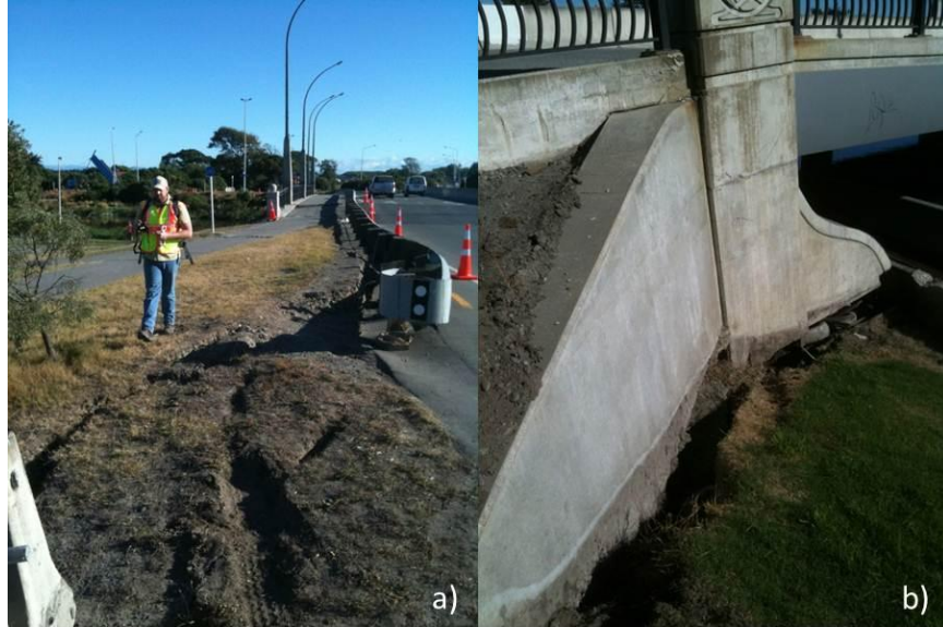
Figure 7-22. Photograph of the south approach and abutment. Note the (a) longitudinal cracks in the approach and (b) back rotation of the abutment and the gap between the soil and the abutment. (-43.5009°, 172.7012°)
