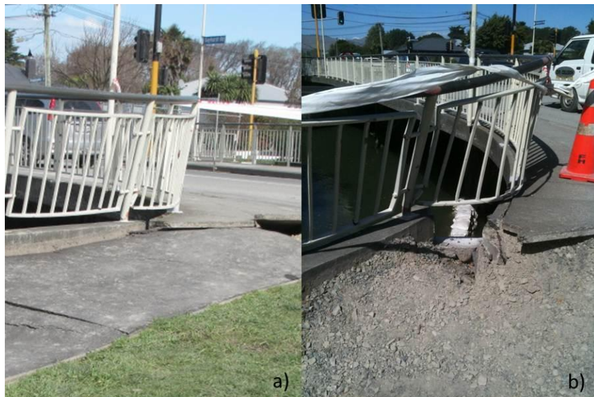
Figure 7-16. Photograph of the north approach of Gayhurst Road Bridge looking southwest. Note the displacement of the wingwall in the (a) Darfield event (GEER 2010) and (b) Christchurch event. (-43.5216°, 172.6728°)
