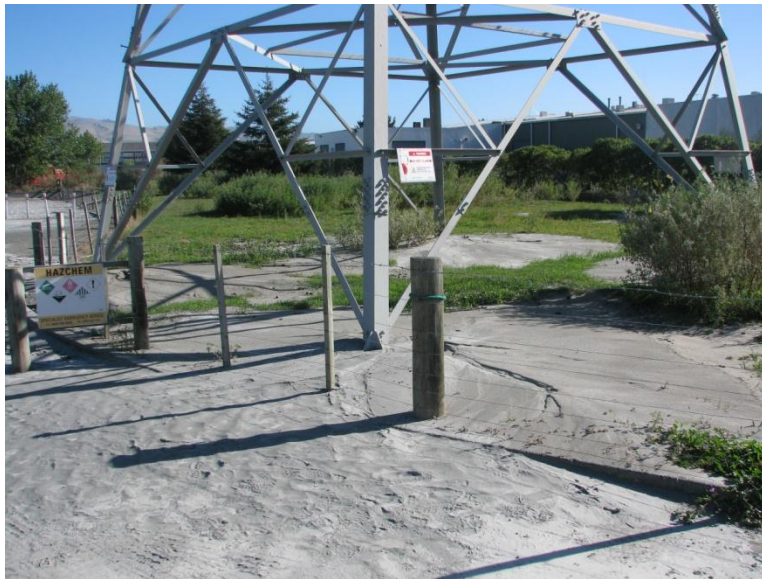
Figure 8-11. Liquefaction ejecta at the base of an electrical tower (-43.531764°, 172.697467°)
