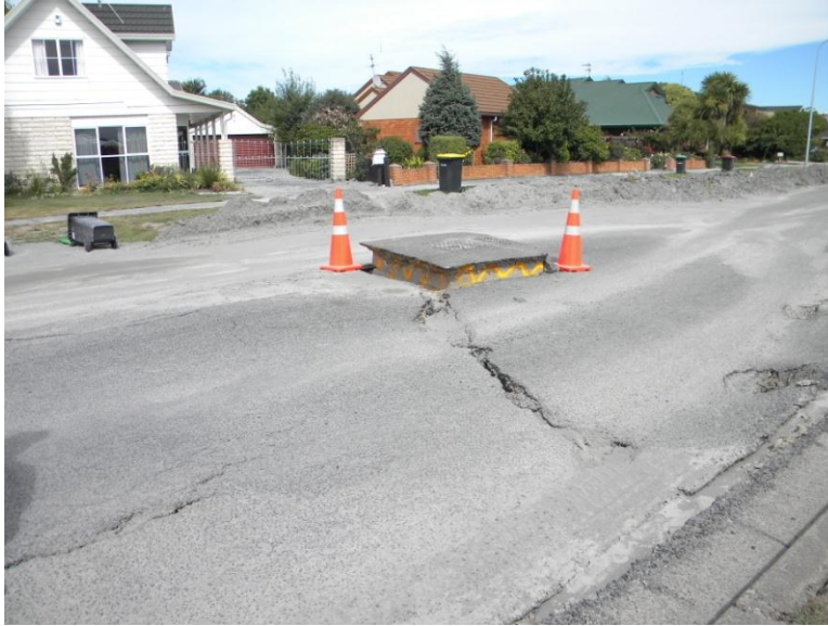
Figure 8-1. Floated manhole on Orrick Crescent (-43.50174°, 172.696487°).
