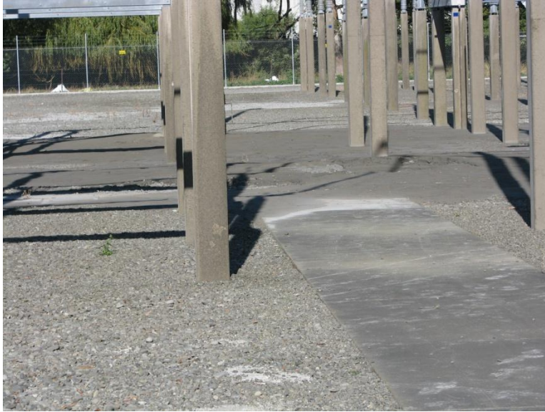
Figure 8-12. Liquefaction ejecta around concrete (-43.532629°, 172.698029°)
