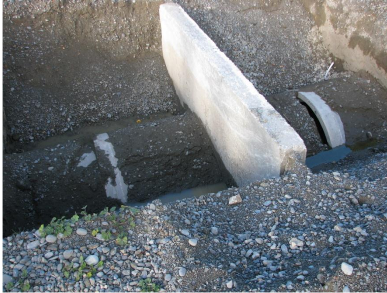
Figure 8-9. Pipe damage at the oxidation ponds (-43.3145211°, 172.430083°)
