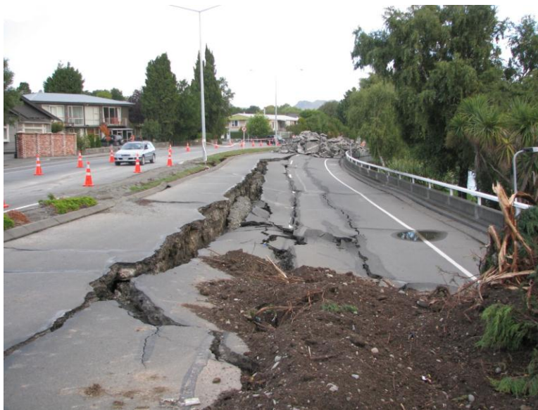
Figure 8-2. Lateral spreading at Fitzgerald Avenue along the Avon River (-43.524048°, 172.650851°).
