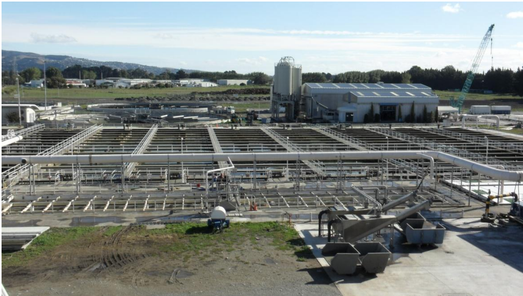
Figure 8-7. Waste Water Treatment Plant Settling Basins (-43.526016°, 172.700922°)
