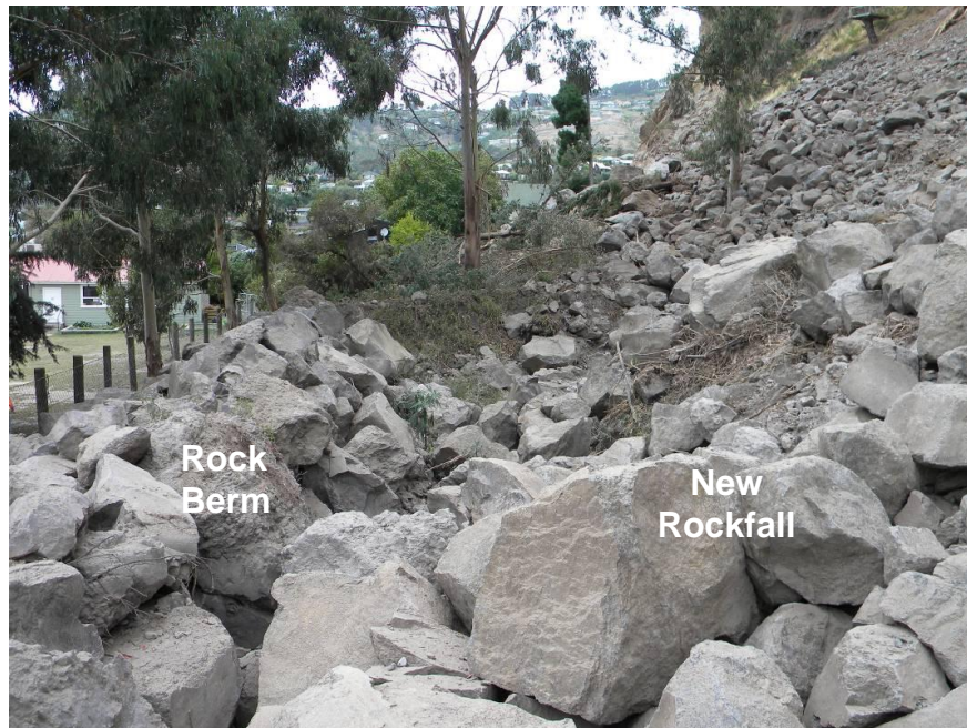
Figure 9-11. Photo showing rock berm constructed to protect schoolyard at base of cliff in Redcliffs. The berm apparently performed well in stopping rockfall and talus as the fence bounding the school field (note wood posts at center left) was not significantly damaged and no rocks were observed on the field (-43.55972°, 172.73298°).
