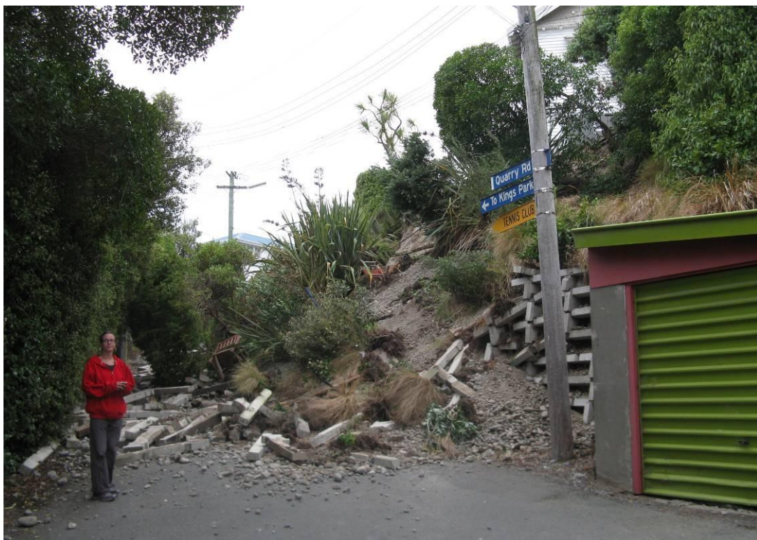
Figure 9-3. Failed retaining wall and slumping in loess, blocking a road on lower Mt Pleasant (-43.55617°, 172.7156°).
