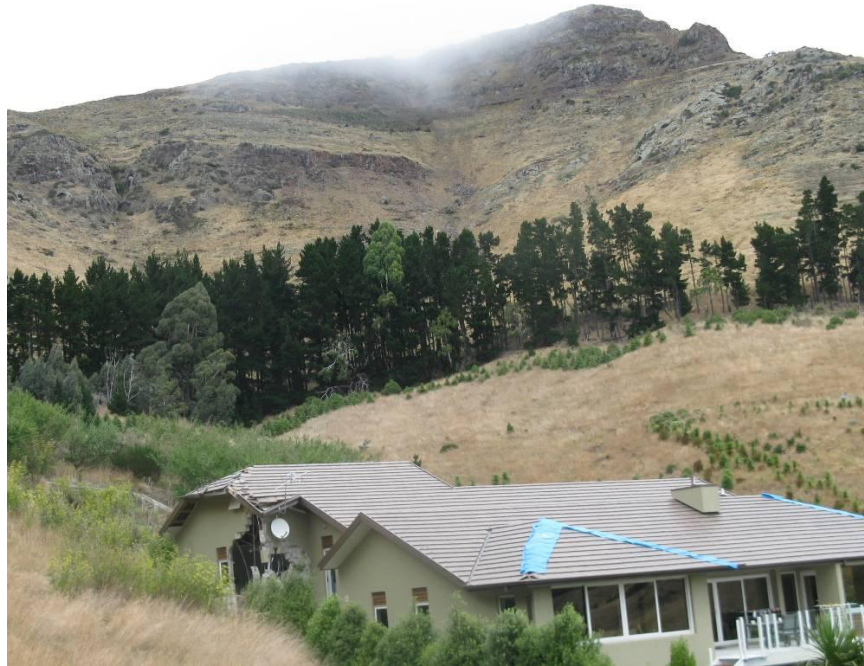
Figure 9-16. House with hole on left side from rockfall, note cliff source areas above with fresh talus. ( -43.58126^{\circ} , 172.71672^{\circ} ).
