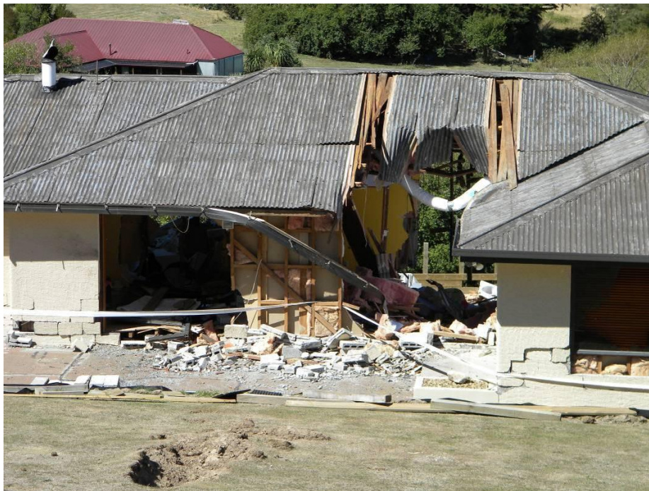
Figure 9-20. House in Rapaki damaged by rockfall. Note impact mark on lawn at bottom of photograph. Boulder may have fractured into two or more blocks as there appear to be two impact areas on the up-slope facing wall of the house ( -43.6044^{\circ} , 172.6780^{\circ} ).
