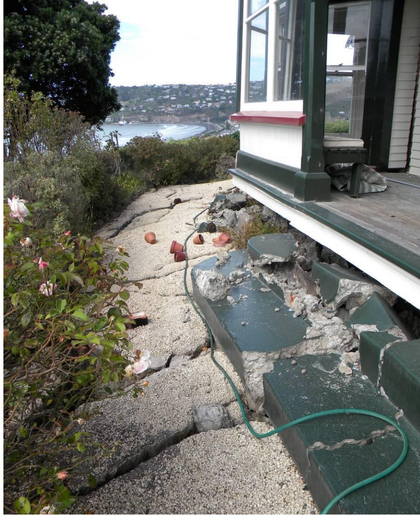
Figure 9-24. Landslide headscarp extending beneath house on Clifton Terrace. House was thrown off foundation, and foundation was cracked in several places along headscarp (-43.56586°, 172.75256°).
