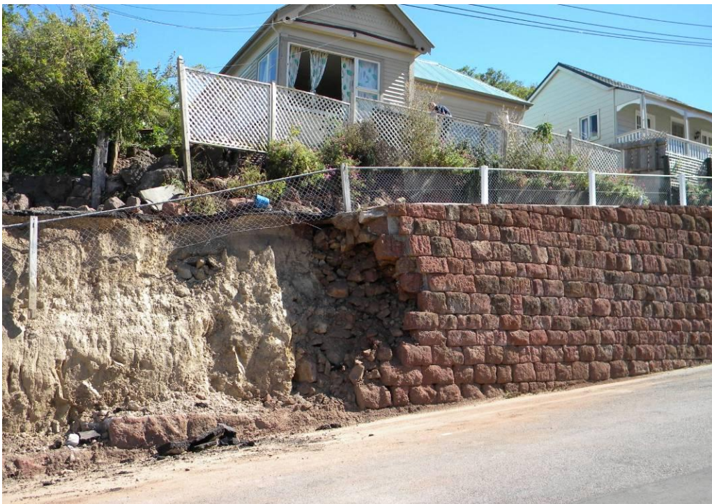
Figure 9-22. Rockwall collapse in Lyttelton. Top: Angular random size block wall ( -43.59949^{\circ} , 172.71717^{\circ} ). Bottom: Rectangular block wall ( -43.60069^{\circ} , 172.71903^{\circ} ).
