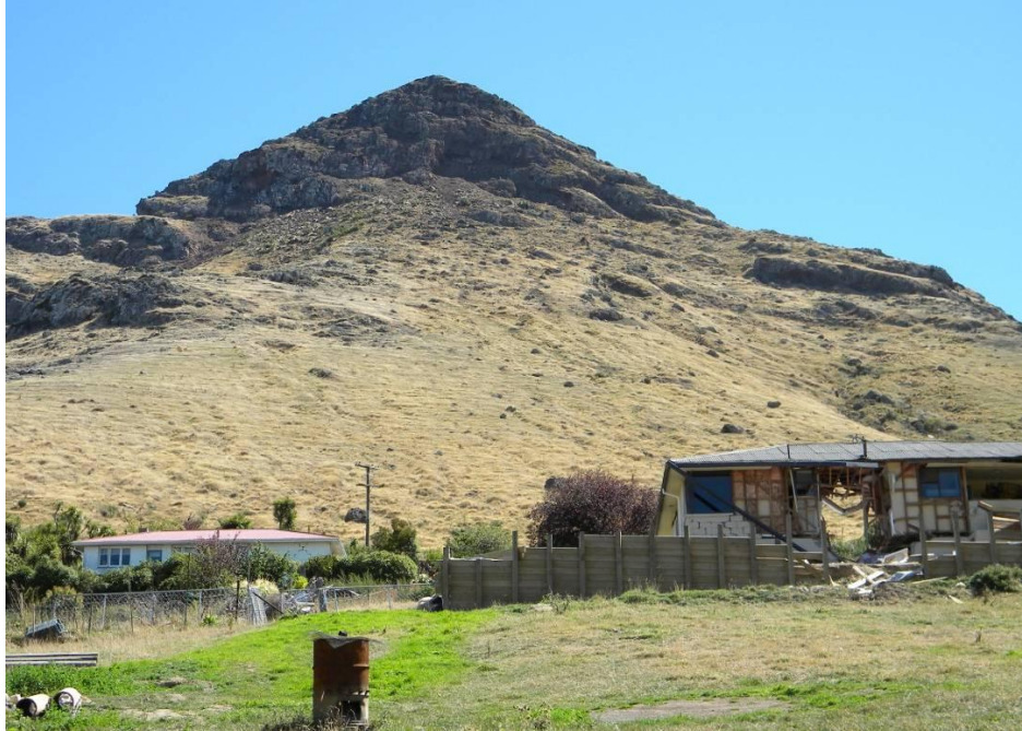
Figure 9-19. House in Rapaki damaged by rockfall. Rockfall originated from cliffs at an elevation approximately 250 to 300 m above house ( -43.60475^{\circ} , 172.67920^{\circ} ).
