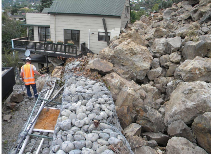
Figure 9-10. Photo showing slight movement of upper part of gabion behind house at base of cliff in the suburb of Redcliffs. Gabion performed well in stopping rockfall and talus from impacting house (-43.56067°, 172.73367°).
