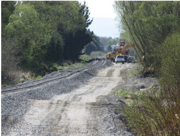
Figure 4.33 Damage to train tracks due to ground movement. (Position 3; -43.4068°, 172.6489°)
