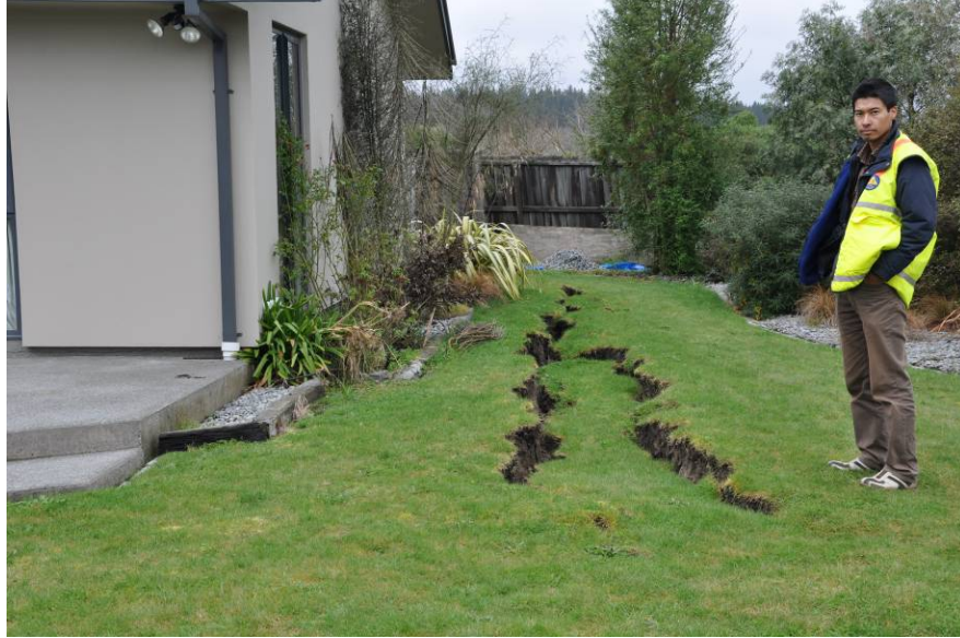
Figure 5.46. Lateral spread adjacent to residence at Riverside Ln. The location of this fissure is ~26 m from the nearby Styx River. (-43.4308°, 172.6930°; 1230 hrs on 13 September 2010)
