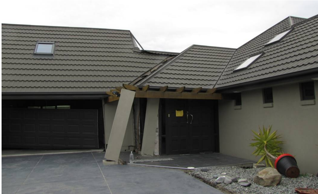
Figure 5.47. House with fissured floor slab with damage carried through to the roof line, which is no longer weather proof. (Riverside Ln, Spencerville). (-43.4311°, 172.6935°; 1600hrs on 28 September 2010)
