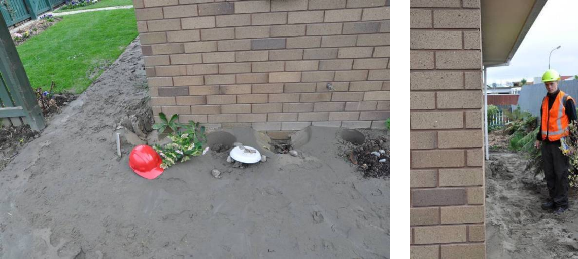
Figure 5.18 Red tagged residence on Charles St. Extensive surrounding ejecta at perimeter of house (43.3838°S, 172.6607°E; 1130 hrs on 11 September 2010)
