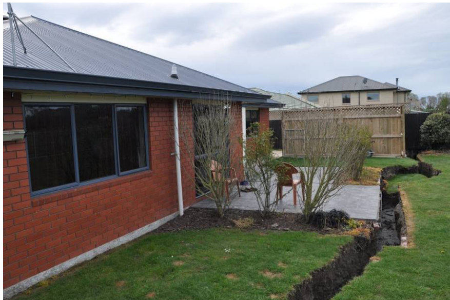
Figure 5.20 Ground failure feature extending through the backyard of a house on the south side of Courtenay Dr in the South Kaiapoi residential community. (-43.3894°, 172.6633°; 1500 hrs on 11 September 2010)
