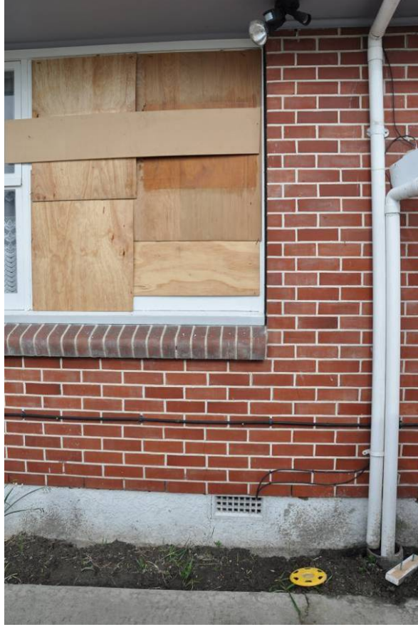
Figure 5.16 Residence along Charles St (same structure as Figure 5.16). Damage to glass windows and between window and wall. (-43.3836°, 172.6604°; 1115 hrs on 11 September 2010)
