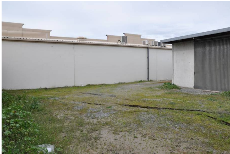
Figure 5.9 Surrounding ground failure patterns directly adjacent to the Property and Family Law Offices in Kaiapoi business district. View looking southeast (43.3819°S, 172.6593°E; 1100 hrs on 11 September 2010)
