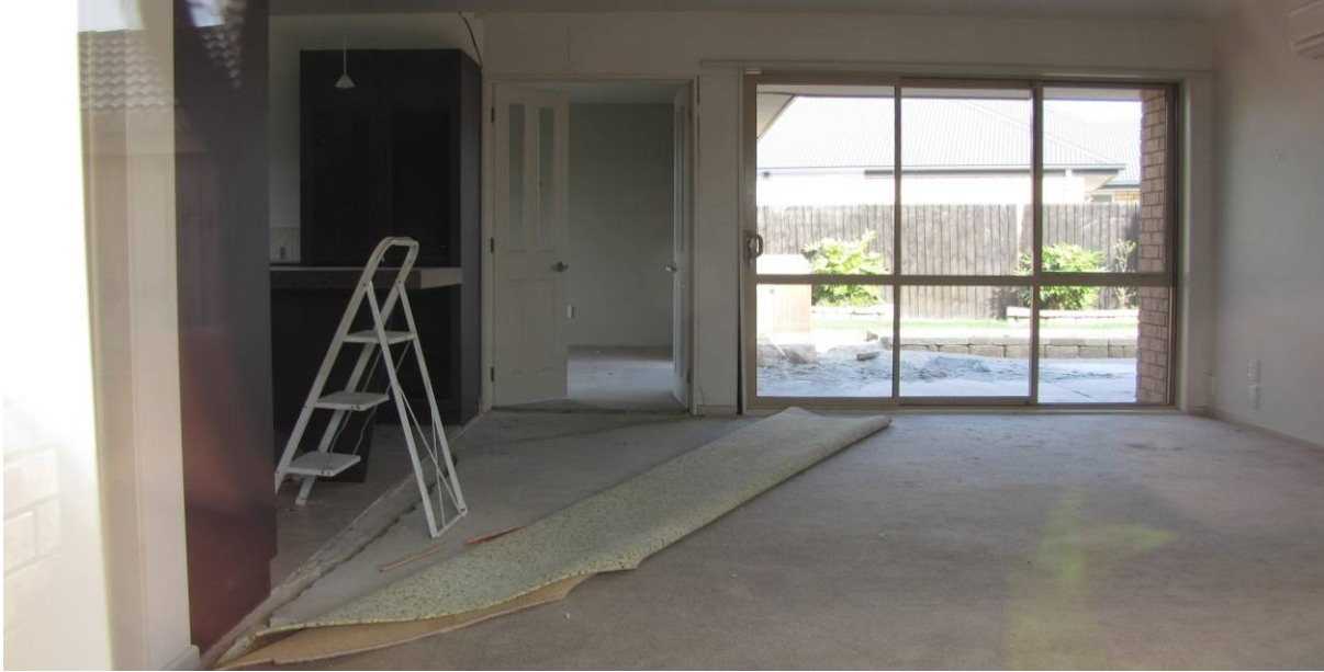
Figure 5.39. Fissure in concrete floor slab (to the left hand side passing beneath the ladder). (Same house as in Figure 5.38.) (Kokopu St; -43.5183°, 172.7220°; 1030hrs on 12 September 2010)
