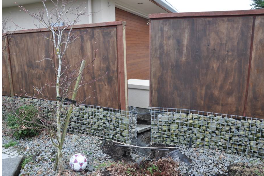
Figure 5.48 Separated fence line due to propagating ground fissure meandering between houses along Riverside Ln. (-43.43096°, 172.6931°; 1230hrs on 13 September 2010)
