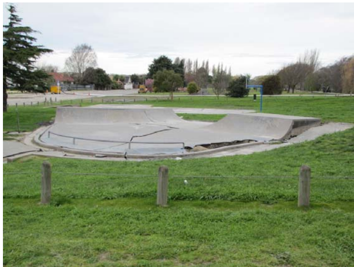
Figure 6.22 Photo 21: Skate park on the levee on the north side of the Kaiapoi River. The location of this photograph is denoted in Figure 6.4. ( -43.384094^{\circ} , 172.660370^{\circ} )
