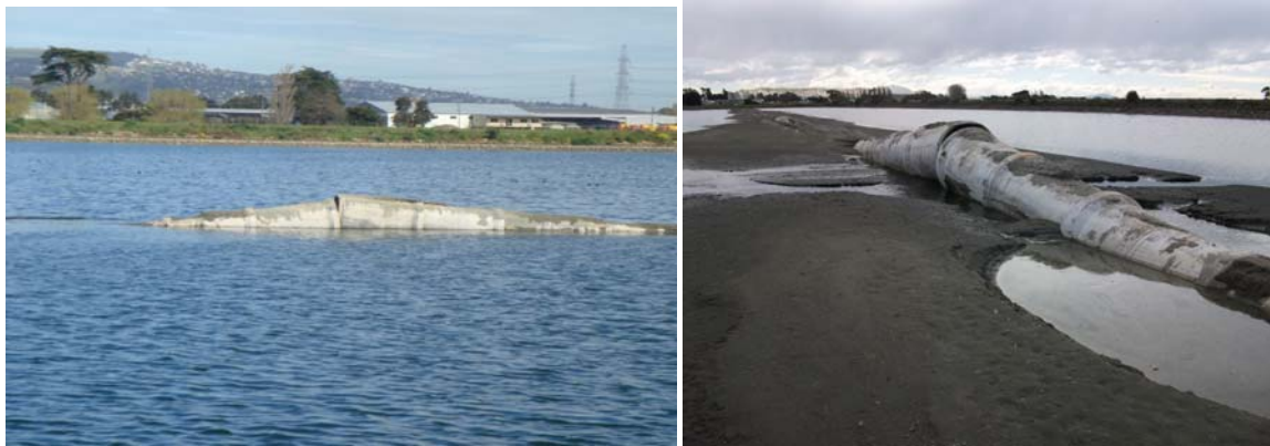
Figure 6.34 Buckled pipe protruding from Pond 1 during pond dewatering, and after pond level was lowered. Pipeline crown was at the pond invert prior to the earthquake. (-43.530867°, 172.705190°)
