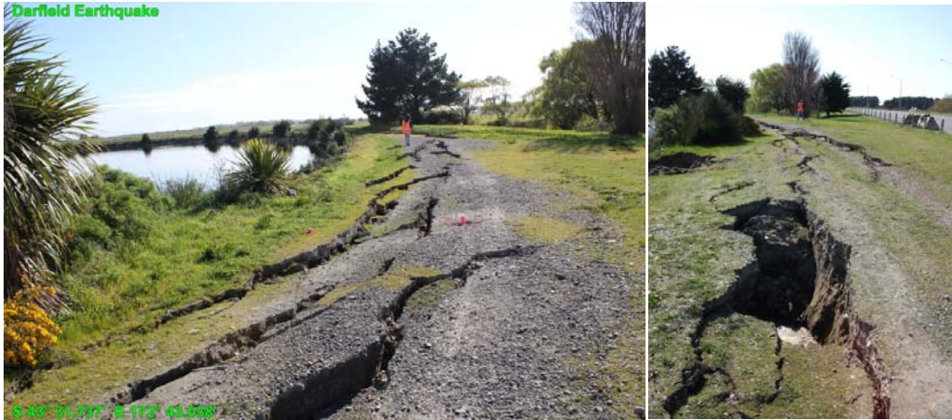
Figure 6.35 Lateral spread cracks at the eastern end of Pond 2B. The sinkhole in the foreground of the photo on the right formed over the top of two outlet pipelines. (-43.52895°, 172.717300°)
