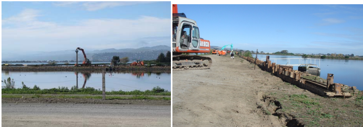
Figure 6.36 Sheet piles being driven to stabilize the pond embankment to arrest further movement. (-43.530563°, 172.718349°)
