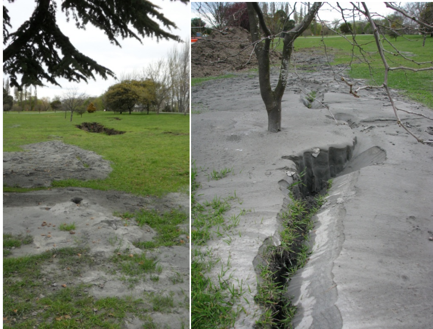
Figure 6.21 Photo 19 and 20: Lateral spread cracks along landside of the levee on the north side of the Kaiapoi River. The locations of these photographs are denoted in Figure 6.4. ( -43.384633^{\circ} , 172.661231^{\circ} )
