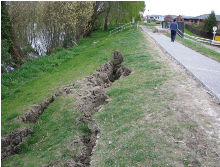
Figure 6.25 Photo 25: Lateral spread cracks along riverside levee on the south side of the Kaiapoi River. The location of this photograph is denoted in Figure 6.4. (-43.385254°, 172.660131°)
