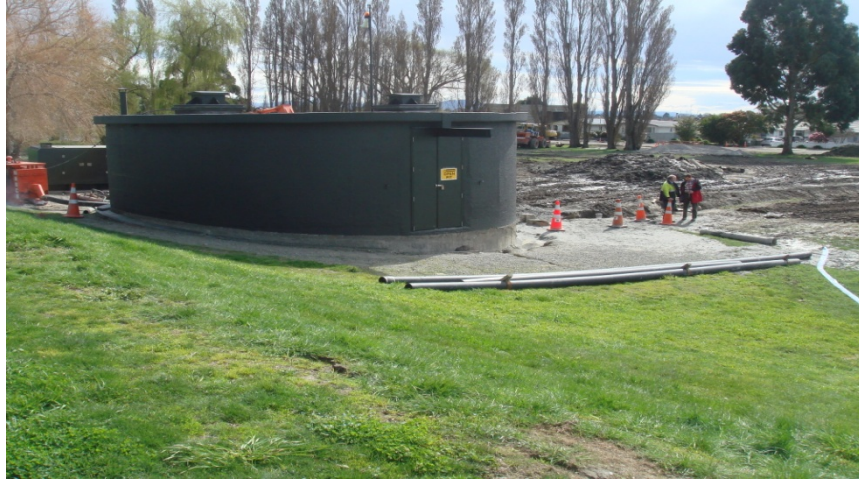
Figure 6.23 Photo 22: Tank that settled ~30 cm resulting in damage to attached pipes. The photograph numbers correspond to the locations denoted in Figure 6.4. (-43.386918°, 172.664412°)
