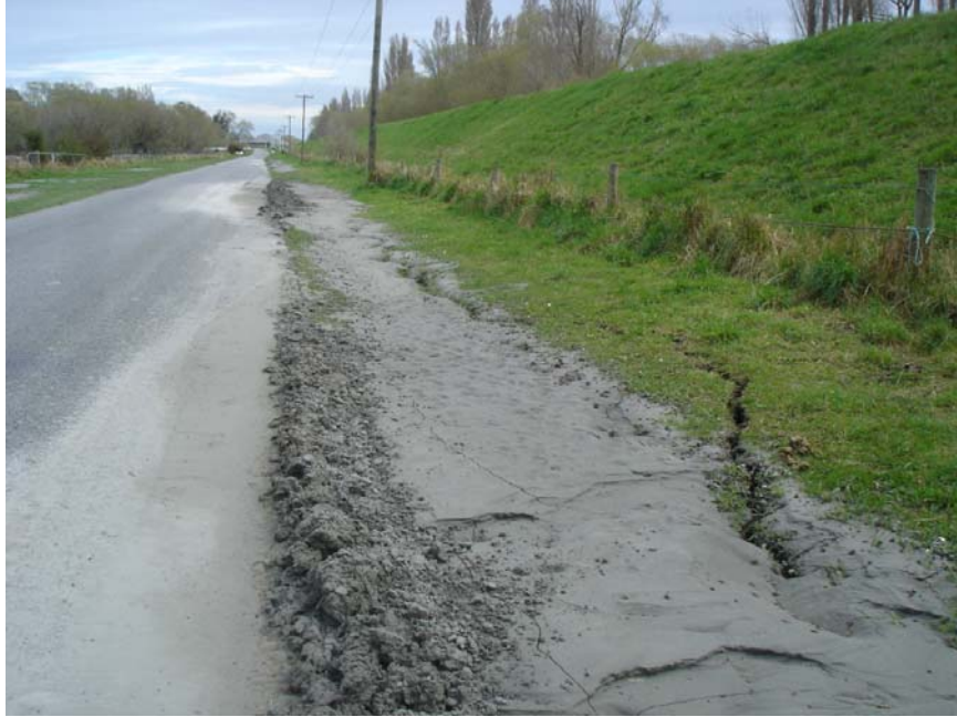
Figure 6.7 Photo 2: Crack running along base of levee on Coutts Island Rd (landside) and liquefaction ejecta. The location of this photograph is denoted in Figure 6.4. (-43.424466°, 172.629907°)
