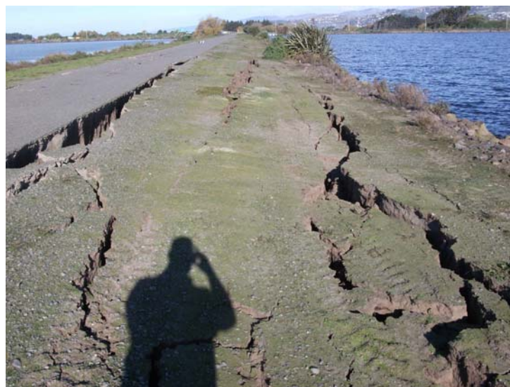
Figure 6.33 Lateral spread cracks running parallel to Dyers Road adjacent to Pond 2A. (-43.531393°, 172.712473°)
