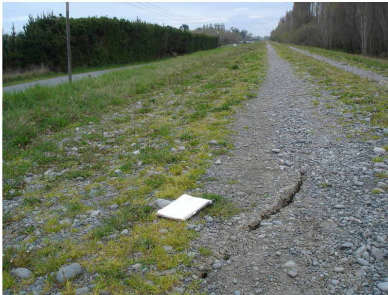
Figure 6.10 Photo 5: ~2-cm wide crack running lengthwise along the top of the levee on Coutts Island Rd. This crack was at the edge of the ~0.5 km stretch of the levee where significant liquefaction was observed. Photo taken looking southwest. The location of this photograph is denoted in Figure 6.4. (-43.423440°, 172.632349°)
