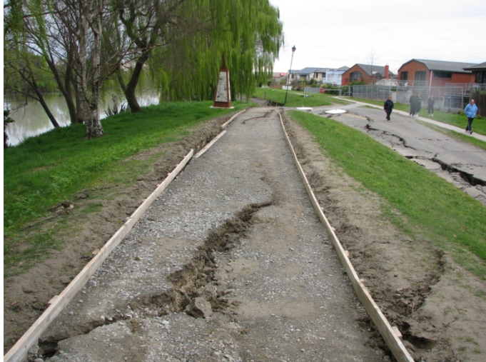
Figure 6.27 Photo 27: Lateral spread cracks along the top of the levee on the south side of the Kaiapoi River. The location of this photograph is denoted in Figure 6.4. (-43.385693°, 172.660688°)
