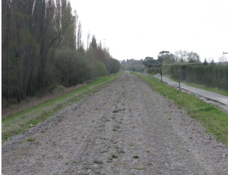
Figure 6.9 Photo 4: Road on top of levee that had recently been reggraded, presumably after the earthquake to fill in longitudinal cracks formed during the earthquake. Liquefaction was observed along the base of both sides of the levee along this stretch. The location of this photograph is denoted in Figure 6.4. (-43.423943°, 172.631045°)
