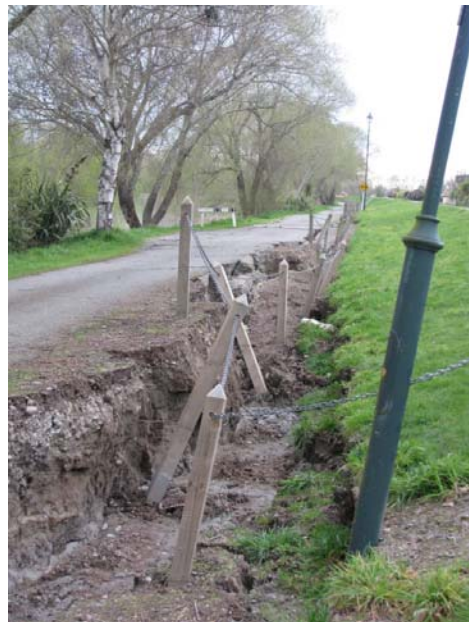
Figure 6.26 Photo 26: Lateral spread cracks along riverside levee on the south side of the Kaiapoi River. The location of this photograph is denoted in Figure 6.4. (-43.385839°, 172.660941°)
