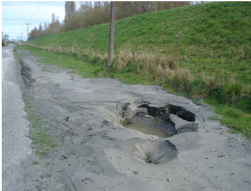
Figure 6.6 Photo 1: Large sand boil at the base of the landside of the levee on Coutts Island Rd. The location of this photograph is denoted in Figure 6.4. (-43.425018°, 172.628442°)
