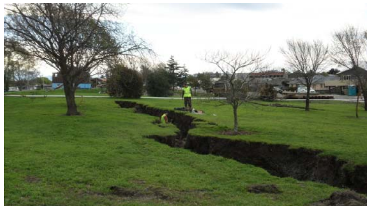
Figure 6.20 Photos 16-18: Lateral spread cracks along landside of the levee on the north side of the Kaiapoi River. The locations of these photographs are denoted in Figure 6.4. (-43.384484°, 172.660653°)
