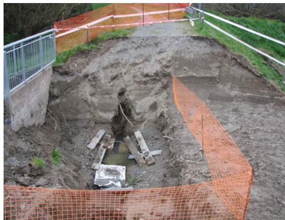
Figure 6.28 Photo 28: Failed drainage conduits running underneath the levee on the southside of the Kaiapoi River. The location of this photograph is denoted in Figure 6.4. (-43.388679°, 172.666203°)
