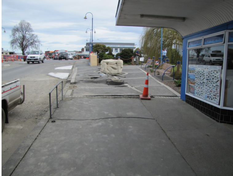
Figure 7.17 Cracking of east approach roadway, Williams Road Bridge. (-43.3825°, 172.6575°)
