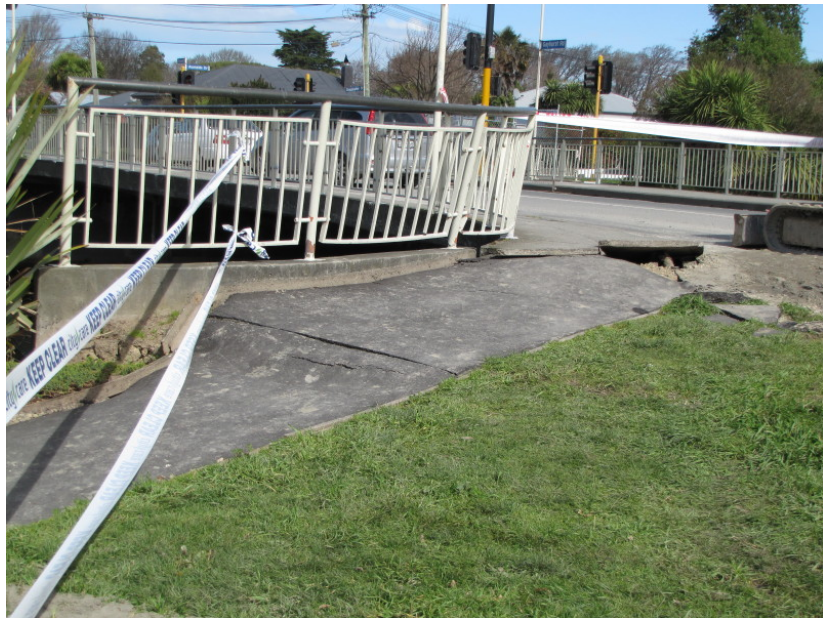
Figure 7.12 Incipient lateral spreading at west abutment, Swanns Road Bridge. (-43.5222°, 172.6600°)
