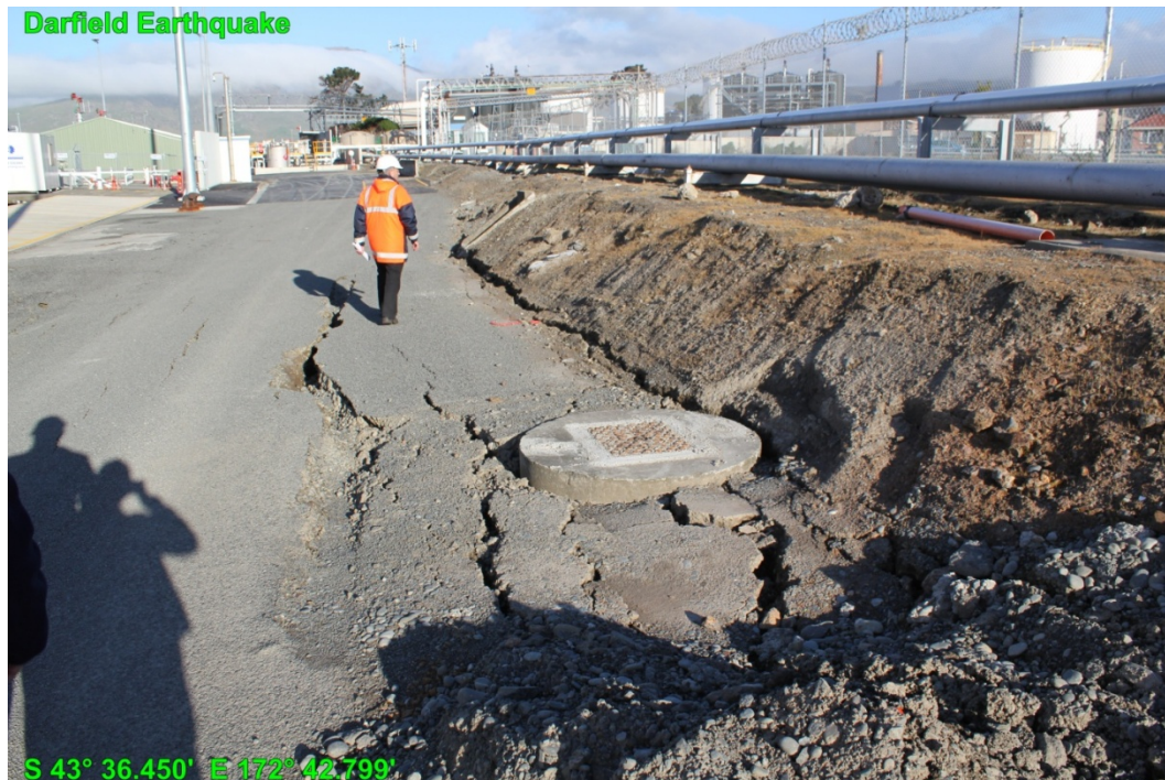
Figure 7.37 Settlement and lateral deformation at fuel transfer facility (-43.60750°, 172.71332°).
