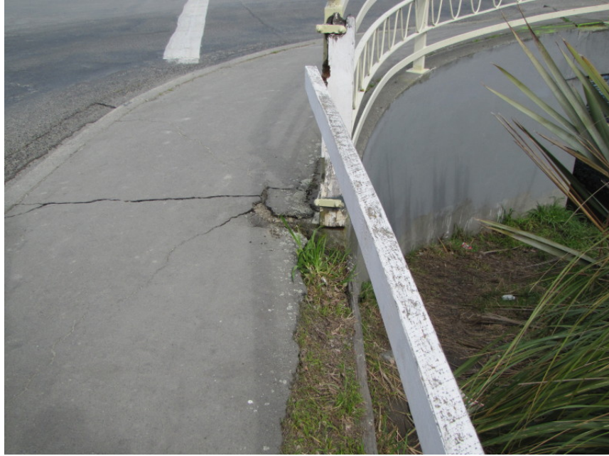
Figure 7.13 Incipient lateral spreading at north abutment, Gayhurst Road Bridge. (-43.52172°, 172.6728°)
