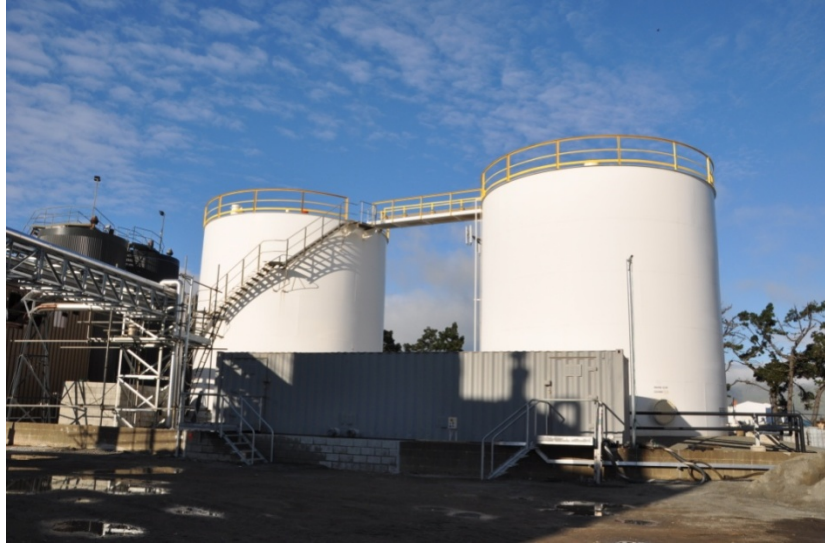
Figure 7.42 Tank 2 (right most large white tank) with Tanks 3 and 4 shown to the left (smaller grey tanks) at the Fulton Hogan Bitumen Plant (-43.6088°, 172.7147°).
