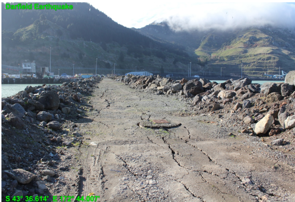
Figure 7.39 Cracking along jetty at eastern end of port (-43.61023°, 172.73345°).
