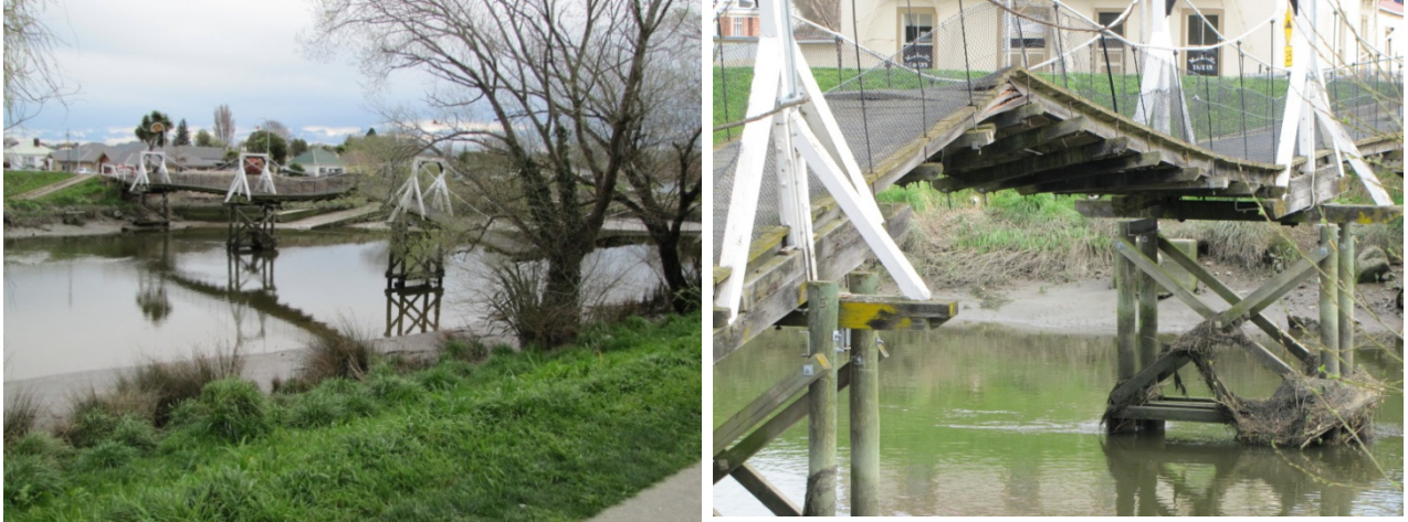
Figure 7.19 Buckling of footbridge near Trousselot Park. (-43.3811°, 172.6558°)
