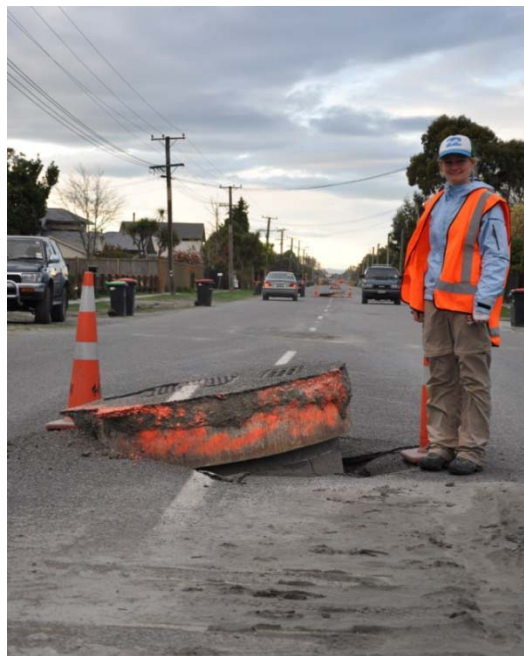
Figure 7.47 Uplifted manholes along Lower Styx Road, note the uplifted manholes in the background too. ( -43.4113^{\circ} , 172.6930^{\circ} ).
