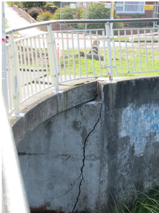
Figure 7.14 Cracking of north abutment, Swanns Road Bridge. (-43.5222°, 172.6600°)
