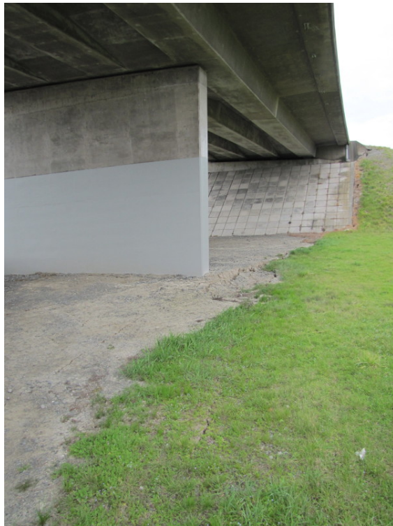
Figure 7.24 Evidence of liquefaction beneath Chaney's Overpass. (-43.4300°, 172.6464°)
