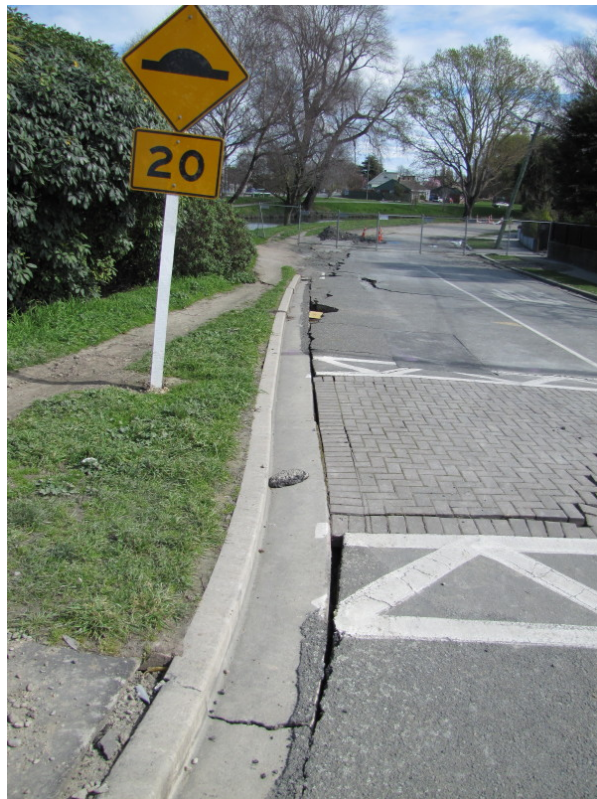
Figure 7.10 Cracking of roadway on west approach fill, Swanns Road Bridge. (-43.5222°, 172.6600°)
