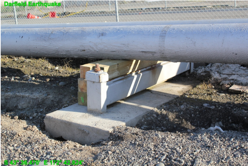
Figure 7.38 Temporary wooden support to accommodate settlement under fuel line (-43.60783°, 172.71373°)
