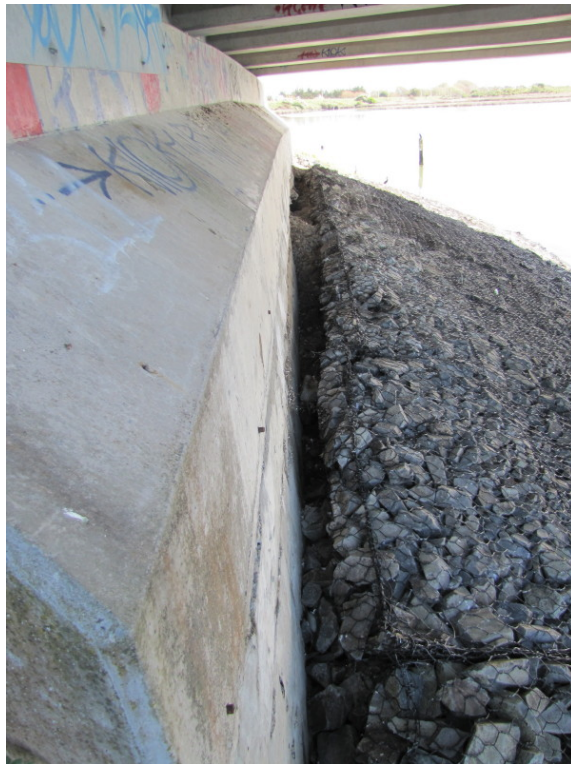
Figure 7.8 Gap between west abutment backwall and end embankment, Bridge Street Bridge. (-43.5253°, 172.7242°)
