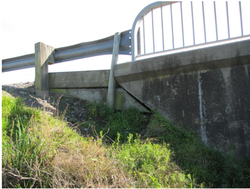
Figure 7.9 Back rotation of west abutment, Bridge Street Bridge. (-43.5253°, 172.7242°)
