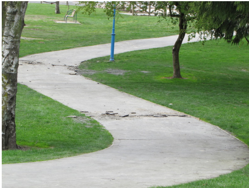
Figure 7.20 Cracking of sidewalk and evidence of liquefaction in Trousselot Park. (-43.3811°, 172.6558°)
