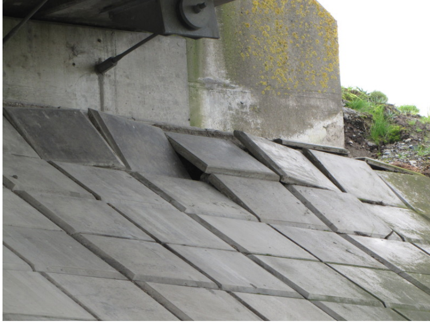
Figure 7.23 Displaced concrete tiles on end embankment for north abutment, Chaney's Overpass. (-43.4300°, 172.6464°)
