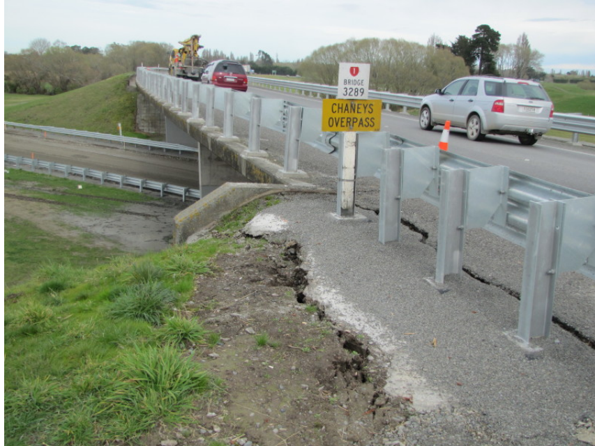
Figure 7.21 Incipient lateral spreading at Chaney's Overpass north abutment. (-43.4300°, 172.6464°)
