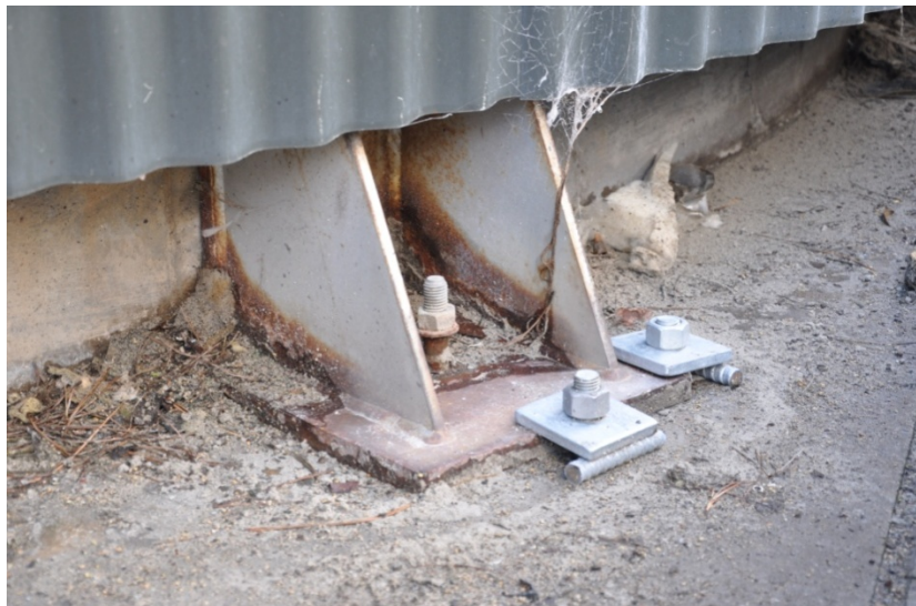
Figure 7.43 Typical repair to Tank 3 and 4 (addition of clamp plates). Note the pullout of the original anchorage. Fulton Hogan Bitumen Plant. (-43.6085°, 172.7149°).
