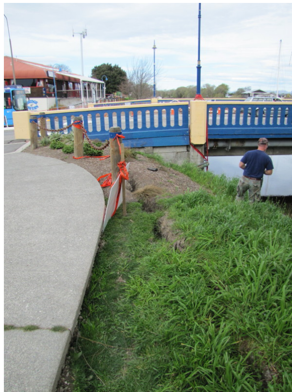
Figure 7.18 Incipient lateral spreading of east abutment, Williams Road Bridge. (-43.3825°, 172.6575°)
