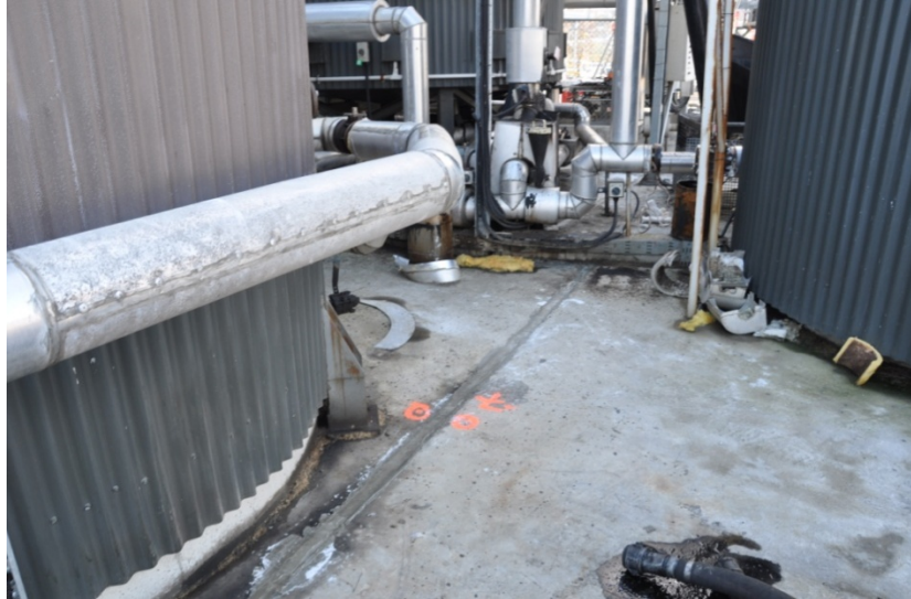
Figure 7.44 Repair of lateral spread cracks within the Fulton Hogan Bitumen Plant, nearby Tank 3. (-43.6085°, 172.7150°)
