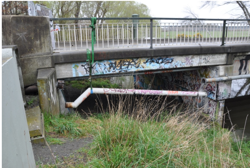
Figure 7.31 Damage to sewage pipe at the Kainga Road Bridge (-43.3997°, 172.6916°)
