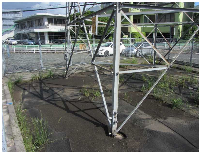
Figure 7-9. Transmission tower in a heavily liquefied zone with no observed tilting or foundation settlement. (32.768987, 130.691186).
