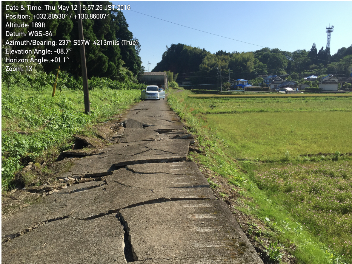
Figure 4-14. Roughly 1.8 m of right-lateral offset along the Futagawa Fault through a concrete road and fields.
