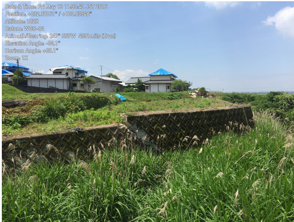
Figure 4-10. Southern strand of Futagawa Fault through fields and unreinforced masonry retaining wall.
