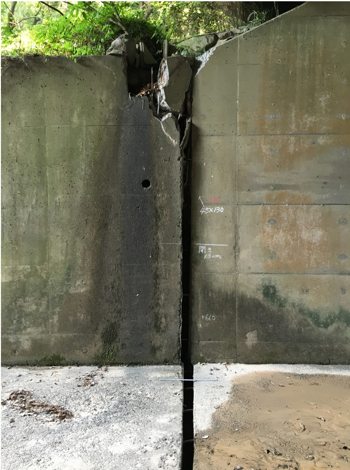
Figure 9-14. Another offset at a joint in the spillway outlet channel due to the movement and rotation of the spillway.
