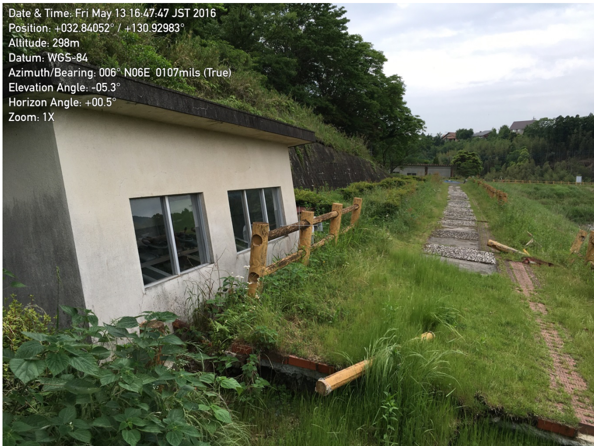
Figure 9-5. Significant back tilting of the gatehouse and forward tilting of the reservoir bench in front of the gatehouse.
