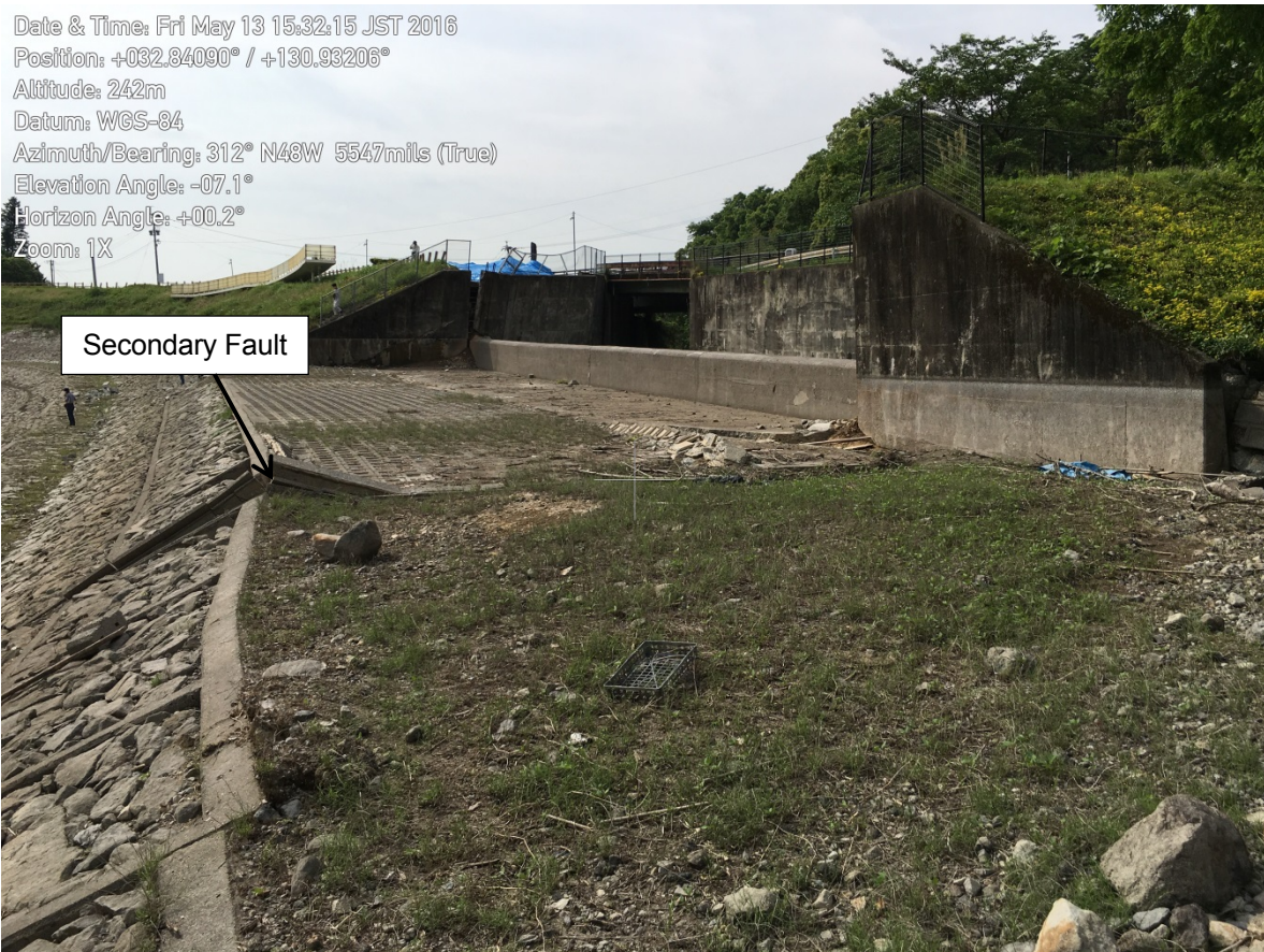
Figure 9-18. Side view of the spillway, with an apparent secondary rupture in the foreground running through the right side of the spillway.
