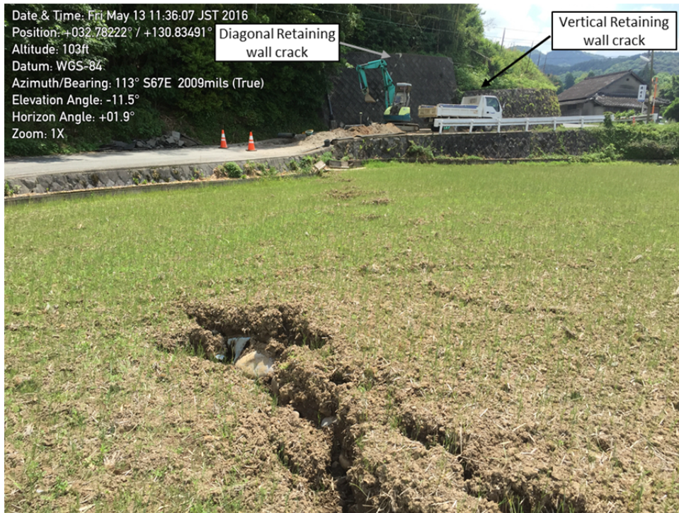
Figure 4-8. Northern strand of the Futagawa surface rupture through a field, road, sewer main, and retaining wall.
