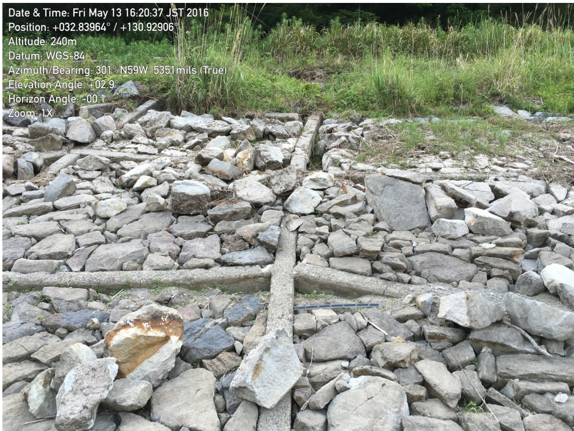
Figure 9-8. Deformation caused largely by the fault at the location of the fault entrance into the reservoir, as seen by the riprap dilation and bending of the concrete gridwork.
