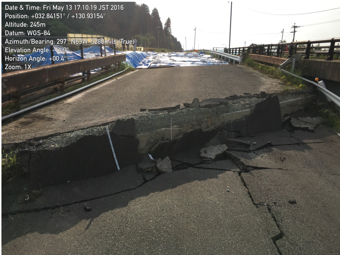
Figure 9-22. Differential settlement at one of the bridges crossing the spillway outlet channel, possibly caused by movement of the spillway walls in response to fault displacement.
