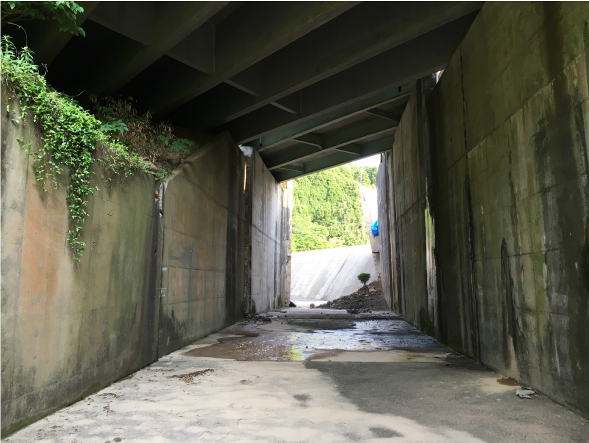
Figure 9-15. Overview of the offsets and rotations in the spillway outlet channel joints, facing back towards the spillway.
