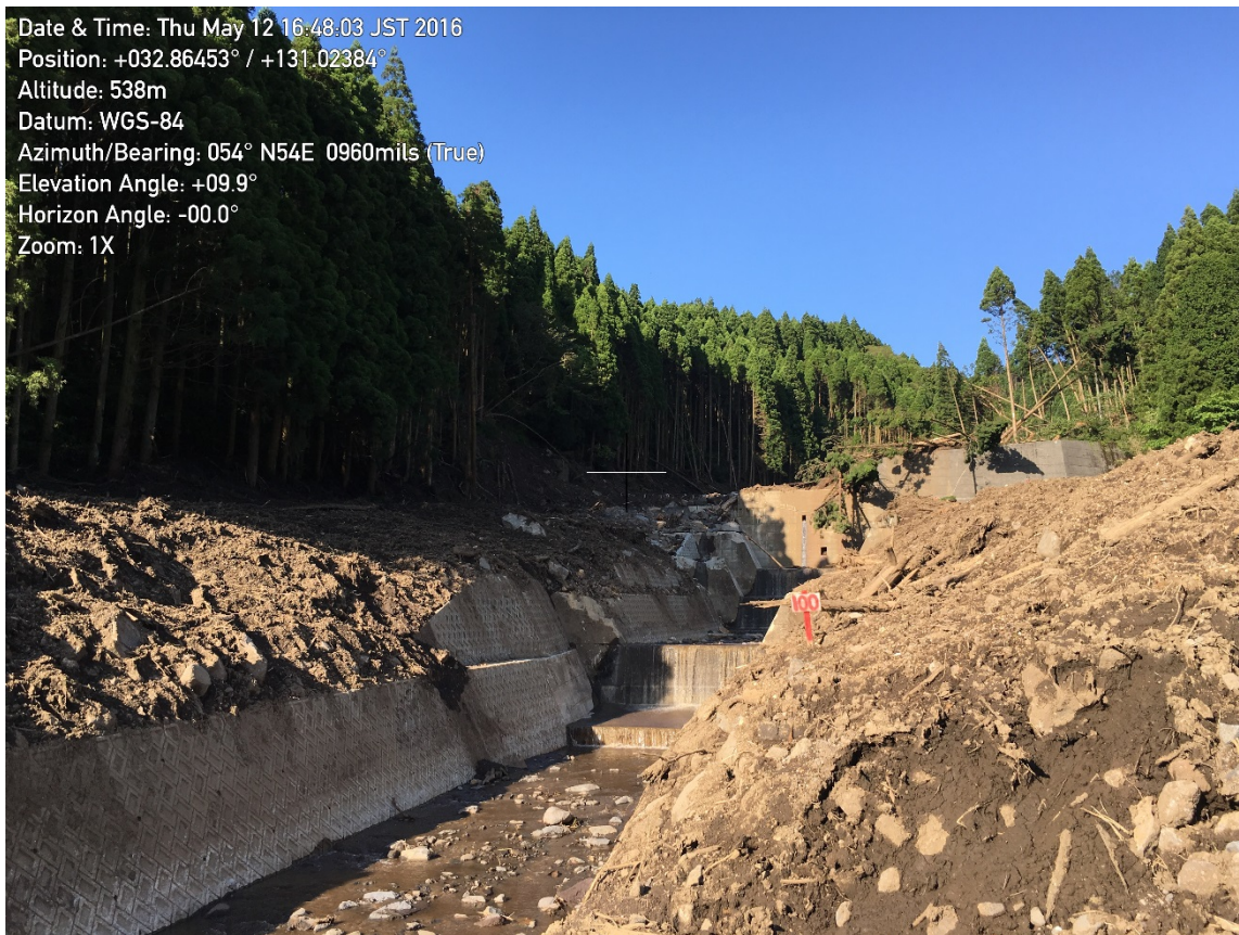
Figure 5-10. Sabo Dam that overflowed and partially collapsed as a result of sediment flows.
