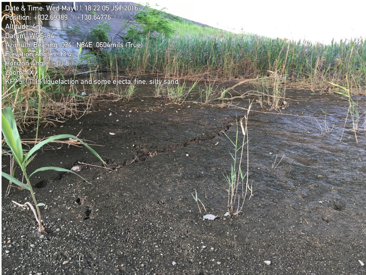
Figure 9-55. Evidence of liquefaction beneath the northern abutment of the Route 501 bridge. No evidence of significant lateral spread was observed by the research team.
