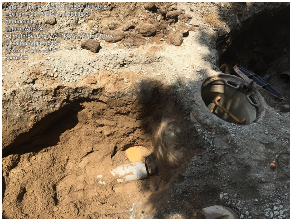
Figure 7-6. Ongoing repairs of a sewer main where surface rupture caused differential movement and disengagement of a 200-mm PVC main at both the north and south sides of a concrete manhole structure. (32.78212, 130.83507).
