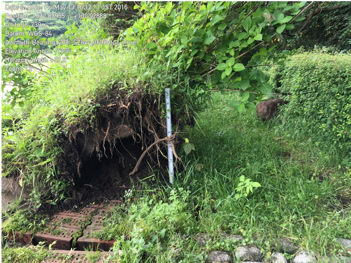
Figure 9-7. The reservoir bench at the location of the fault entrance into the reservoir. Note the vertical offset of this staircase, possibly resulting from the combination of fault movement and slope movement here.
