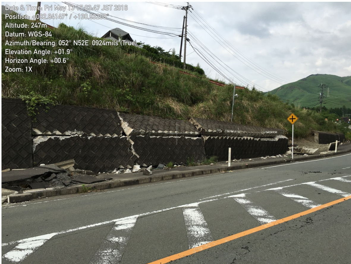
Figure 9-20. Partial collapse of an unreinforced concrete block retaining wall at the location of fault rupture, above the spillway.
