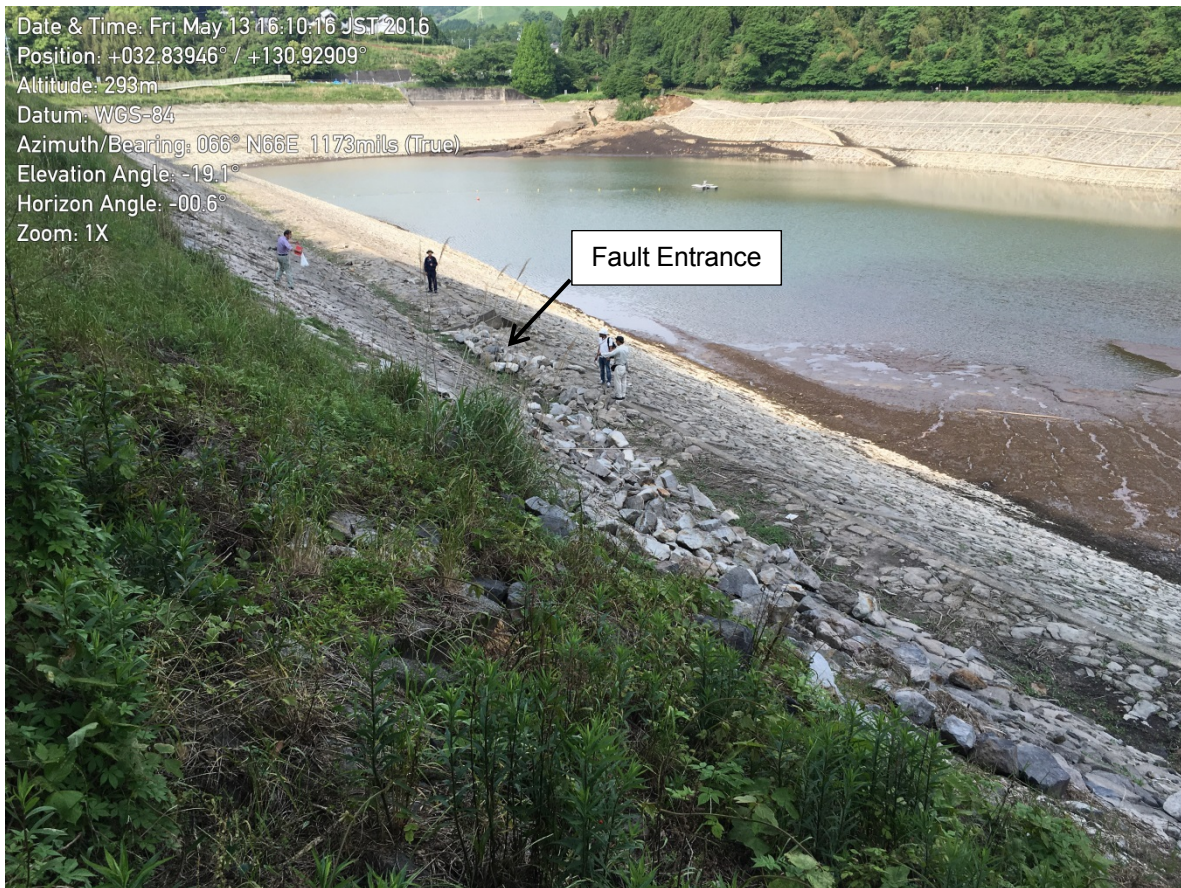
Figure 9-6. The location of the main fault strands entrance into the reservoir, visible by the “dilation” of the riprap side slope armoring.
