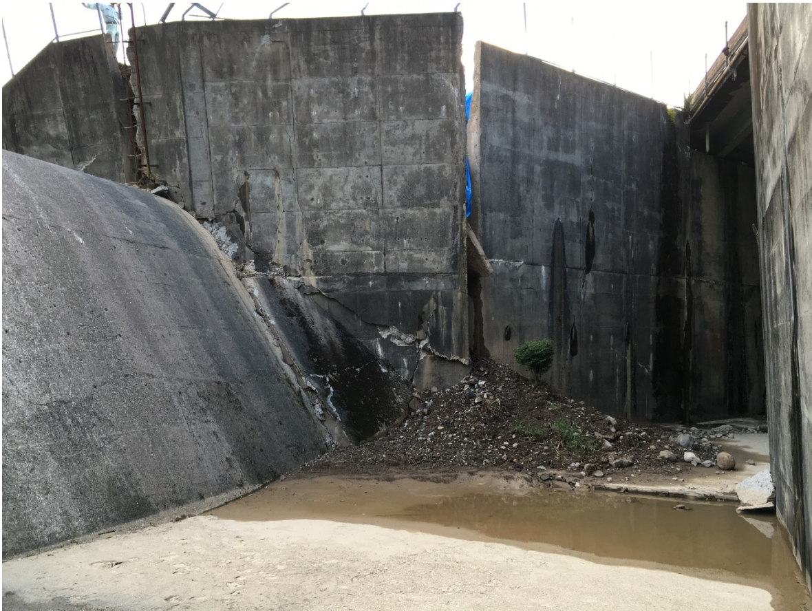
Figure 9-10. Damage and offsets at the location of fault rupture, between the spillway and the spillway outlet channel.
