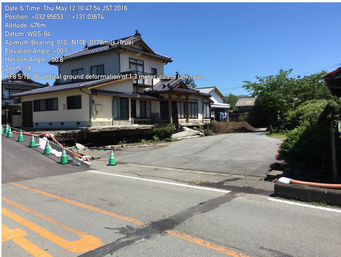
Figure 9-31. One edge of the zone of depression caused a large grade change immediately adjacent to a residential structure.
