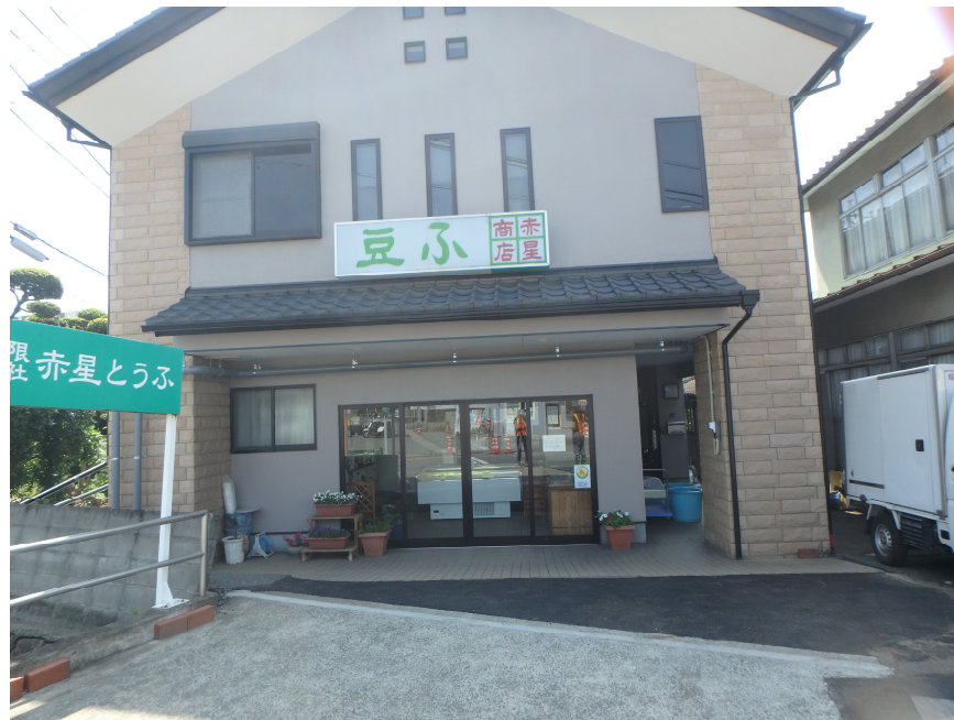
Figure 6-11. Picture of building settlement due to soil liquefaction in the south-east corner of the Shirakawa River (coordinates: 32.770086°N; 130.692403°E). Building settlement with respect to the surrounding ground on the order of 10 cm and 2 degrees tilt.
