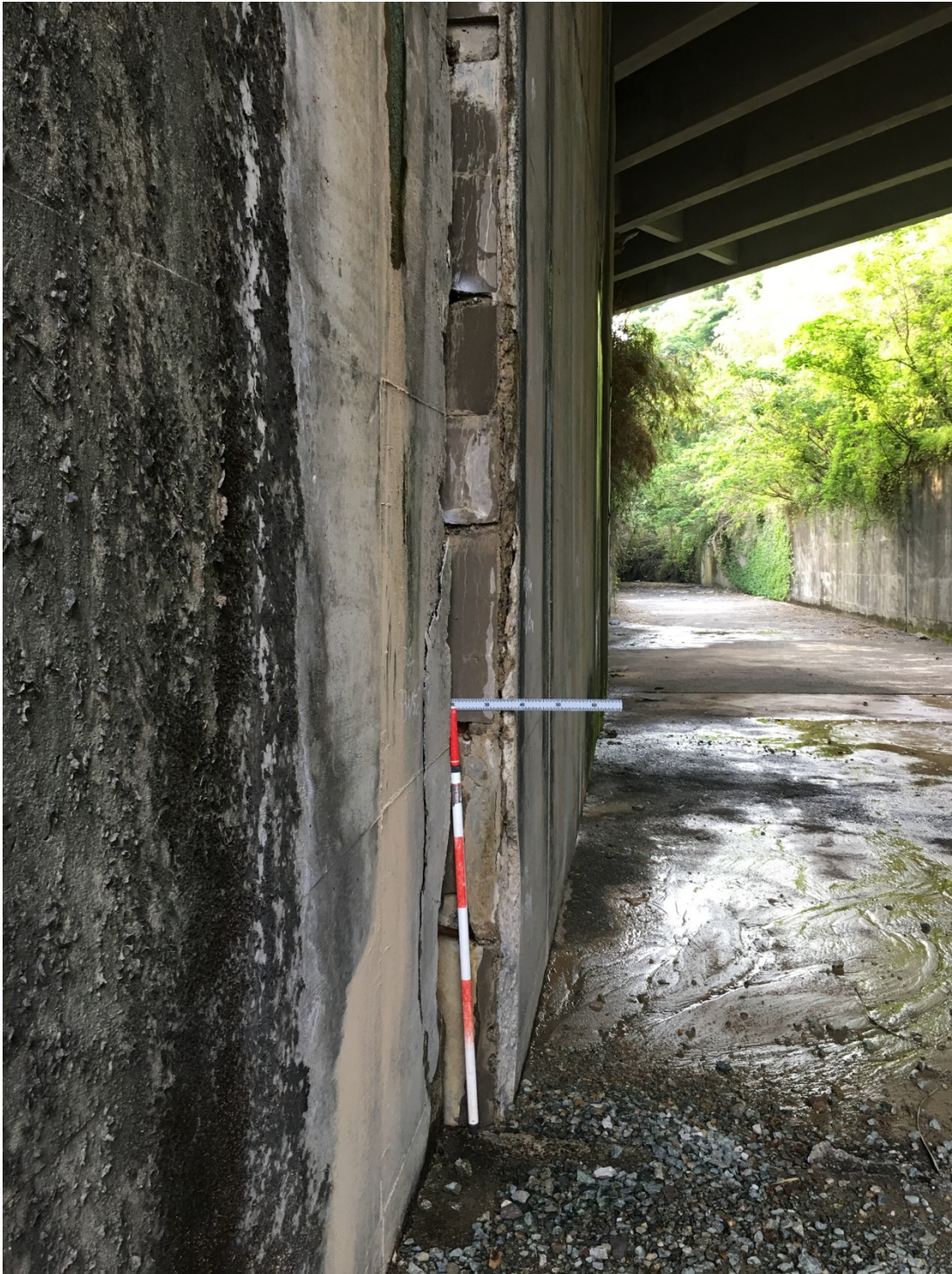
Figure 9-12. A smaller offset at a joint in the spillway outlet channel due to the movement and rotation of the spillway.
