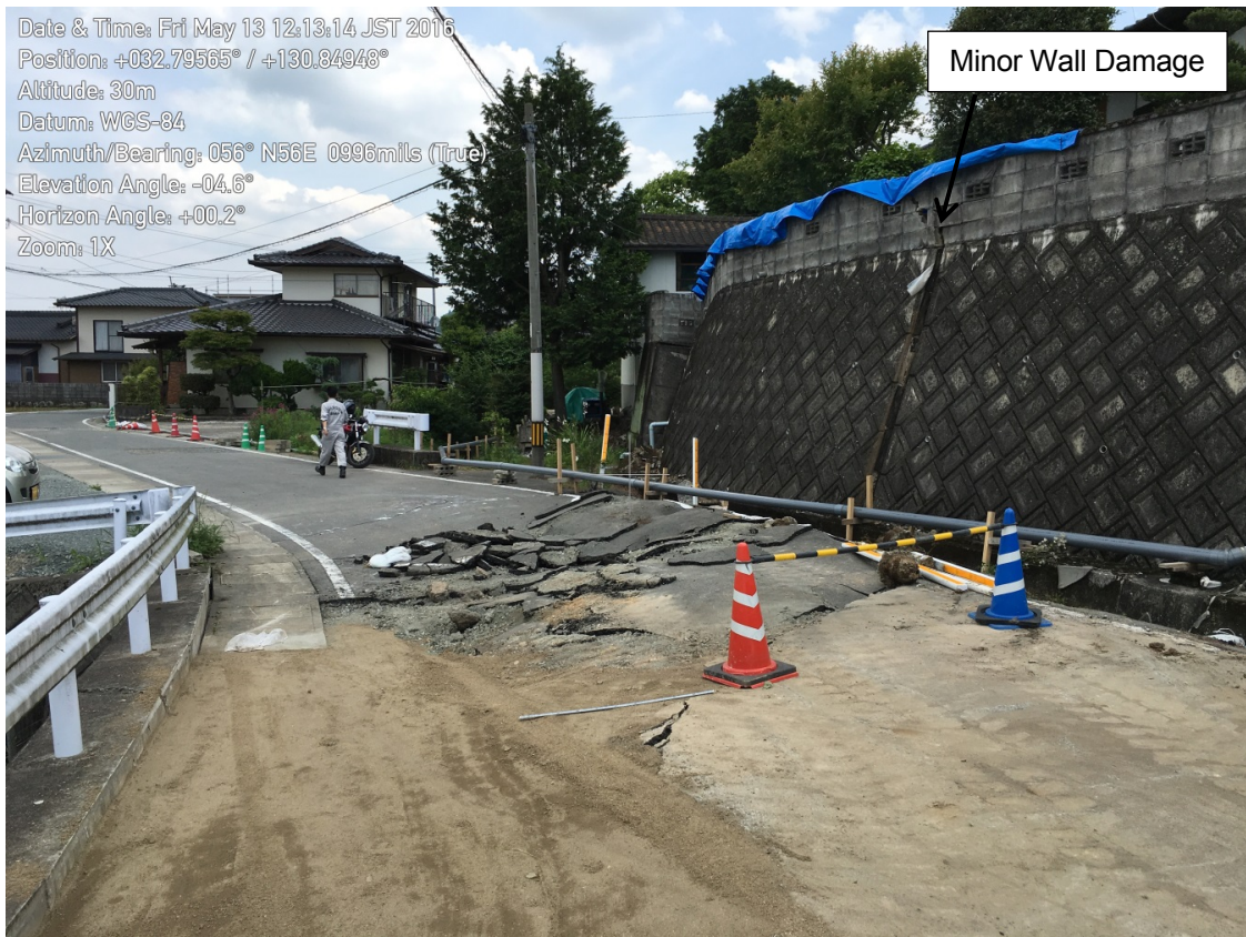
Figure 4-11. Right-lateral offset along the Futagawa Fault through a road and retaining wall, which performed relatively well.
