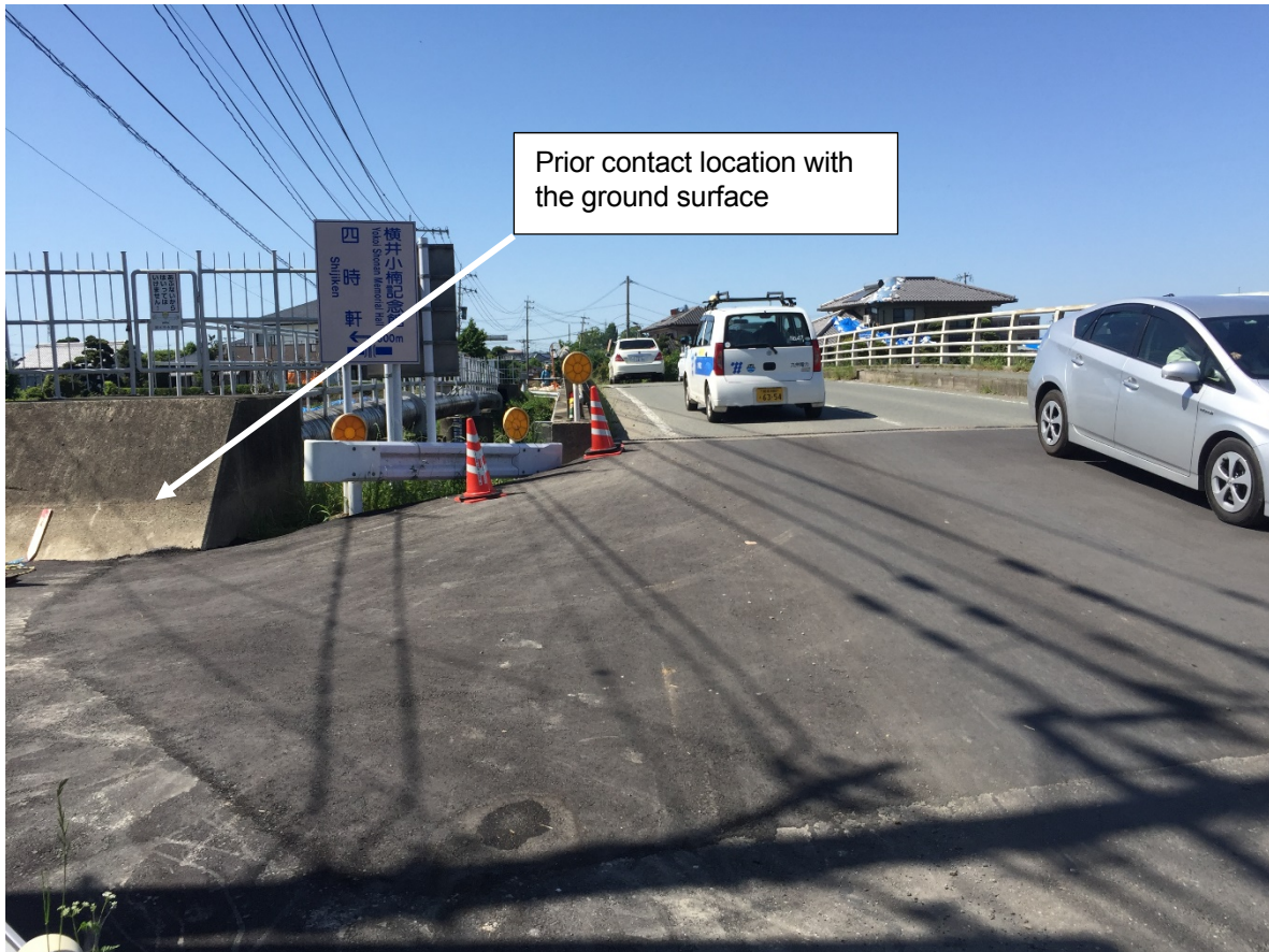
Figure 6-8. Liquefaction-induced settlement at bridge approach. Estimated settlements of 36 cm were observed at this site. Location: 32.77322° N 130.78433° E
