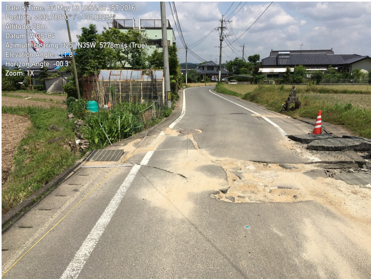
Figure 4-6. Roughly 0.65 m to 0.70 m of right-lateral offset along the Futagawa Fault through a road.
