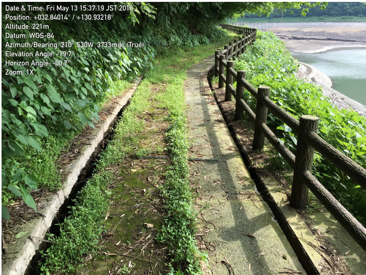
Figure 9-2. Slope displacements typical of nearly the entire bench running the circumference of the dam.
