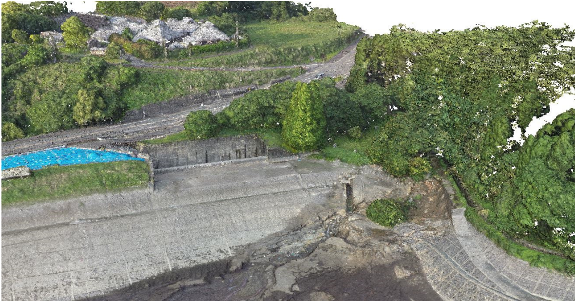
Figure 9-26. Screenshot of the 3D dense point cloud of the dam developed from UAV-based imagery (32.84123, 130.93158).
