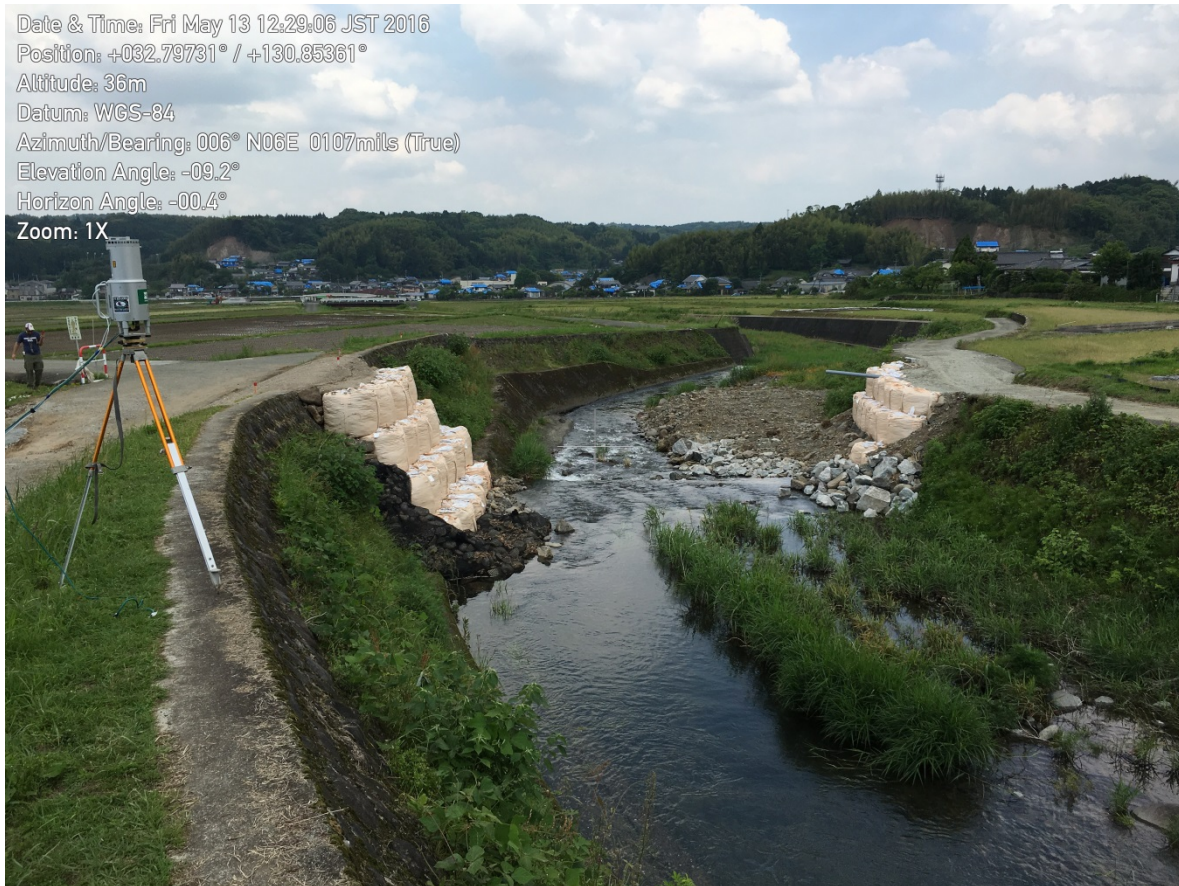
Figure 9-47. Terrestrial LIDAR setup at the fault crossing of the canal. Vertical movement of the fault strands and the associated popup block can be seen in the photo. Repair work is evident at the location of the main southern strand fault crossing.
