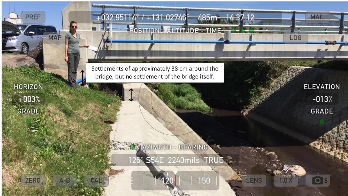
Figure 9-34. No foundation settlement at the west bridge abutment located in the depression zone.
