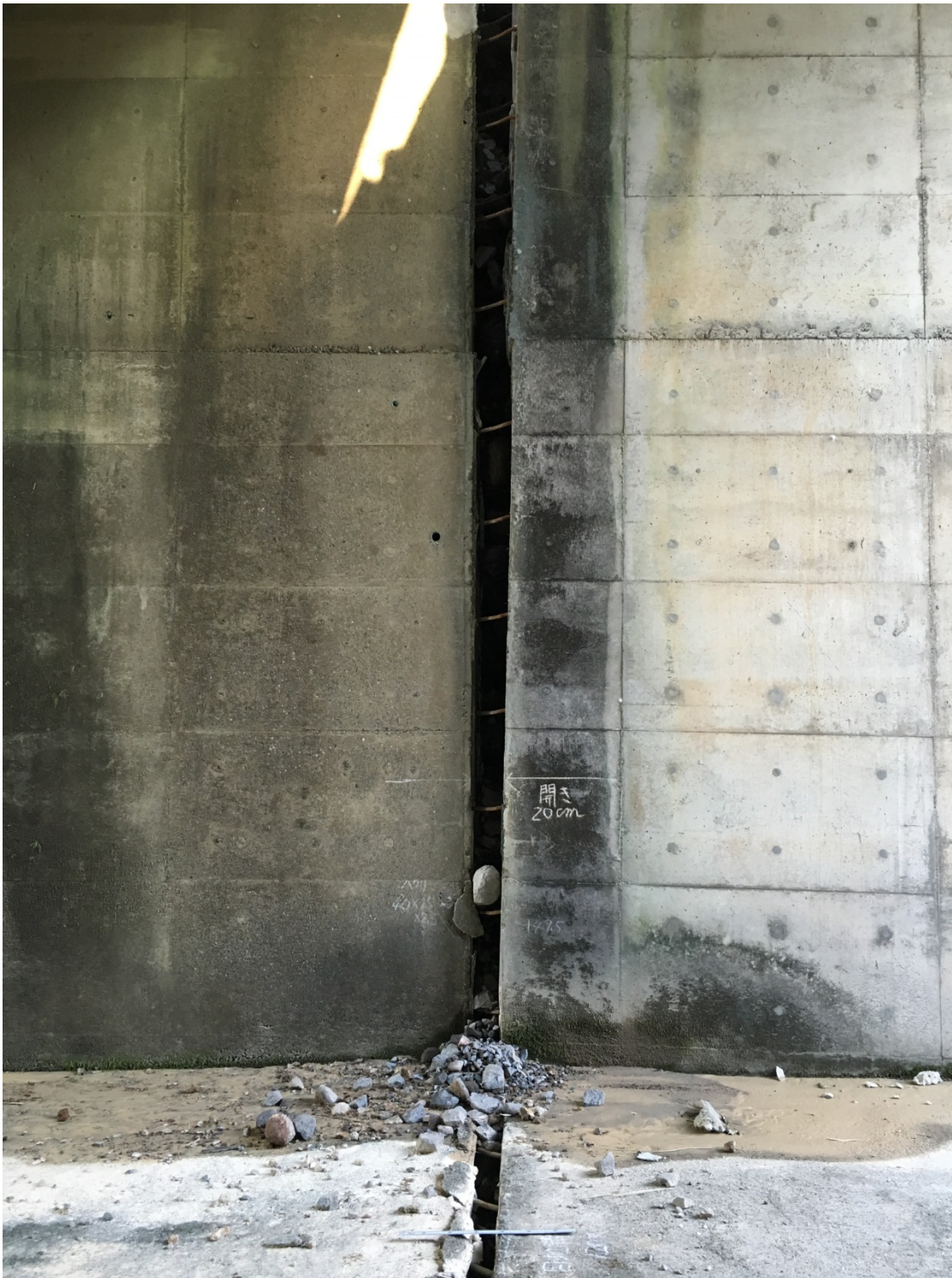
Figure 9-13. Another offset at a joint in the spillway outlet channel due to the movement and rotation of the spillway. Note the change in horizontal separation from top to bottom.
