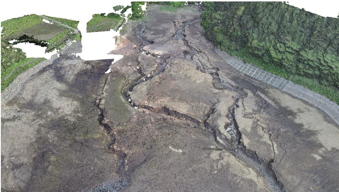
Figure 9-27. Screenshot of the 3D dense point cloud of the erosion zone in the dam; developed from UAV-based imagery (32.84123, 130.93158 ).
