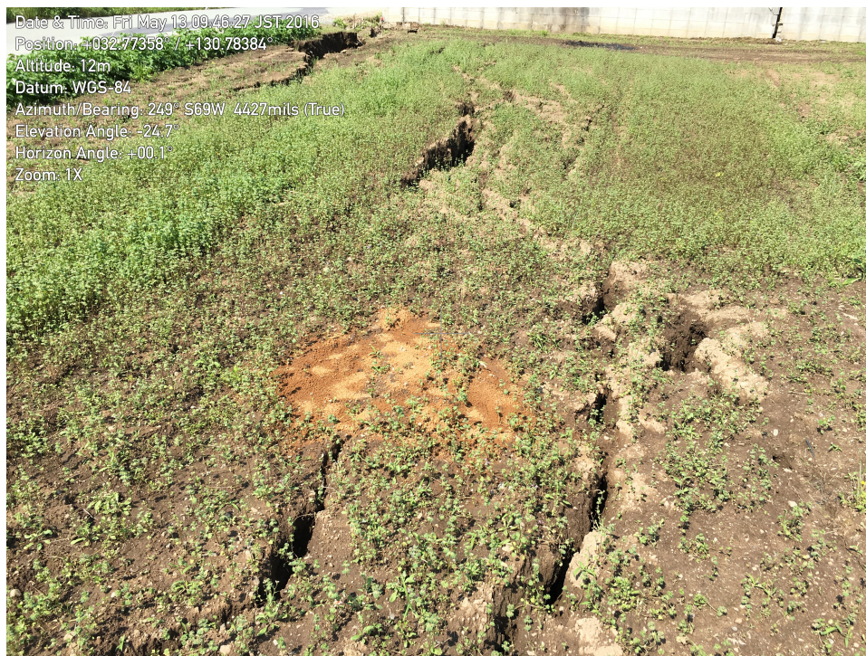
Figure 6-16. Ground cracking from lateral spread and observed ejecta.
