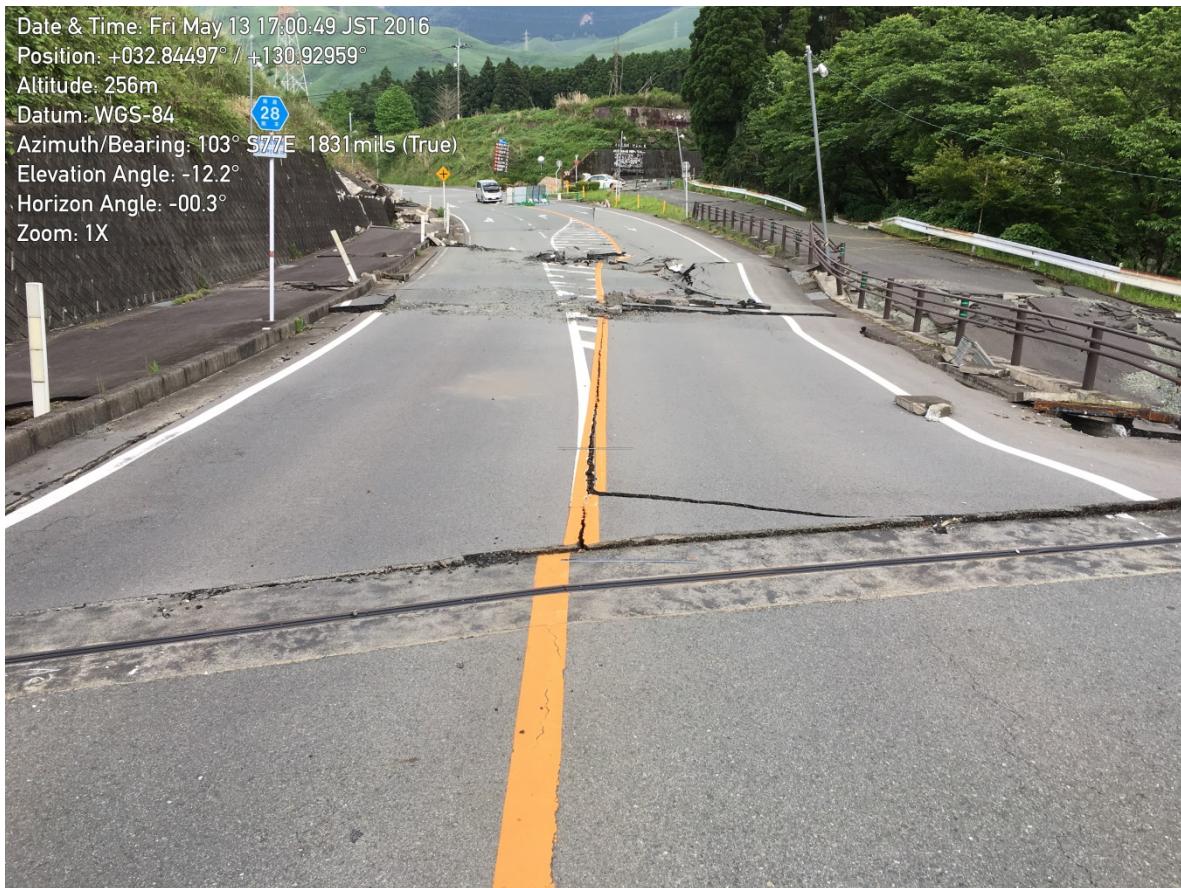
Figure 9-19. Fault rupture through the highway above the dam spillway.
