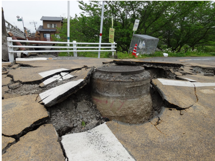
Figure 7-5. Differential movement between sewer manhole and ground surface likely caused by liquefied pipeline backfill (photo courtesy of JSCE).
