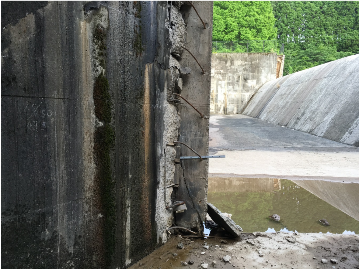
Figure 9-11. Detail of the main fault offset, through the intersection of the spillway and spillway outlet channel.
