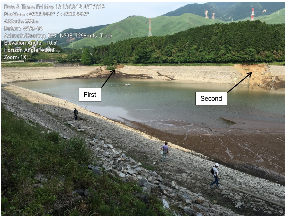
Figure 9-4. The two collapsed side slopes of the reservoir.
