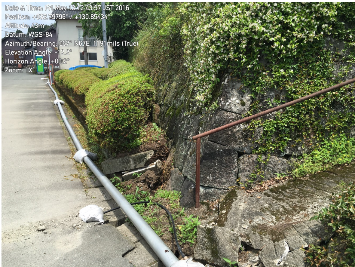
Figure 9-48. Fault rupture through a road and a retaining wall on the Futagawa Fault. No significant damage observed in the stone block retaining wall.
