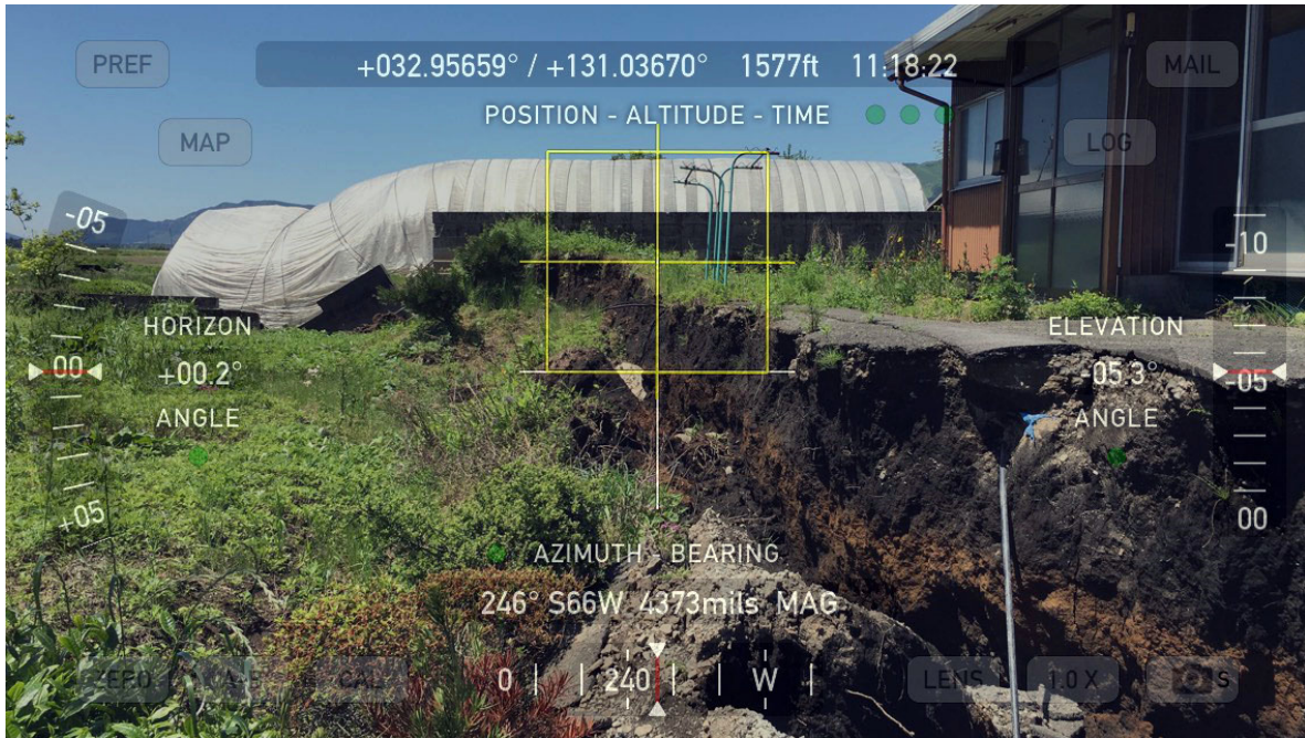
Figure 9-32. One edge of the zone of depression crosses next to a residential structure and beneath a greenhouse structure.
