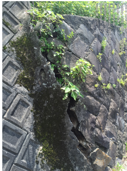
Figure 4-9. Roughly 0.4 m of right-lateral offset along the Futagawa Fault through a concrete block retaining wall.
