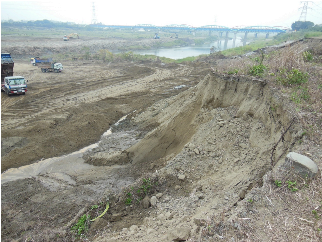
Figure 8-8: Seepage at Base of Scarp at Impervious Contact (23.1537, 120.3434).
