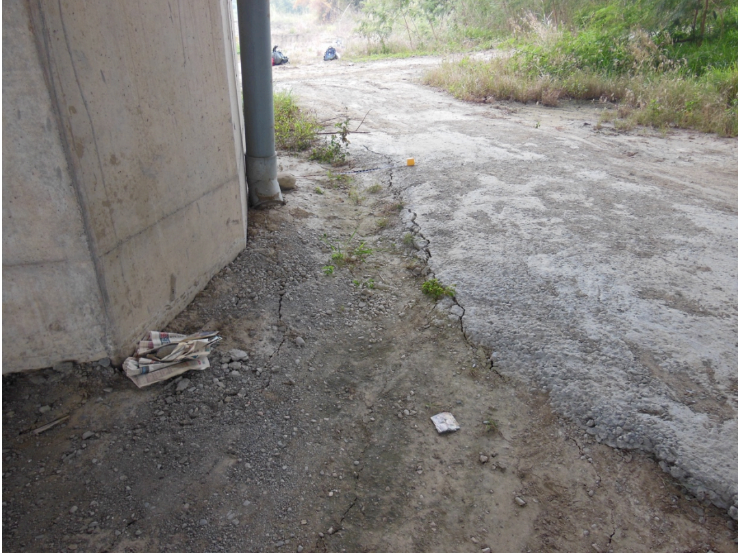
Figure 8-11: Nested Arcuate Cracking Behind the Piers (looking northwest) (23.153514, 120.343736).
