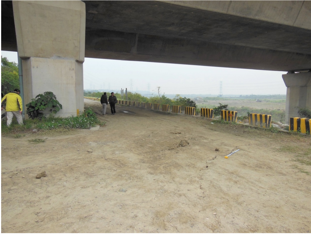
Figure 8-10: Arcuate Crack Extending to the Bridge Piers (23.153583, 120.343650).
