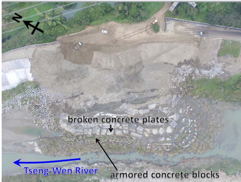
Figure 8-14: Aerial View of failure No.2. Notice the long runout distance of the materials. (Photo: W.-K. Huang) ( 23^{\circ} 9'3.26'' , 120^{\circ}20'47.59'' ).
