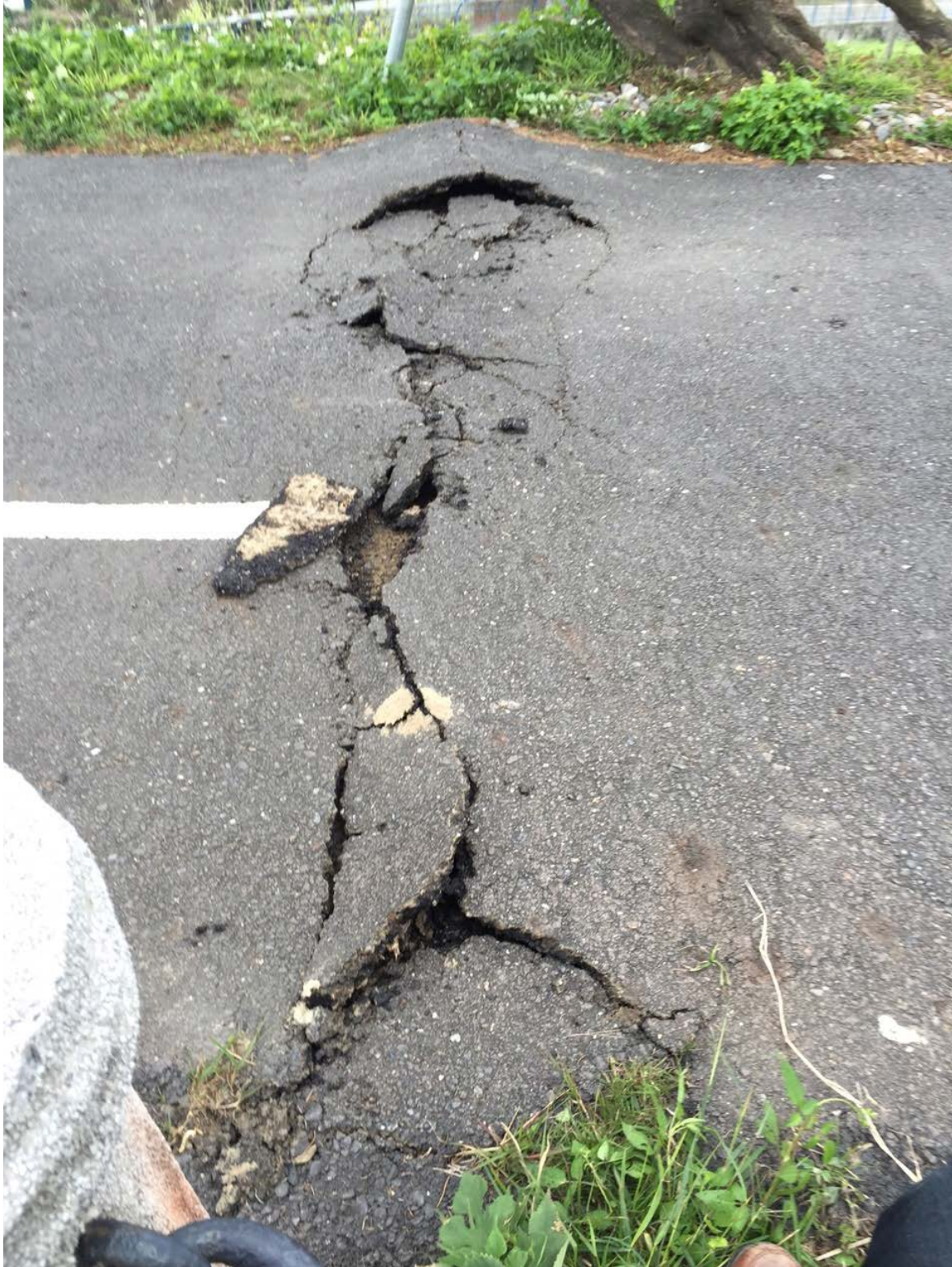
Figure 9-14: Cracking of the AC Pavement (Lat: 23.025606, Long: 120.337445).
