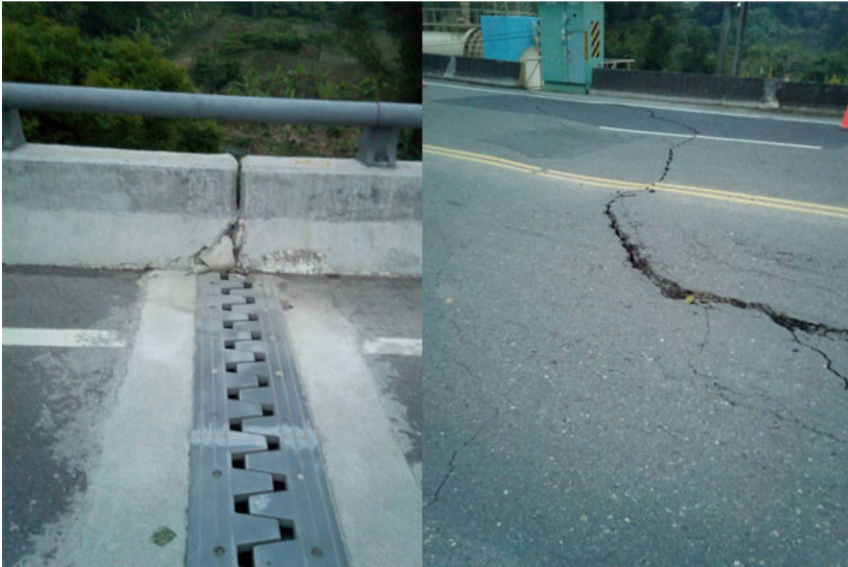
Figure 6-7: Pavement and Bridge Deck Distress along Tai-3 Highway.
