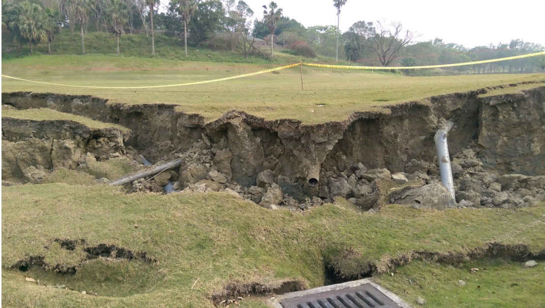
Figure 8-43: Watering pipes along the surface rupture. (23.151721, 120.370245)
