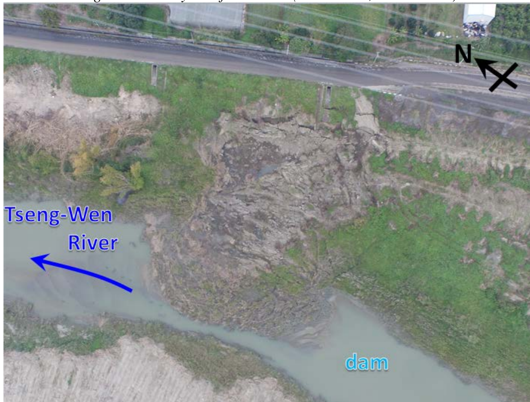
Figure 8-27: Aerial view of failure No.3. (Photo: W.-K. Huang). ( 23.148325, 120.347631)
