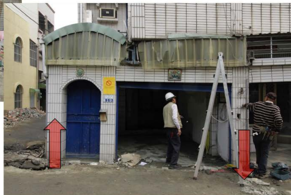
Figure 7-25: Structural hinge mechanism developed due to movement of unconnected foundations at carport add-ons at the Xinshi site. ( 23.08096, 120.30258 ).
