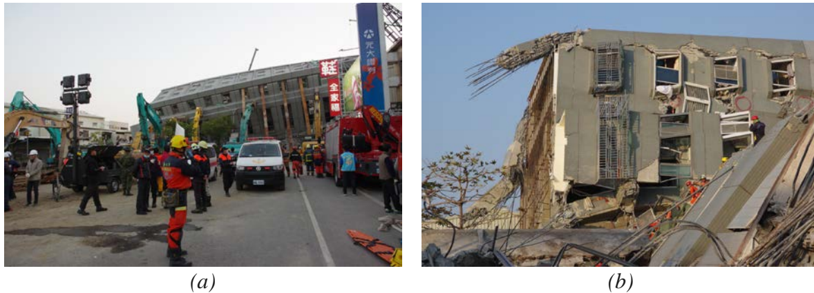
Figure 5-9: Weiguan Jinlong complex (120.261,23.0052): (a) North column damage to building and (b) close-up of building column reinforcement, which directly pulled out at the first floor. (images courtesy of Justin Shih).
