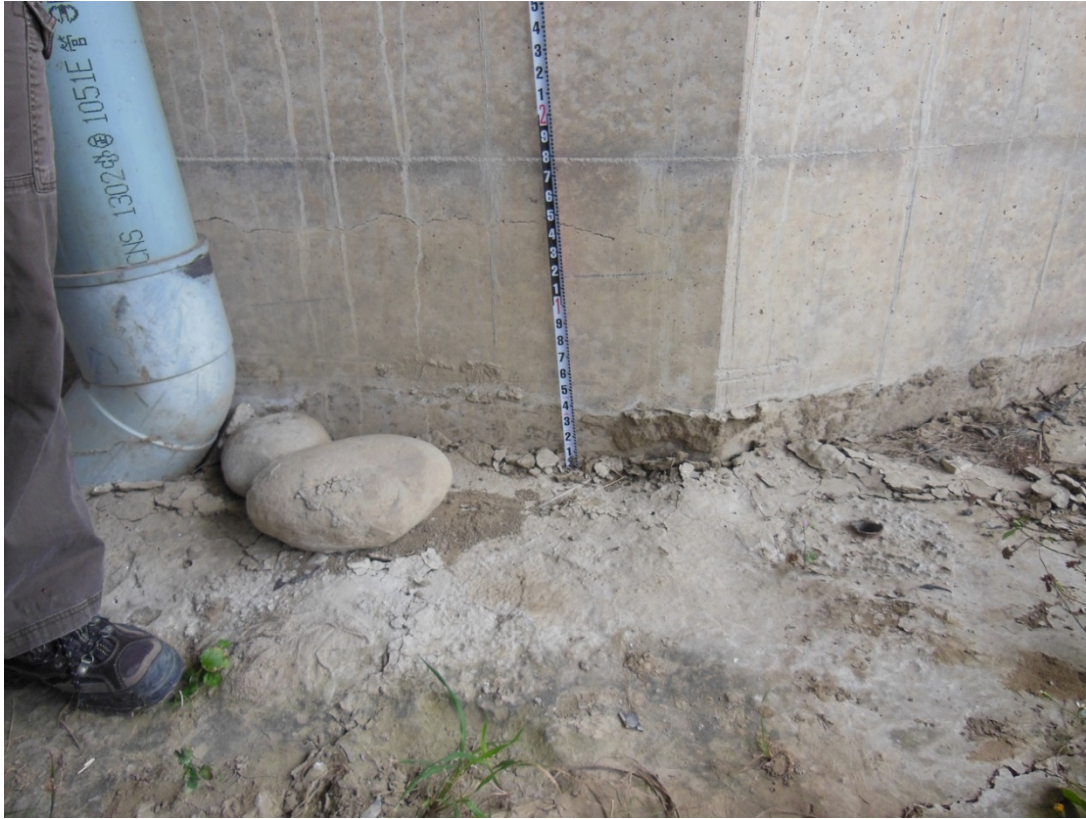
Figure 8-12: Settlement Around Bridge Prier is about 4 to 5 inches (23.153514, 120.343736).
