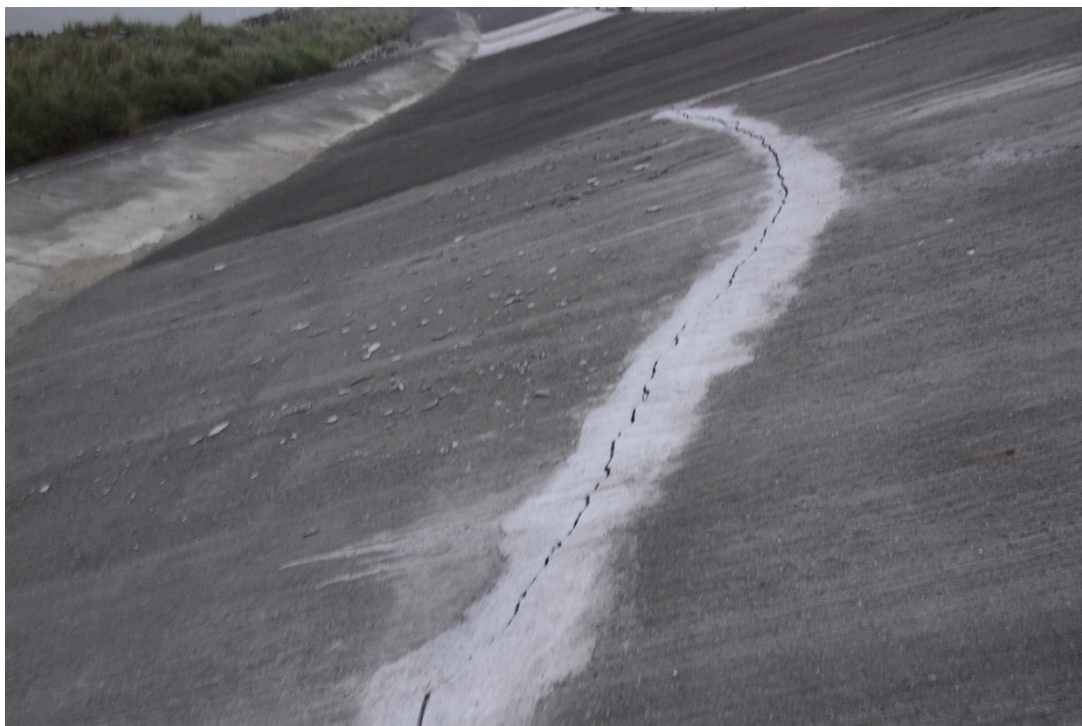
Figure 8-34: Re-cracking of Recently Repaired Cracking (23.121176°,120.379569°).
