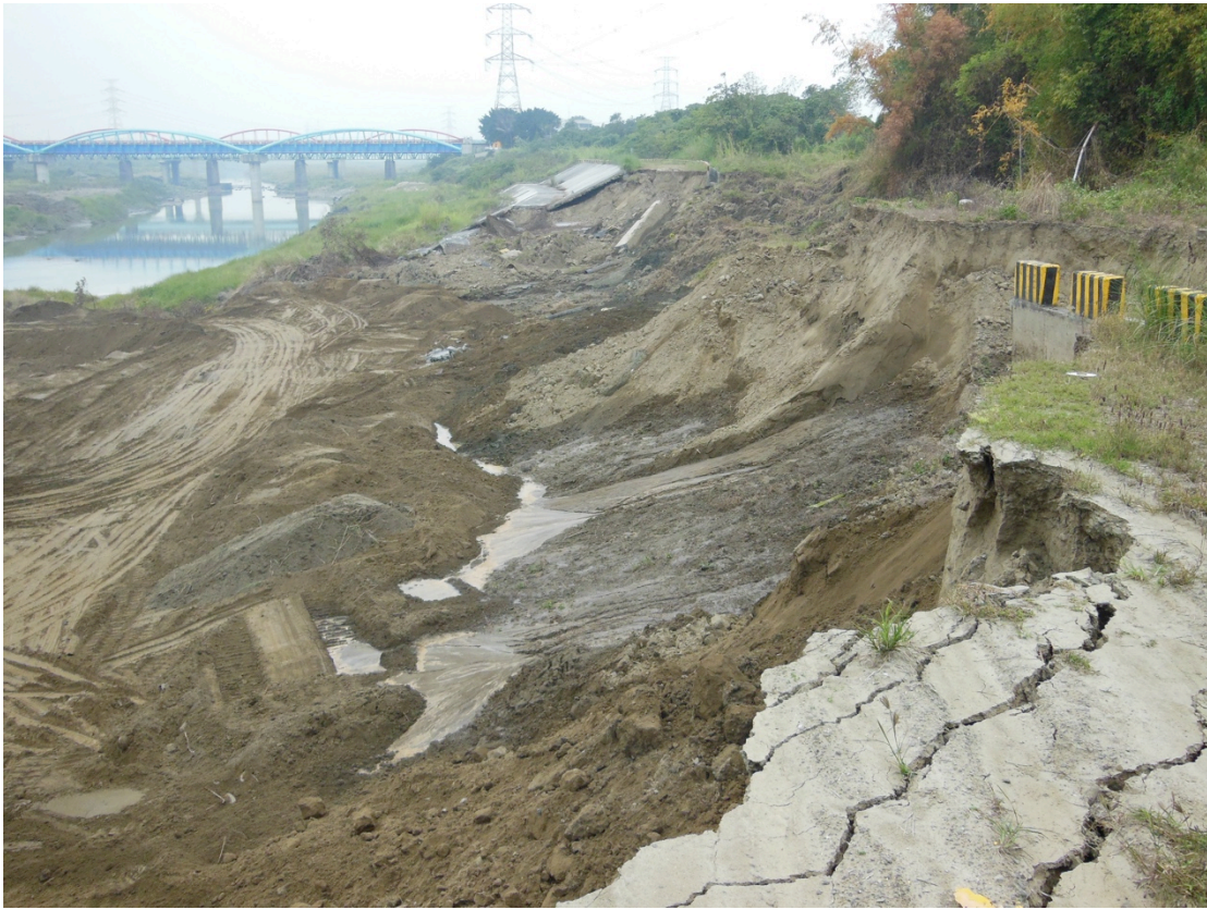
Figure 8-6: Failure 1 Looking Northwest (23.1537, 120.3434).
