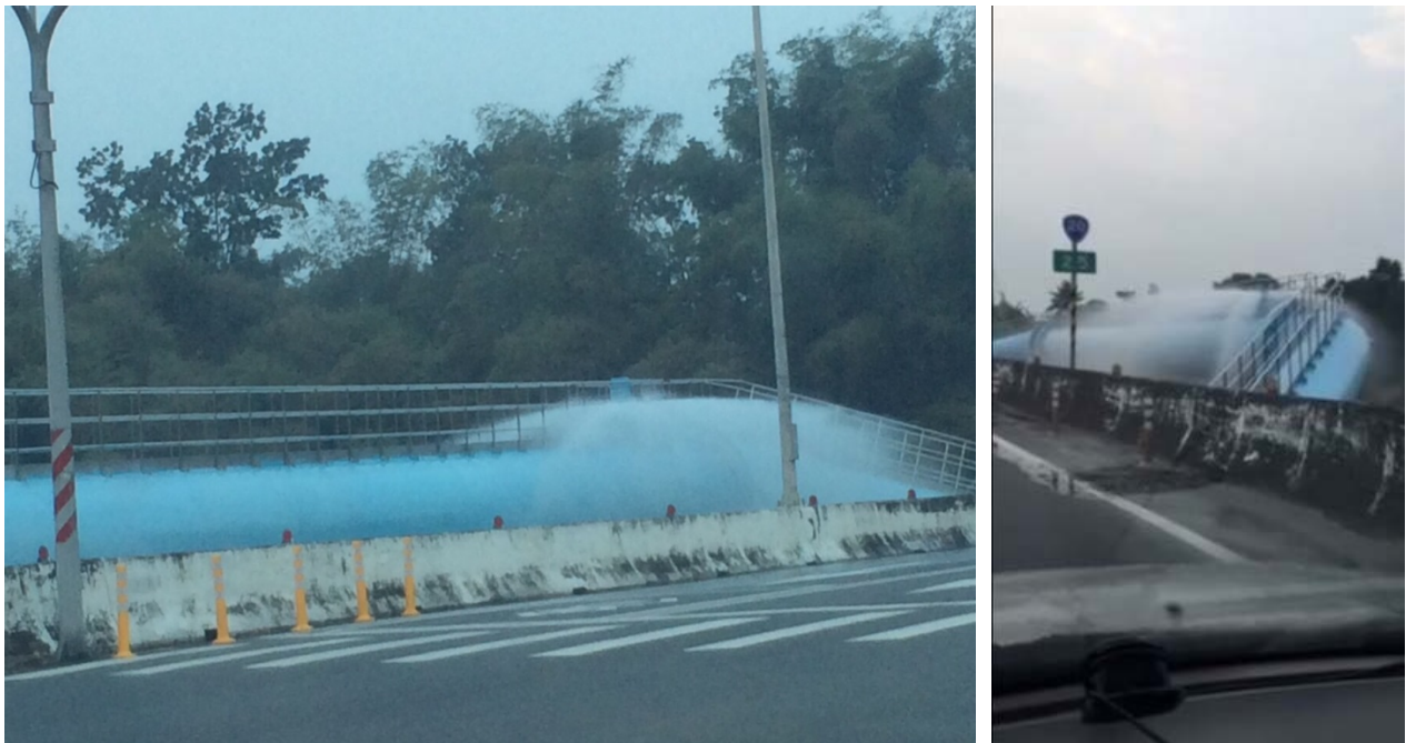
Figure 6-4: Damaged 2000 mm Water Pipeline near Bridge in Yung Kang District (開運橋頭永康側) (23.034244, 120.286719).
