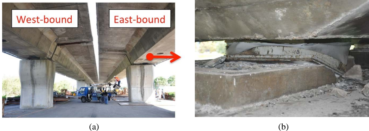
Figure 6-1: Provincial highway 86 bridge # 24: (a) separation of east and west bound elevations and (b) failure of hinge bearing at RP9. (Images courtesy of Dr. Kuang-Yen Liu, NARLabs).
