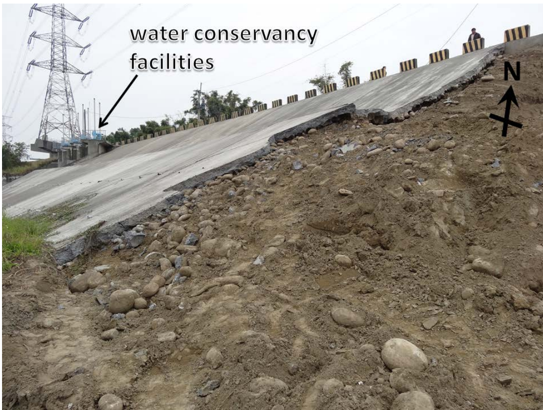
Figure 8-16 Concrete Slab and Piles Used to Protect Area near Levee Failure No.2. (23.151245, 120.346236).
