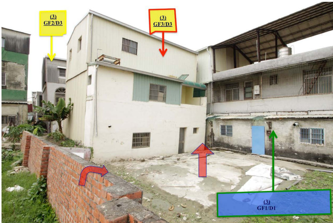
Figure 7-8: Example of mapping GF1 through GF3; demonstrating various structural damage states. (23.025409°, 120.207565°).
