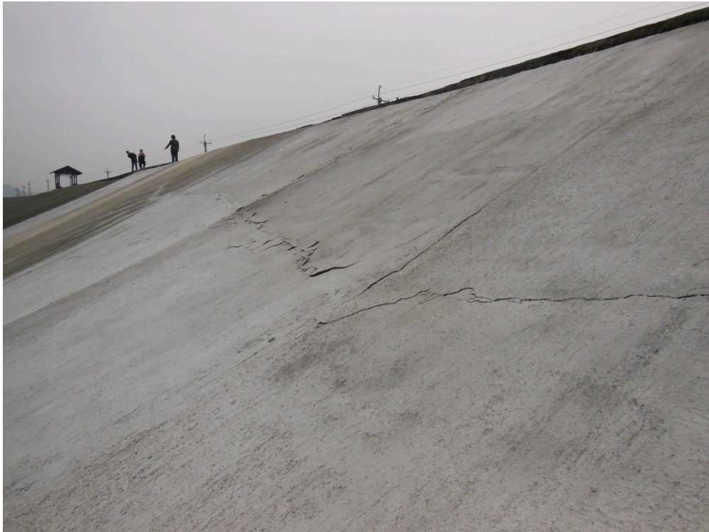
Figure 8-33: Shear Cracking of the Repaired Concrete Slab (23.121176°,120.379569°).
