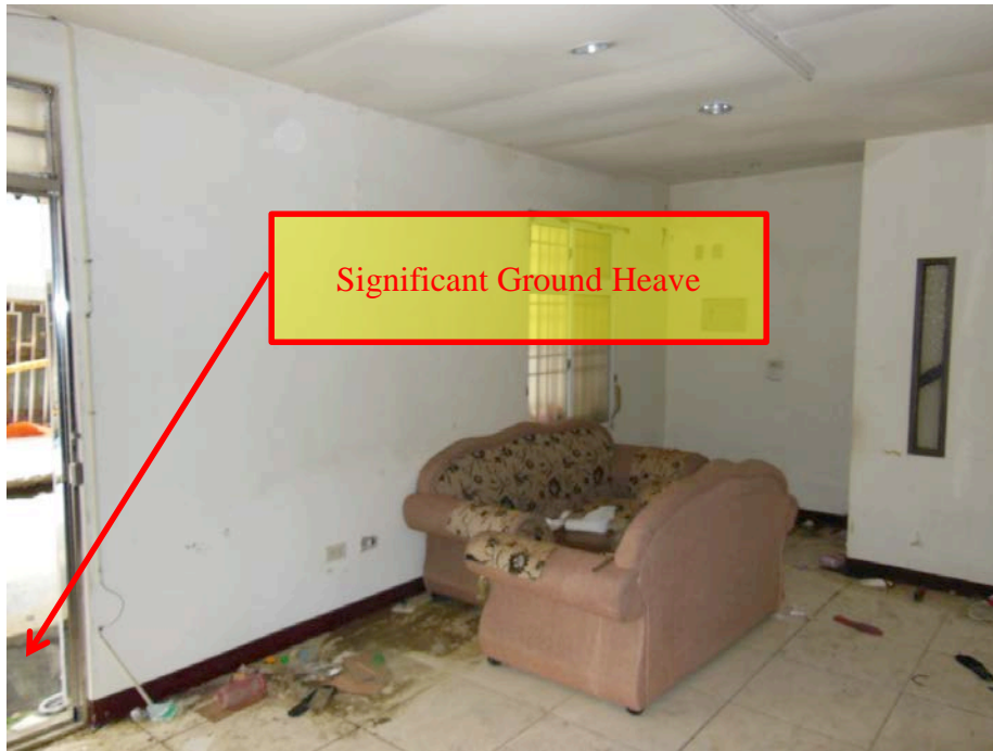
Figure 7-11: Building that survived liquefaction-induced settlement and ground heave ( 23°01'31.5"N 120°12'25.8"E ).
