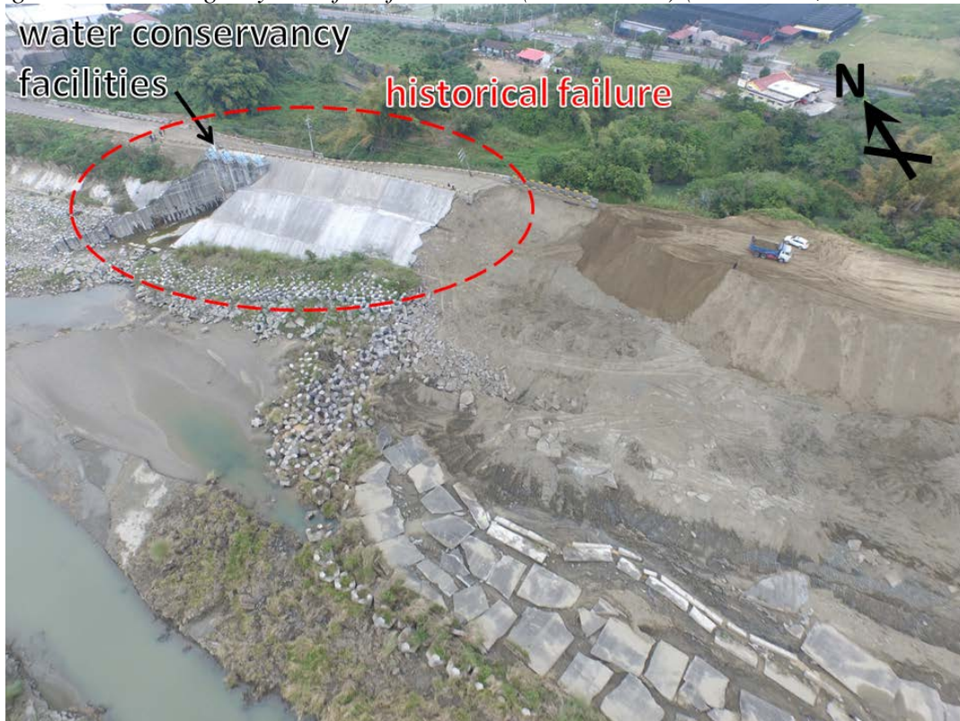
Figure 8-25: Historical Failure Near Failure No.2. (Photo: W.-K. Huang). (23.150949, 120.346590).
