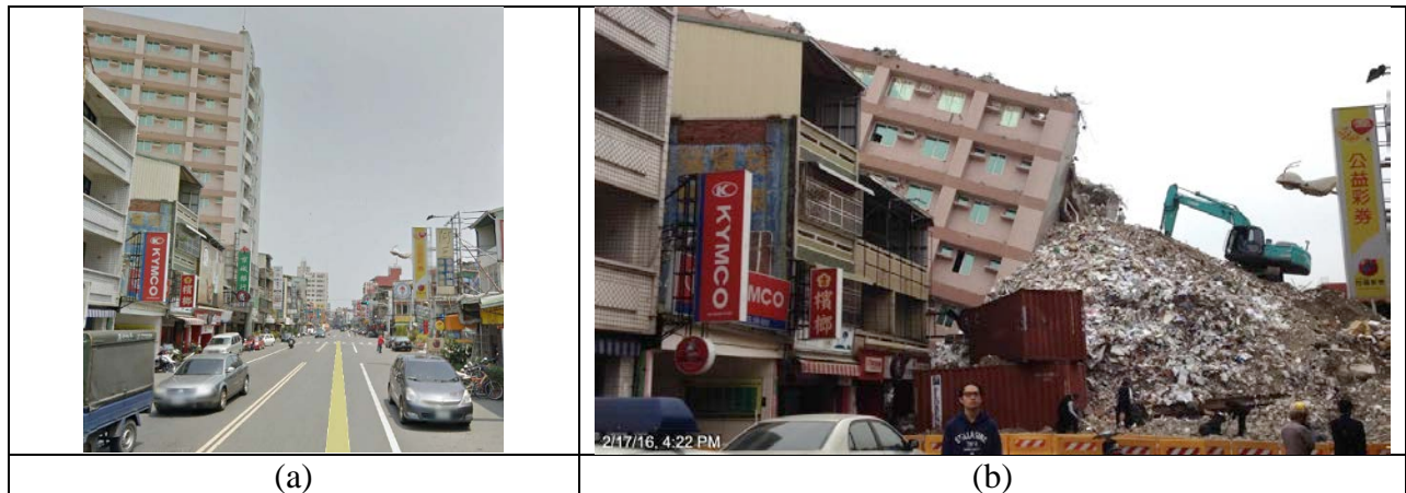
Figure 5-11: King's Town Bank (a) prior to earthquake and (b) during demolition (February 18, 2016) – both views looking East (23.036, 120.301).
