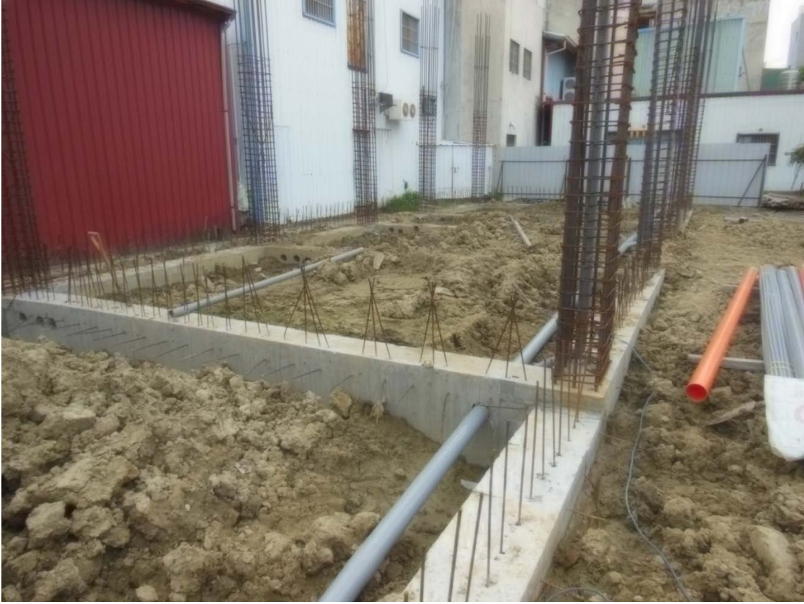
Figure 10-4: Modern grade beam design in Taiwan (building under construction in Tainan City).
