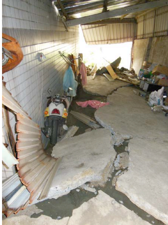
Figure 7-12: Damaged unreinforced slab in liquefied soil of the illegal expansion behind the building shown in the left portion of Figure 7-9 (23.0253°, 120.2074°).
