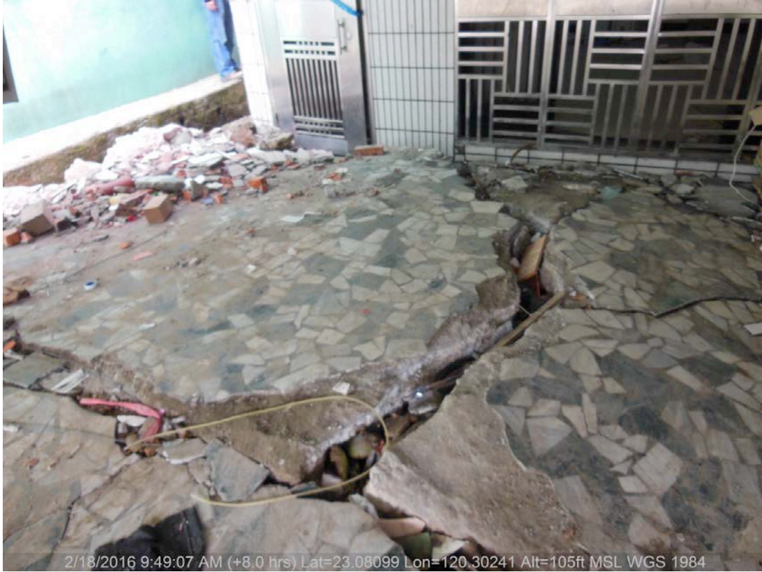
Figure 7-27: Damaged unreinforced car port slab due to ground heave ( 23.08099, 120.30241 ).
