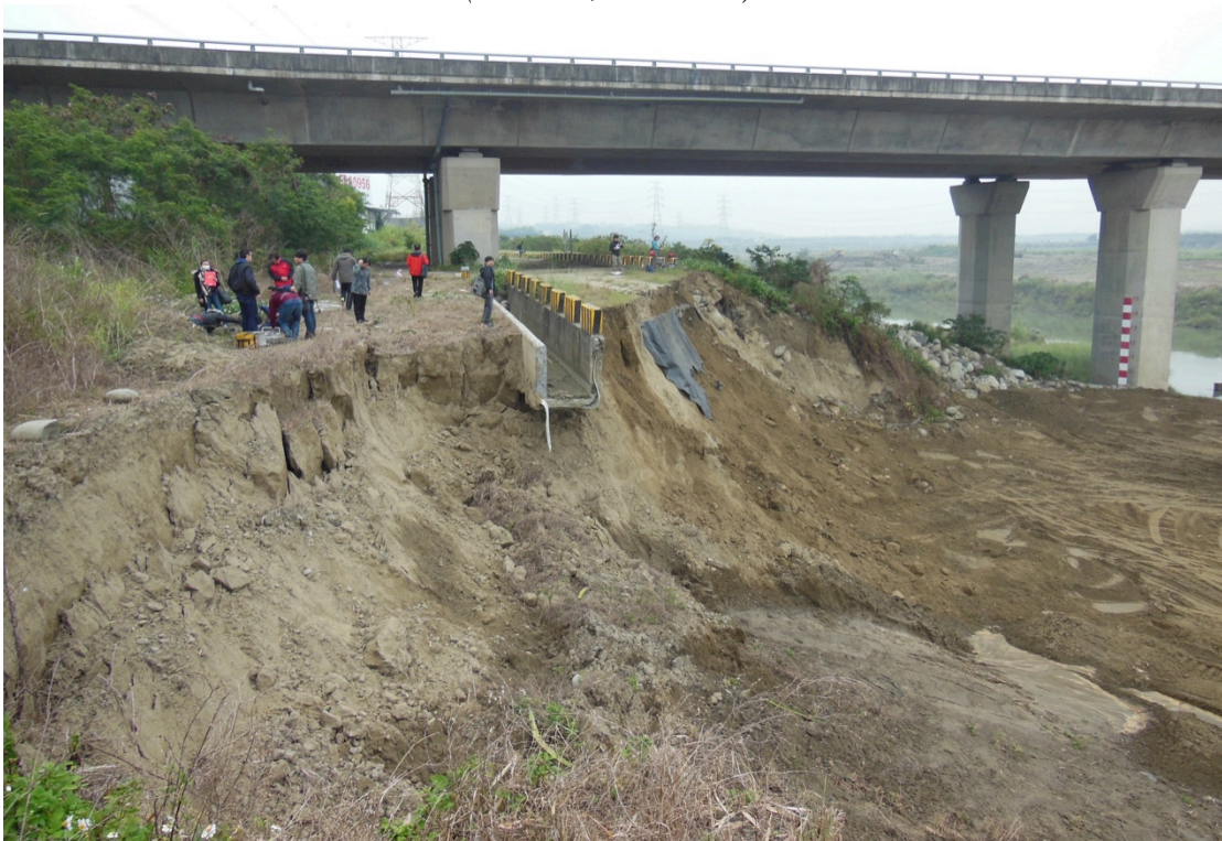
Figure 8-9: Southwest Margin of Failure 1 (23.153889, 120.343178).
