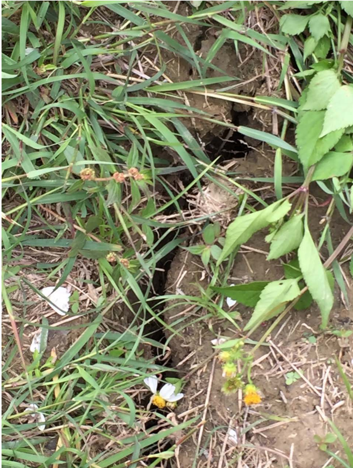
Figure 9-15: Cracking Developed in the Downstream Embankment (Lat: 23.025497, Long: 120.337569).
