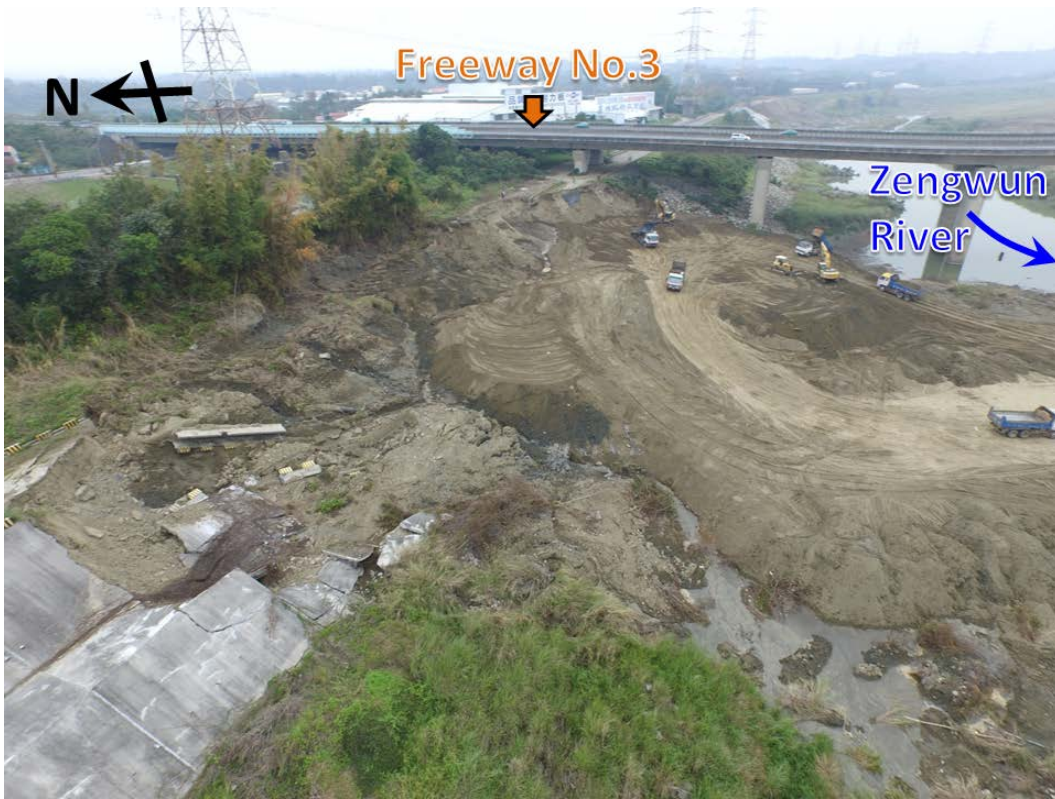
Figure 8-4: Bird's View of Failure No.1. (Photo provided by W.-K. Huang) (23.154135, 120.342255).
