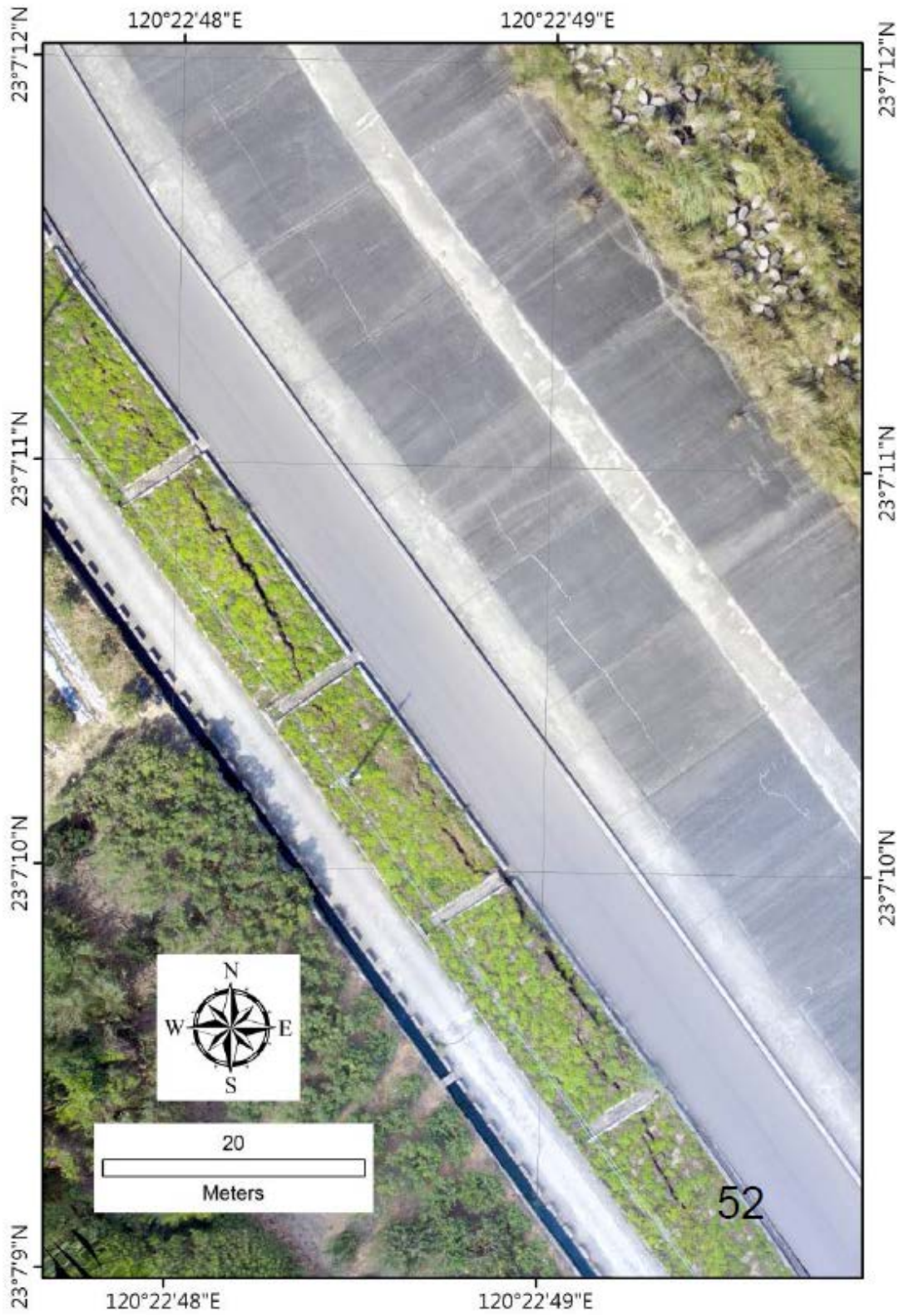
Figure 8-39: Cracking Occurring along Landslide Toe (Photo from NCREE ).
