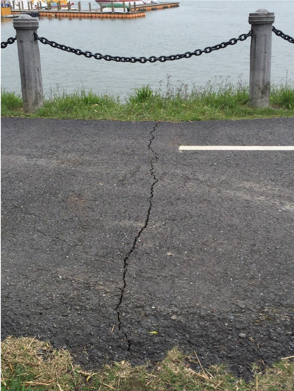
Figure 9-16: Cracking Developed in the Embankment (Lat: 23.026056, Long: 120.336966).
