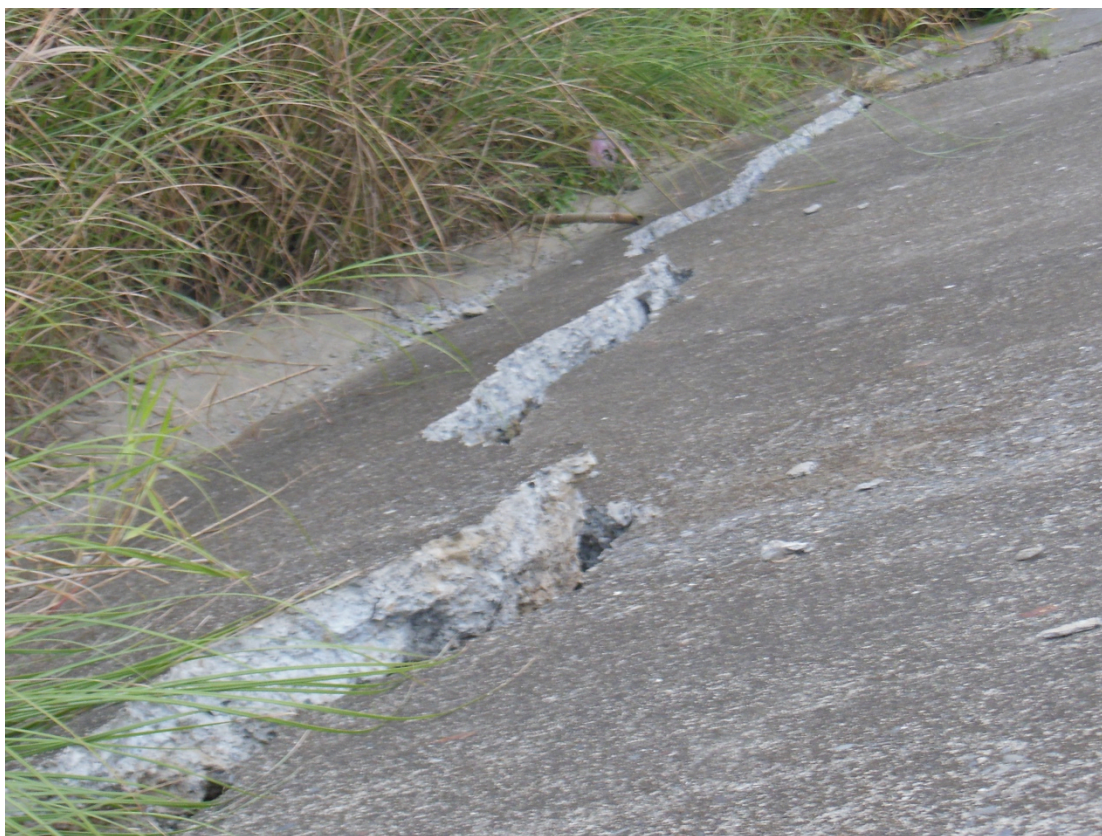
Figure 8-35: Slab Damage at Levee Toe (23.121176°,120.379569°).
