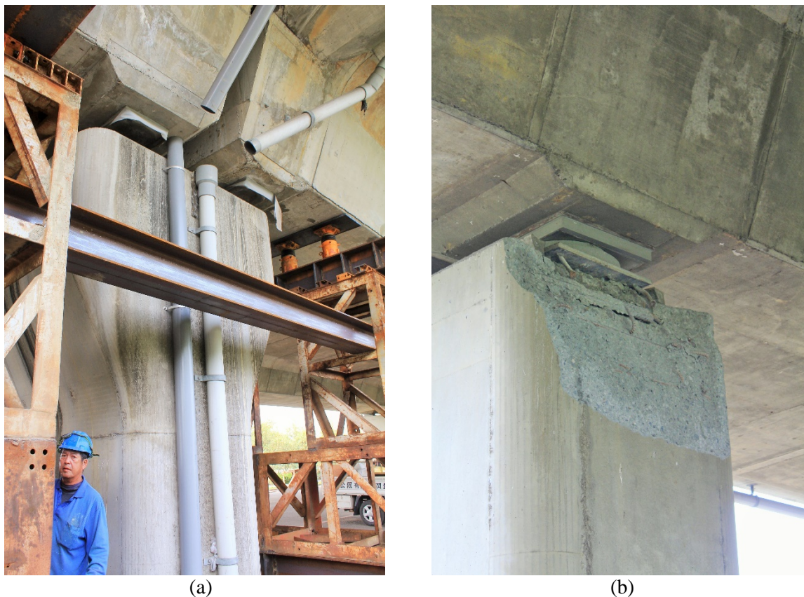
Figure 6-2: Provincial highway 86 bridge # 24: (a) east bound direction support repair (note separation of drainage lines and sheared hinges) and (b) failure of hinge and concrete support for west bound direction.
