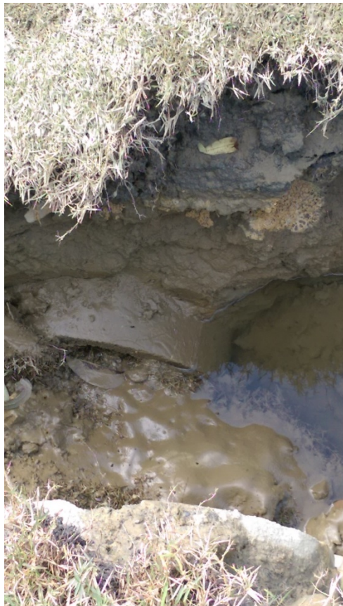
Figure 8-44: broken drainage pipe.( 23.151721, 120.370245)
