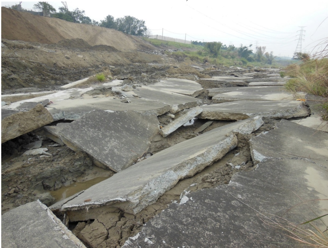
Figure 8-17: Area of the Pushed Out Toe (23.150801, 120.345807).
