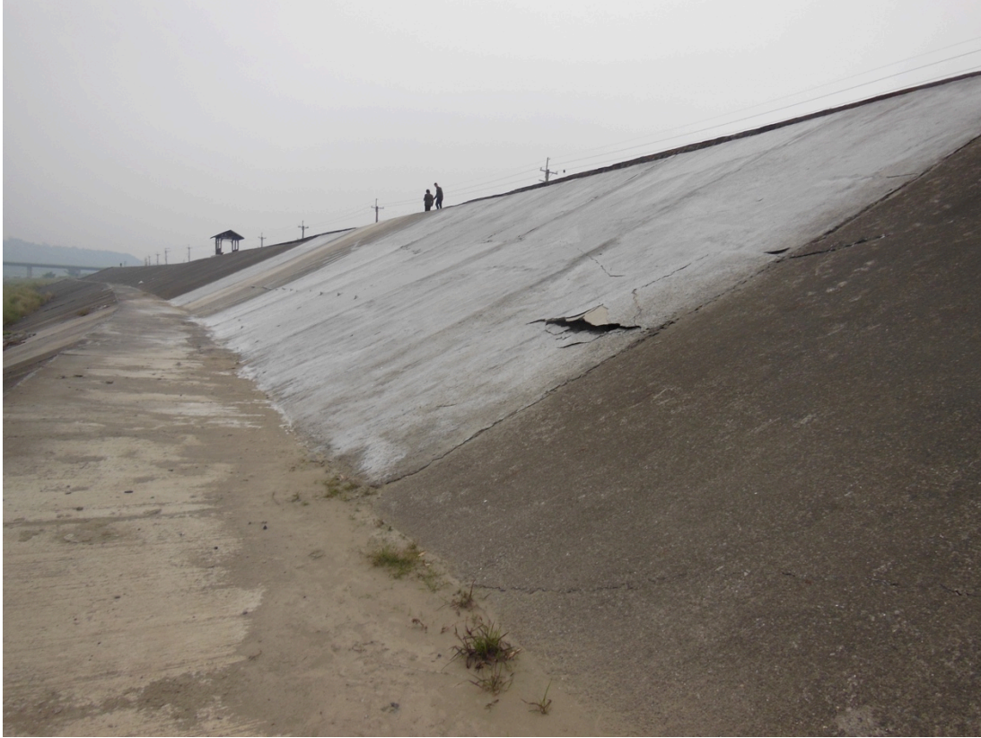
Figure 8-32: Buckling of Repaired Slab (23.121176°,120.379569°).
