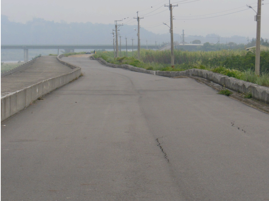
Figure 8-38: Undulation of Levee Crest Road (23.120114, 120.379819).
