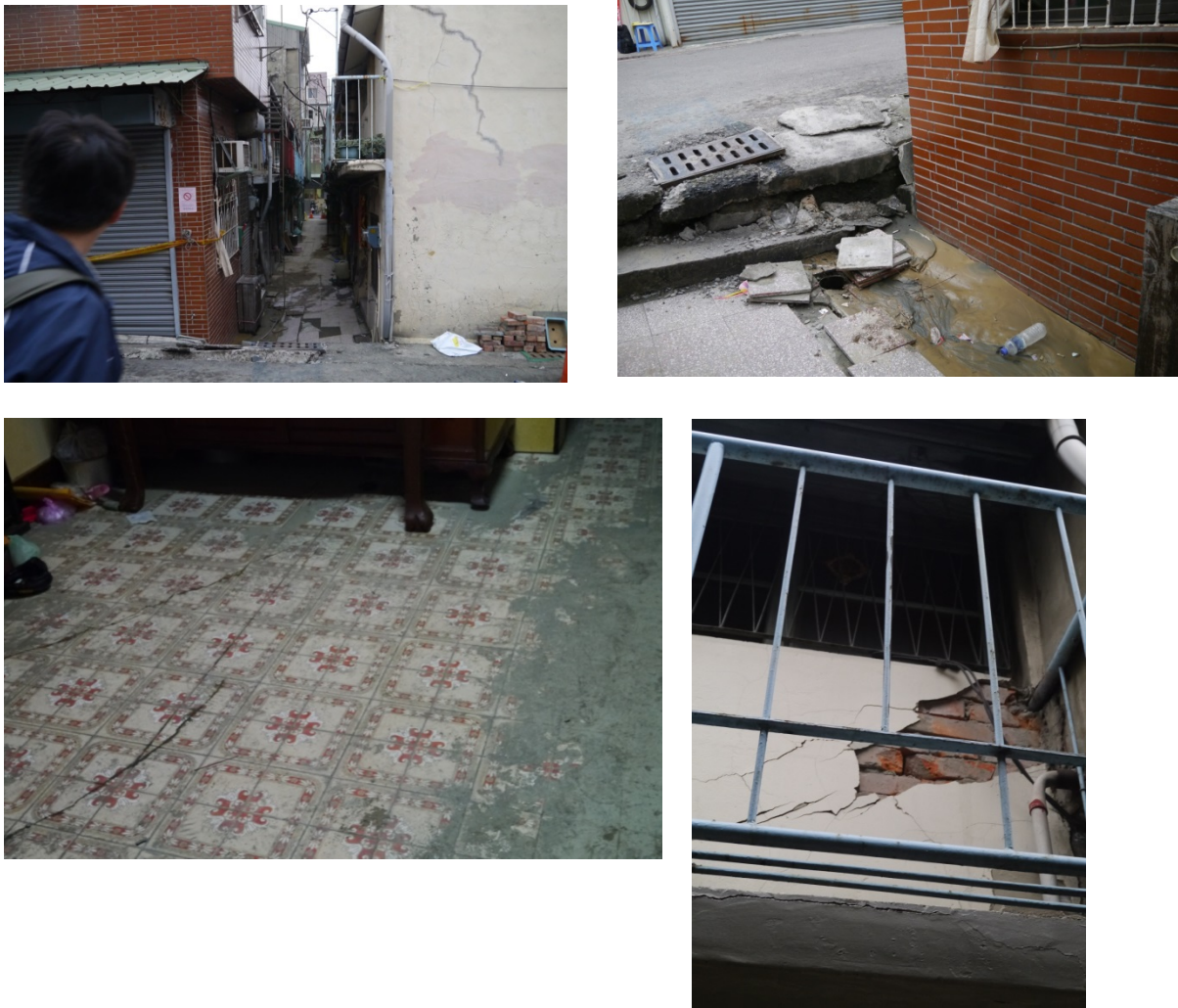
Figure 7-16: Damage features at the Wenhe site ( 23°00'12.7"N 120°11'30.5"E ).
