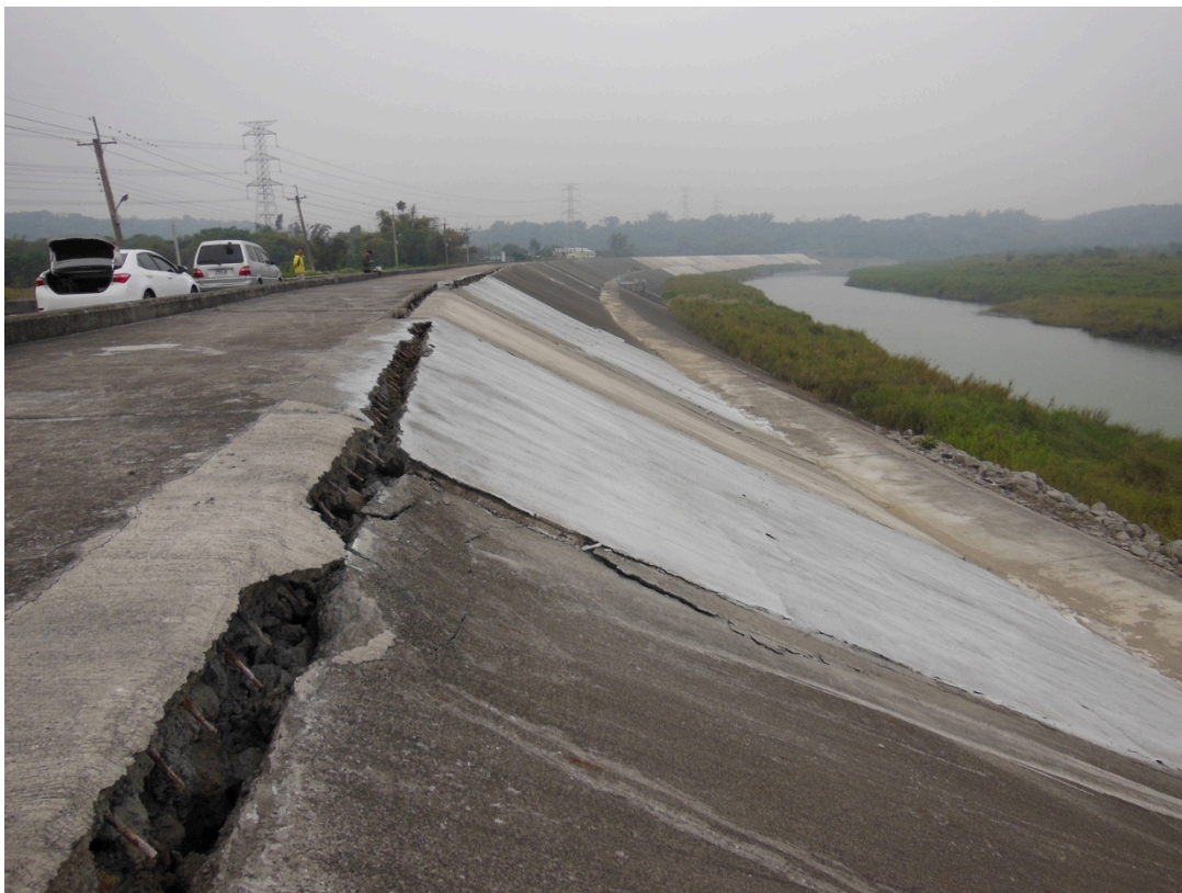
Figure 8-31: Distress of Concrete Slab Bank Protection (23.121176°,120.379569°).
