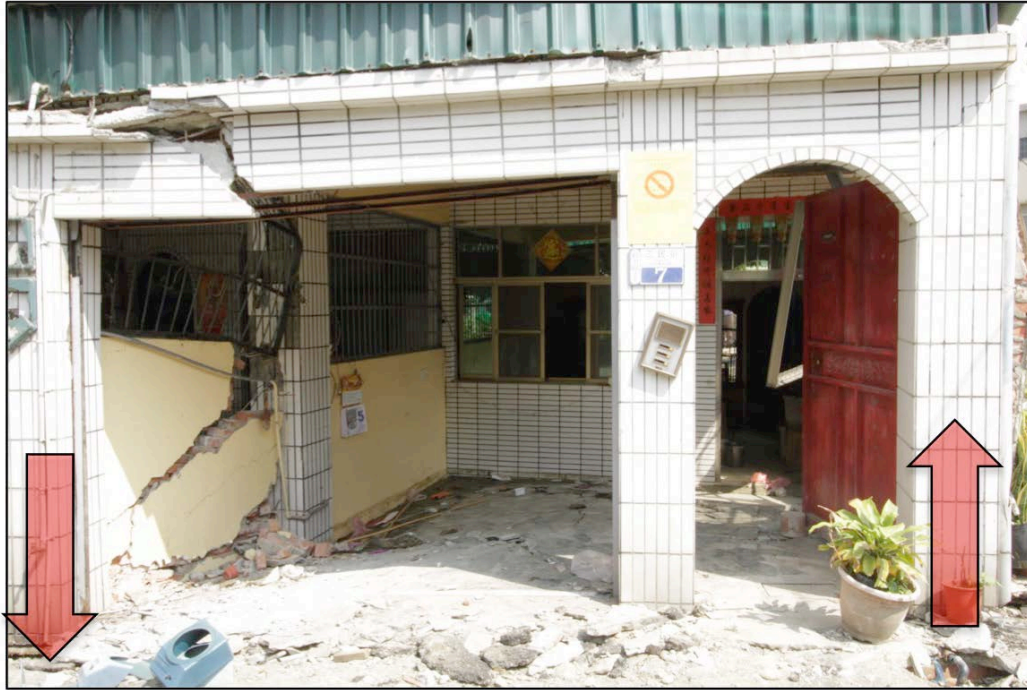
Figure 10-3: Development of a structural hinge within a beam supporting a carport at the Xinshi site due to column heave (right side) and settlement (left side) of structure. This carport was demolished, while the interior of the building supported on grade beams connecting spread footings performed well ( 23.08096 , 120.30258 ).
