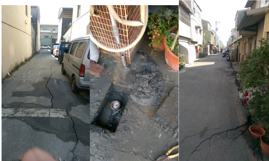
Figure 7-4: Typical failure patterns of pavement crack, breakage of water pipe, and foundation settlement in the Annan district.
