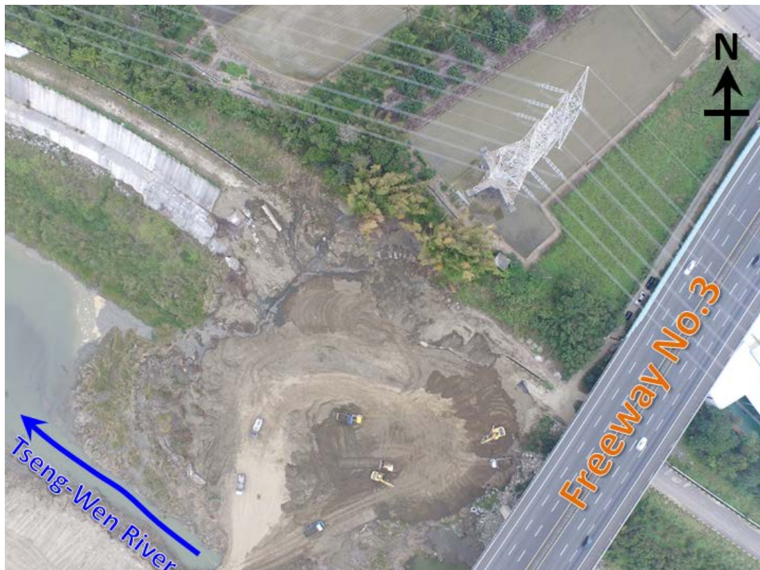
Figure 8-3: Aerial View of Failure No.1. (Photo provided by W.-K. Huang) ( 23^{\circ} 9'12.40'' , 120^{\circ}20'37.68'' ). Note the construction repair operation underway.
