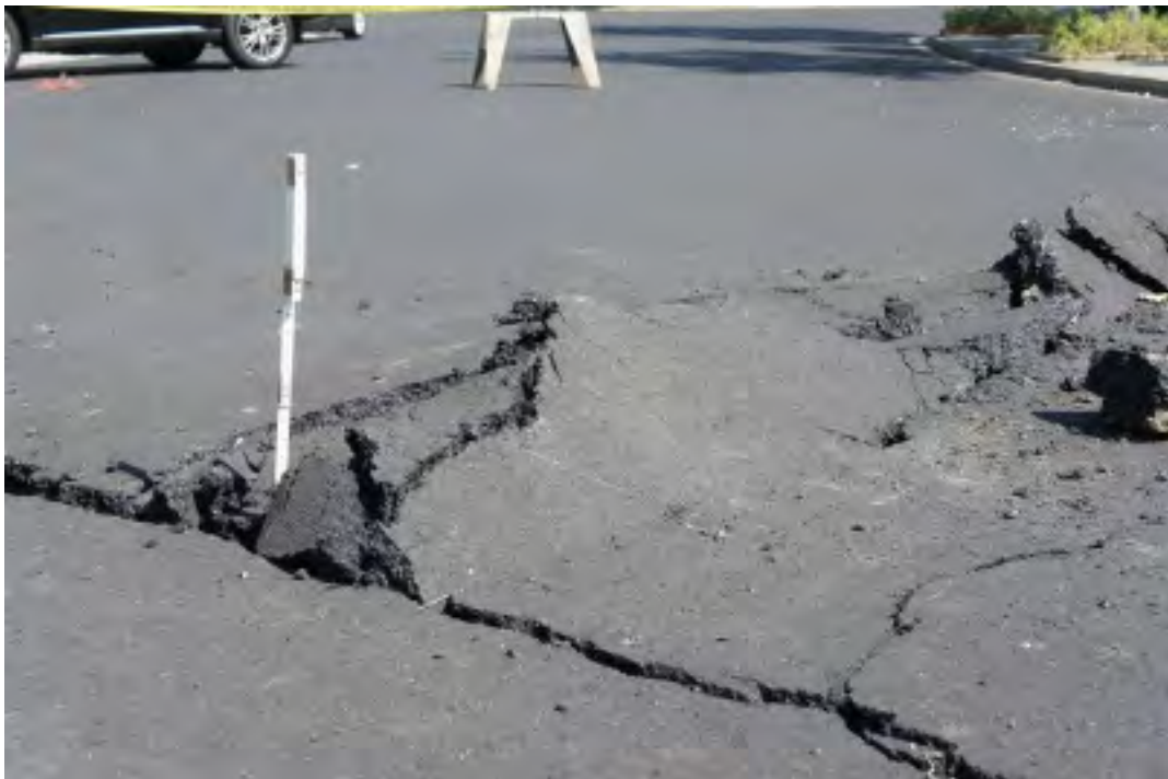
Figure C-P3-3: [NSF-GEER; N 38.3046 W 122.3428; 08/25/14 15:28]
