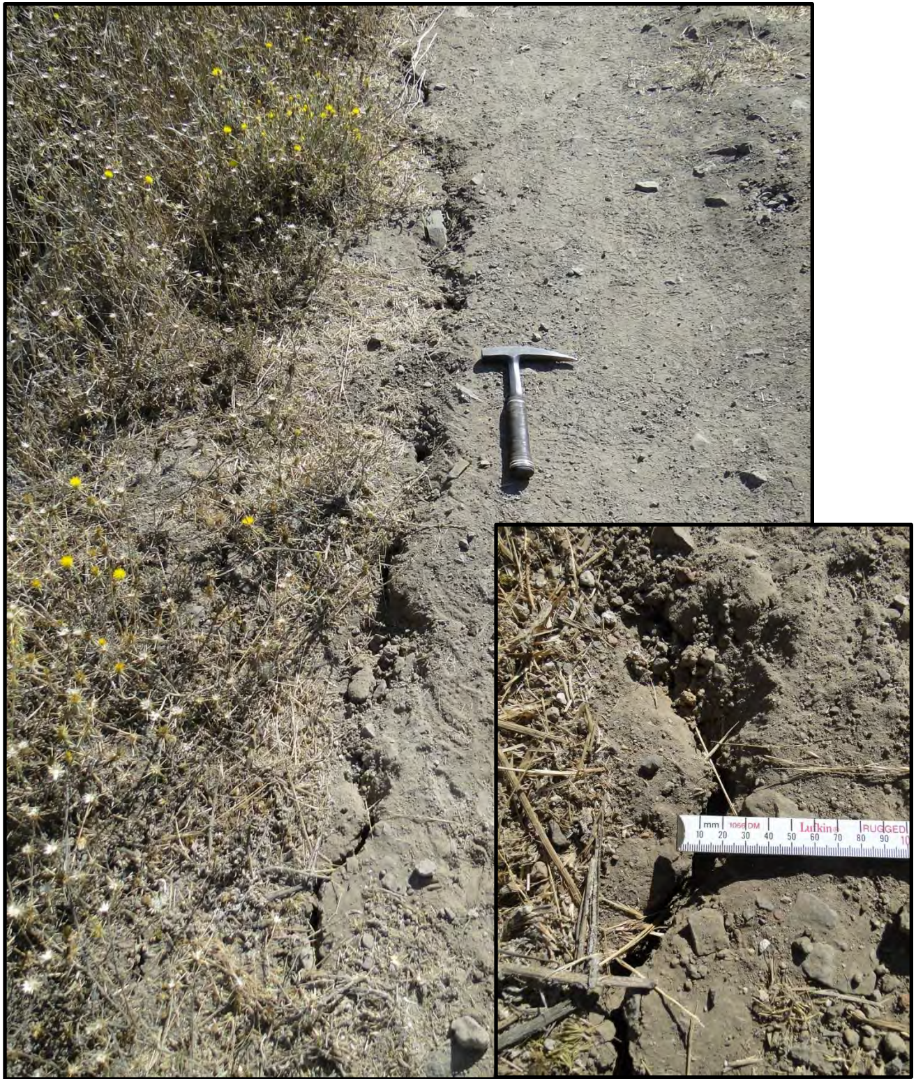
Figure F-4: Photograph of cracking on the upstream edge of the crest of Lake Marie Dam looking southeast [NSF-GEER; Napa, CA; N38.260 W 122.230; Harder, L. F.; 09/01/14]
