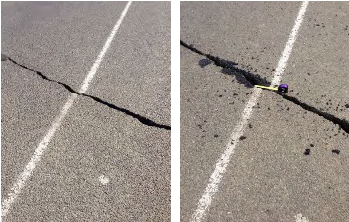
Figure 3-14. Offset painted stripe on the side of Highway 12 is shown by these two photos taken approximately 24 hours apart on Aug. 24, 2014 and Aug. 25, 2014. The fracture opening is narrower and the paint stripe offset by a lesser amount on the day of the earthquake. During the ensuing day, the fracture grew and the offset of the paint stripe increased. The increase of offset along the surface rupture of an earthquake has been observed in previous earthquakes. What is different in the case of the South Napa earthquake is that in this case, afterslip in the first day after the earthquake was rapid, but then afterslip appeared to stop in the following days. In the southern half of the surface rupture zone, the initial evidence for rapid afterslip was pronounced, whereas in the northern portion there was little to no afterslip [NSF-GEER; GPS: 38.2559°, -122.3272°; 08/24/2014 and 08/24/2014.
