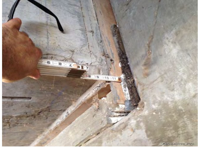
Figure E.38: of the deck in 3 rd St. Bridge East abutment [NSF-GEER; N 38.2981 W -122.284; 08/24/14 14:44]
