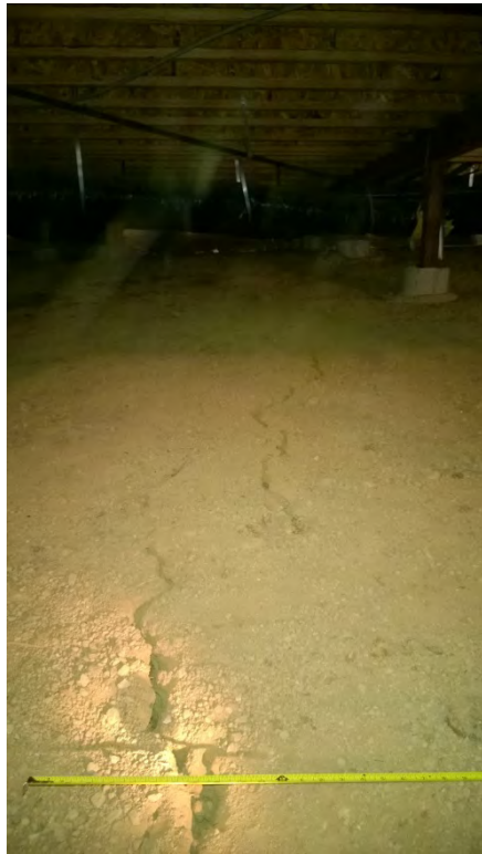
Figure C-H04-5: Soil fissure in basement. [NSF-GEER; N 38.3128 W 122.3431; 08/28/14, 12:08]
