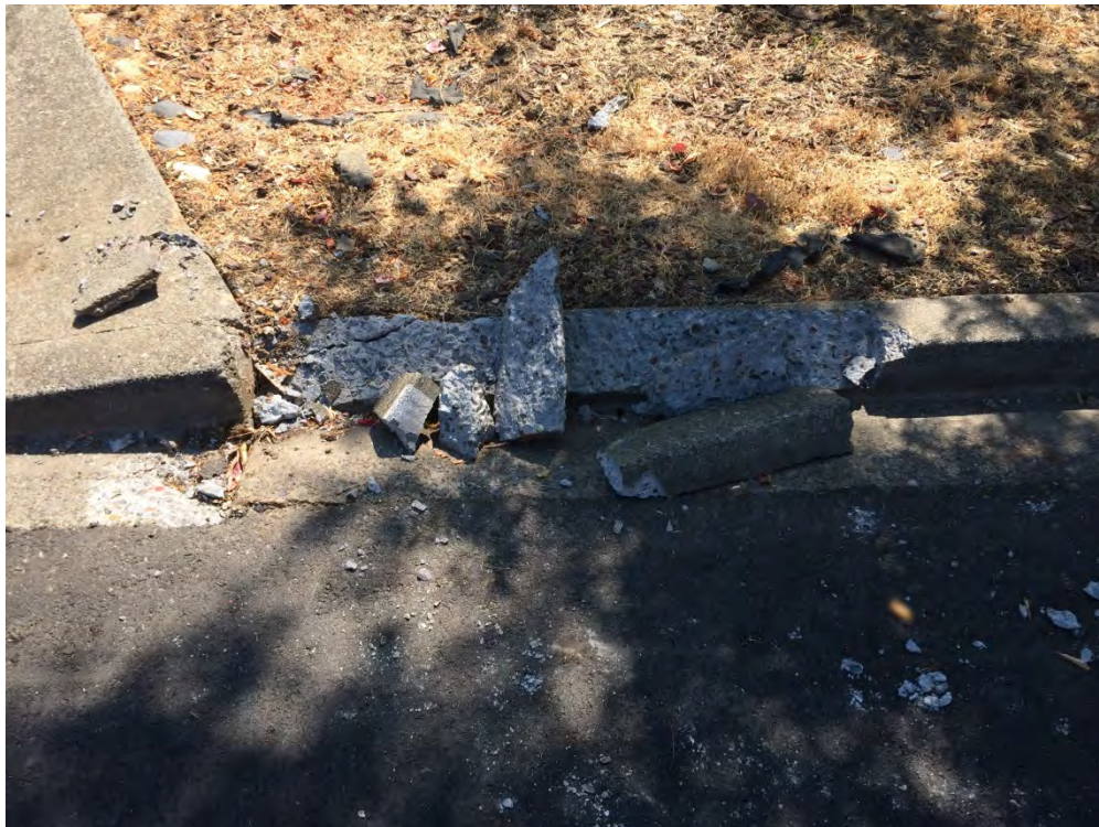
Figure D-16: Crushed curb perpendicular to fault trace [NSF-GEER; N 38.3035 W 122.3411; 8/25/2014 14:47]
