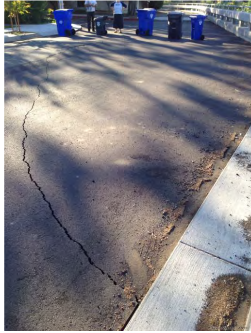
Figure E.42: Crack in pavement behind the retaining wall in the Pedestrian Bridge [NSF-GEER; N 38.3003 W -122.2881; 08/24/14 17:58]
