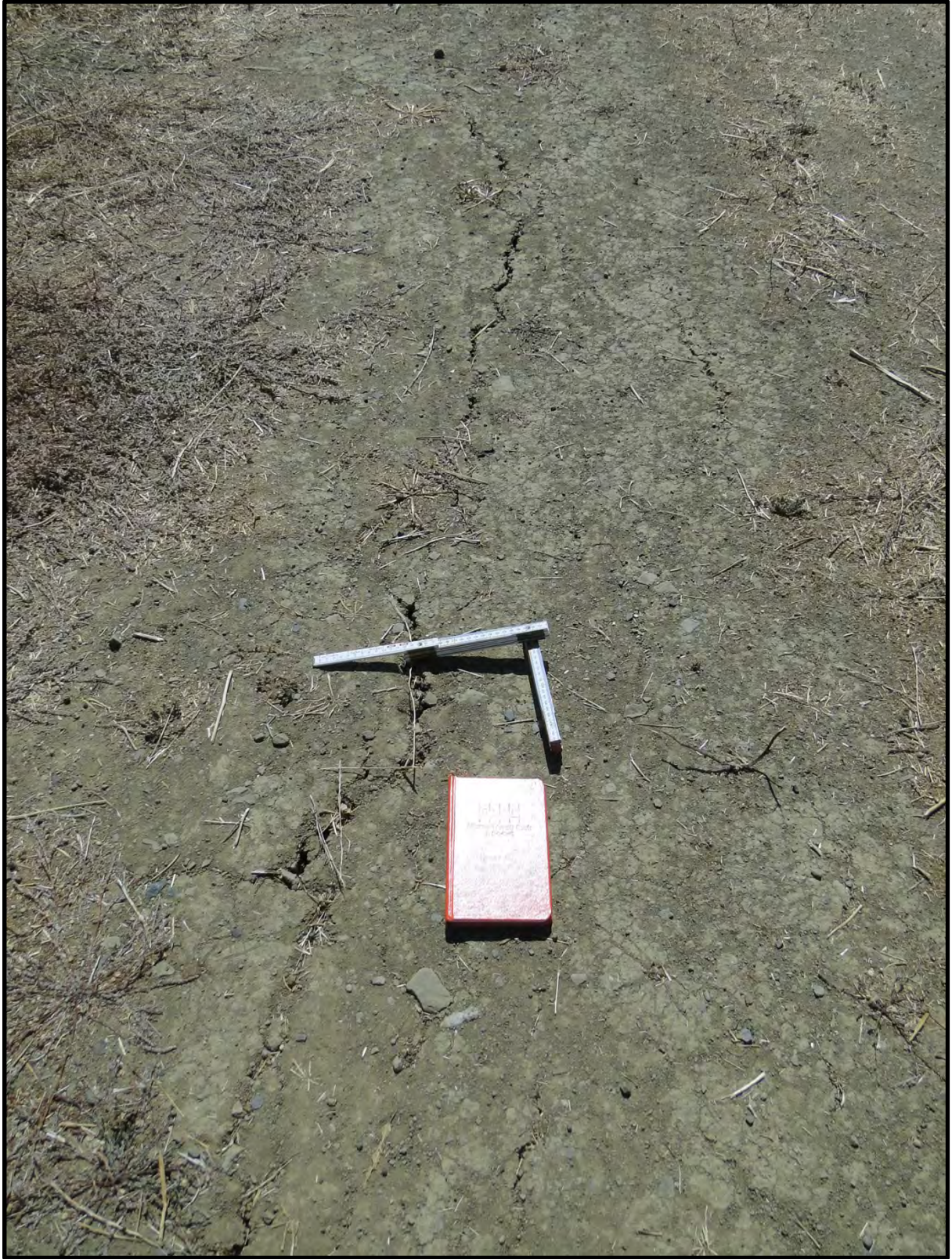
Figure 7-7: Close-up photograph of minor longitudinal cracking on the crest of Lake Chabot Dam looking southeast [NSF-GEER; Napa, CA; N38.141 W 122.241; Harder, L. F.; 08/27/14]
