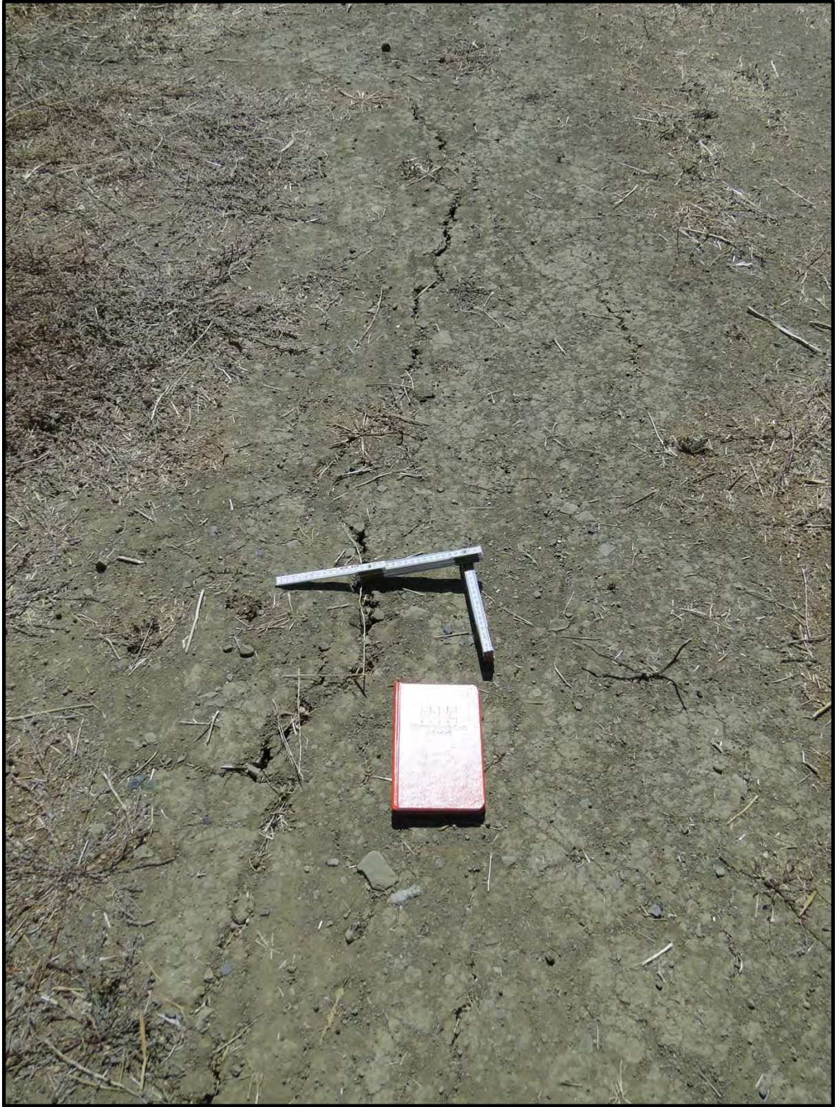
Figure F-7: Close-up photograph of minor longitudinal cracking on the crest of Lake Chabot Dam looking southeast [NSF-GEER; Napa, CA; N38.141 W 122.241; Harder, L. F.; 08/27/14]
