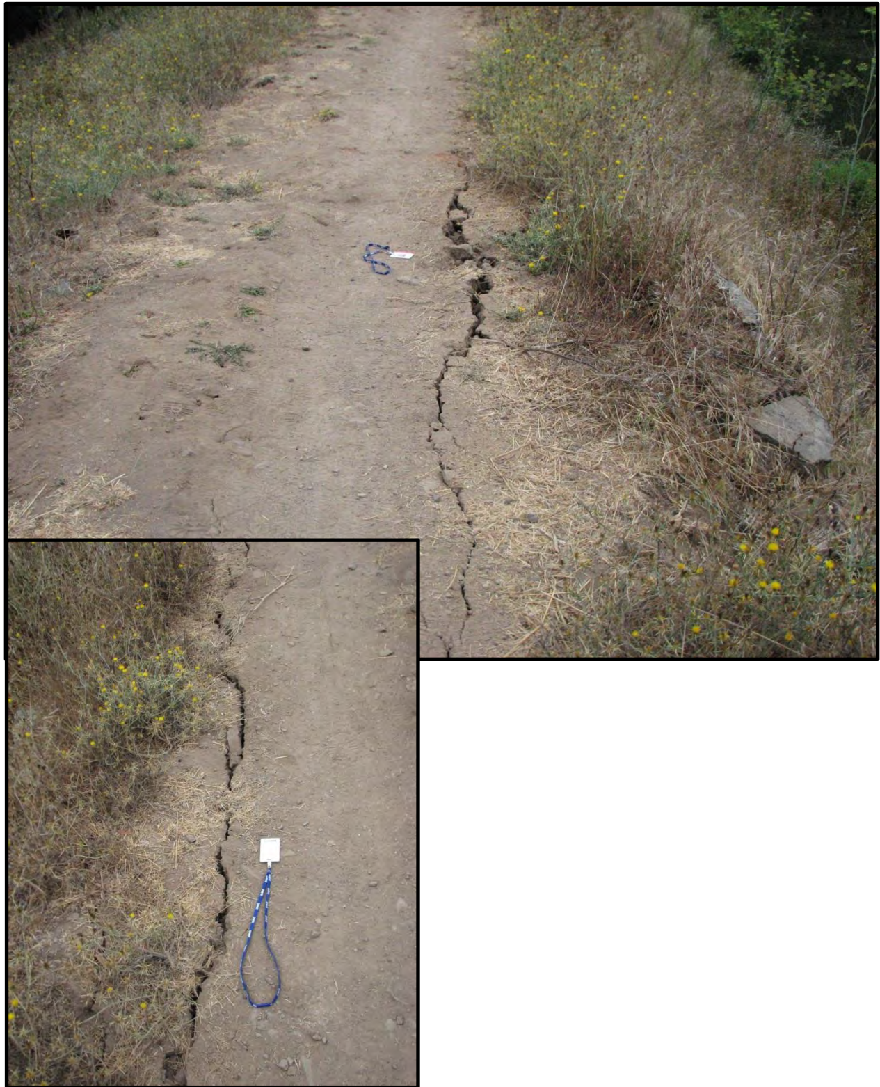
Figure F-3: Photographs of longitudinal cracking on the upstream edge of the crest of Lake Marie Dam [Napa, CA; N38.260 W 122.230; from DSOD files; 08/24/14]
