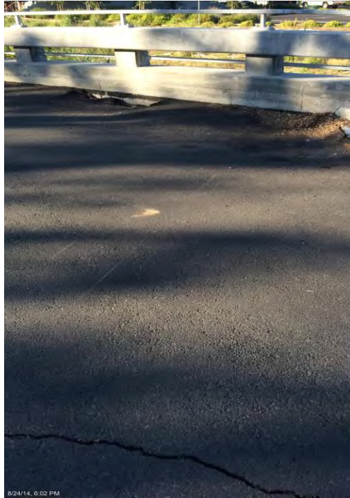
Figure 6.12: Settlement of backfill near the retaining wall in the pedestrian bridge [NSF-GEER; N 38.3003 W -122.2881; 08/24/14 17:58]
