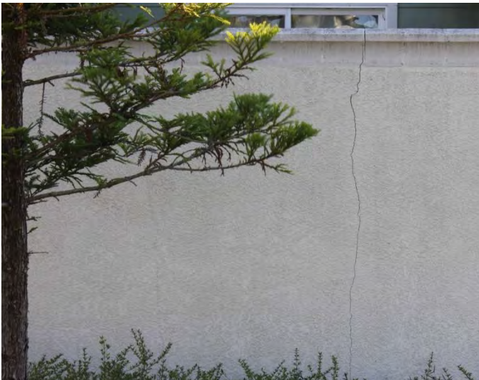
Figure E.20: Soundwall, minor crack [NSF-GEER; GPS N38.096 W122.276; 08/24/14; 17:31]
