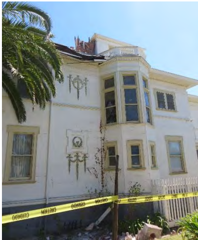
Figure E.8: Brick chimney damage [NSF-GEER; GPS N38.100 W122.274; 08/24/14; 14:13]
