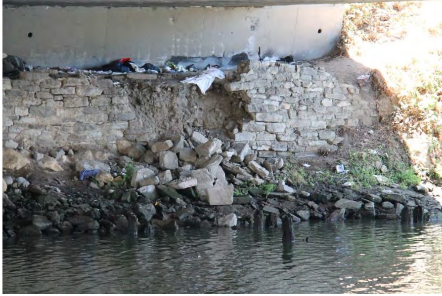
Figure 6.6: Failure of masonry retaining wall below the south abutment of Soscol Bridge [NSF-GEER; N 38.2997 W -122.2834; 08/24/14 13:09]
