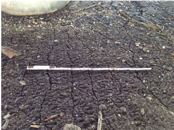
Figure E.39: Ground cracking due to liquefaction in Napa River point bar below 3 rd St. Bridge, between the two columns of the eastern pier. [NSF-GEER; N 38.2980 W -122.2840; 08/24/14 14:44]
