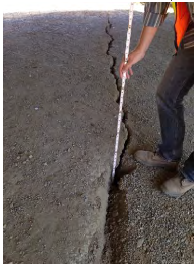
Figure E.31: Railroad Bridge. Crack observed in the interface between the North abutment foundation and the soil. [NSF-GEER; N 38.3002 W -122.282; 08/25/14 12:41]
