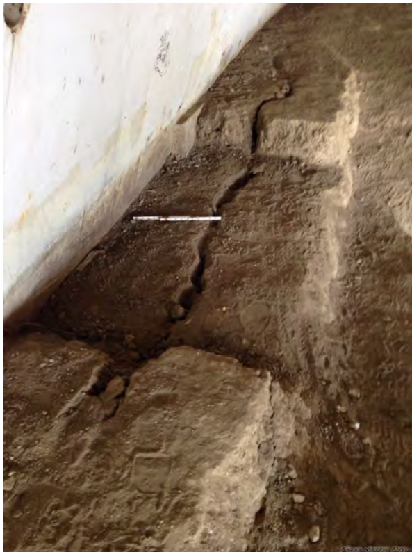
Figure E.35: Crack parallel to the River in North abutment of Soscol Bridge [NSF-GEER; N 38.2997 W -122.283; 08/24/14 13:09]
