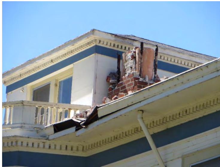
Figure 6.3: Brick chimney damage; [NSF-GEER; Mare Island, Vallejo, CA; GPS N38.099 W122.273; 08/24/14; 14:19]
