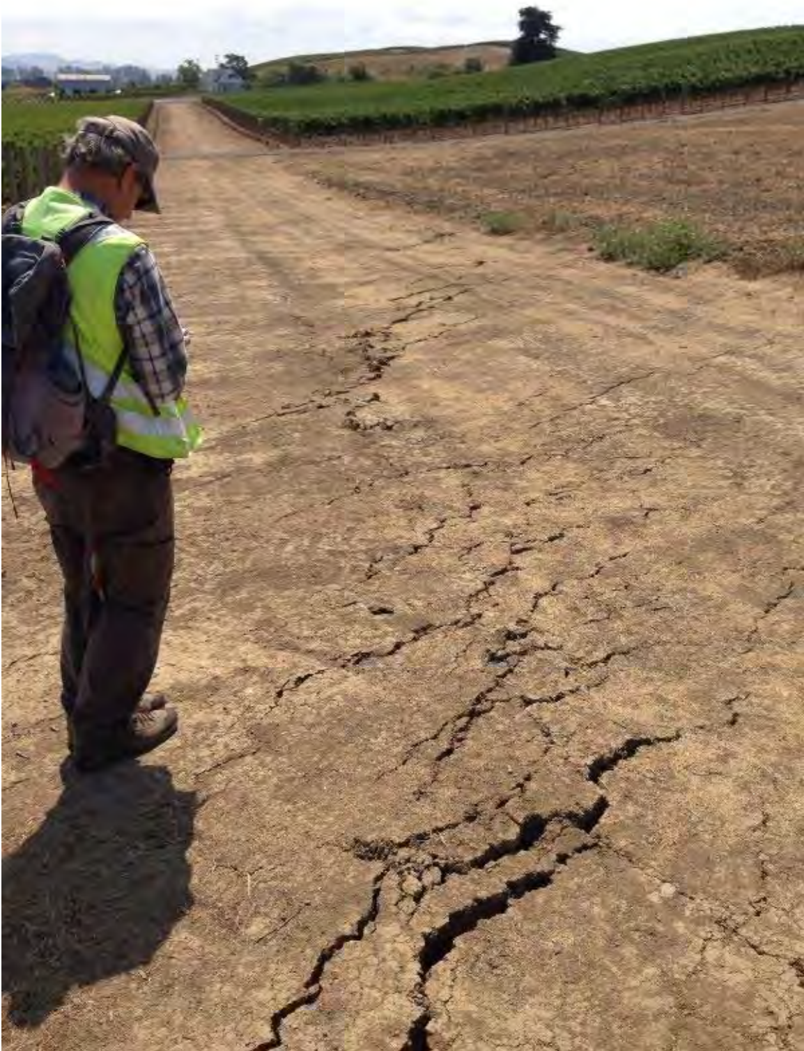
Figure 7. Surface fault rupture at central part of Clos du Val Vineyard (5.9 km NW of epicenter), showing left-stepping pattern of transensional cracking within compacted dirt farm road. View to south-southeast. [NSF-GEER; GPS N38.271 W122.335; 08/25/14: 12:10 pm]
