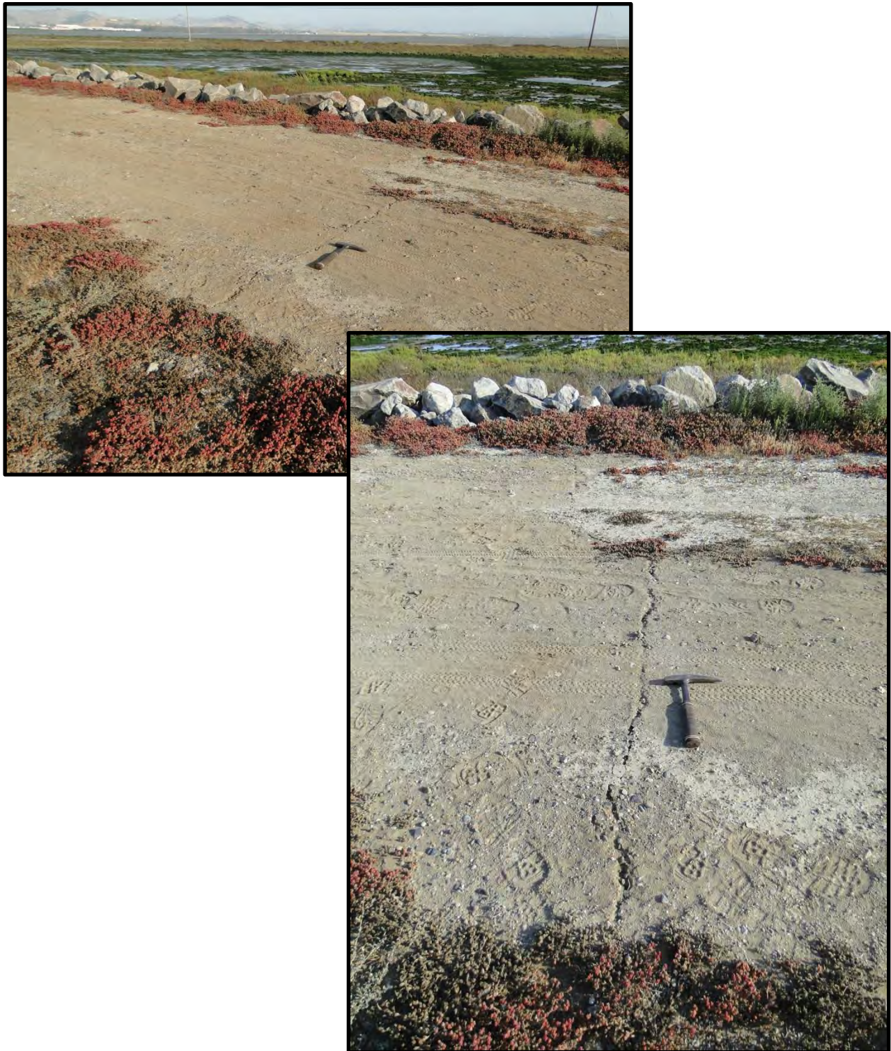
Figure F-24: Photographs of transverse cracking on crown of salt pond retaining dike on western edge of Green Island south of the epicenter [NSF-GEER; Napa, CA; N38.201 W 122.302; Harder, L. F.; 09/04/14]
