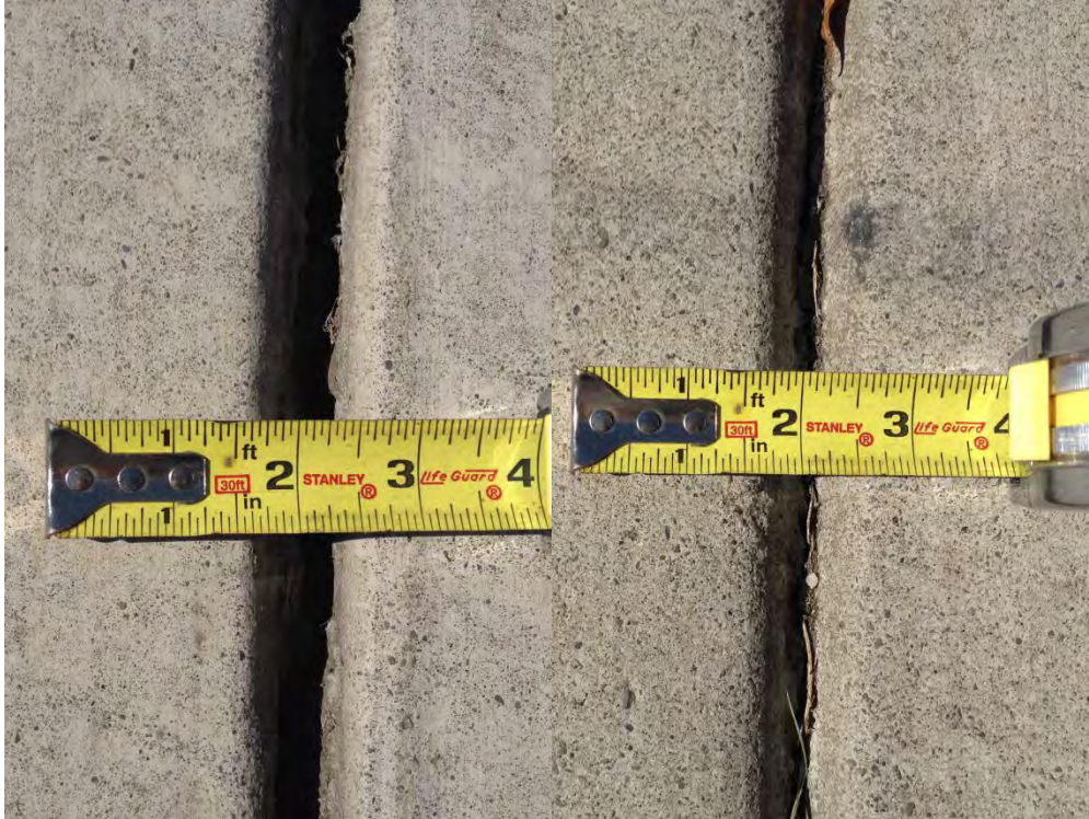
Figure D-9: Typical extension cracks in thermal joints of sidewalk pavement parallel to fault; ~13mm gap (left), ~7mm gap (right) [NSF-GEER; N 38.3067 W 122.3464; 8/28/2014 15:18]
