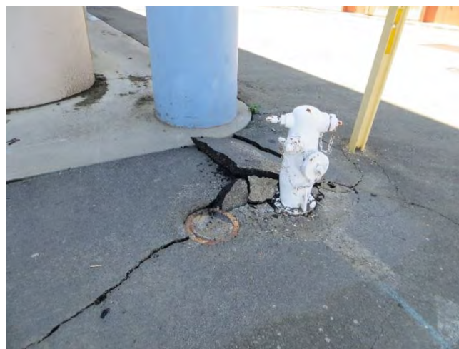
Figure 6.5: Pavement damage at hydrant; [NSF-GEER; Mare Island, Vallejo, CA; GPS N38.098 W122.269; 08/24/14; 14:37]
