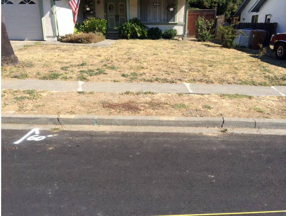
Figure D-19: Buckled curb adjacent to pavement perpendicular to fault trace; visible cracking in soil aligns with cracks in curb [NSF-GEER; N 38.3027 W 122.3407; 8/28/2014 10:25]
