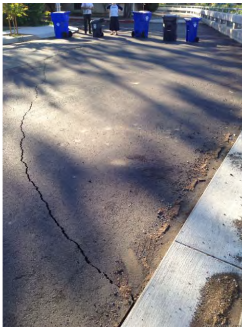
Figure 6.11: Crack in pavement behind the retaining wall in the pedestrian bridge [NSF-GEER; N 38.3003 W -122.2881; 08/24/14 17:58]
