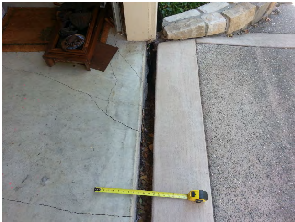
Figure C-H02-3: West looking view of driveway/garage slab separation and crack extending through 6 inch reinforced slab. [NSF-GEER; N 38.3133 W 122.3431; 08/28/14 12:44]
