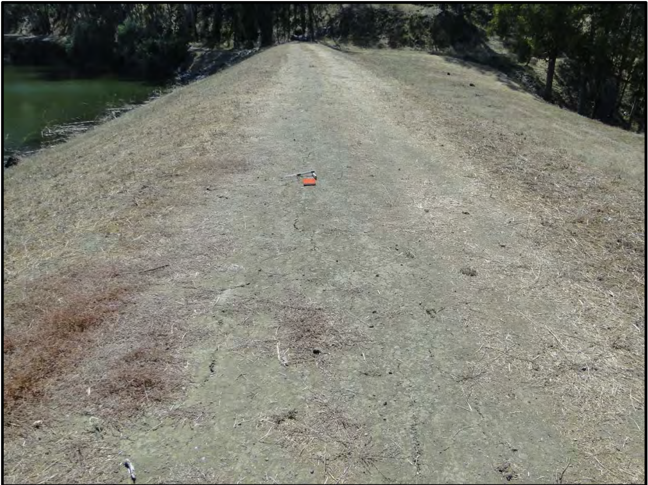
Figure 7-6: Photograph of minor longitudinal cracking on the crest of Lake Chabot Dam looking southeast [NSF-GEER; Napa, CA; N38.141 W 122.241; Harder, L. F.; 08/27/14]
