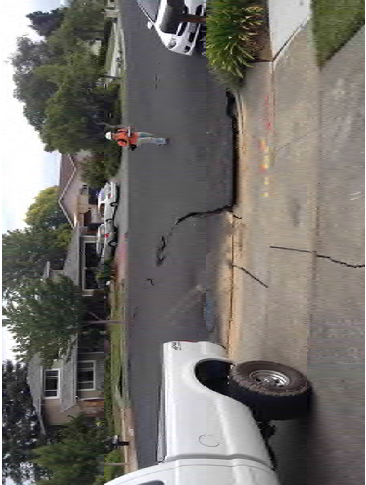
Figure C-P1-2: General view of fracturing [NSF-GEER; N 38.3016 W 122.3441; 08/25/14 10:24]
