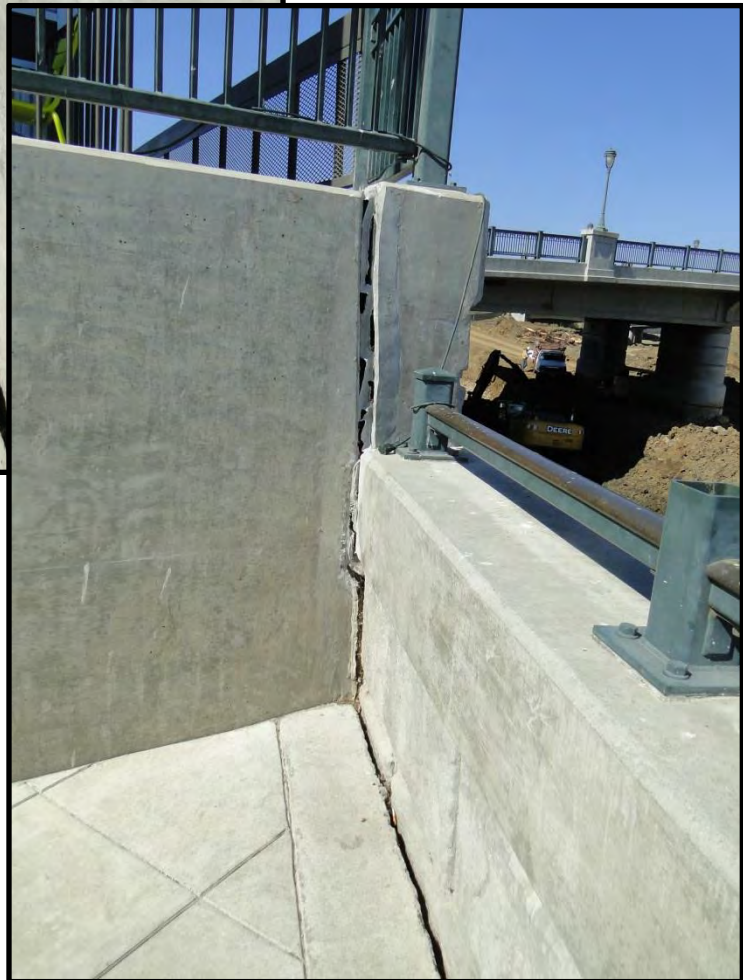
Figure F-19: Separation of concrete slab and retaining wall from Napa River floodwall along right bank of Napa River looking upstream from Third Street Bridge [NSF-GEER; Napa, CA; N38.299 W 122.285; Harder, L. F.; 09/04/14]
