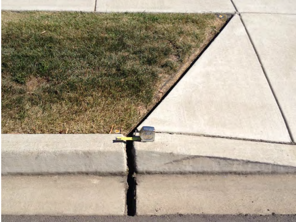
Figure D-17: Extension crack in curb parallel to fault trace [NSF-GEER; N 38.3066 W 122.3465; 8/28/2014 15:08]
