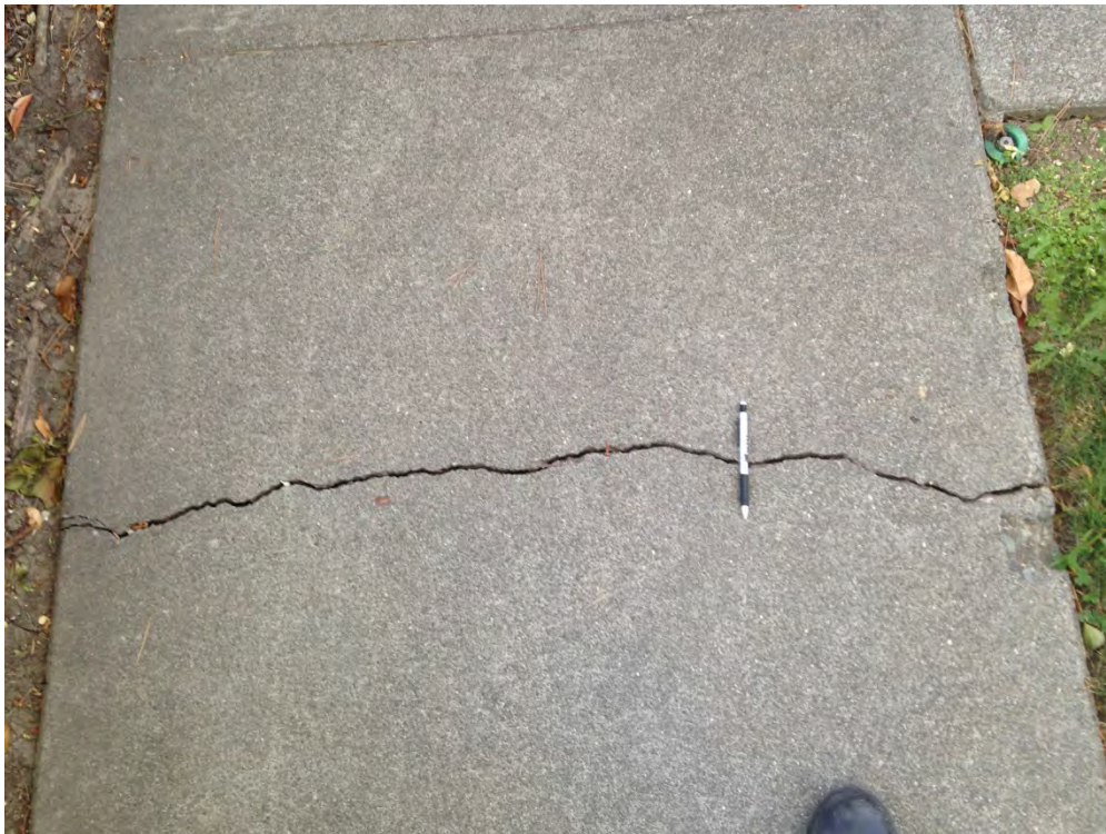
Figure D-10: Extension crack in sidewalk pavement parallel to fault; ~3mm gap [NSF-GEER; N 38.3055 W 122.3454; 8/26/2014 18:30]
