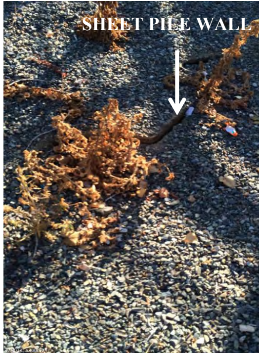
Figure 6.10: Crack along sheet pile wall behind the retaining wall in the Pedestrian Bridge [NSF-GEER; N 38.3003 W -122.2881; 08/24/14 17:58]
