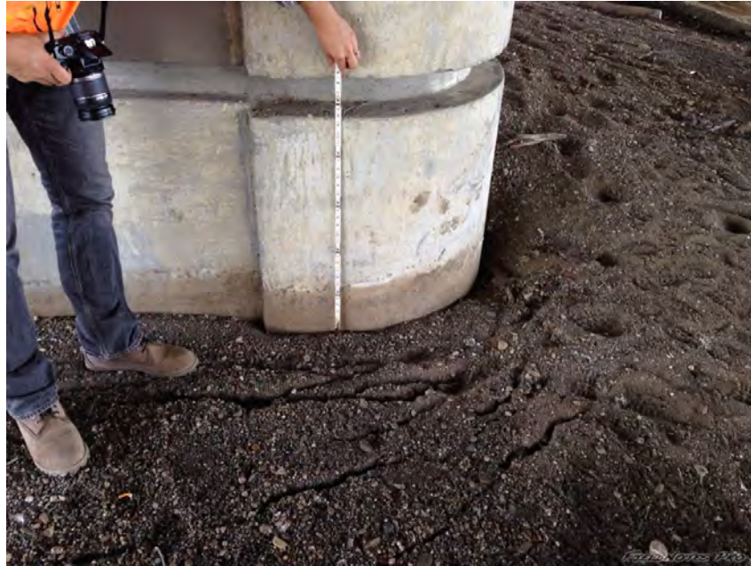
Figure 6.9: Ground cracking and settlement due to liquefaction in Napa River point bar below 3 rd St. Bridge [NSF-GEER; N 38.2980 W -122.2840; 08/24/14 14:44]
