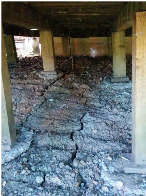
Figure C-H01-3: South looking view of ground rupture under deck coming from under severely damaged house on pier foundations. [NSF-GEER; N 38.3135 W 122.3431; 08/28/14 17:15]
