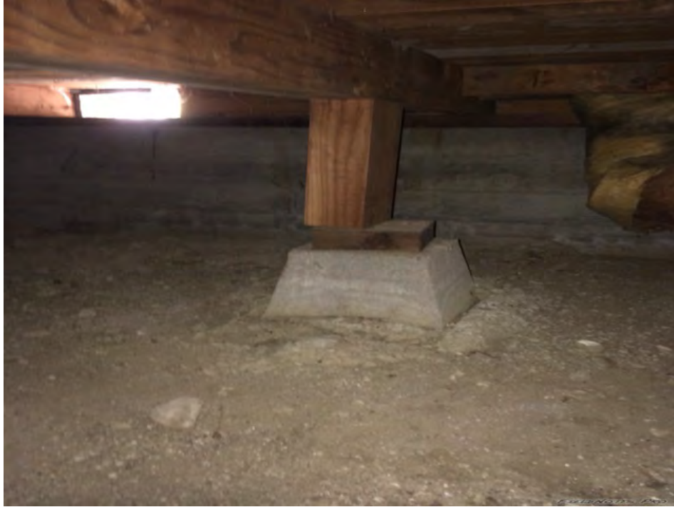
Figure C-H15-2: Shifted wooden column. The column was shifted towards west. [NSF-GEER; N 38.3061 W 122.3427; 08/29/14 10:02]
