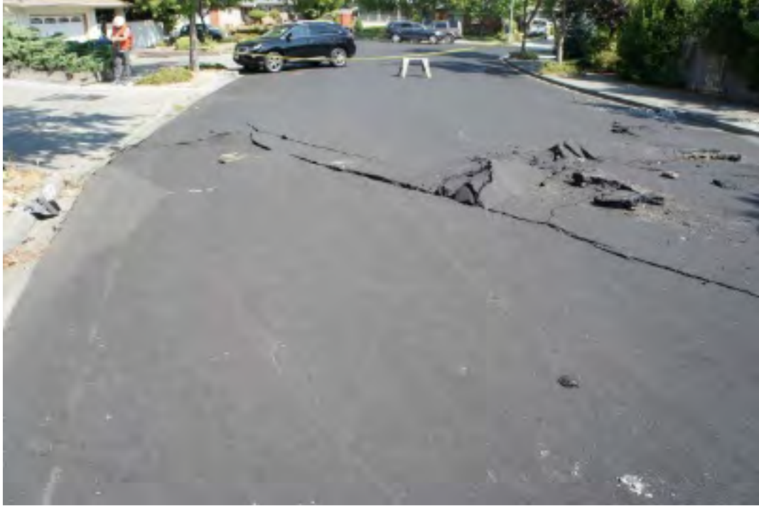
Figure C-P3-2: [NSF-GEER; N 38.3046 W 122.3428; 08/25/14 15:26]
