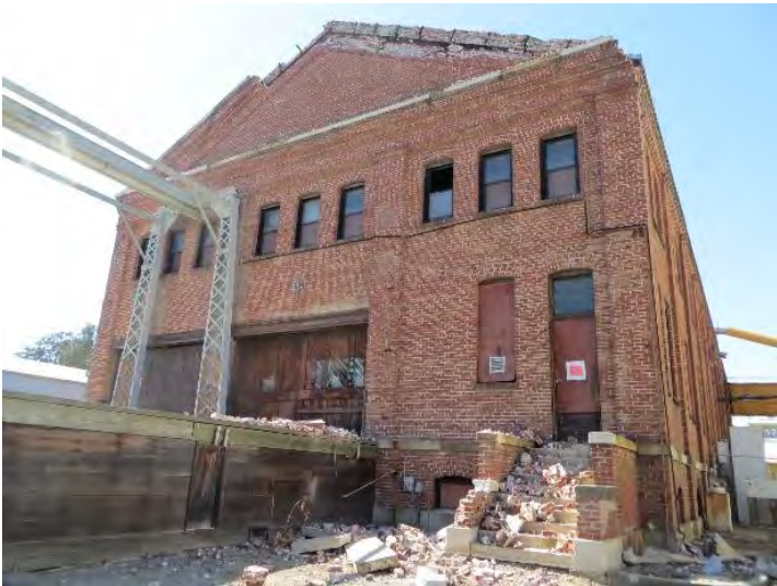
Figure E.12: Brick facade damage [NSF-GEER; GPS N38.095 W122.268; 08/24/14; 15:38]
