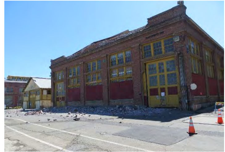
Figure E.11: Brick facade damage [NSF-GEER; GPS N38.097 W122.268; 08/24/14; 14:43]
