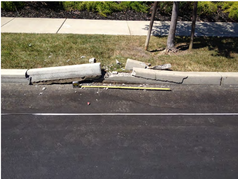
Figure D-18: Buckled curb parallel to fault trace [NSF-GEER; N 38.3073 W 122.3443; 8/28/2014 13:41]
