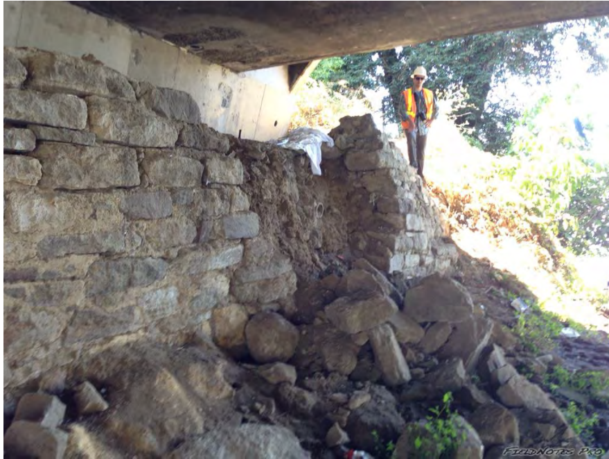
Figure E.34: Failure of the stone retaining wall in South abutment of Soscol Bridge [NSF-GEER; N 38.2994 W -122.282; 08/24/14 13:44]
