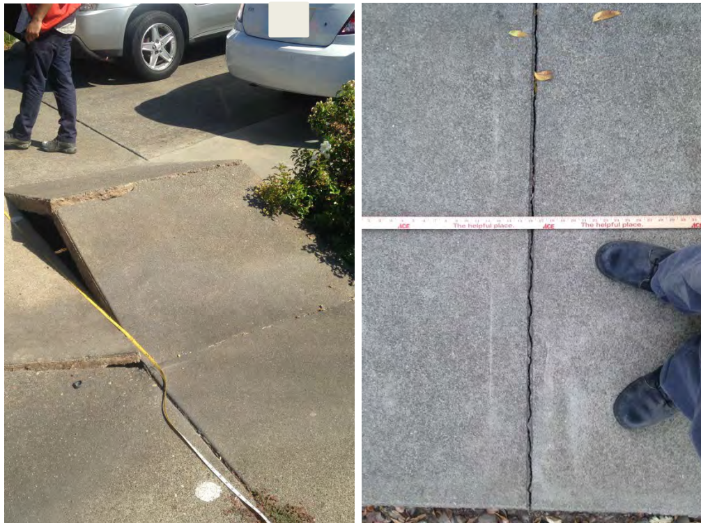
Figure 5.2: Typical buckled compression zone (left) and extension crack (right) [NSF-GEER; N 38.3037 W 122.3433; 8/26/2014 15:41 (left); N 38.3055 W 122.3455; 8/26/2014 18:34 (right)]
