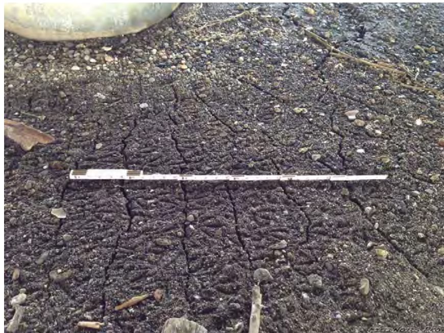
Figure 6.8: Ground cracking due to liquefaction in Napa River point bar below 3 rd St. Bridge, between the two columns of the eastern pier. [NSF-GEER; N 38.2980 W -122.2840; 08/24/14 14:44]
