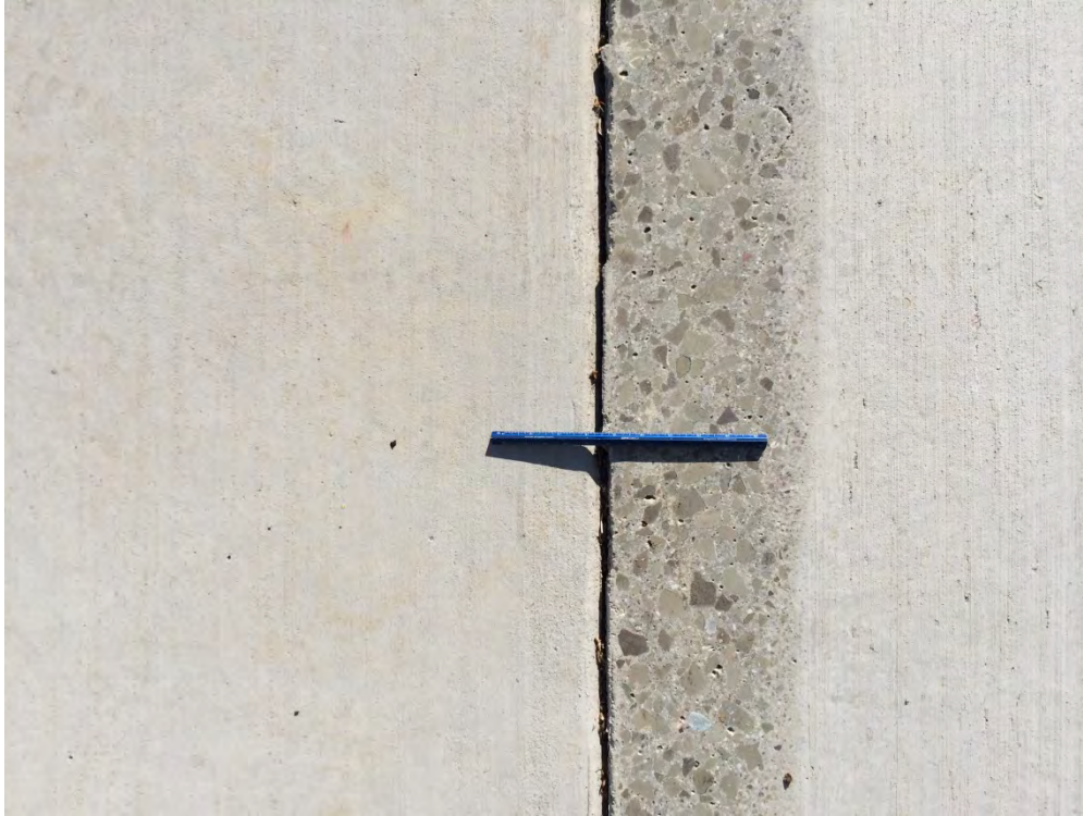
Figure D-11: Example of extension crack not considered due to shaved concrete [[NSF-GEER; N 38.3021 W 122.3430; 8/28/2014 09:17]
