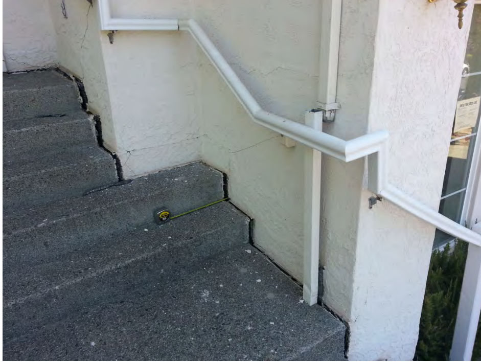
Figure C-H03-2: SE looking view of stair case/structure separation and cracks. [NSF-GEER; N 38.3131 W 122.3431; 08/28/14 11:52]
