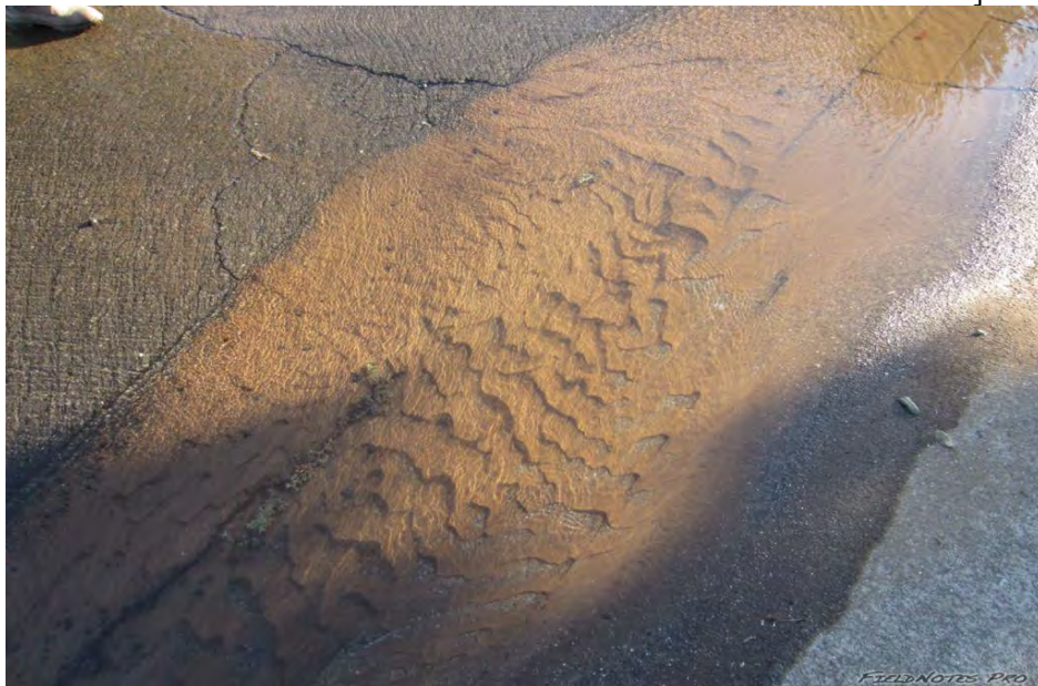
Figure E.28: Water break at Arroyo Dr. (Downtown Napa). Soil below asphalt ejected by water. [NSF-GEER; N 38.3008 W -122.289; 08/25/14 18:34]
