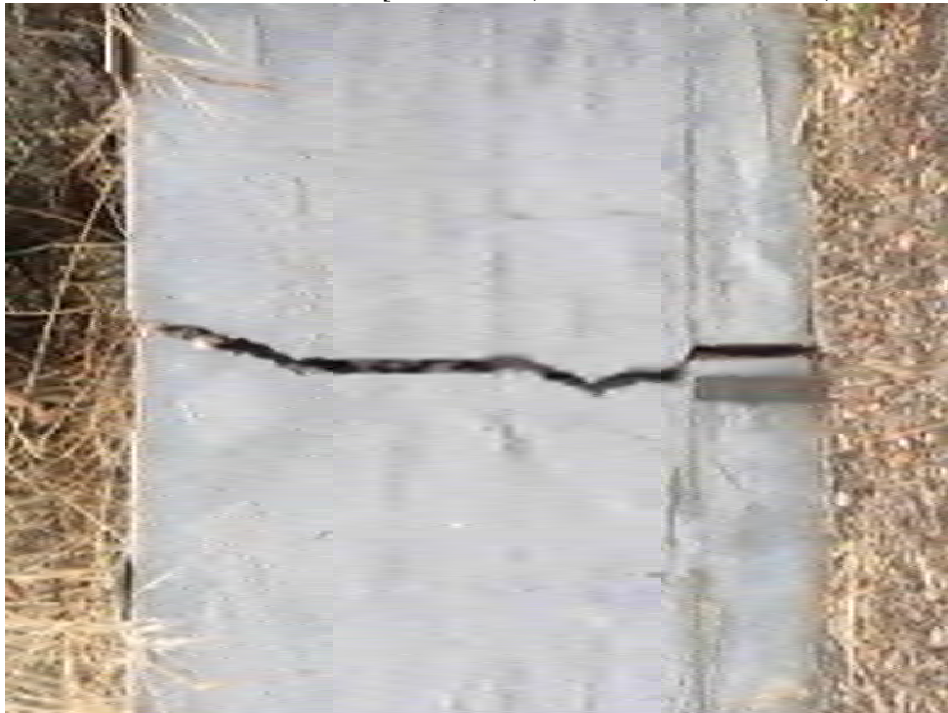
Figure C-H35-4: Retaining wall crack [NSF-GEER; N 38.3015 W 122.3440; 08/25/14 10:58]
