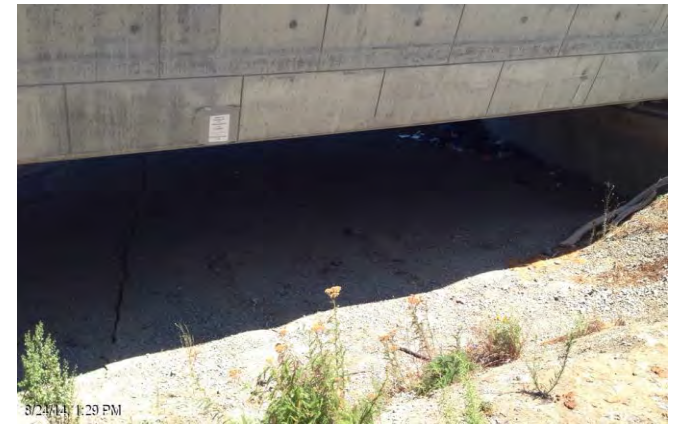
Figure E.33: Railroad Bridge. Crack observed in the interface between the South abutment foundation and the soil. [NSF-GEER; N 38.2995 W -122.2821; 08/25/14 13:28]
