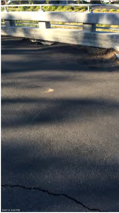
Figure E.41: Settlement of backfill near the retaining wall in the Pedestrian Bridge [NSF-GEER; N 38.3003 W -122.2881; 08/24/14 17:58]
