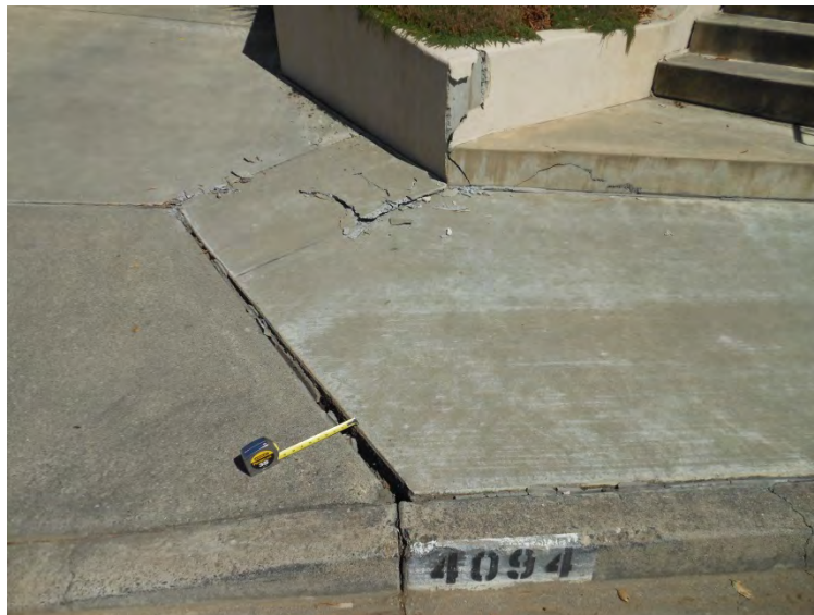
Figure C-H07-3: Crack extending along stair case and joint. [NSF-GEER; N 38.3122 W 122.3432; 08/28/14]
