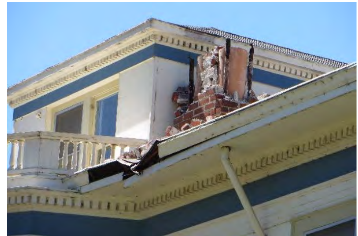
Figure E.9: Brick chimney damage [NSF-GEER; GPS N38.099 W122.273; 08/24/14; 14:19]
