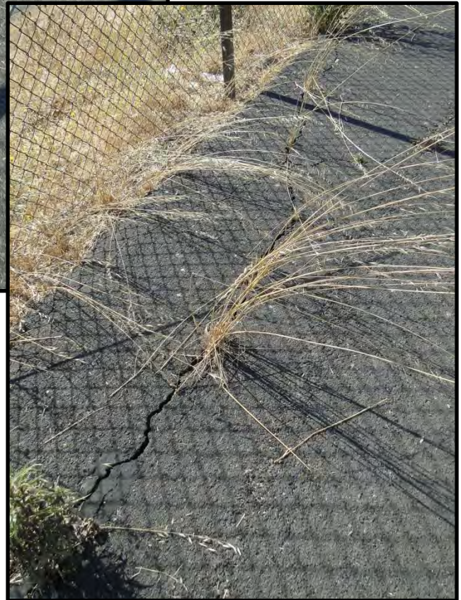
Figure F-9: Photographs of pre-existing longitudinal cracks on the crest of the maximum section of Summit Reservoir Dam [NSF-GEER; Napa, CA; N38.153 W 122.225; Harder, L. F.; 08/27/14]
