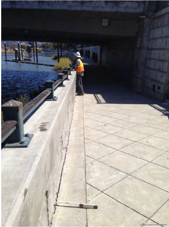
Figure E.37: Crack parallel to the River in West abutment of 3 rd St. Bridge [NSF-GEER; N 38.2980 W -122.2840; 08/24/14 14:44]
