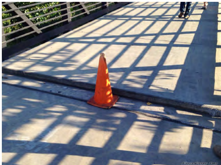
Figure E.44: Step between bridge's deck and access ramp in North abutment. [NSF-GEER; N 38.3003 W -122.2881; 08/24/14 17:58]
