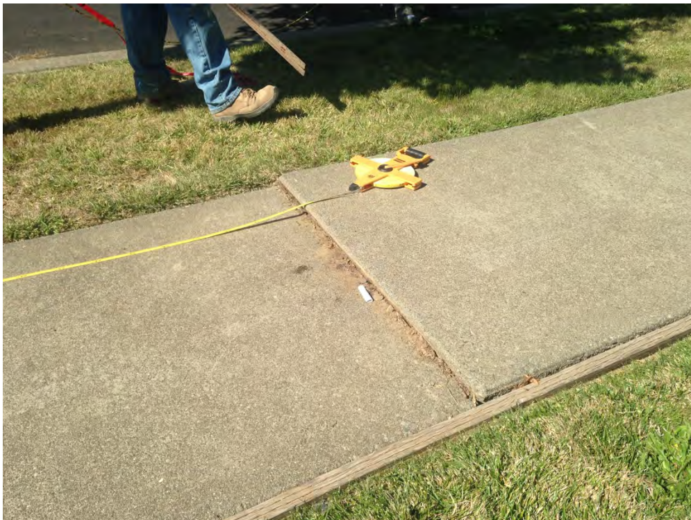
Figure D-8: Slight uplift in compressed zone of pavement perpendicular and near fault [NSF-GEER; N 38.3037 W 122.3430; 8/26/2014 15:48]
