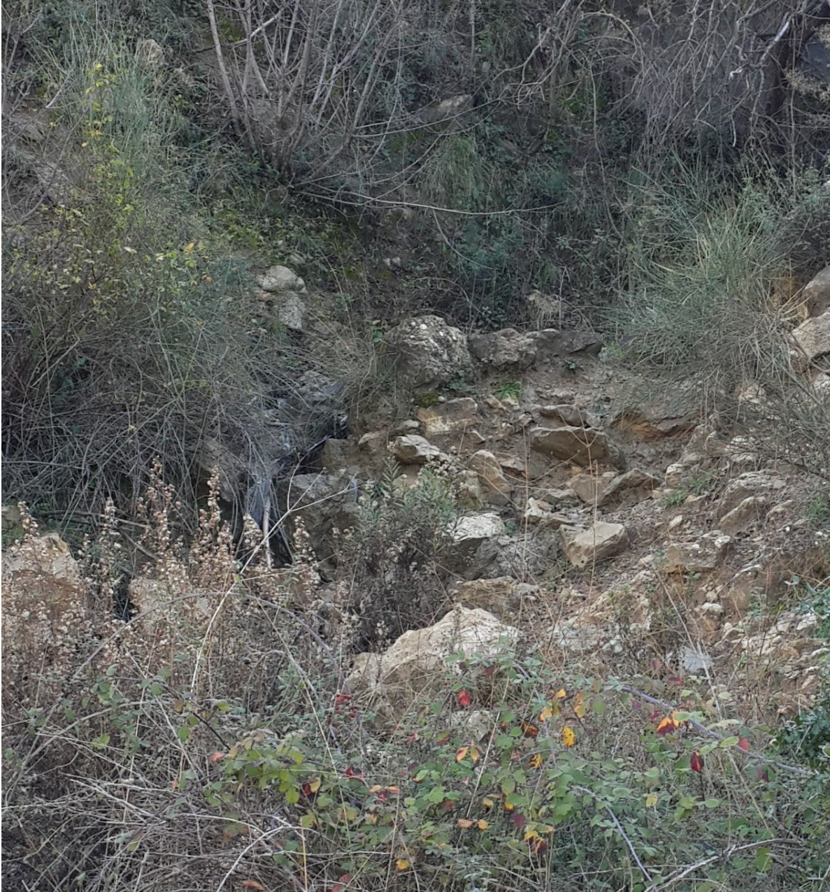
Figure A.5: Surface water runoff at the base of the cliff
