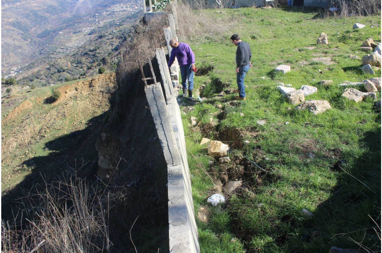
Figure A.6: Damage to backyard fence after 2015 landslide
