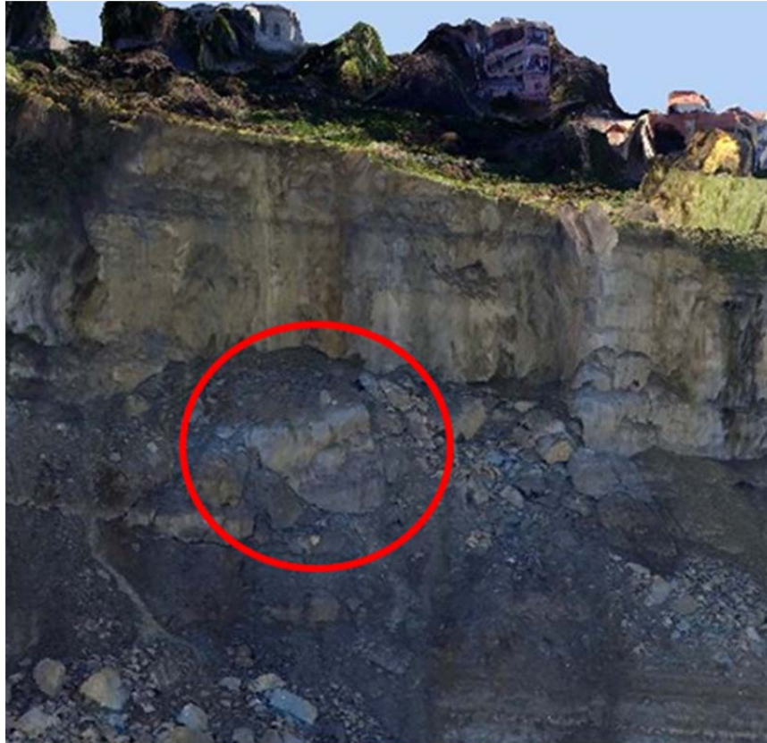
Figure 17: Wedge previously supporting the Blue Marl (Picture generated form Point cloud 3D representation)
