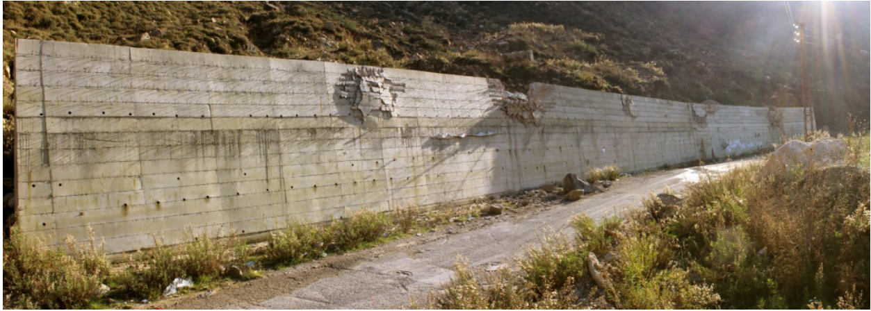
Figure 4: Damage to the Retaining wall following Nov. 2015 landslide (Picture taken at from 33°42'13"N 35°37'36"E)
