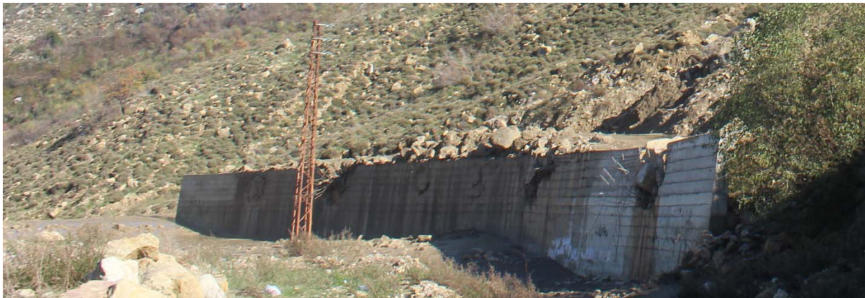
Figure 5: Overtopping of wall due to debris flow following heavy rainfall in January 3 rd , 2016 (Picture taken at 33°42'10"N 35°37'33"E)
