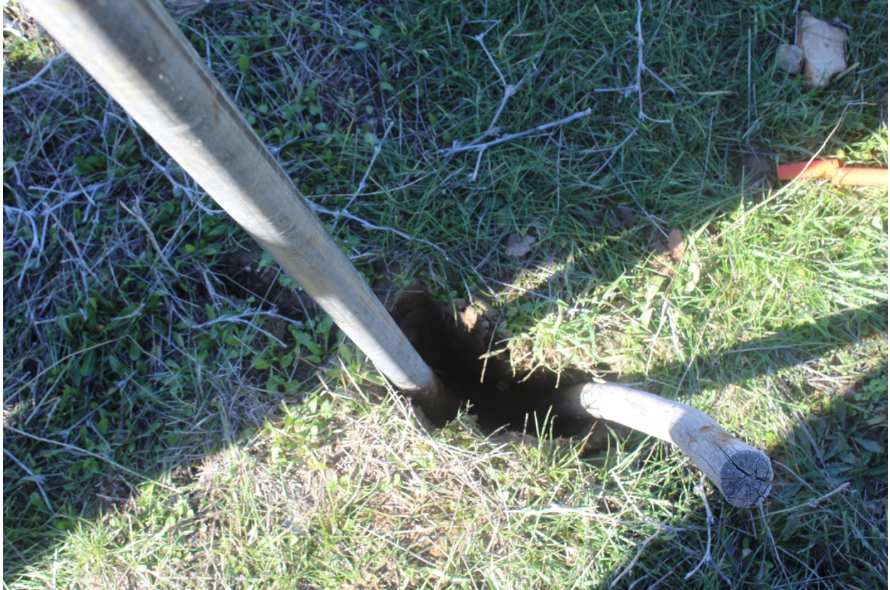
Figure A.4: Surface cracks already well developed in the area between 2012 and 2015 failure.
