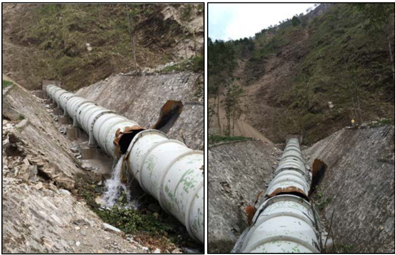
Figure 7-16 Penstock punctured by rock fall (a) 27°54'48.89" N, 85°55'38.25" E, (b) 27°54'46.11" N, 85°55' 38.28" E.
