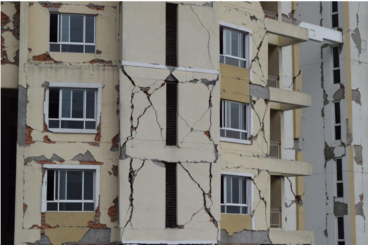
Figure 9-19 Close view of the structural damage (27°44.4'0"N, 85°19.4'0"E).
