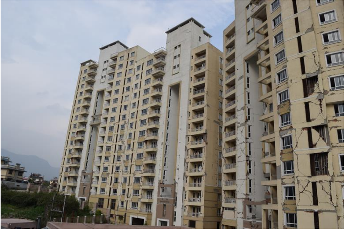
Figure 9-18 Structural damage to the park Horizon Apartment Building at Dhapasi due to the strong ground motion. Eye witness said that the buildings were pounding due to story drift due to ground shaking.
