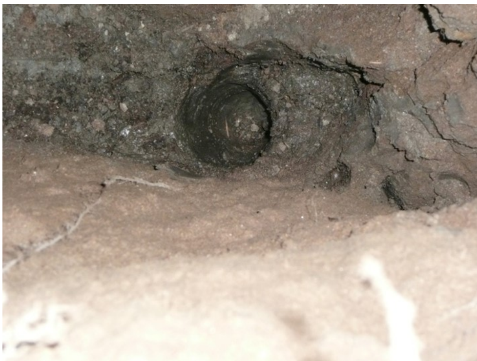
Figure 6-17. Bottom of crack at 2m depth where the "black cotton soil" was sampled. (27.674816° N, 85.362646° E).
