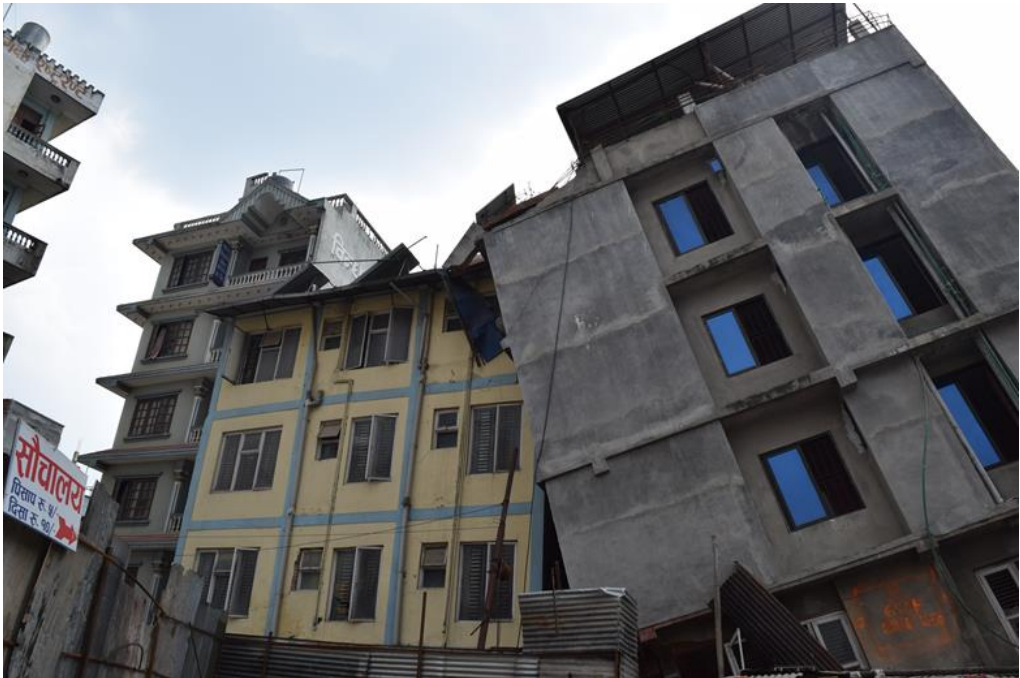
Figure 9-5 Soft-story collapse of a five story building at Gogabu area (27°44'2" N, 85°18'42" E).
