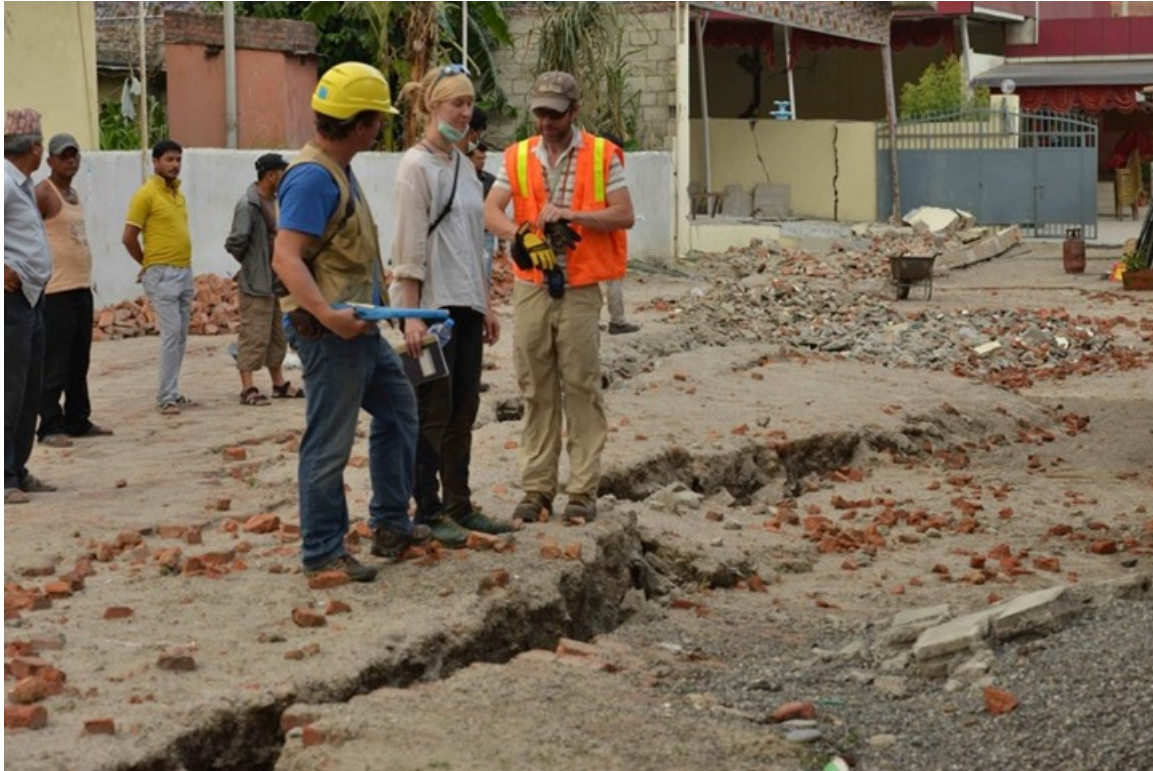
Figure 6-15 Cracks near the top of the rise in Lokanthali ( 27.674816^{\circ} 85.362646^{\circ} and surrounding region). Depth of cracks 2 to 3 m deep. Most of the deformation was reported to have occurred during the first aftershock, with only a small amount of deformation from the mainshock.
