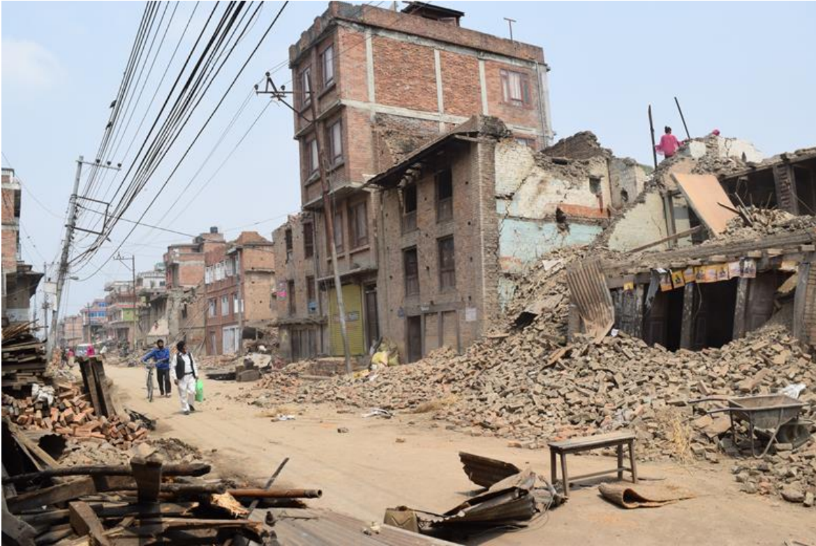
Figure 9-32 Unreinforced brick masonry in mud mortar at Bhaktapur collapsed due to ground shaking whereas the modern RCC structures did not sustain much damage (27°40'33.64" N, 85°24'26.18" E).
