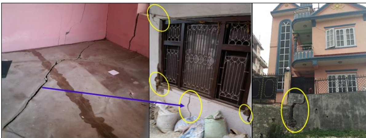
Figure 6-37 Cracks on the floor and walls due to lateral spreading in Syuchatar.
