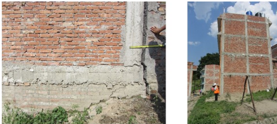
Figure 6-31 (a) Observed cracked in the wall of a RC building due to lateral deformation of ground (b) no damage on a building within the same location as cracks could not pass through the foundation (Location: 27°40'43.22" N, 85°26'10.52" E)
