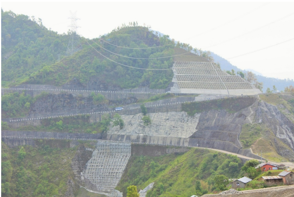
Figure 8-7 Extensive concrete retaining walls and drainage systems of the B.P. Koirala Highway performed very well during the Gorkha earthquake (27° 16' 05.98" N; 85° 56' 40.56" E).
