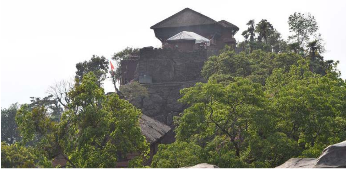
Figure 9-43 Retaining walls of Gorkhna Temple/Gorkha Palace showing shear cracks.
