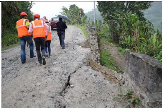
Figure 5-29 Damage to retaining wall due to excessive settlement and ground shaking.
