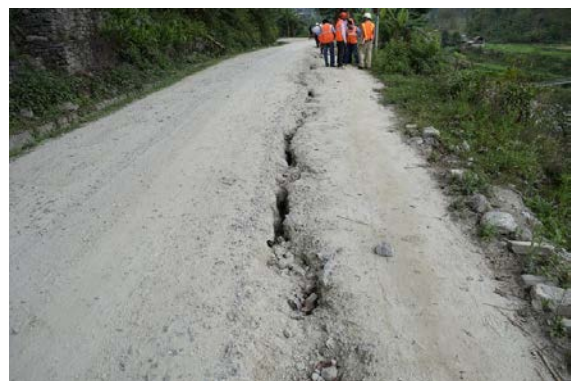
Figure 5-26 Settlement crack along the roadway.
