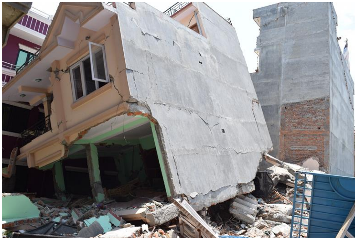
Figure 9-16 More than 5 buildings were collapsed near this building at Sitapaila area (next to the building shown in Figure 9-15).
