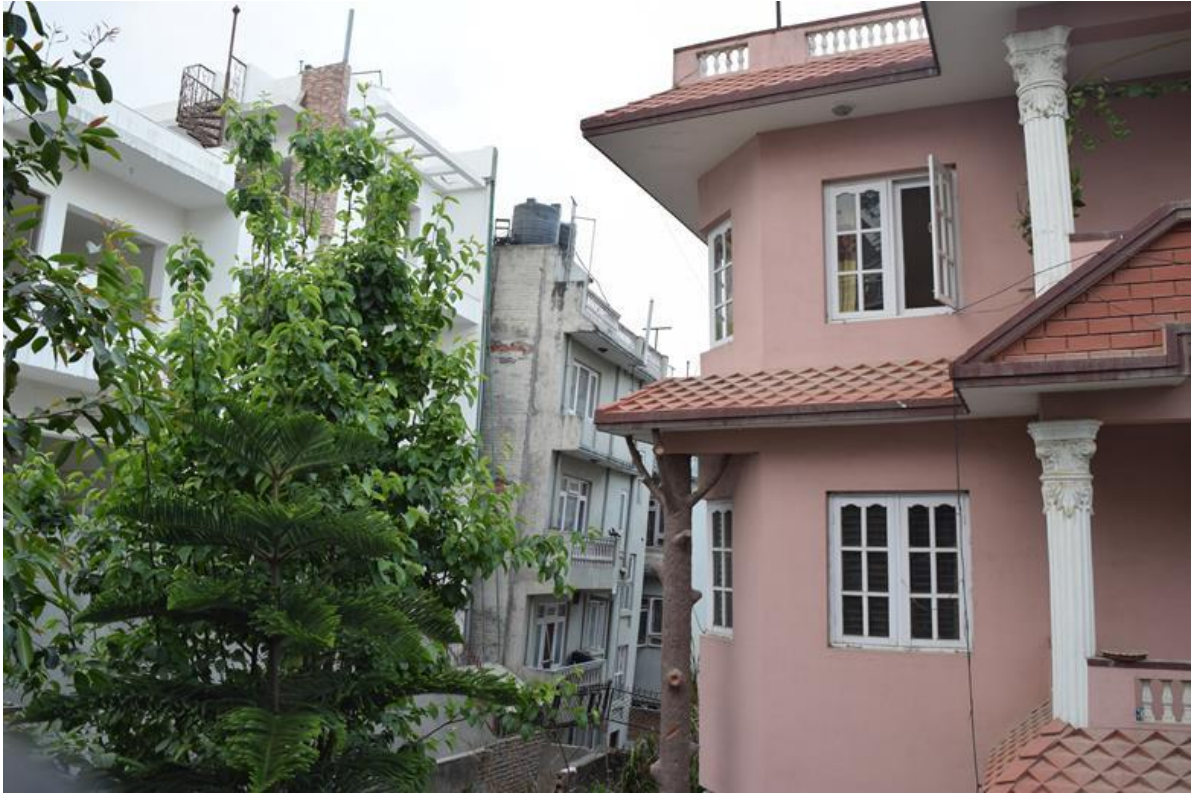
Figure 9-29 Buildings tilted at Lokanthali area (opposite side of the one presented in Figure 9-28) due to ground failure ( 27^{\circ}40'25.83'' N, 85^{\circ}21'44.3'' E).
