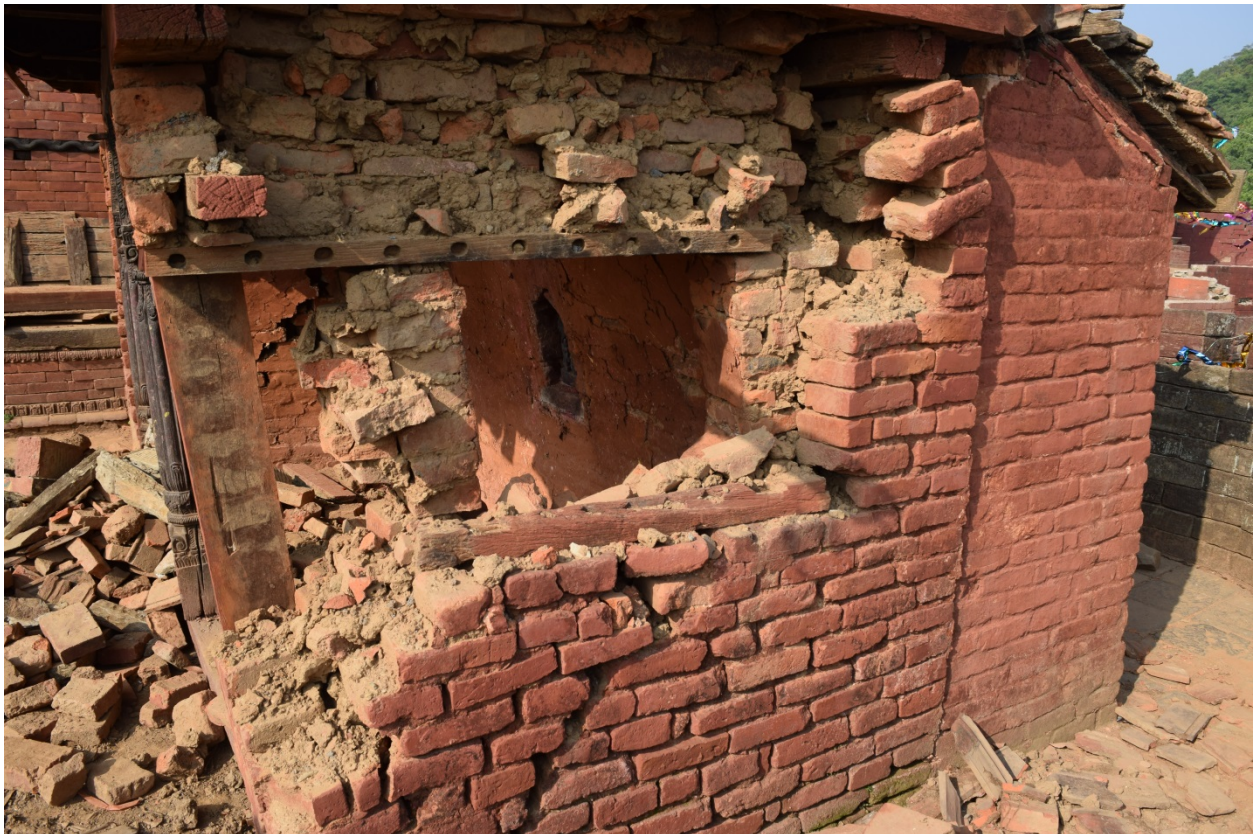
Figure 9-44 Damage to Gorakhnath Temple walls due to the earthquake shaking (28°0.217'0" N, 84°38.3'0" E).
