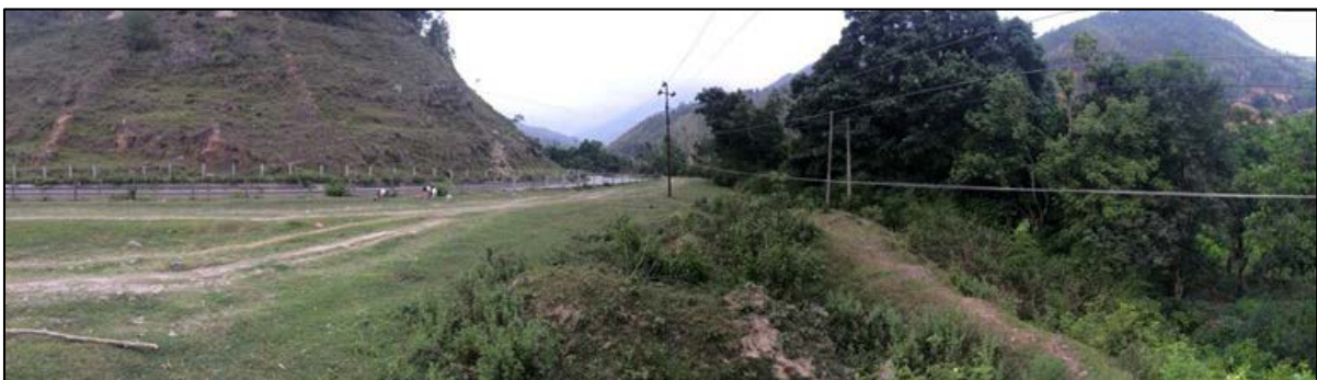
Figure 7-14 Section of Trishuli canal that leaked after the April 25th earthquake. Fresh head scarp (hummocky vegetated area left of power lines) along the outer edge of the fluvial terrace to the right of the canal suggest that this area is unstable and may have mobilized during the earthquake, possibly causing extension along cold joints in the canal liner (27°56'49.48"N, 85° 9'37.79"E).
