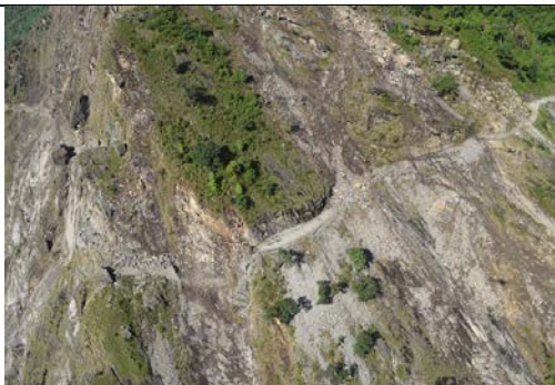
Figure 5-48 Charikot-Lamabagar road sector affected by landslides triggered due to the earthquake.
