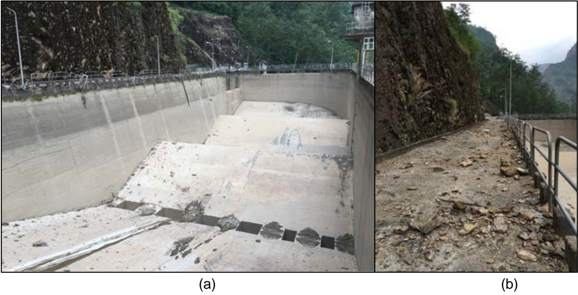
Figure 7-15 The Upper Bhotekoshi Headworks - Handrail damage, surficial debris impact and debris inundation from rock fall was observed at the gravel catchers. Remaining risks of damage and danger to life safety in this area are remaining risks. (a) 27°56'17.80" N, 85°56'42.88" E, (b) 27°56'17.39" N, 85°56'43.10" E
