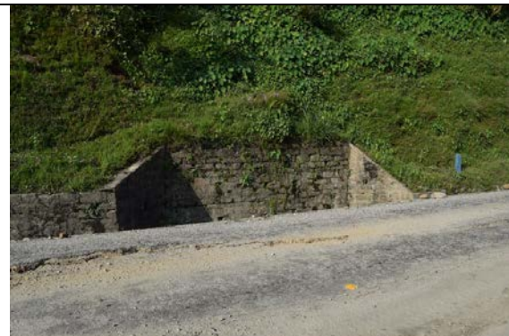
Figure 5-16 A subsurface drainage work installed at a landslide site along the Araniko Highway performed well during the earthquake.
