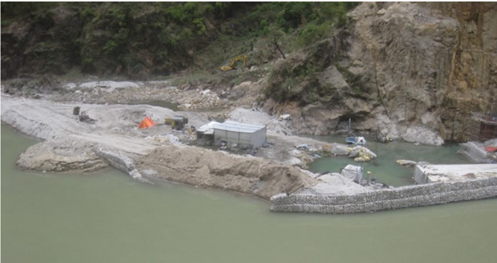
Figure 8-18 Lost diversion wall at Upper Tamakoshi Hydropower Plant ( 27 55'29.1"N, 86 12'47.26"E)
