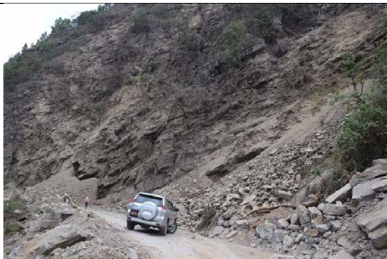
Figure 5-31 A rockslide that poses a potential hazard to the roadway and below.
