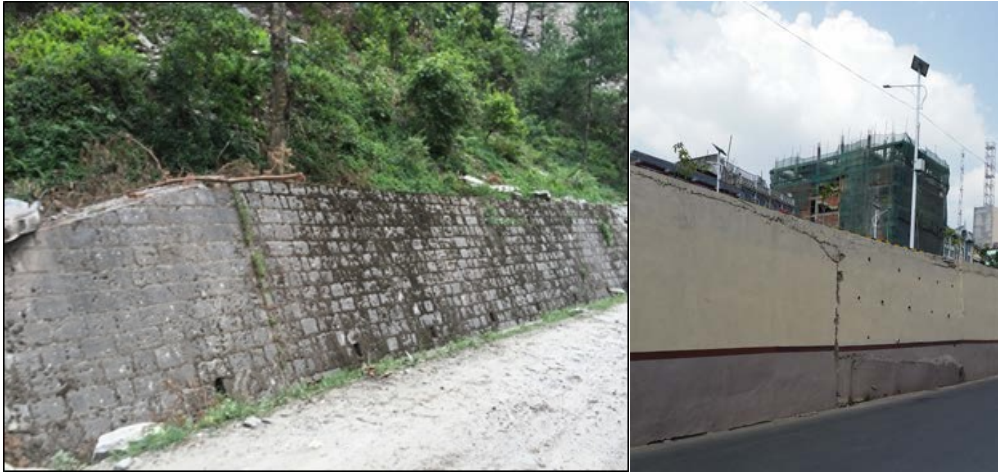
Figure 8-14 Retaining walls generally behaved well during after the April 25 mainshock and aftershocks with limited cracking (a) 27 54' 59.2"N 85 55' 48.4"E, (b) 27 41' 20.1"N 85 19' 51.2".
