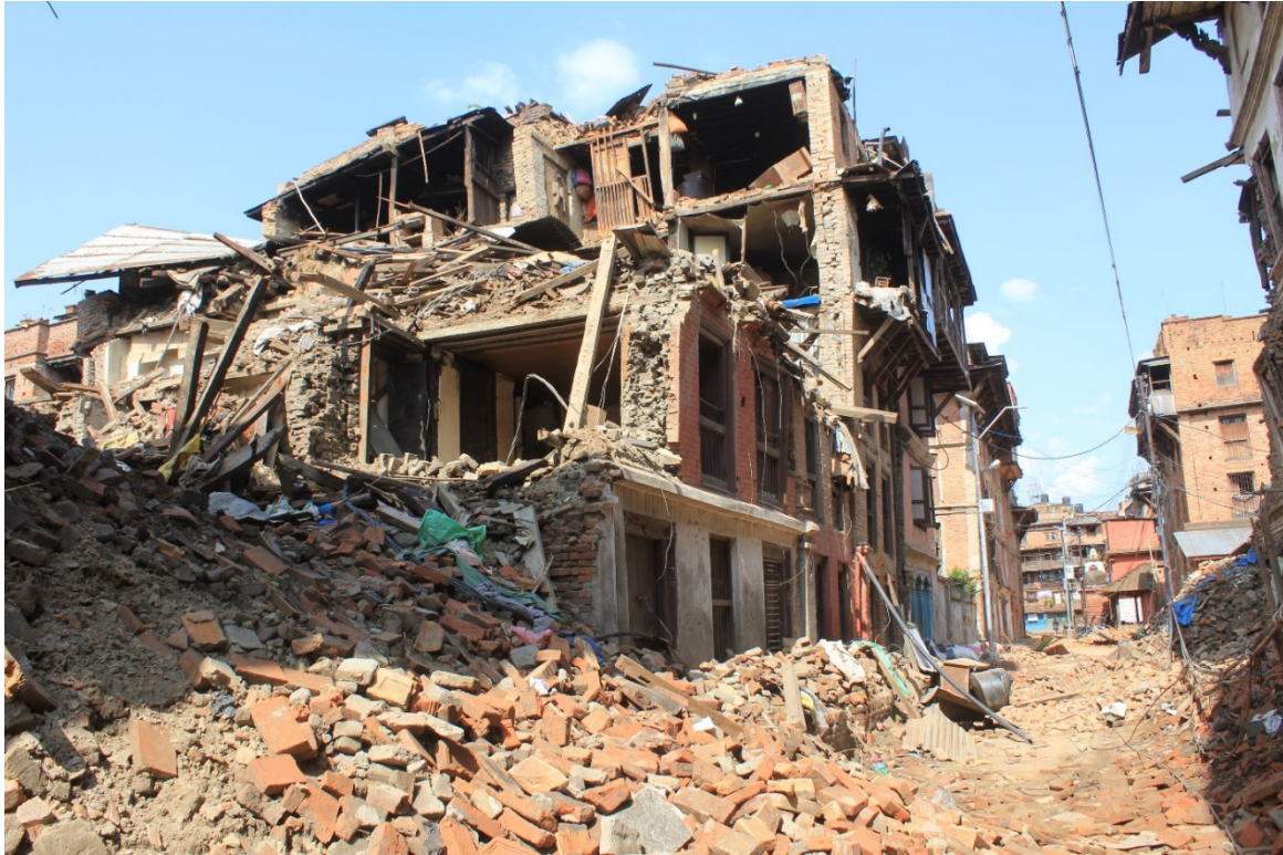
Figure 9-35 Collapsed unreinforced masonry building in Bhaktapur following the Gorkha earthquake (27° 40' 21.64" N; 85° 25' 58.24" E).
