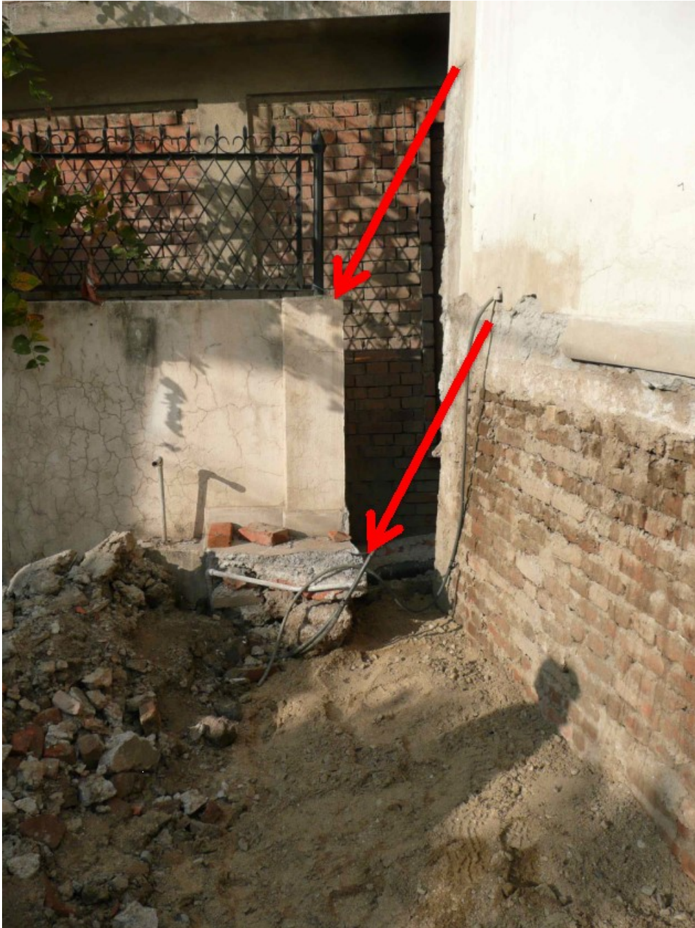
Figure 6-19. House on the hanging wall of the crack. The ground pulled away from the structure dropping upwards of 3/4 m and moving laterally 1/2 m. Before the earthquake the brick foundation was completely below the ground surface.
