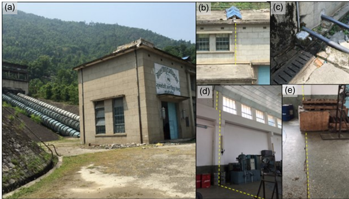
Figure 7-22 A continuous crack running through the walls and the floor is observed in the powerhouse structure. This observed crack can be potentially due to the differential settlement across the power plant structure, which can be further supported by the cracks and slight vertical offset observed in the pavement shown on the upper left side (7-21 27°45'13.96"N, 85°50'17.26"E).
