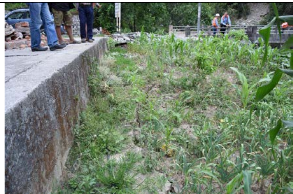
Figure 5-30 Settlement cracks observed along a bridge abutment.
