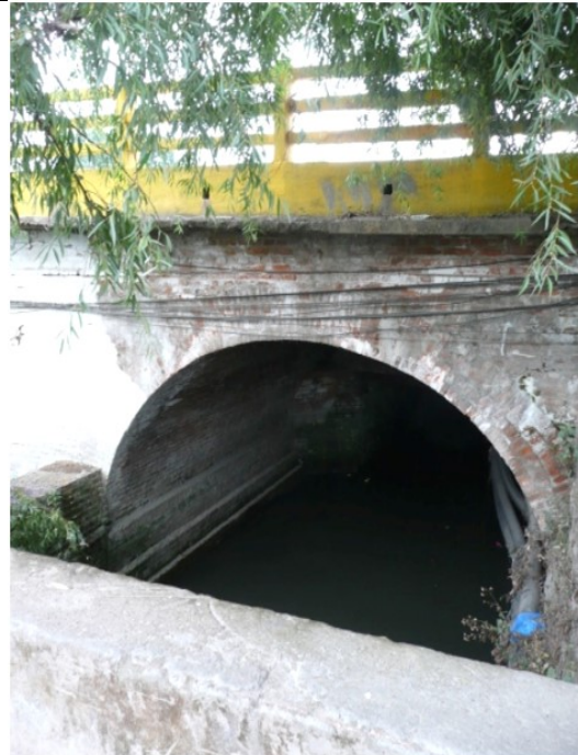
Figure 6-9. Creek below the bridge (27.698793° 85.320060°). The flood plain of this creek defines the extent of the cracking, with the cracks parallel to the creek alignment.
