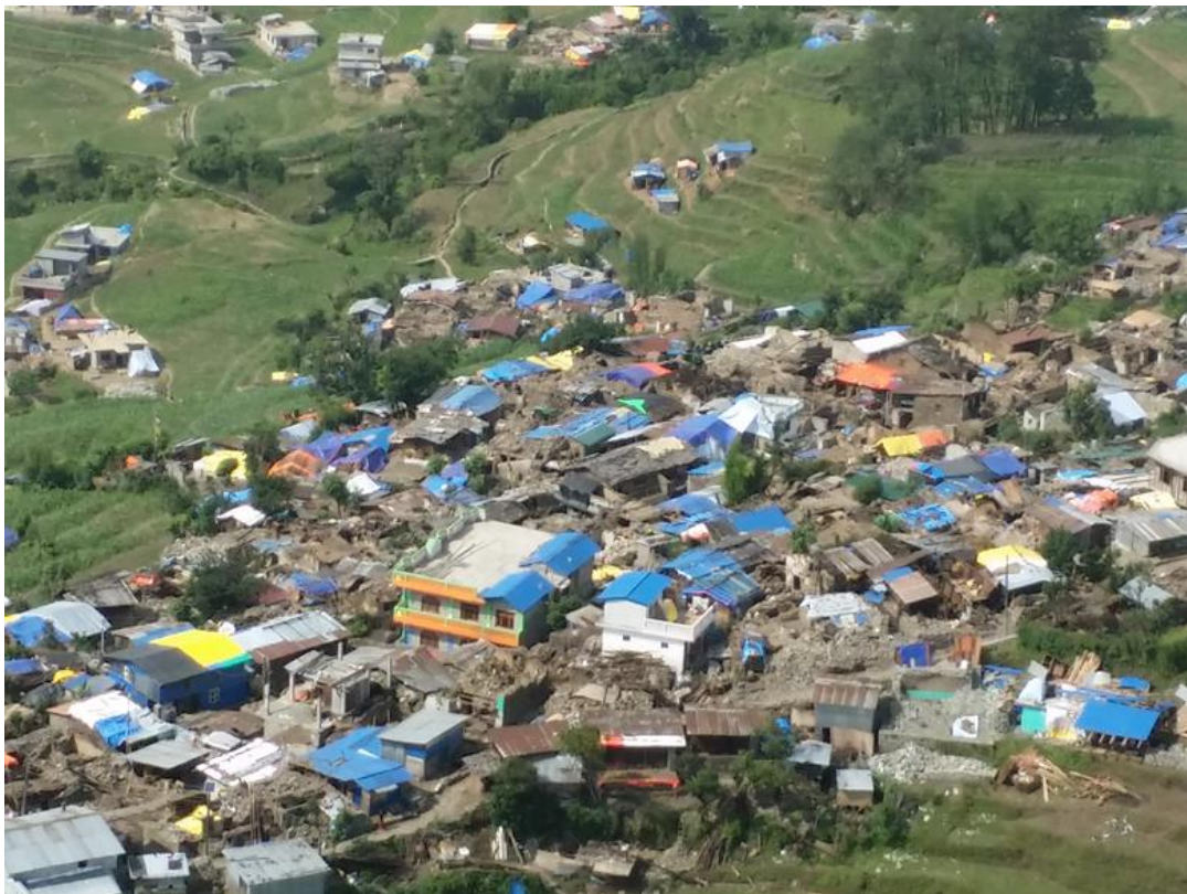
Figure 9-48 Closer look at the earthquake damage to stone masonry and RCC buildings.
