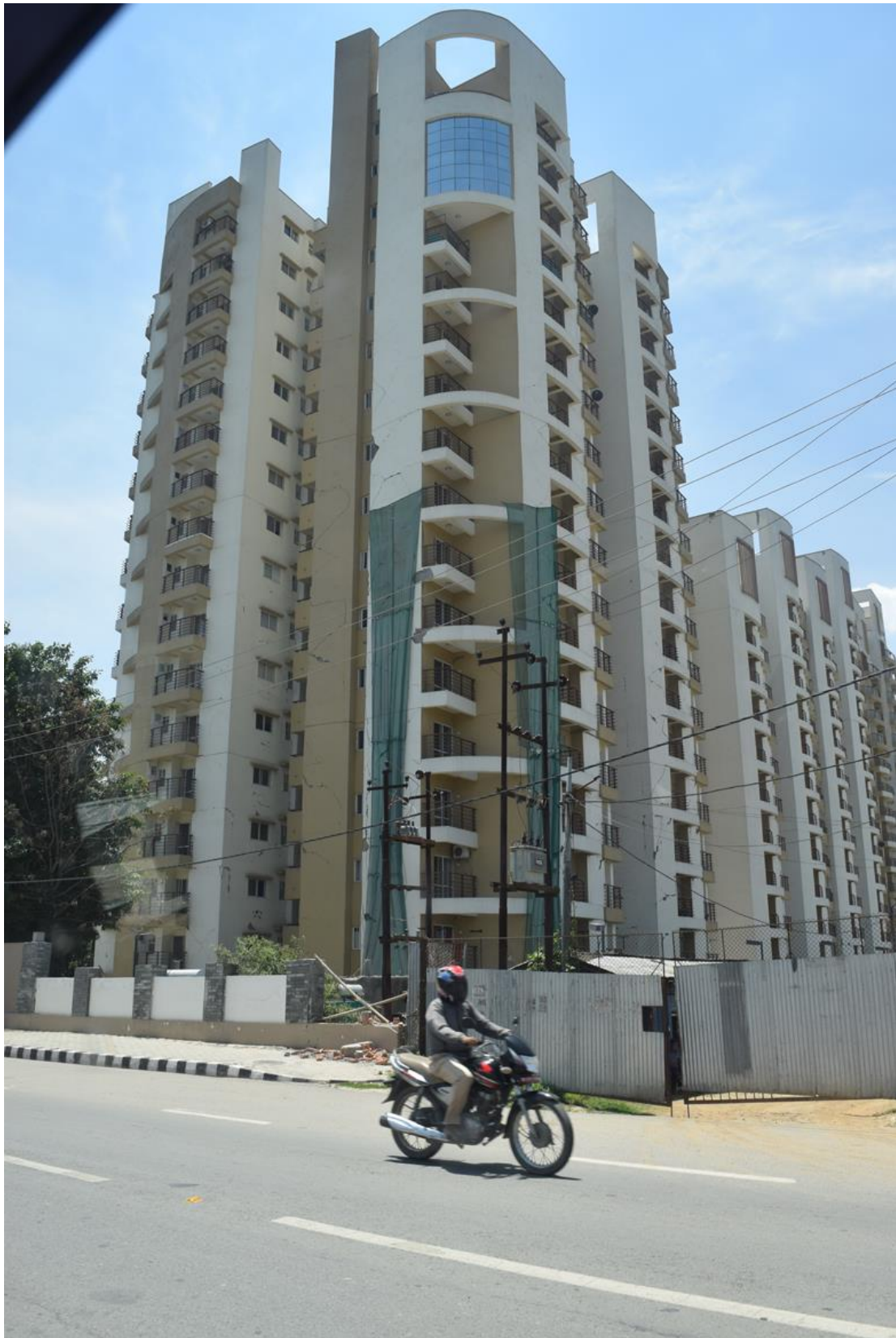
Figure 9-22 A high rise apartment building at Hattiban, Lalitpur. This building also sustained some major damage due to the earthquake.
