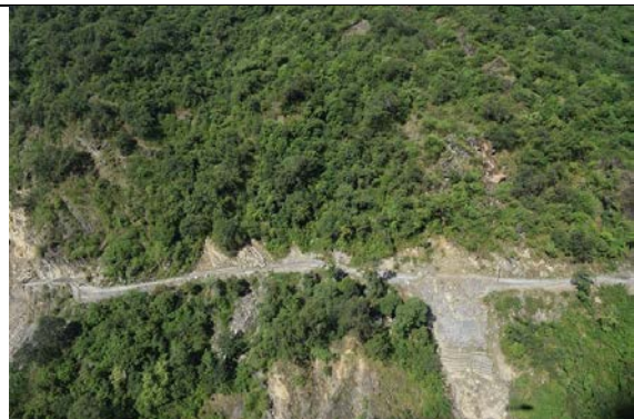
Figure 5-49 Gabion retaining walls that did not perform well along the Charikot-Lamabagar Road.
