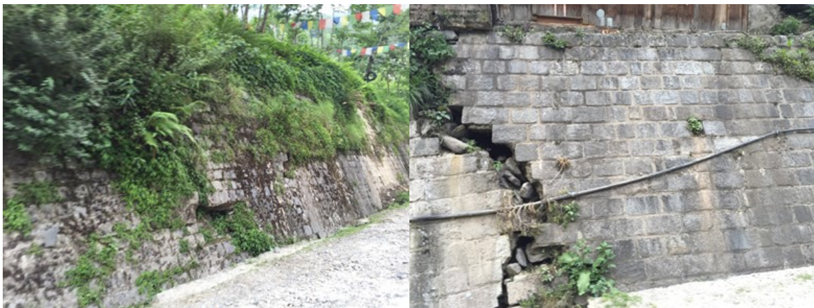
Figure 8-16 Damaged Retaining Wall (a) 27 57' 36.4"N 85 57' 24.2"E, (b) 27 56' 57.2"N 85 57' 8.28"E.
