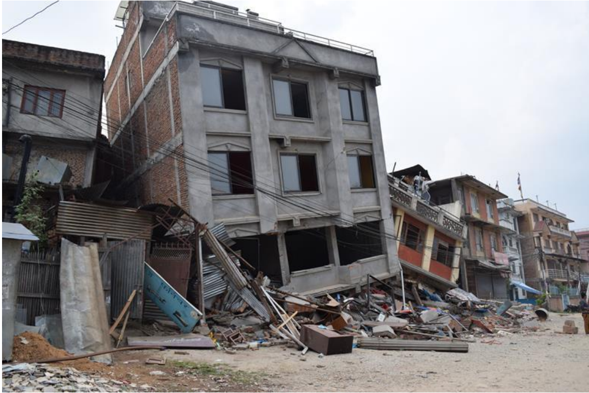
Figure 9-13 Five buildings collapsed along the ridge line at Sitapaila area near Ring Road at Swayambhunath. One building at the rightmost part of the picture was not damaged ( 27^{\circ}42.7'0'' N, 85^{\circ}17'0'' E).
