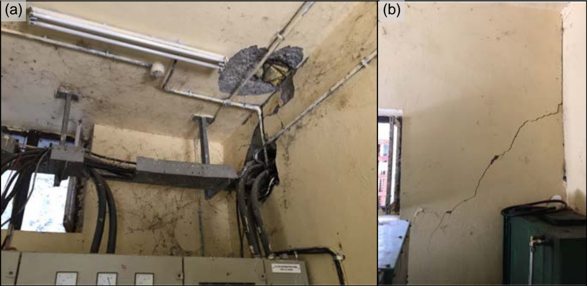
Figure 7-5 Secondary buildings at Chilime exhibited minor shaking. Damage was limited to cracks in infill walls and holes in the roofs of some structures. (a) 28°9'27.30" N, 85°16'54.38" E, (b) 28°9'27.30" N, 85°19'54.38" E
