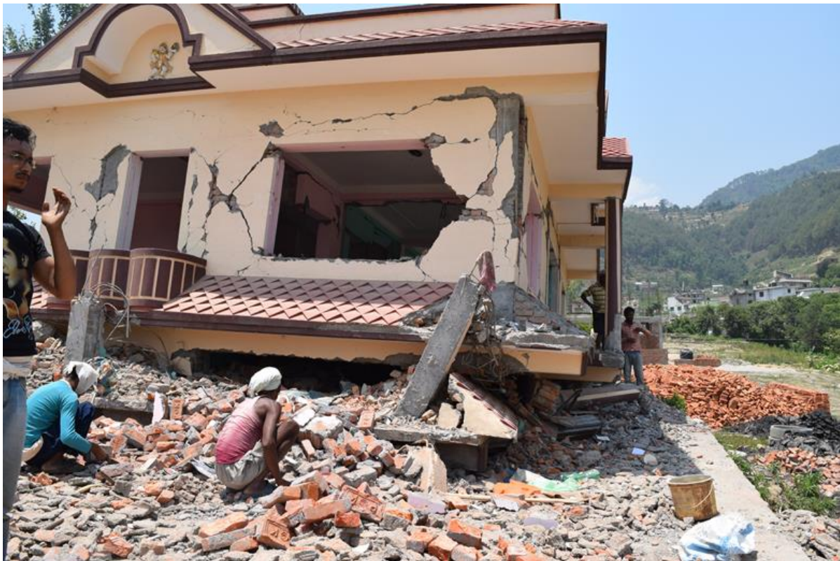
Figure 9-17 Typical modern building collapse pattern at Ramkot, Kathmandu.
