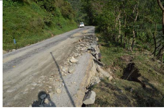
Figure 5-18 Typical road fill settlement observed along the Araniko Highway.
