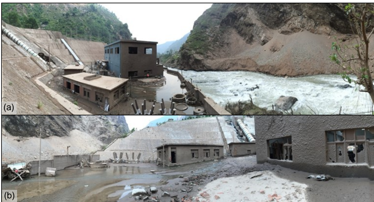
Figure 7-18 A debris plume and water from the impact of the rock fall across the river is hypothesized to have broken windows and resulted in the silt coating on river-facing walls of the powerhouse (contrast blue walls facing away from river with brown, silt coated walls)
