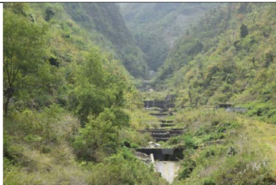
Figure 5-5 Check dams near the powerhouse of Marshyangdi Hydropower Project, which performed well during the 2015 earthquake (27°52.5'0"N 84°32.4'0"E).
