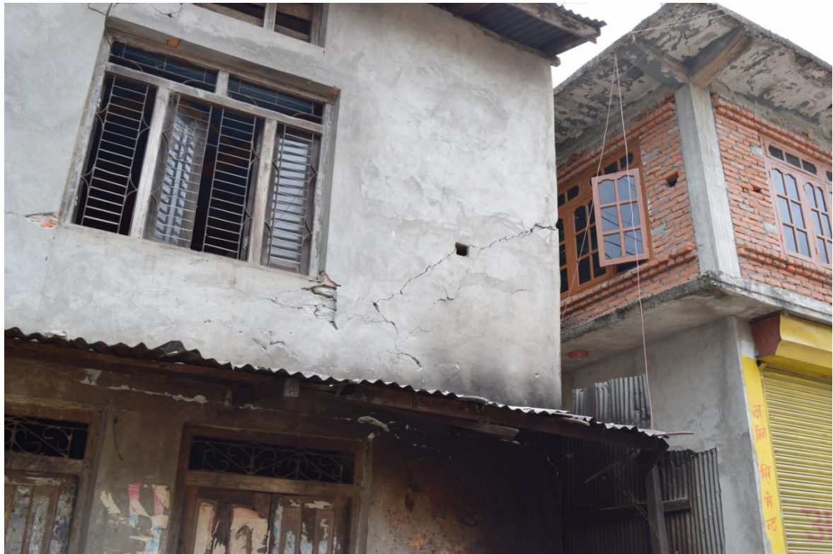
Figure 9-56 Another example of comparative performance of unreinforced and reinforced buildings in Melamchi, Sindhupalchowk.
