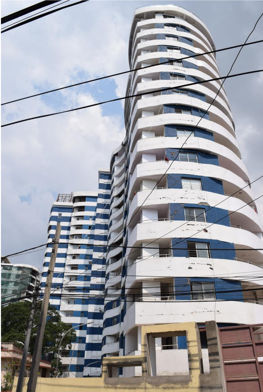
Figure 9-25 Damage observed at an apartment complex in Kalikasthan ( 27^{\circ}42'13'' N, 85^{\circ}19'38.3'' E).
