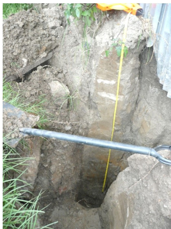
Figure 6-18. Hand trench to 2m depth to acquire bulk sample of "black cotton" silty clay. Depth coincides with slip surface of nearby houses that experienced vertical deformation of up to 0.75 m. Here the trench is dug into the hanging wall of the crack (27.674316° N, 85.362654° E).
