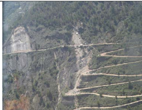
Figure 5-60 Gabion retaining walls on the feeder road to the Trishuli-Rasuwegadi Road damaged by the earthquake.
