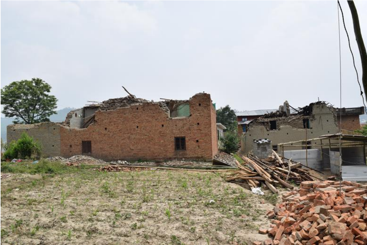
Figure 9-34 Old buildings with unreinforced brick masonry at Indrayeni Village got damaged due to ground shaking (27°43.7'0" N, 85°26.2'0" E).
