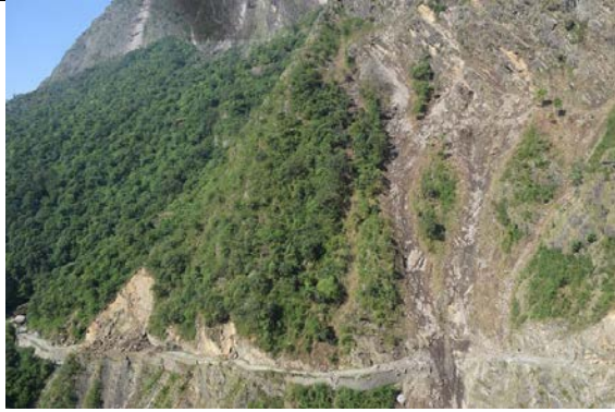
Figure 5-50 landslides observed along the road alignment constructed along steep terrain.
