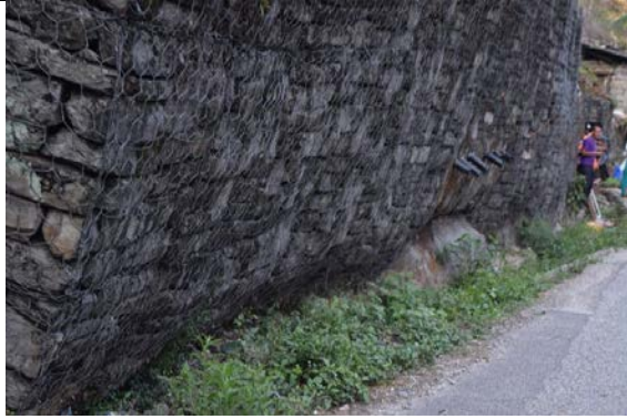
Figure 5-17 Gabion Retaining wall implemented as the landslide prevention work for existing landslide tilted after the 2015 earthquake.
