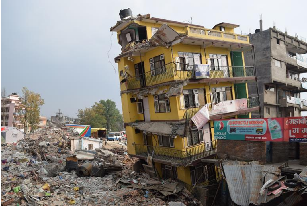
Figure 9-9 Collapse of a six-story lodge at Balaju killed more than 20 people ( 27^{\circ}44'06'' N, 85^{\circ}18'20'' ).
