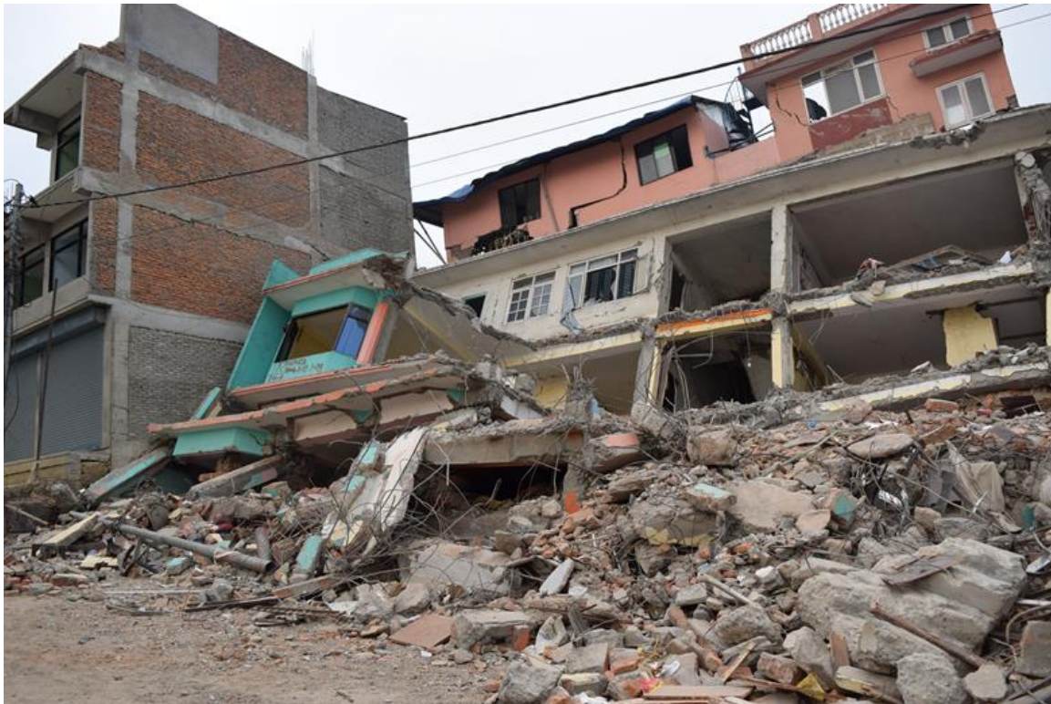
Figure 9-15 Collapse of two multi story buildings at Sitapaila killed over 20 people (27°42.7'0"N, 85°17'0"E).
