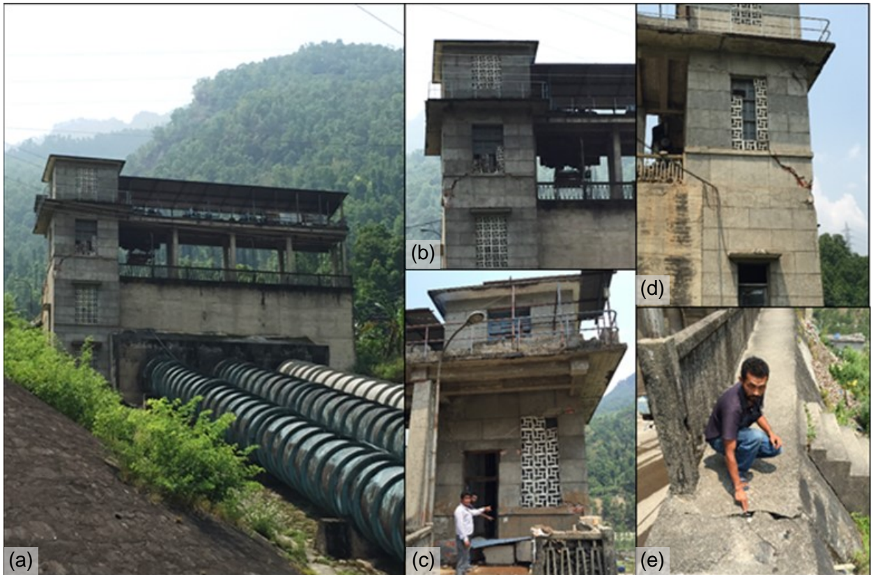
Figure 7-21 Structural damage observed in the intake structure of Sunkoshi powerhouse. Significant shear cracks were observed in the upper structure after the May 12 th M 7.3 aftershocks. No significant damage was observed in the penstock ( 27^{\circ}45'10.66''\text{N} , 85^{\circ}50'17.70''\text{E} ).
