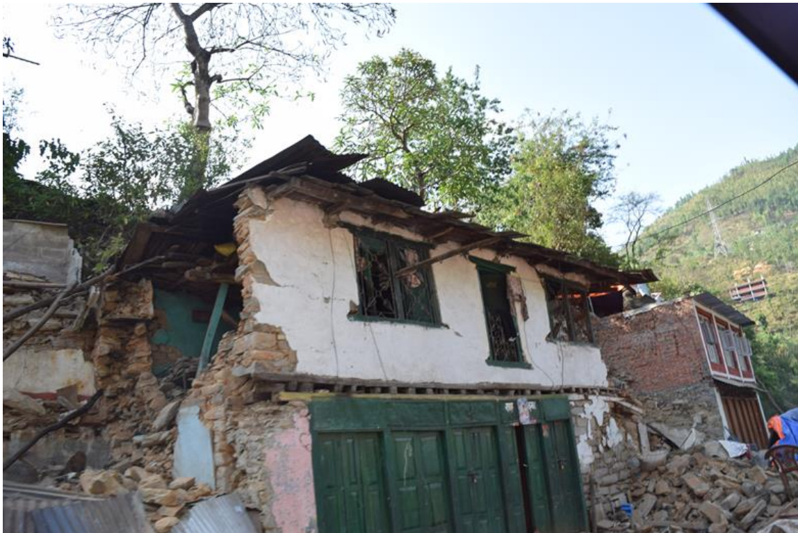
Figure 9-53 Old unreinforced masonry buildings sustained massive damage while modern buildings performed relatively better at Dolalghat, Kavre District, along Araniko Highway.
