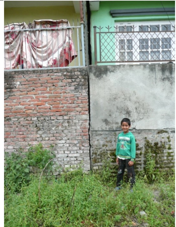
Figure 6-11. Tilt of left building away from right building, measured at roughly 2 degrees (27.745523° N, 85.302223° E).
