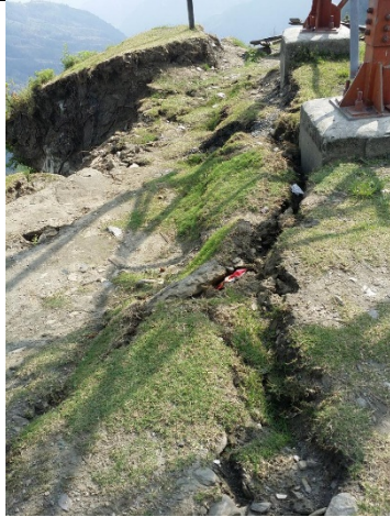
Figure 5-110 Main scarp of a seismically induced landslide observed at the north east edge of the Barpak Village, epicenter of the April 2015 Gorkha earthquake.
