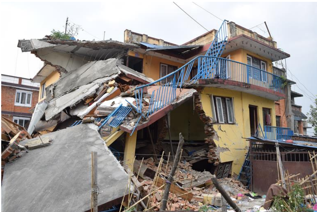
Figure 9-10 Building damage pattern at the ridge of Balaju Baisdhara area. This area is considered a rock site ( 27^{\circ}44'6.71'' N, 85^{\circ}18'11.51'' E).
