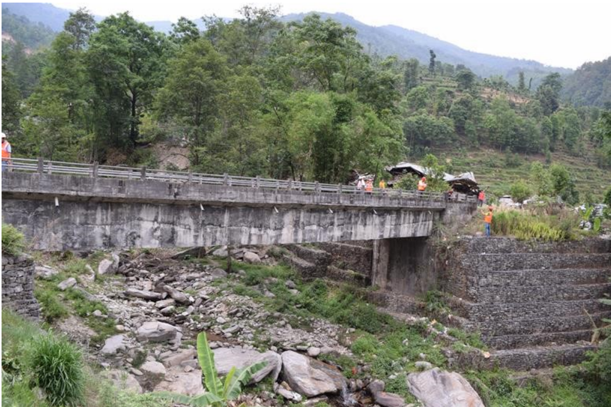
Figure 8-12 Bridge along the access road of Melamchi Water Supply Project being threatened by potential landslides along river banks and seismic settlement of road fill materials ( 27^{\circ}55'38.43''\text{N} 85^{\circ}33'14.510''\text{E} ).
