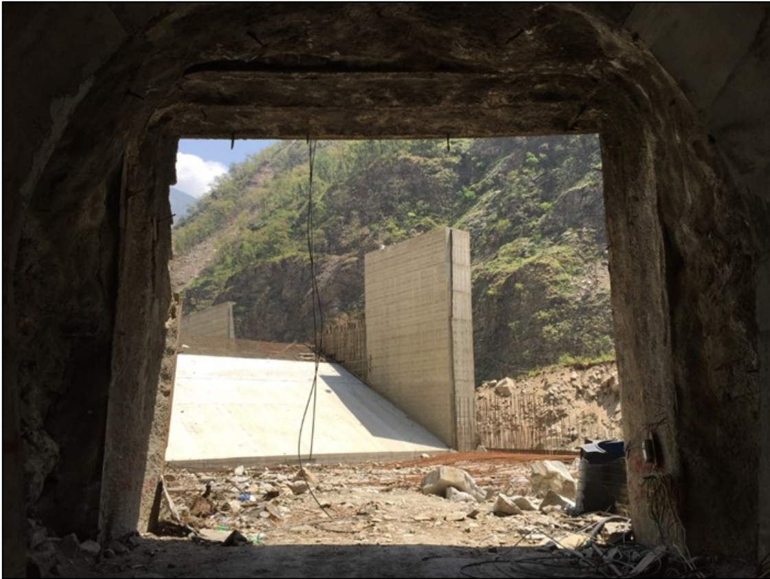
Figure 7-10 Scattered rockfall debris observed outside portal entrance with risk of continued rock fall evident. View is upstream toward dam (not shown) (28°3'36.20" N, 85°12'24.21" E).
