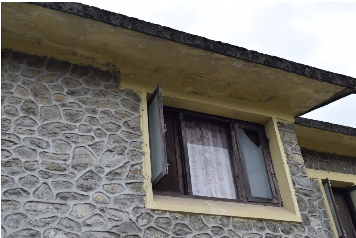
Figure 9-40 Damage to stone masonry walls under heavy roof at the staff quarter of Western Region Campus of the Institute of Engineering.
