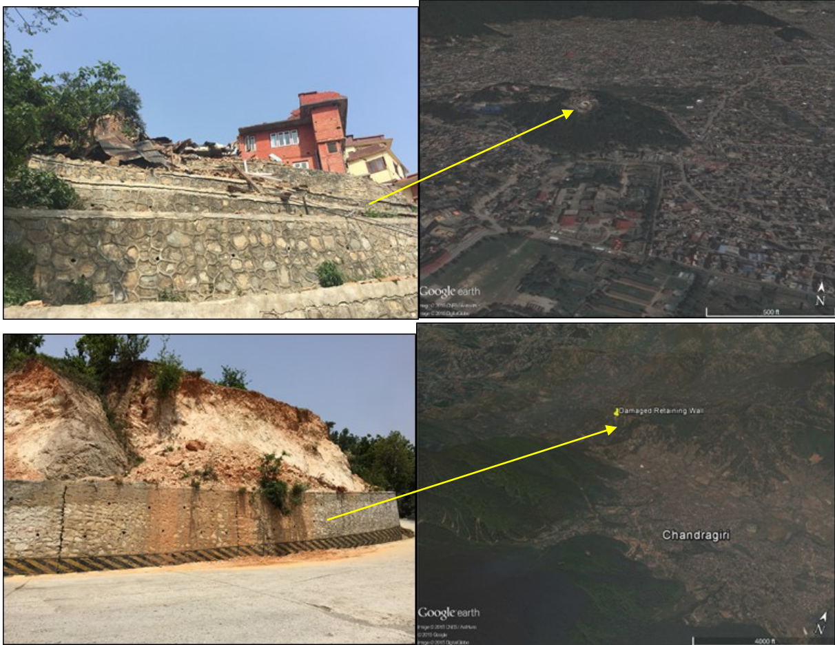
Figure 8-17 Retaining wall damage observed at the ridges (a) around Monkey Temple, Kathmandu (27 42' 54"N 85 17' 23.5"E) (b) around western basin edge of Kathmandu valley (27 42' 51.5"N, 85 11' 59.7"E).
