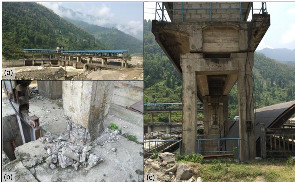
Figure 7-19 (a) Headworks damaged by June 2014 landslide and the 2015 earthquake (27°45'30.24" N, 85°52'5.39" E), (b) Concrete spalling expected to be as a result of earthquake induced shaking (27°45'26.85" N, 85°52'3.33" E), and (c) Headworks structure shifted to the right ) on top of the beam column base structure ( 27°45'29.40" N, 85°52'3.25" E)
