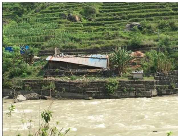
Figure 8-15 Damage in retaining walls due to the slope failures (a) 27 45' 22.2"N 85 51' 8.18"E
