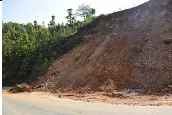
Figure 5-11 Typical landslide observed at the Panchkhal-Dolalghat sector of the Araniko Highway.
