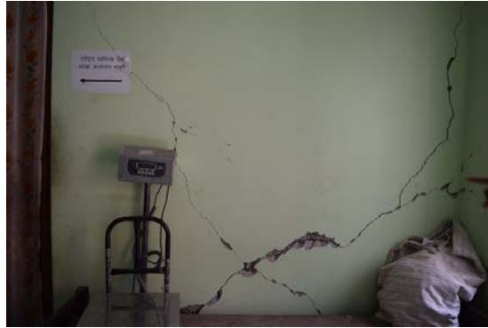
Figure 9-52 Structural damage pattern at a building in Gajuri, Dhading.
