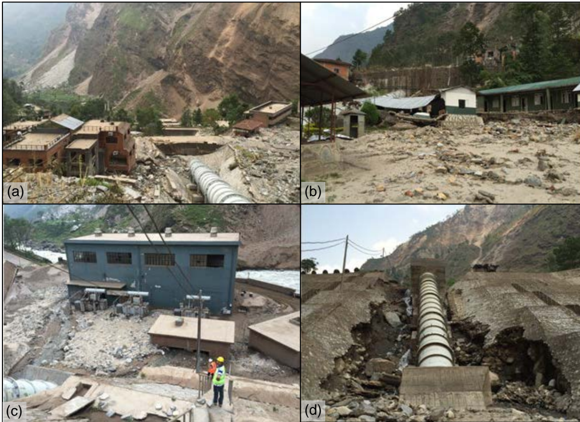
Figure 7-17 (a) Debris flow damage (27°54'45.77" N, 85°55'38.00" E), (b) Debris flow damage the workers colony (27°54'44.47" N, 85°55'32.87" E ), (c) powerhouse, showing debris that has accumulated to the top of doorways in the powerhouse area (27°54'45.67"N, 85°55'28.23"E ), (d) penstock liner (27°54'45.32" N, 85°55'27.15" E)
