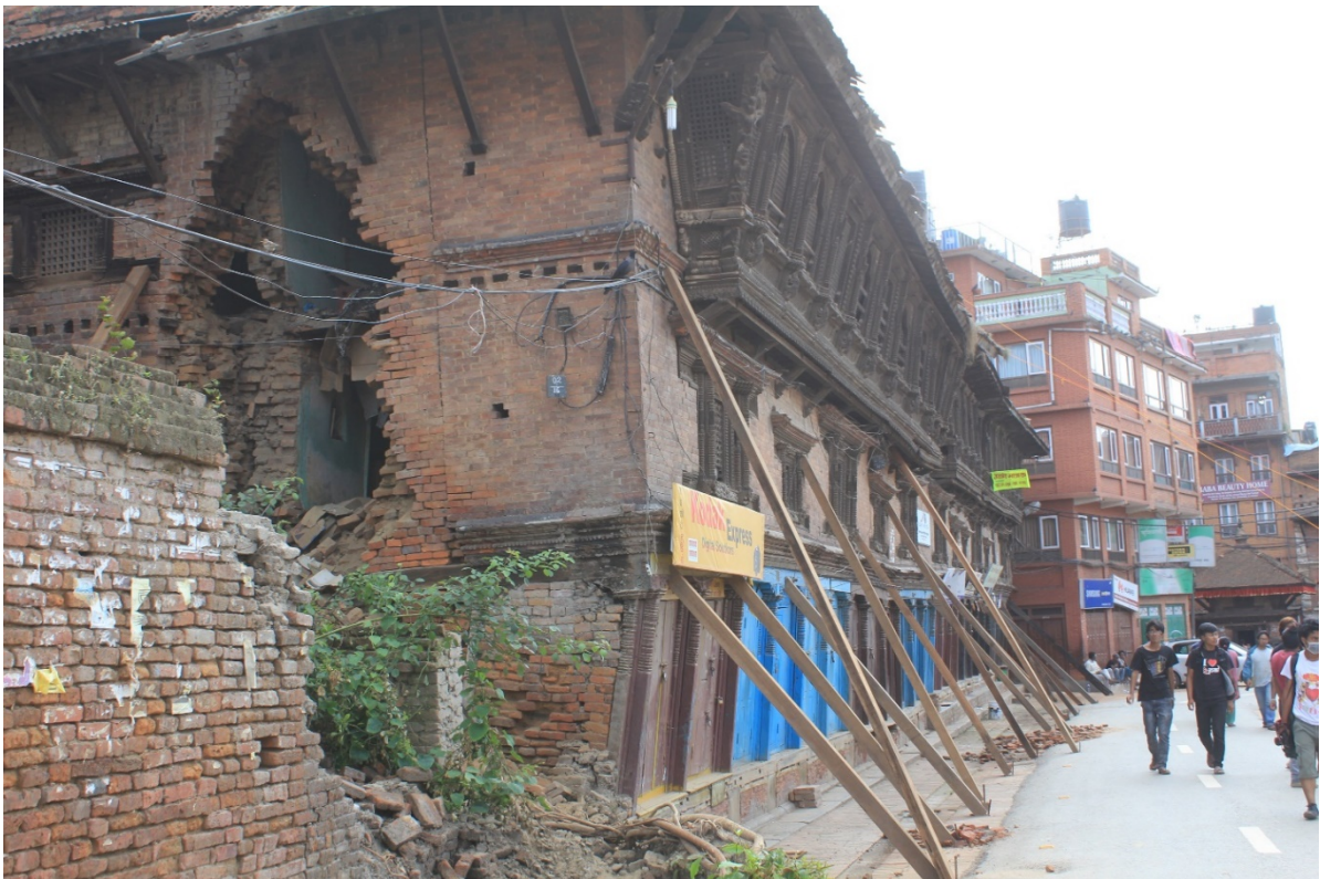
Figure 9-36 Distressed unreinforced masonry building and façade following the May 12, 2015, M_w 7.3 aftershock (27° 40' 19.45" N; 85° 25' 40.80" E).
