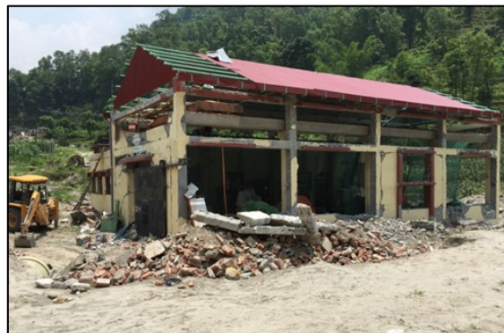
Figure 7-23 Shaking damage to powerhouse building observed. Infill walls collapsed. Concrete reinforced frame appeared to suffer little damage. Some liquefaction also evident in the area around the structure. (27°46'36.05" N, 85°53'25.62" E)
