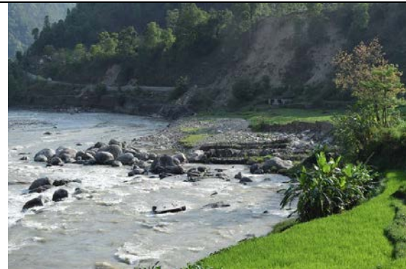
Figure 5-14 Reactivation of an existing landslide along the Araniko Highway that was triggered due to stream undercutting (27°44.7'0"N 85°47.5'0"E).
