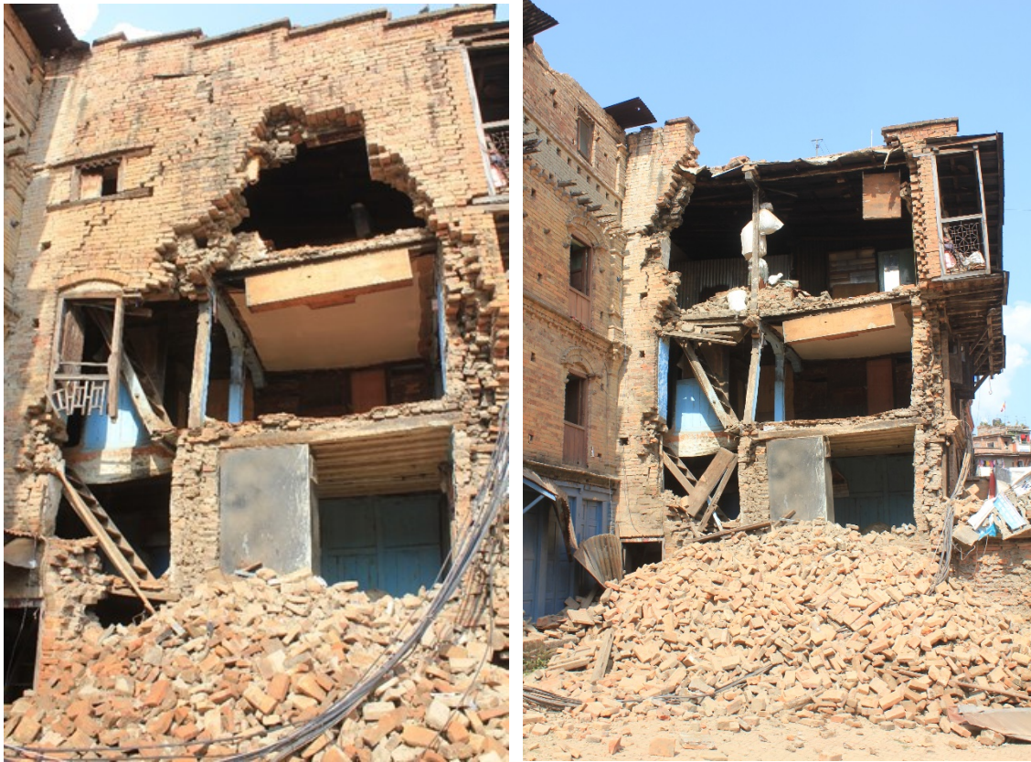
Figure 9-37 Photos on left taken May 11, 2015 and photo on right taken after the May 12, 2015 M_w 7.3 aftershock. Already damaged unreinforced masonry building experienced additional collapse ( 27^{\circ} 40' 21.15'' N; 85^{\circ} 25' 56.23'' E).
