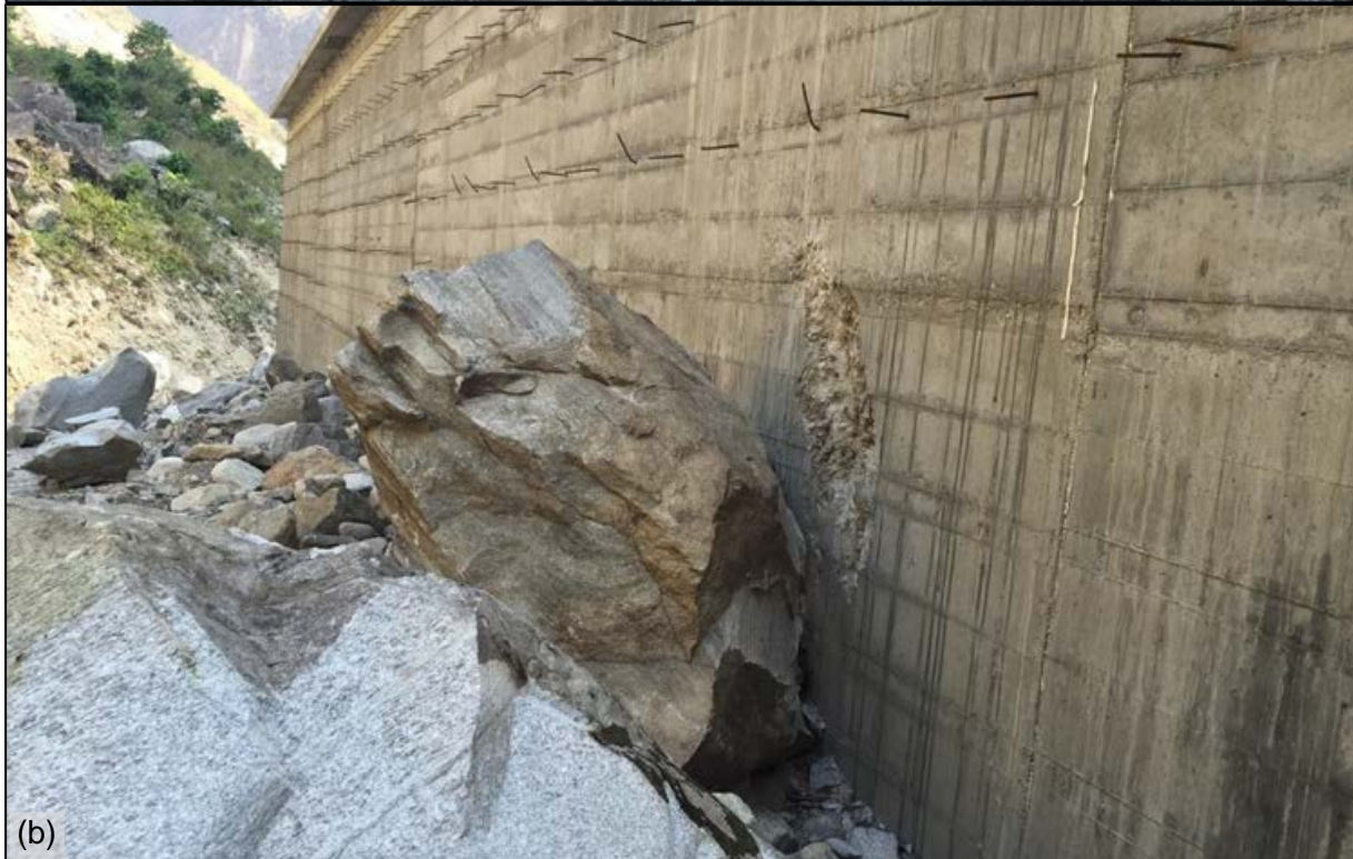
Figure 7-9 Sand trap under construction downstream of the headworks diversion dam were impacted by rockfall from above. Damaged observed was not consequential. (a) 28°3'41.77" N, 85°12'24.74" E, (b) 28°3'40.03" N, 85°12'23.69" E
