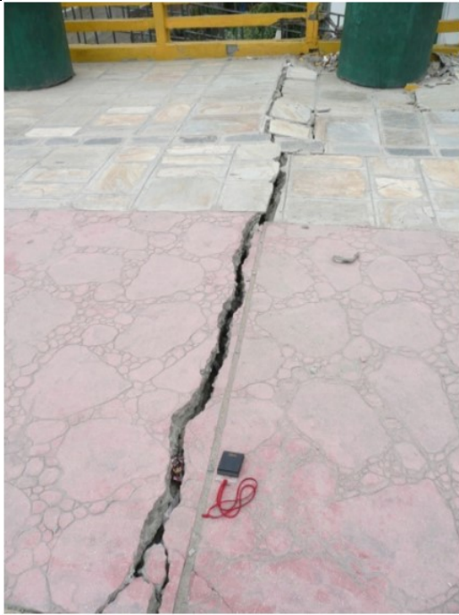
Figure 6-8. Cracking in concrete section of bridge (27.698793° 85.320060°). Cracks on both sides of the bridge line up with the creek below. No cracking in the asphalt over fill section, it behaved in a ductile manner
