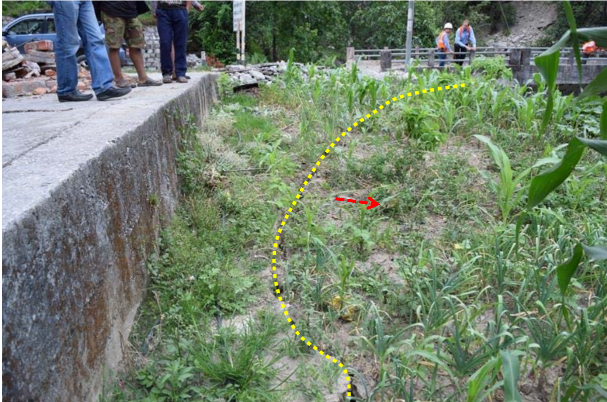
Figure 8-13 Potential landslides along the river bank that are endangering the bridge approach road (27°55'38.988"N 85°33'14.598"E).
