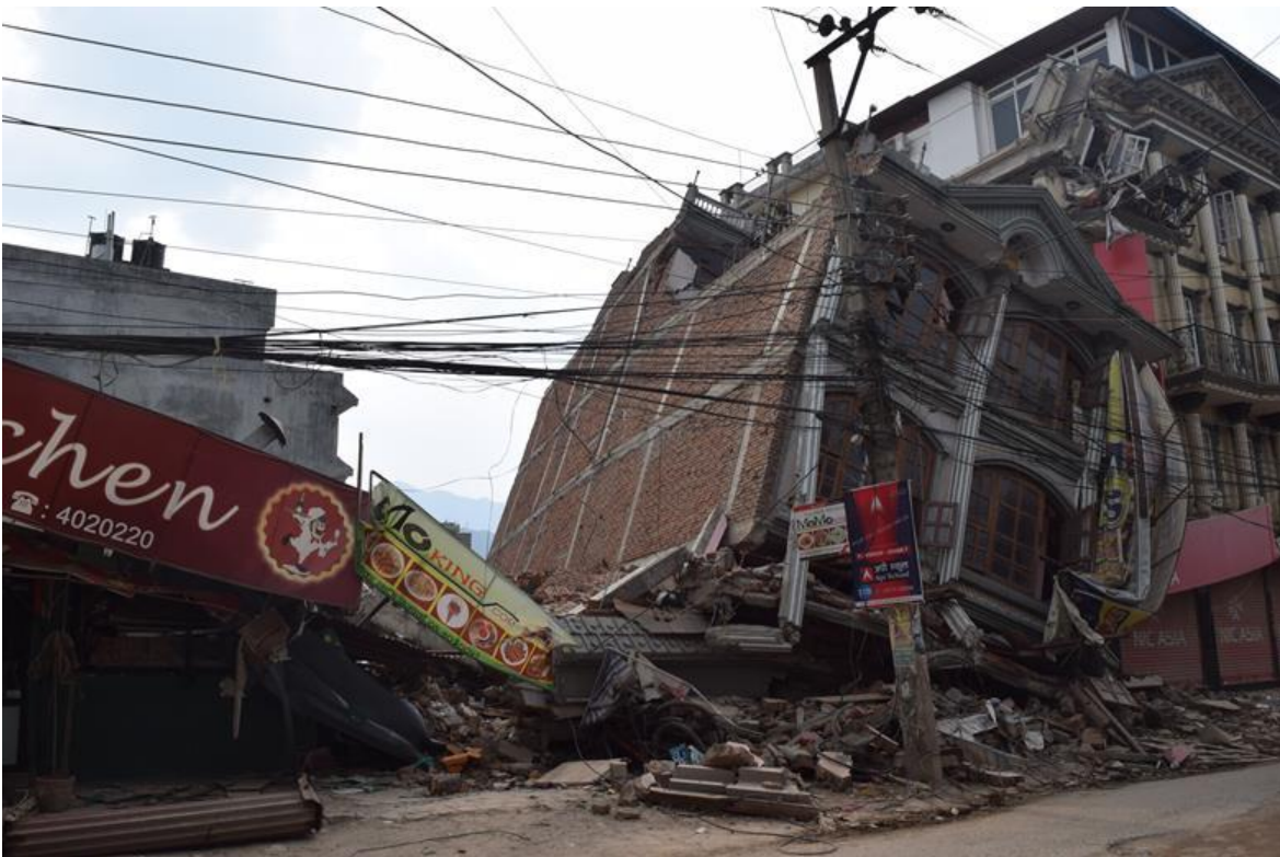
Figure 9-33 A four and half story RCC frame structure collapsed at Samakoshi, Kathmandu (27°43'49" N, 85°18'52" E).
