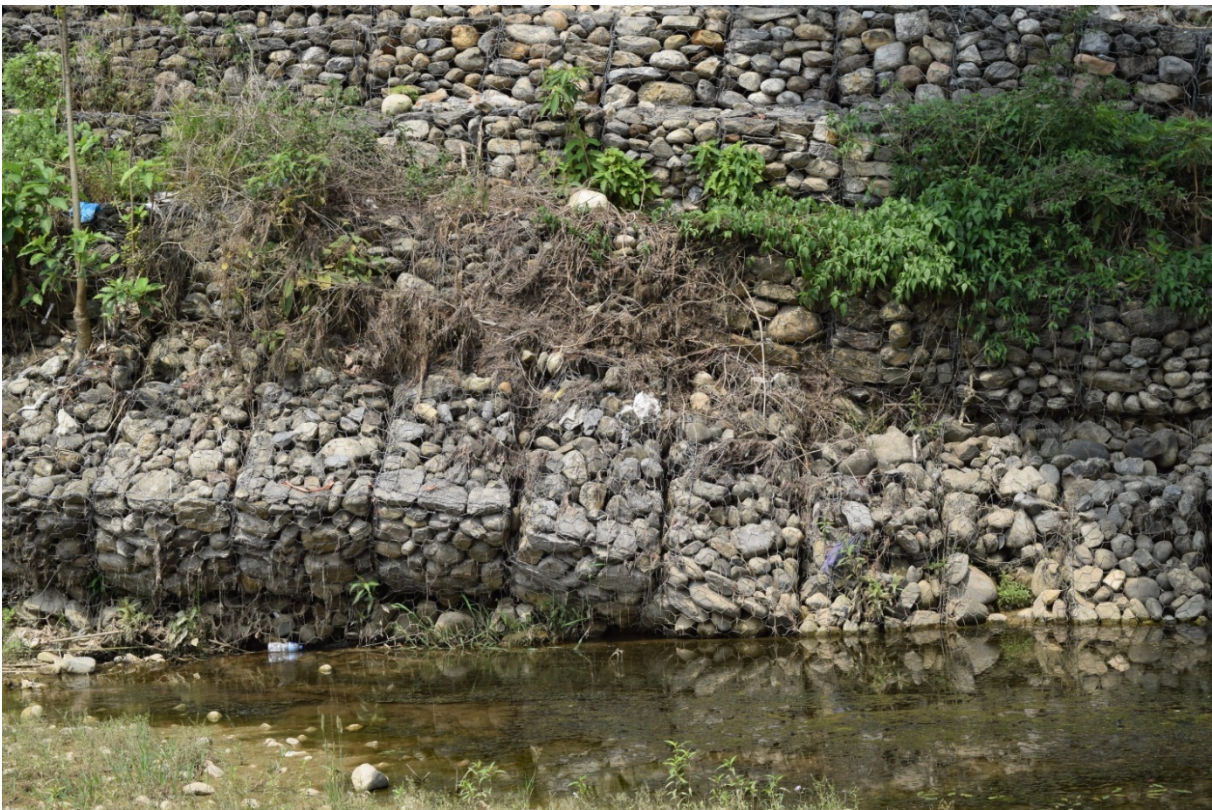
Figure 8-10 Collapse of gabion bank protection retaining wall along Madi Khola due to river bank erosion
