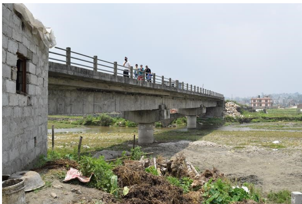
Figure 8-8 Manahara Bridge at Duwakot. This bridge performed well despite of several liquefaction induced sand boils evidenced near the bridge ( 27^{\circ}40'23.1''N , 85^{\circ}20'30.6''E & 27^{\circ}42'49.584''N 85^{\circ}24'42.26''E ).
