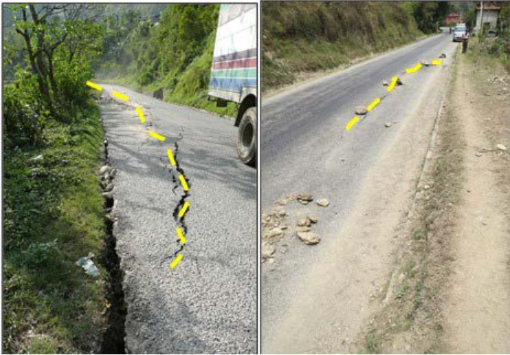
Figure 8-5 Lateral cracks observed on Blacktop roads.
