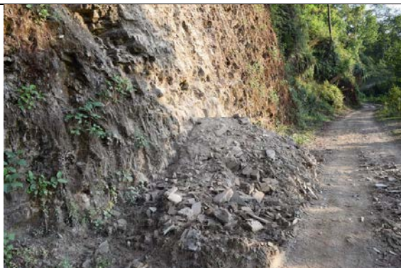
Figure 5-21 Typical rockfall observed along Lamosangu – Manthali Road
