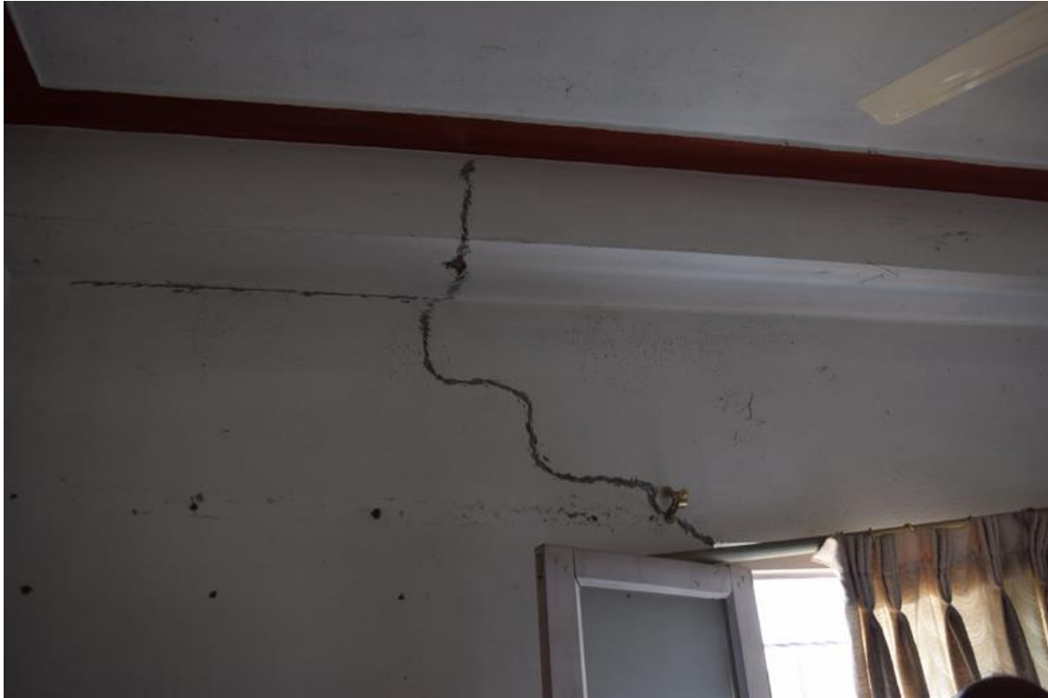
Figure 9-39 Structural damaged observed in a high school building at Pokhara.
