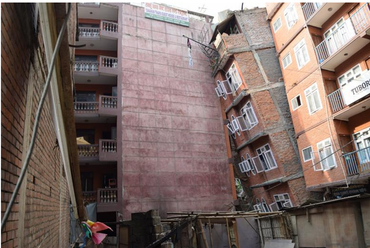
Figure 9-8 Soft story collapse of a six story building near Gogabu Bus Park. Three buildings were completely damaged in the neighborhood that killed over 20 people (27°44'06" N, 85°18'32" E).
