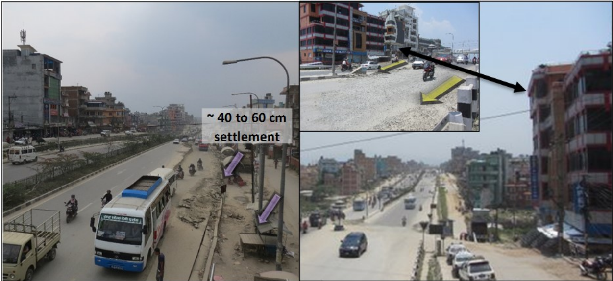
Figure 8-4 Road damage due to liquefaction induced ground failure in Arniko Highway in Lokanthali, 27°40'29.06"N 85°21'36.77"E.
