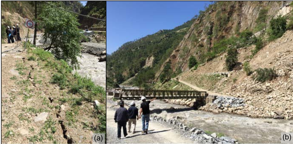
Figure 7-3 Tension cracks were observed along roads built on cut-fill slopes near the powerhouse access tunnel. Rockfall debris locally blocked access roads to this area, especially on steepened slopes. (a) 28^{\circ}14'23.91'' N, 85^{\circ}21'28.67'' E, (b) 28^{\circ}14'28.46'' N, 85^{\circ}21'30.18'' E
