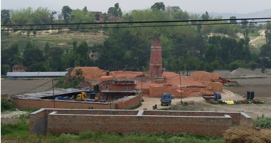
Figure 9-70 Damaged smokestack at a brick kiln in the Kathmandu Valley southeast of Bhaktapur (27° 29' 52.9" N, 85° 26' 52.9" E).
