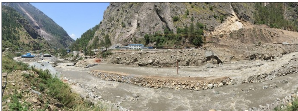
Figure 7-2 Site access roads, infrastructure and equipment including a crane in the Rasawugadhi headworks area were damaged by rockfalls. A temporary coffer dam was damaged by the rockfalls and then breached when flow of the river was diverted around the rockfall, directly toward the dam, causing overtopping and erosion (28°16'27.03" N, 85°22'41.59" E).
