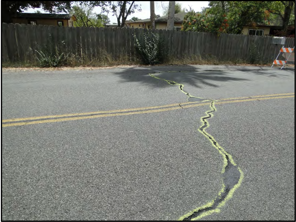
Figure 3: Photograph of cracking across Congress Valley Road in front of residence – looking southerly (Point B4) [NSF-GEER; Napa, CA; N 38.284 W 122.325; Harder, L. F.; 08/29/14]
