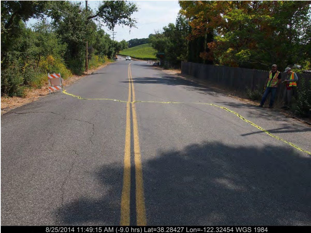
Figure 1. Photograph showing cracking in paved road surface perpendicular and parallel to NE-SW oriented Congress Valley Rd. [NSF-GEER; N38.2842, W122.3245; 08/25/14; 11:49 AM]
