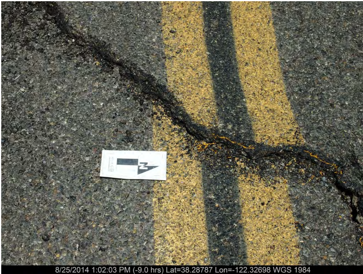
Figure 4. Photograph showing approximately 5 cm apparent right lateral separation of eastern margin of Thompson Ave. centerline. [NSF-GEER; N38.2878, W122.3269; 08/25/14; 1:02 PM]
