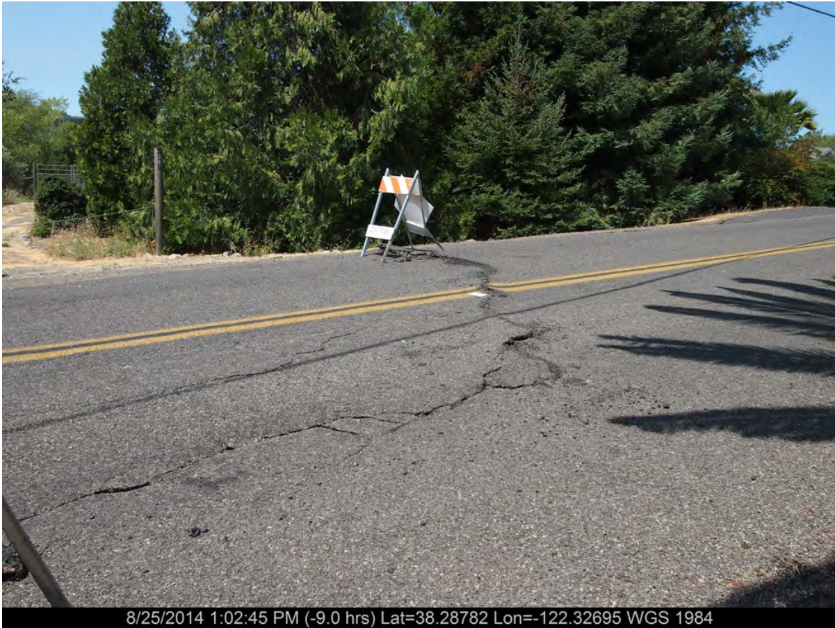
Figure 3. Photograph showing cracking in paved surface of N-S oriented Thompson Rd. [NSF-GEER; N38.2878, W122.3269; 08/25/14; 1:02 PM]
