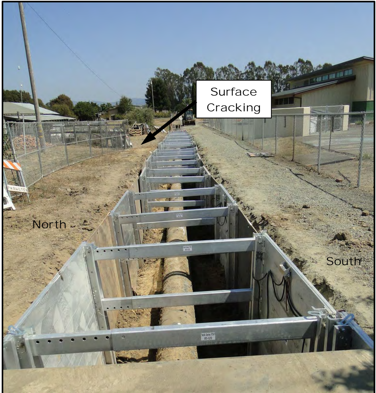
Figure 14: Photograph of excavated and shored PG&E natural gas pipeline crossing Los Carneros Road near Stone Bridge School (Point A12) – view looking towards the east towards alignment of ground cracking [NSF-GEER; Napa, CA; N 38.243 W 122.321; Harder, L. F.; 09/01/14]
