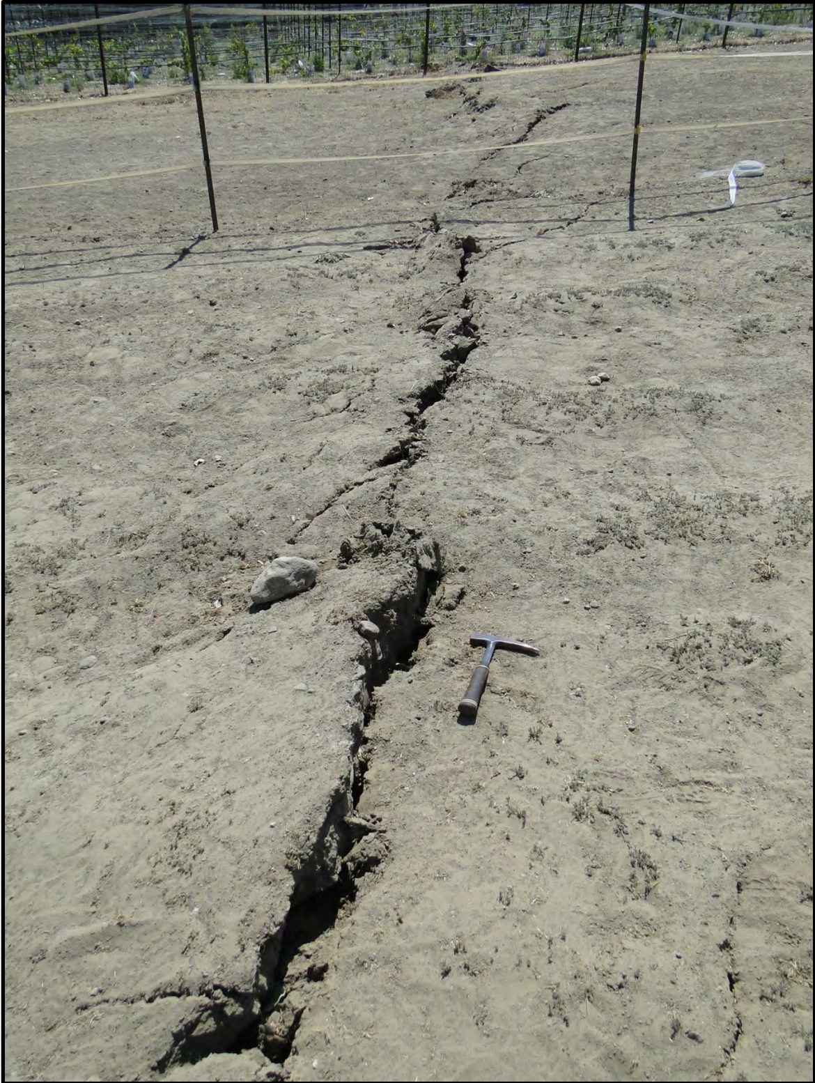
Figure 9: Photograph of linear ground cracking in horse pasture along Cuttings Wharf Road south of Highway 12/121 (Point A10) – view looking towards the southeast [NSF-GEER; Napa, CA; N 38.253 W 122.326; Harder, L. F.; 09/01/14]
