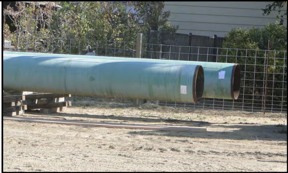
Figure 16: Close-up view of unwrapped/tested PG&E natural gas pipeline crossing Los Carneros Road near Stone Bridge School (Point A12) – note also photograph of replacement pipe on site waiting to be installed [NSF-GEER; Napa, CA; N 38.243 W 122.321; Harder, L. F.; 09/07/14]
