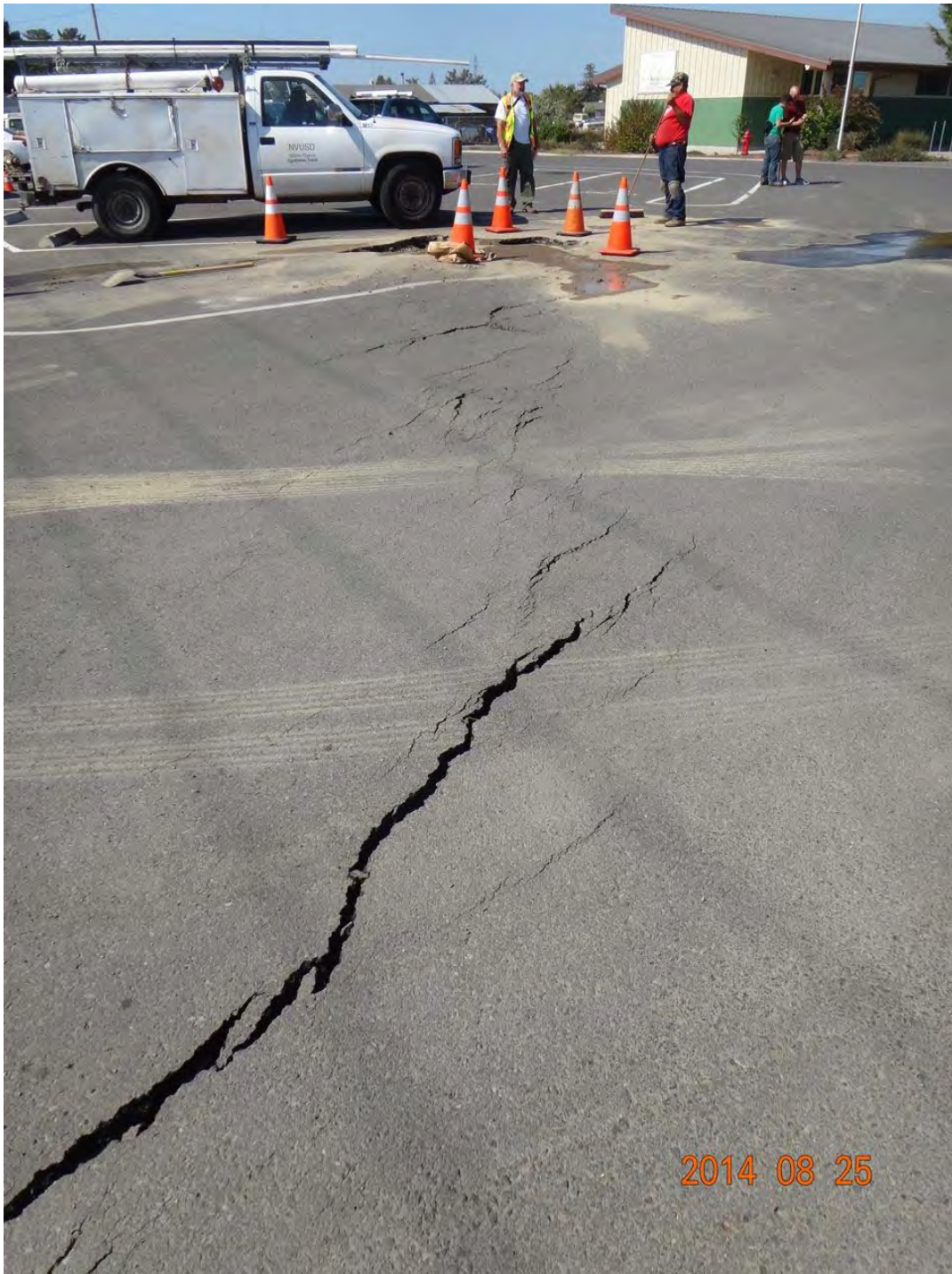
Figure 4. Surface fault rupture at Stone Bridge School (2.7 km NW of epicenter), showing left-stepping pattern of transtensional cracking within asphalt parking lot. View to north-northwest. Overall fault zone strikes 340, cracks strike about 020 to 040. [NSF-GEER; GPS N38.2436 W122.3212; 08/25/14: 3:38 pm]
