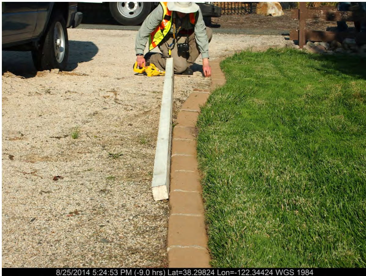
Figure 6. Photograph showing right lateral displacement of aligned bricks at southern margin of crushed granite driveway on Leaning Oak Rd. Measured a maximum of 1.1ft (appx.33) cm of right-lateral displacement. [NSF-GEER; N38.2982, W122.3442; 08/25/14; 4:26 PM]
