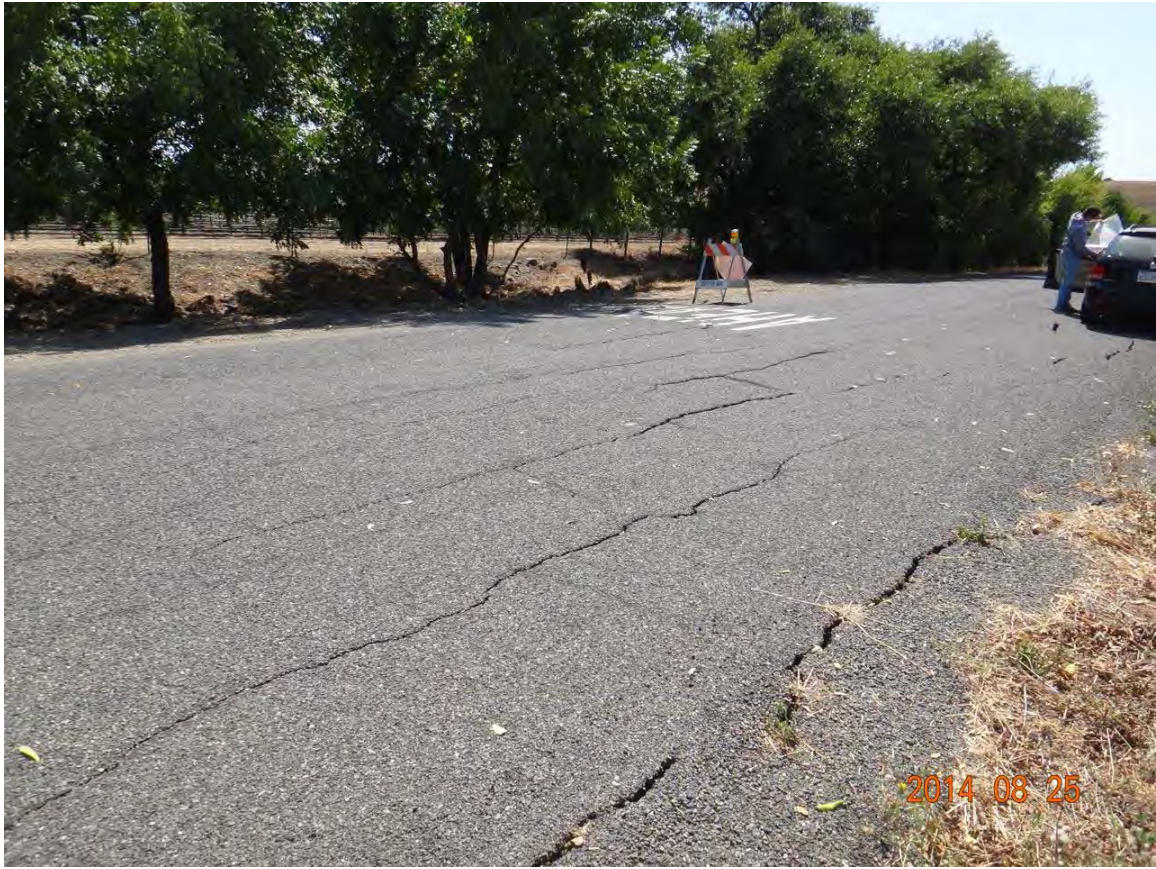
Figure 9. Surface fault rupture at Henry Road (6.2 km NW of epicenter), showing left-stepping pattern of transtensional cracking across asphalt. View to southeast. Offset across most prominent crack within this zone is as much as 6 cm, but offset across entire zone measure in adjacent vineyard is about 40 cm [NSF-GEER; GPS N38.2732 W122.3366; 08/25/14: 1:45 pm]
