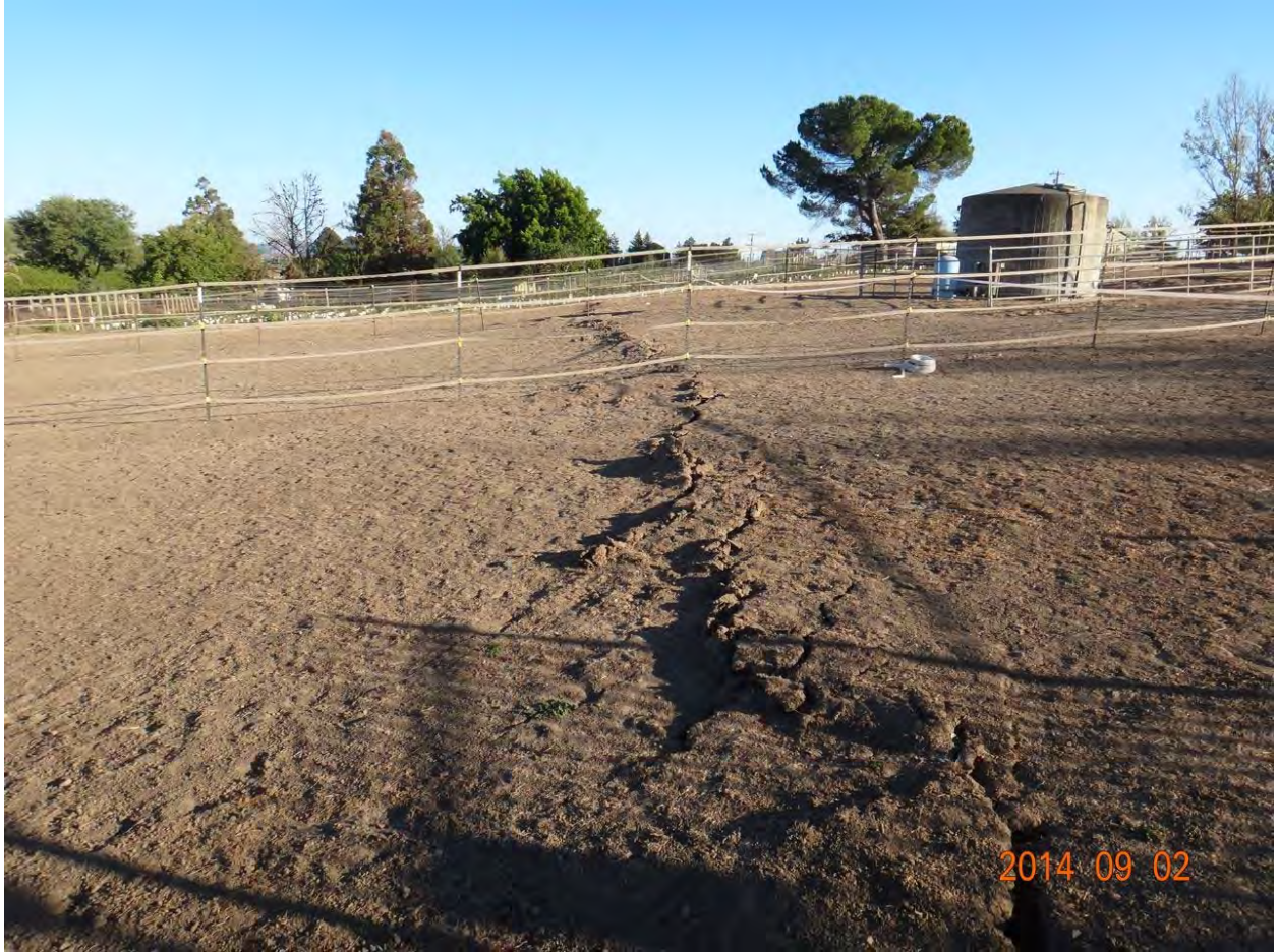
Figure 6. Surface fault rupture at horse corral west of Cuttings Wharf Road (3.9 km NW of epicenter), showing left-stepping pattern of transtensional cracking across compacted dirt slope. View to south-southeast. Individual cracks have as much as 5 cm lateral offset. [NSF-GEER; GPS N38.2536 W122.3262; 09/02/14: 6:07 pm]
