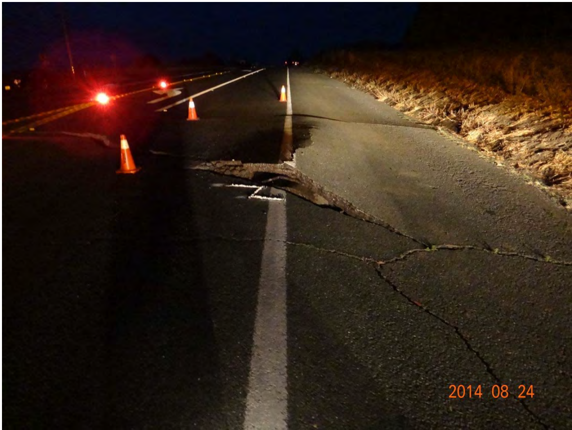
Figure 19. Surface fault rupture at Highway 12 (4.2 km NW of epicenter), showing buckling of asphalt on northern margin and minor lateral offset. Taken at 0554 local time, this photograph precedes road repairs. [NSF-GEER; GPS N38.256 W122.327; 08/24/14: 5:54 am]
