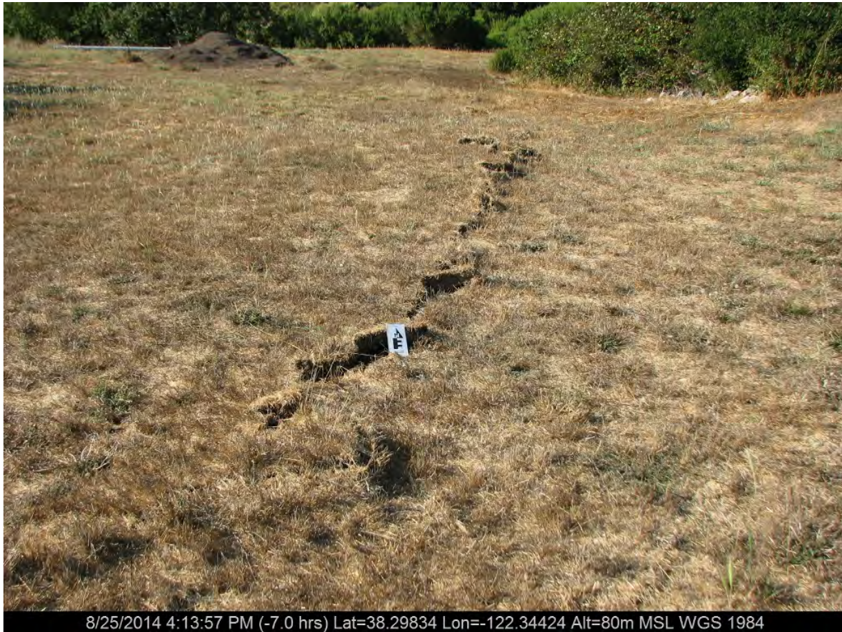
Figure 5: Photograph showing linear deformation of ground surface in natural ground surface / graded lot as linear mole track. Deformation apparently confined to zone appx.1-2 m wide and extends appx.50-60 m. [NSF-GEER; N38.2983, W122.3442; 08/25/14; 4:13 PM]
