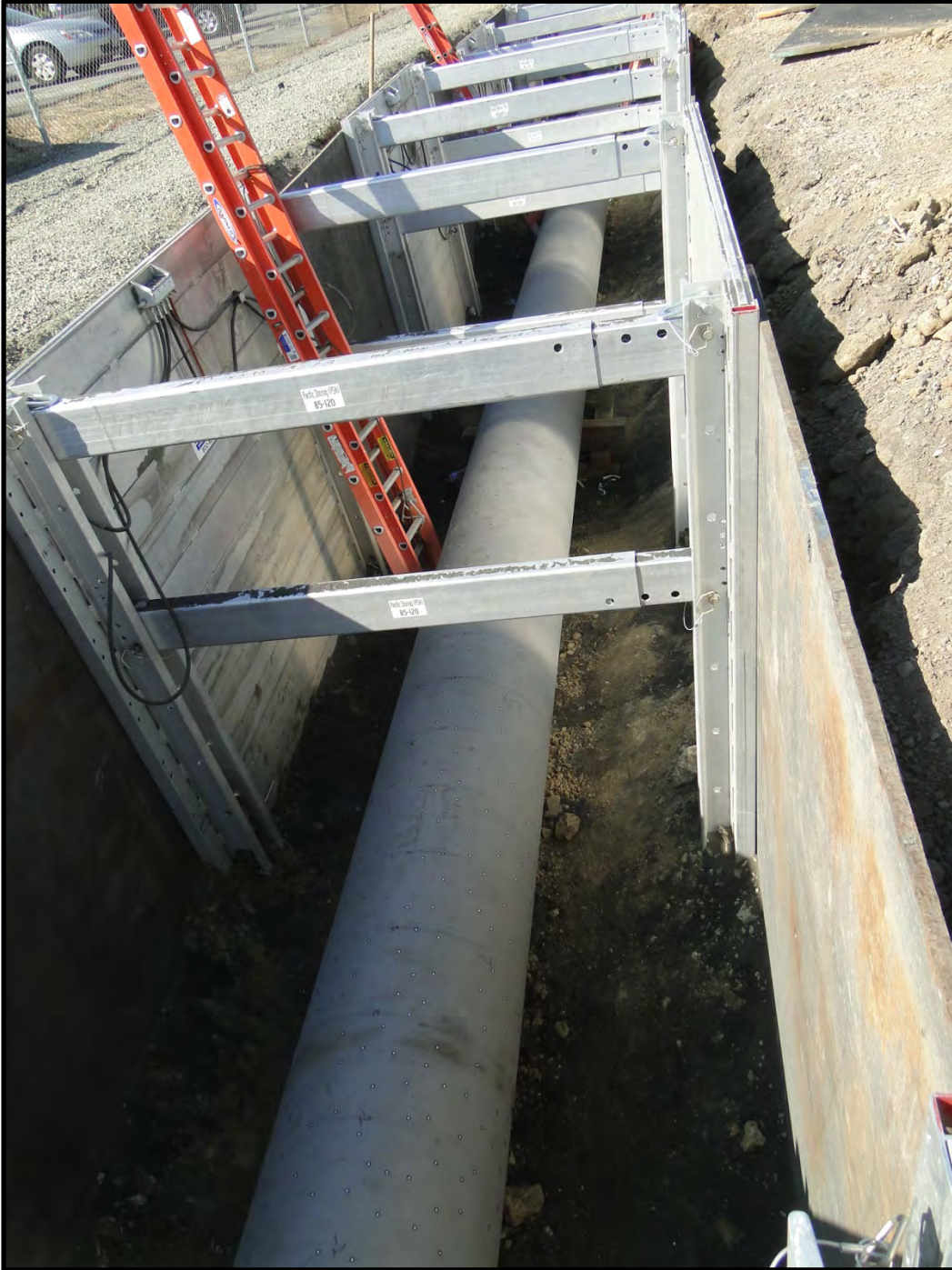
Figure 15: Photograph of unwrapped/tested PG&E natural gas pipeline crossing Los Carneros Road near Stone Bridge School (Point A12) – view looking towards the west [NSF-GEER; Napa, CA; N 38.243 W 122.321; Harder, L. F.; 09/07/14]
