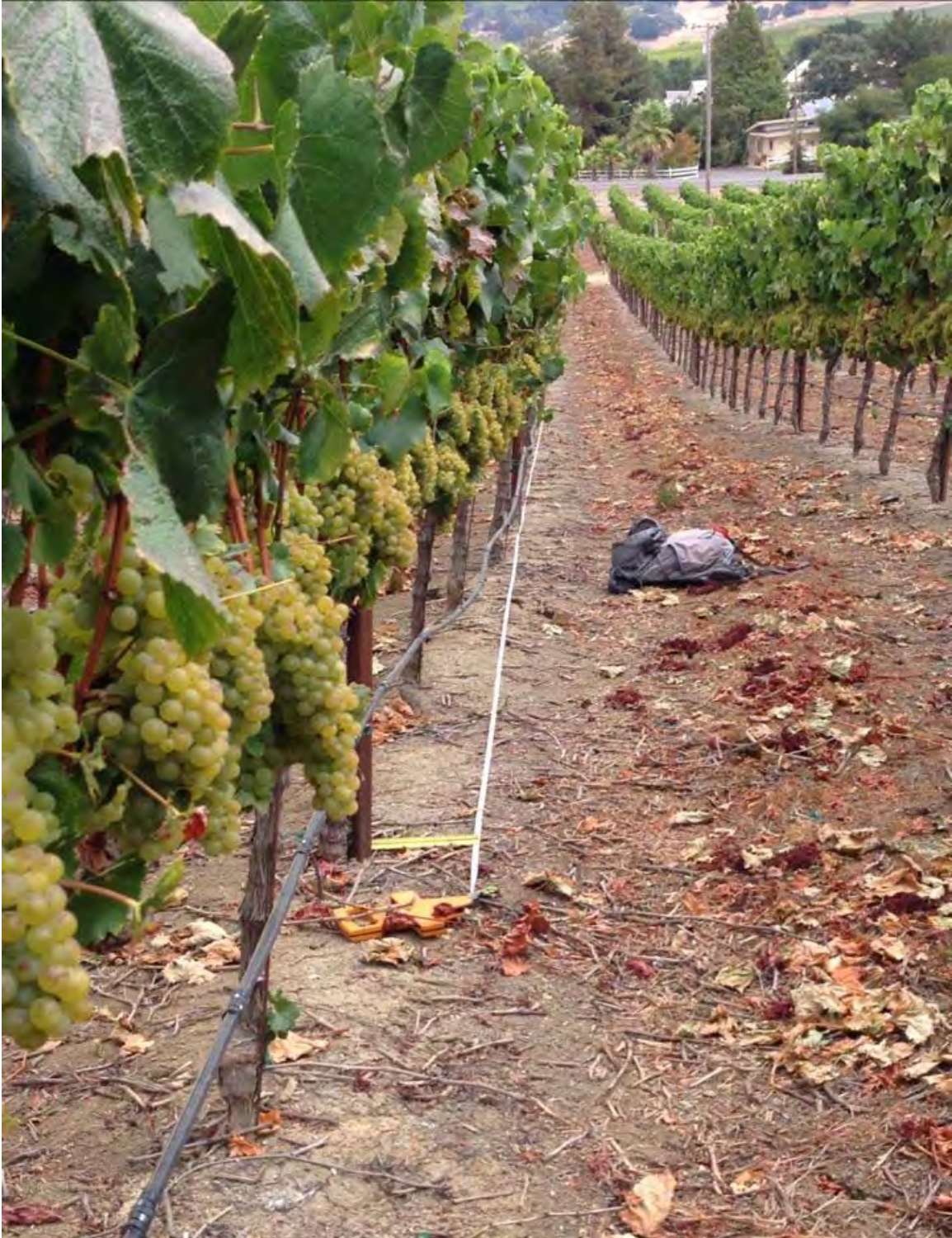
Figure 15. Surface fault rupture at southern part of Clos du Val Vineyard near Old Sonoma Road (5.6 km NW of epicenter), showing measurement alignment along azimuth 058. Yellow engineer's scale is located west of fault zone, showing 20 to 25 cm of apparent lateral offset. Tape was aligned at base of metal stakes east of fault zone. [NSF-GEER; GPS N38.2669 W122.3341; 08/25/14: 11:19 am].
