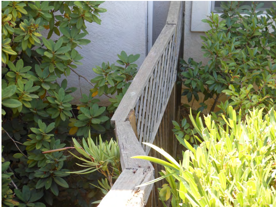
Figure C-H03-5: Fence buckled in compression. [NSF-GEER; N 38.3131 W 122.3431; 08/28/14]
