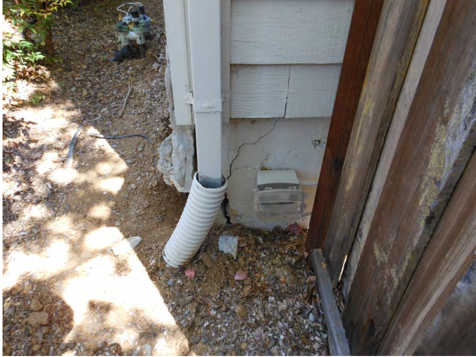
Figure C-H04-4: Cracked foundation. [NSF-GEER; N 38.3128 W 122.3431; 08/28/14]
