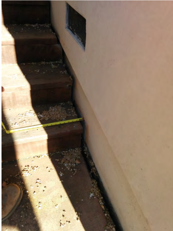
Figure C-H06-3: Staircase displaced from structure. [NSF-GEER; N 38.3124 W 122.3431; 08/28/14]
