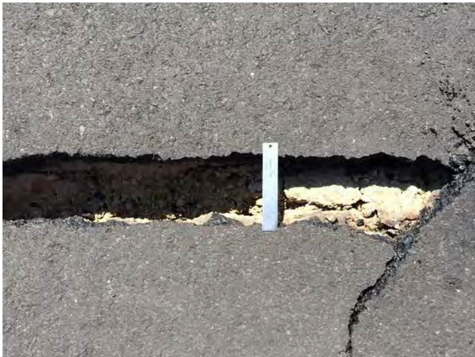
Figure C-P1-4: Asphalt fracture [NSF-GEER; N 38.3017 W 122.3440; 08/25/14 11:33]
