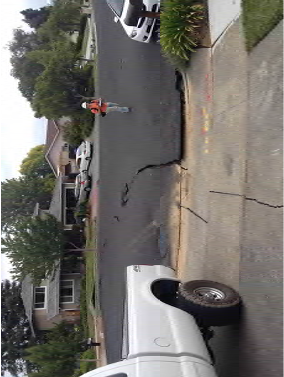
Figure C-P1-2: General view of fracturing [NSF-GEER; N 38.3016 W 122.3441; 08/25/14 10:24]
