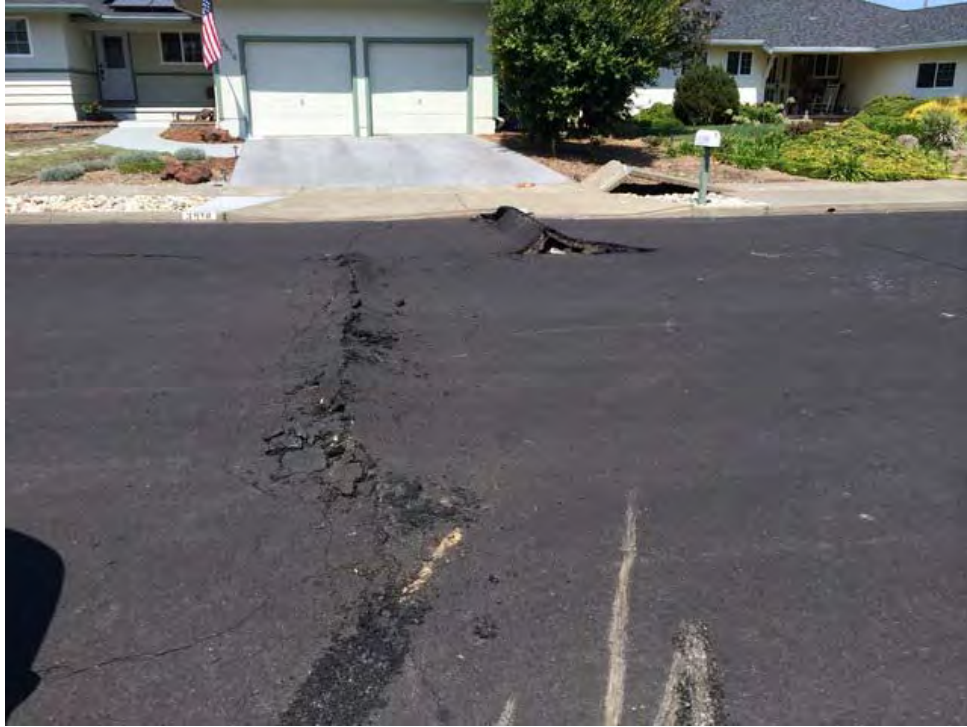
Figure C-P2-2: General view of fracturing [NSF-GEER; N 38.3038 W 122.3441; 08/25/14 13:18]
