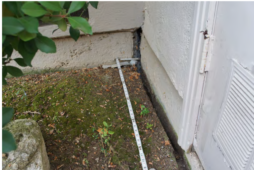
Figure C-H31-3: Structure shifted on foundation and foundation crack [NSF-GEER; N 38.3027 W 122.3436; 08/25/14 10:22]
