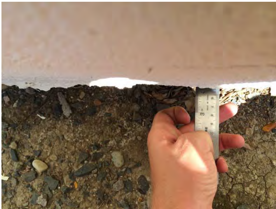
Figure C-H24-4: Offset of wall frame relative to foundation (view from top) [NSF-GEER; N 38.3040 W 122.3431; 08/25/14 14:15]
