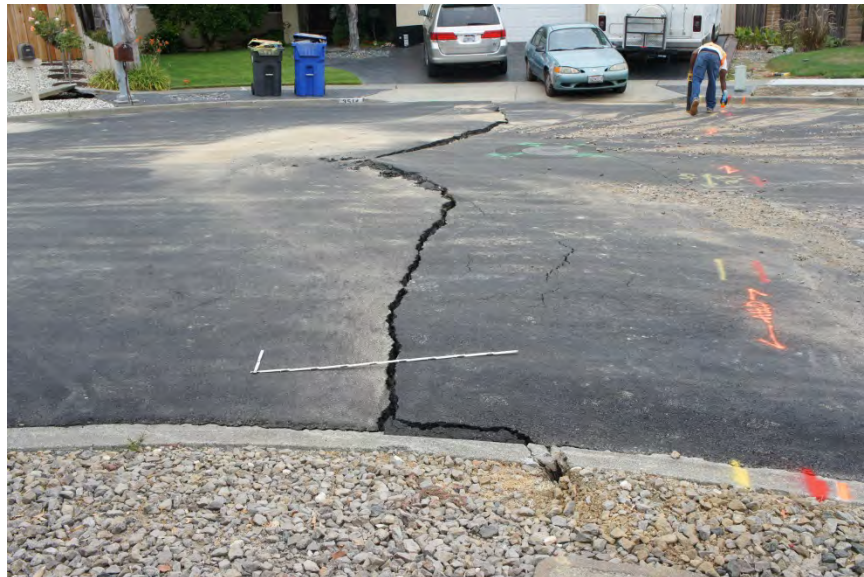
Figure C-H30-3: Severe cracking across White Cliff Circ. [NSF-GEER; N 38.3029 W 122.3435; 08/25/14 09:17]
