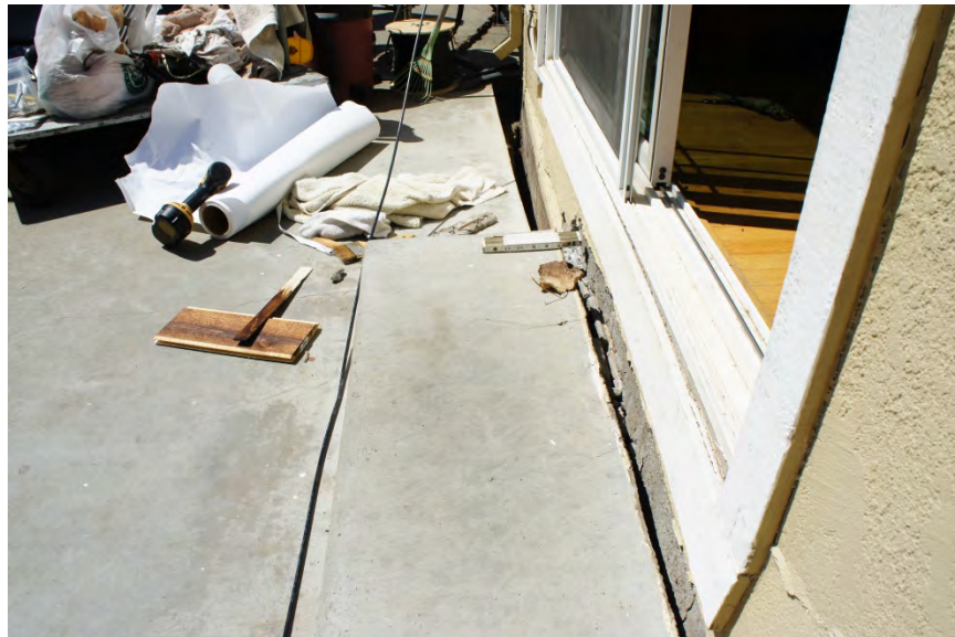
Figure C-H27-3: Gap between structure and patio. [NSF-GEER; N 38.3036 W 122.3432; 08/25/14 13:28]
