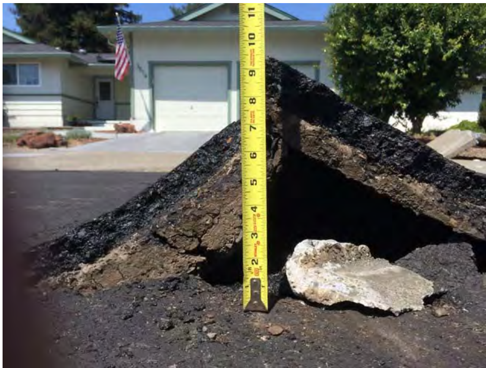
Figure C-P2-3: Asphalt buckling from end [NSF-GEER; N 38.3038 W 122.3430; 08/25/14 13:20]
