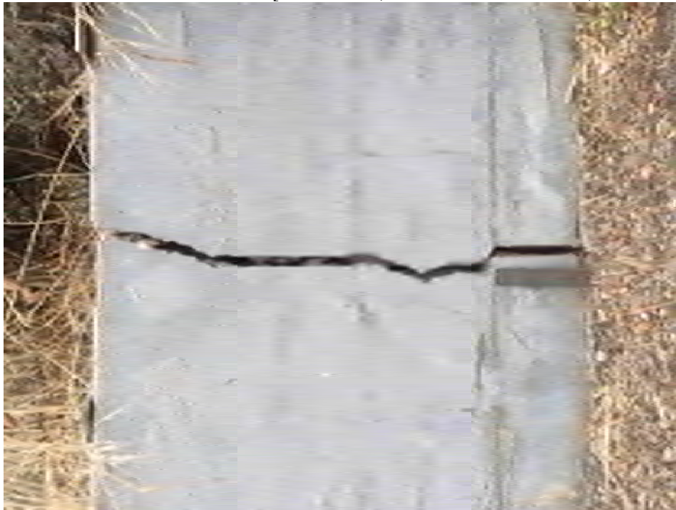
Figure C-H35-4: Retaining wall crack [NSF-GEER; N 38.3015 W 122.3440; 08/25/14 10:58]
