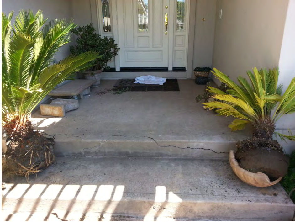
Figure C-H02-2: East looking view of crack extending through walkway and garage. [NSF-GEER; N 38.3133 W 122.3431; 08/28/14 12:46]
