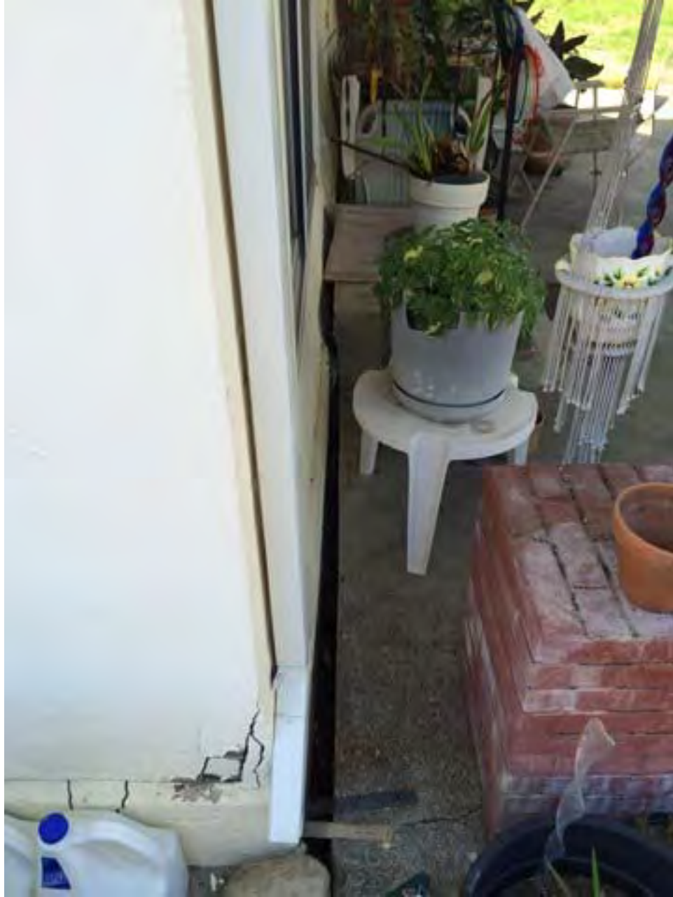
Figure C-H24-2: Displacement of patio slab relative to structure foundation; cracking of corner [NSF-GEER; N 38.3041 W 122.3429; 08/25/14 13:18]
