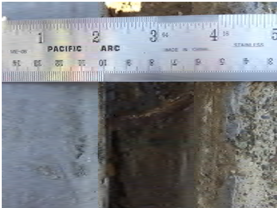
Figure C-H25-3: Deformation of rebar between driveway and sidewalk [NSF-GEER; N 38.3038 W 122.3430; 08/25/14 13:29]
