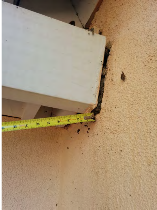
Figure C-H01-2: Roof Beam separated from wall due to shearing. [NSF-GEER; N 38.3135 W 122.3431; 08/28/14 17:08]
