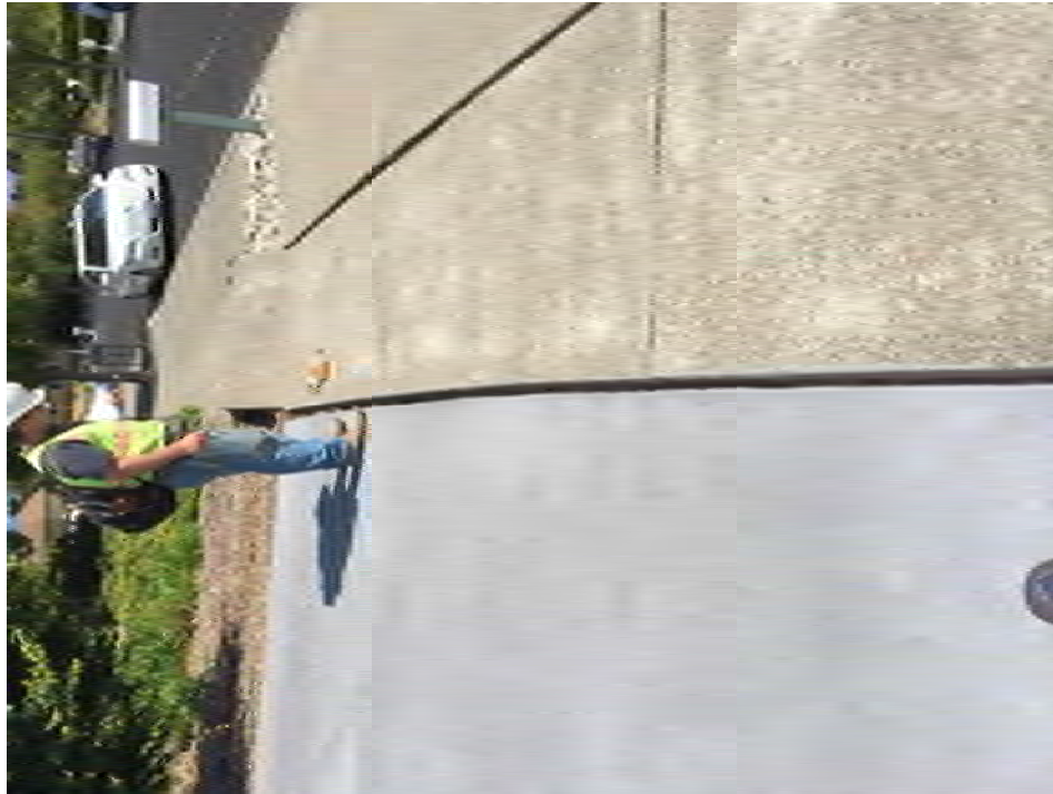
Figure C-H25-2: Offset of driveway, sidewalk and driveway bib [NSF-GEER; N 38.3038 W 122.3431; 08/25/14 13:29]
