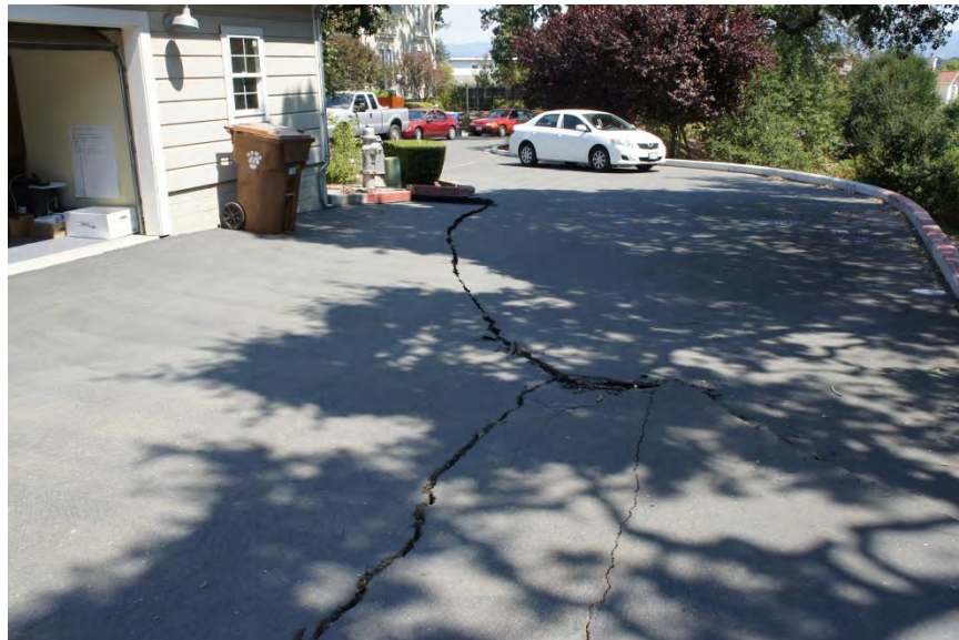
Figure C-H37-3: Open cracks in pavement [NSF-GEER; N 38.3011 W 122.3442; 08/25/14 11:36]
