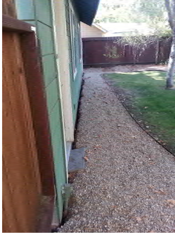
Figure C-H21-2: Open fissure along detached garage causing settlement to the right (West) [NSF-GEER; N 38.3052 W 122.3369; 08/28/14, 10:09]
