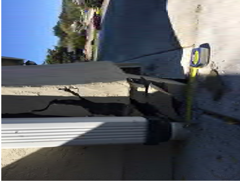
Figure C-H32-4: Damage to strip footing at garage corner [NSF-GEER; N 38.3023 W 122.3438; 08/27/14 11:47]
