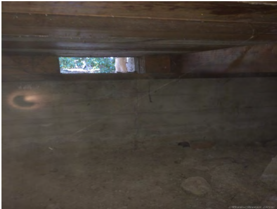
Figure C-H15-3: Crack in the perimeter foundation wall [NSF-GEER; N 38.3066 W 122.3427; 08/31/14 10:02]
