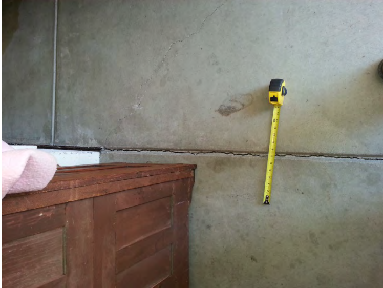
Figure C-H05-2: Cracked slab foundation in garage. [NSF-GEER; N 38.3126 W 122.3431; 08/28/14, 15:20]
