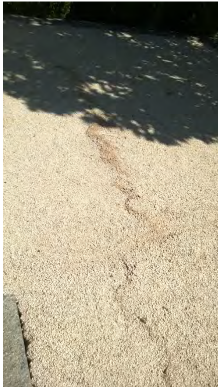
Figure C-H04-3: Compression ridge in gravel above wall. [NSF-GEER; N 38.3128 W 122.3431; 08/28/14, 14:40]
