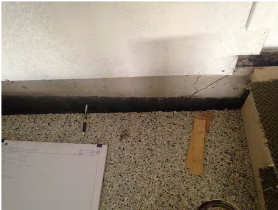
Figure C-H32-3: Separation of garage slab and wall [NSF-GEER; N 38.3022 W 122.3438; 08/27/14 11:33]
