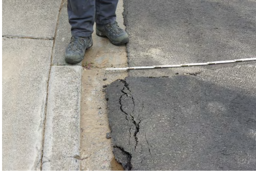
Figure C-H28-H29-2: Compression between asphalt and curb showing right lateral movement. [NSF-GEER; N 38.3033 W 122.3434; 08/25/14 09:29]
