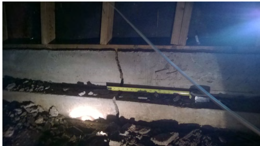
Figure C-H21-3: Strip footing crack and tilted cripple wall (E-W) [NSF-GEER; N 38.3052 W 122.3369; 08/28/14, 10:15]
