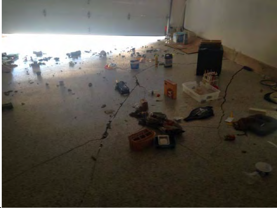
Figure C-H32-2: Garage slab cracking [NSF-GEER; N 38.3024 W 122.3436; 08/27/14 11:33]
