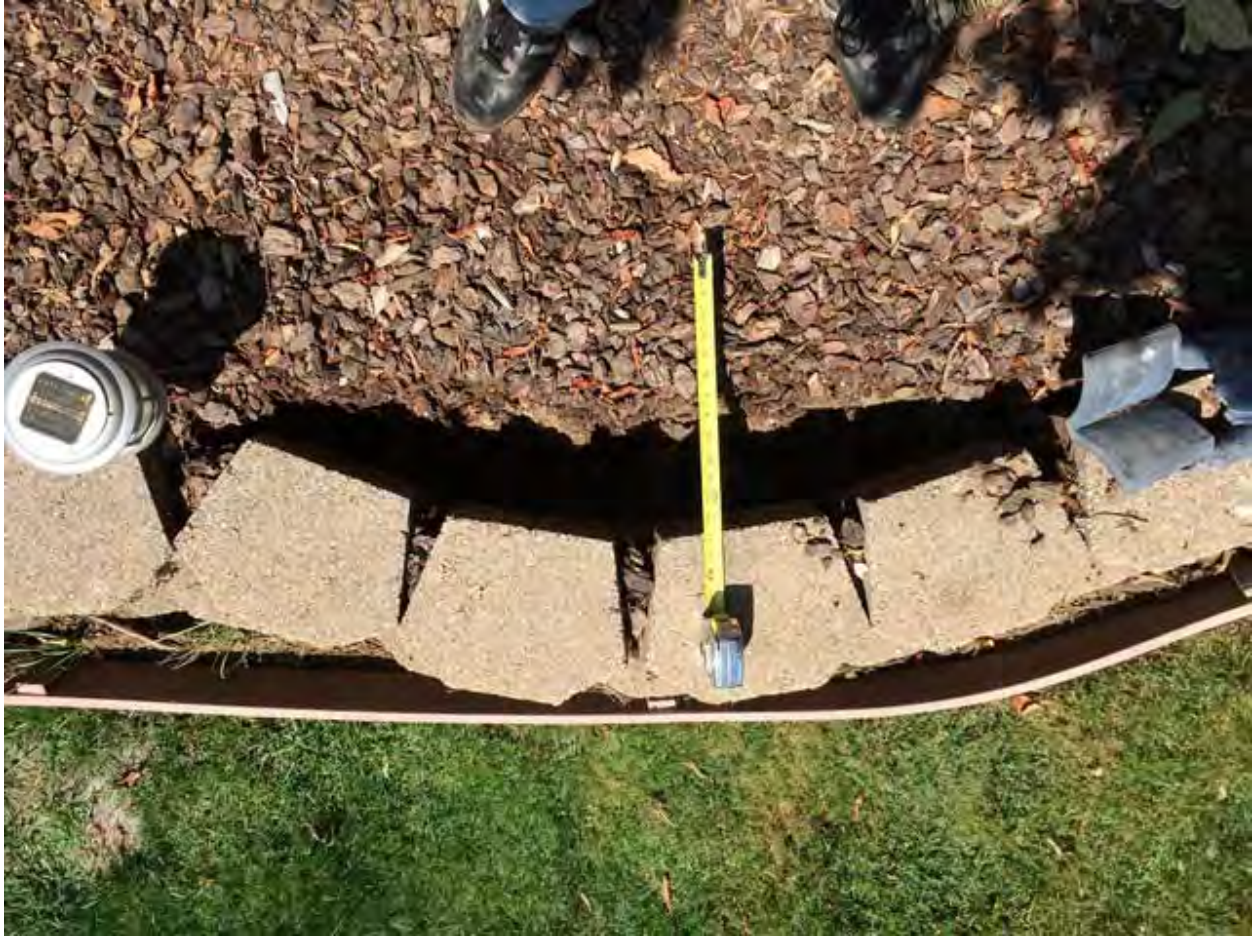
Figure C-H36-2: Buckled retaining wall [NSF-GEER; N 38.3013 W 122.3441; 08/25/14 11:57]
