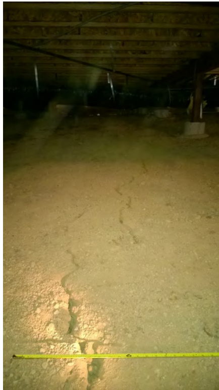
Figure C-H04-5: Soil fissure in basement. [NSF-GEER; N 38.3128 W 122.3431; 08/28/14, 12:08]
