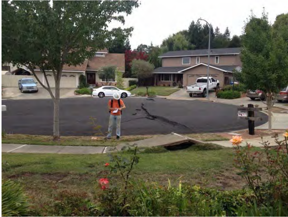
Figure C-P1-3: General view of fracturing [NSF-GEER; N 38.3018 W 122.3437; 08/25/14 10:42]
