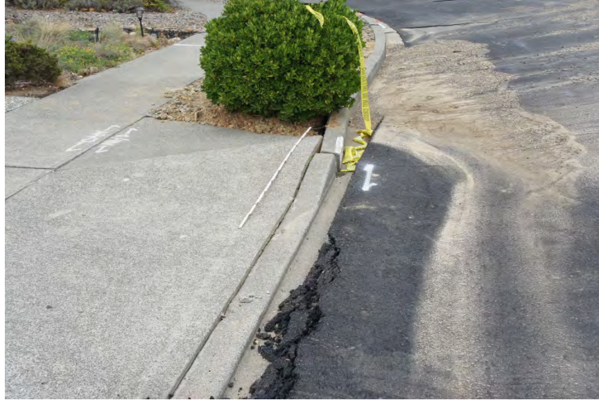
Figure C-H30-2: Compression between asphalt and curb showing. [NSF-GEER; N 38.3029 W 122.3435; 08/25/14 09:15]
