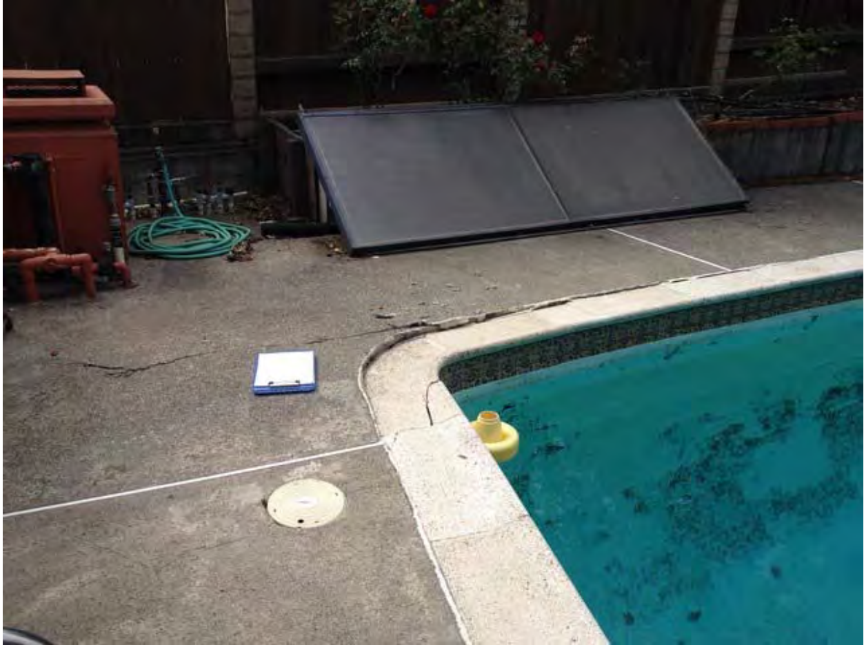
Figure C-H34-2: Concrete cracking at edge of pool
