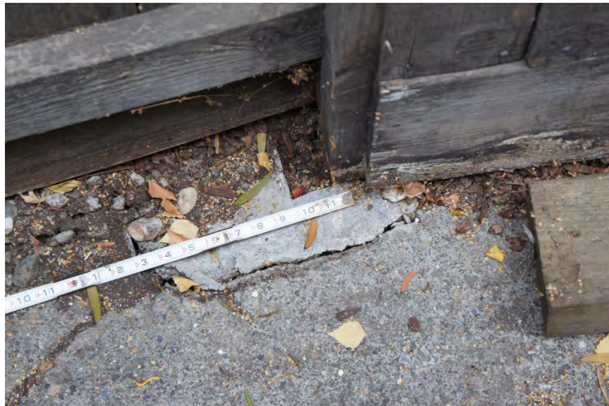
Figure C-H28-H29-3: Buckling of wooden fence showing post displacement [NSF-GEER; N 38.3033 W 122.3434; 08/25/14 09:52]
