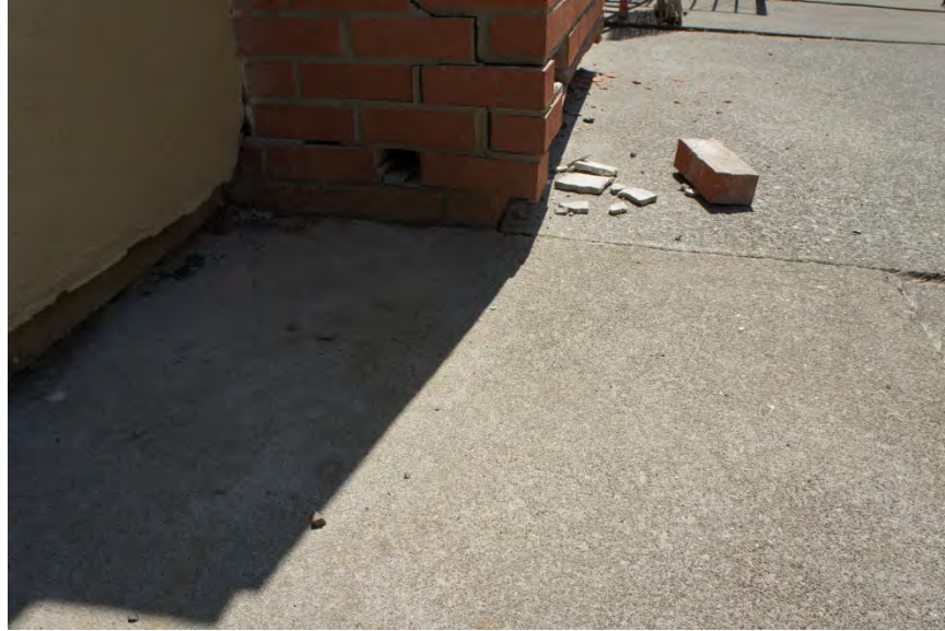
Figure C-H27-2: Structure shifted off of foundation. [NSF-GEER; N 38.3036 W 122.3432; 08/25/14 13:15]
