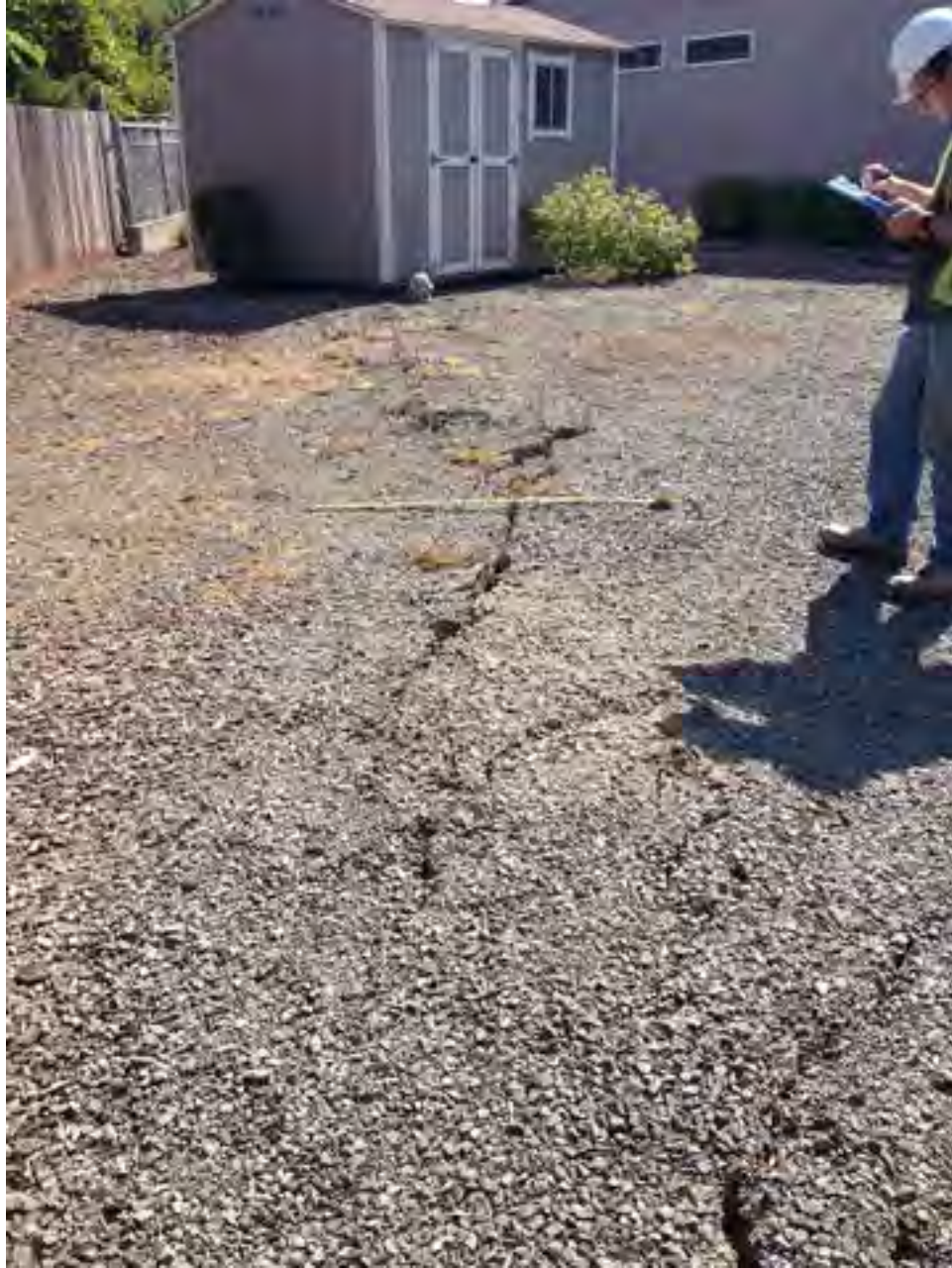
Figure C-H23-2: Ground surface rupture in side-yard [NSF-GEER; N 38.3045 W 122.3427; 08/25/14 15:24]
