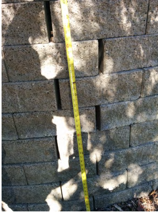
Figure C-H04-2: Displaced masonry wall. [NSF-GEER; N 38.3128 W 122.3431; 08/28/14, 16:32]
