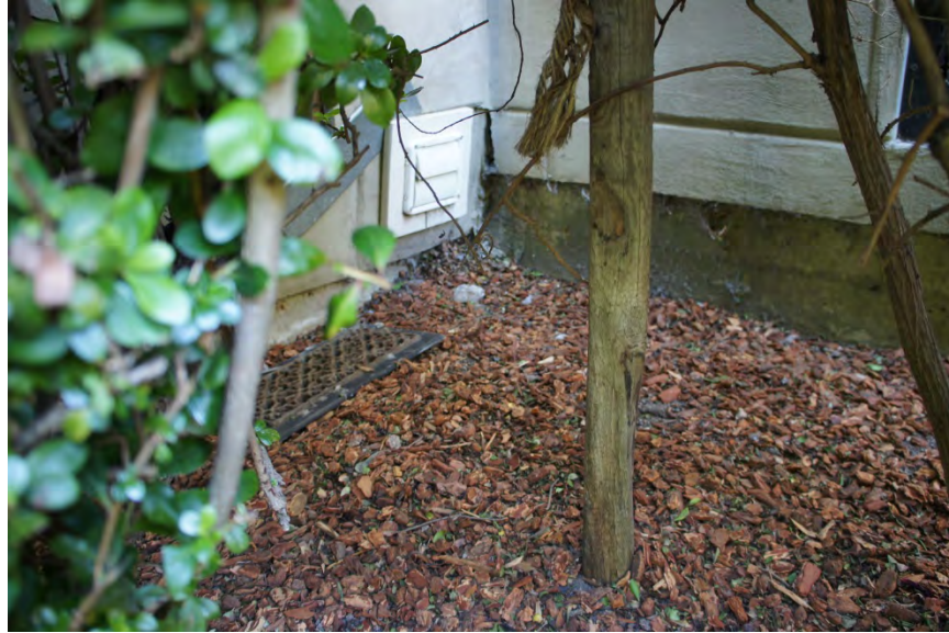
Figure C-H37-2: Cracked and settling strip footing [NSF-GEER; N 38.3011 W 122.3442; 08/25/14 11:41]
