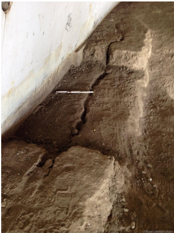
Figure E.35: Crack parallel to the River in North abutment of Soscol Bridge [NSF-GEER; N 38.2997 W -122.283; 08/24/14 13:09]
