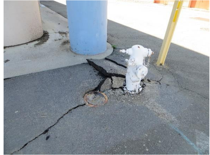
Figure E.15: Pavement damage at hydrant [NSF-GEER; GPS N38.098 W122.269; 08/24/14; 14:37]
