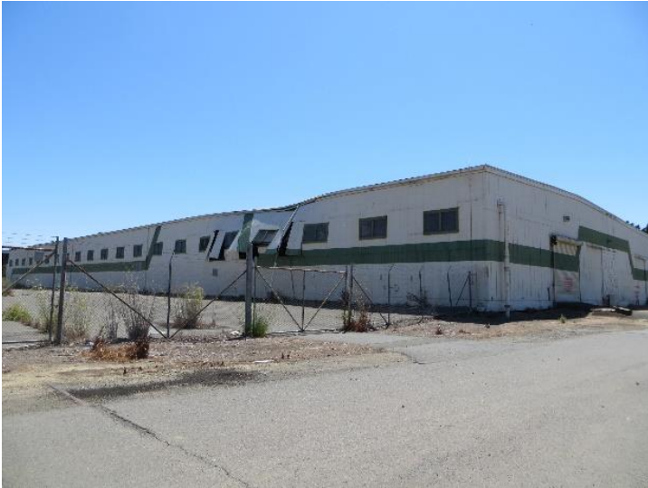
Figure E.6: Corrugated siding damage [NSF-GEER; GPS N38.111 W122.282; 08/24/14; 13:53]
