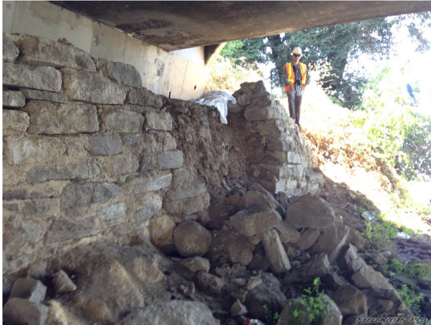
Figure E.34: Failure of the stone retaining wall in South abutment of Soscol Bridge [NSF-GEER; N 38.2994 W -122.282; 08/24/14 13:44]
