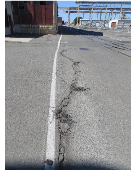
Figure E.13: Possible earthquake damage [NSF-GEER; GPS N38.098 W122.269; 08/24/14; 14:37]
