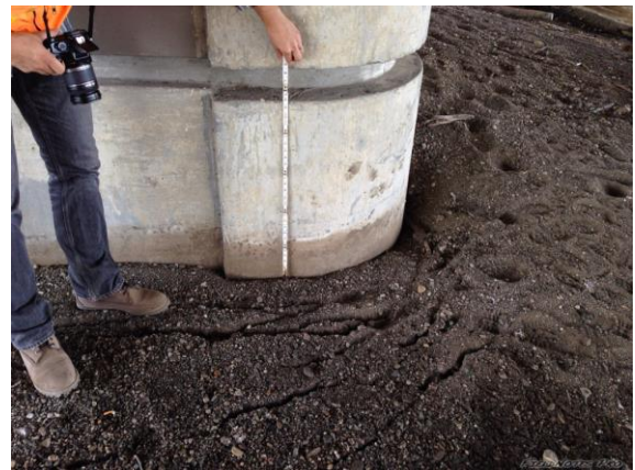
Figure E.40: Ground cracking and settlement due to liquefaction in Napa River point bar below 3 rd St. Bridge [NSF-GEER; N 38.2980 W -122.2840; 08/24/14 14:44]
