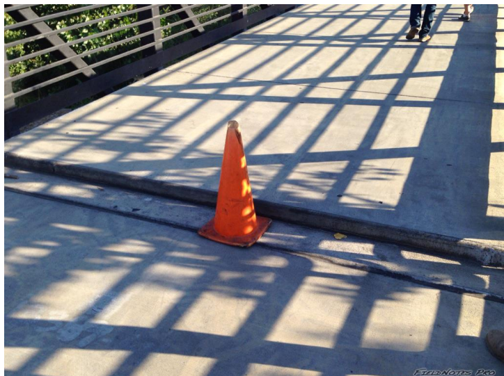
Figure E.44: Step between bridge's deck and access ramp in North abutment. [NSF-GEER; N 38.3003 W -122.2881; 08/24/14 17:58]
