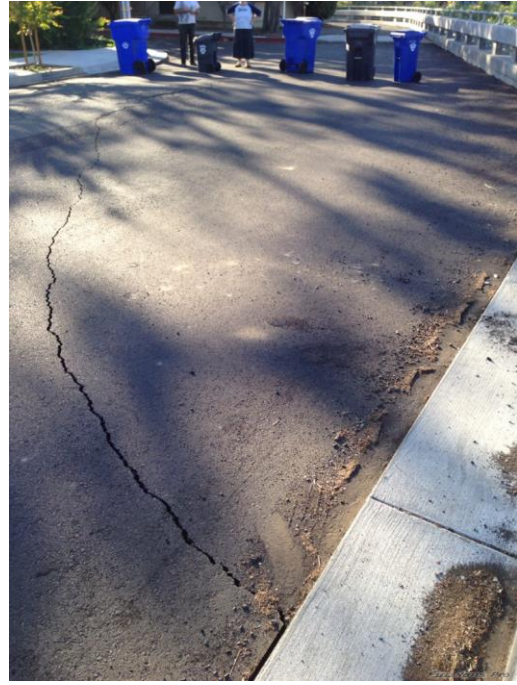
Figure E.42: Crack in pavement behind the retaining wall in the Pedestrian Bridge [NSF-GEER; N 38.3003 W -122.2881; 08/24/14 17:58]
