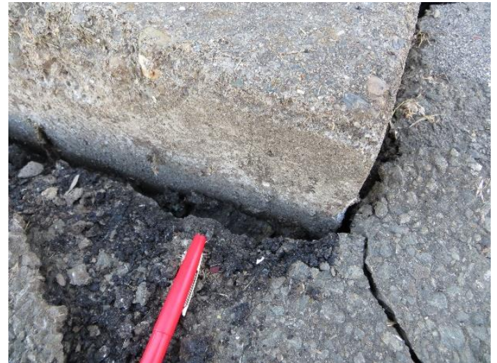
Figure E.17: Pavement damage at concrete corner [NSF-GEER; GPS N38.098 W122.269; 08/24/14; 14:38]
