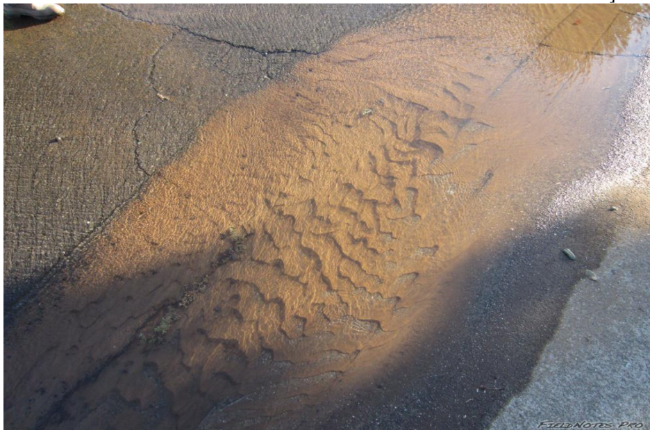
Figure E.28: Water break at Arroyo Dr. (Downtown Napa). Soil below asphalt ejected by water. [NSF-GEER; N 38.3008 W -122.289; 08/25/14 18:34]
