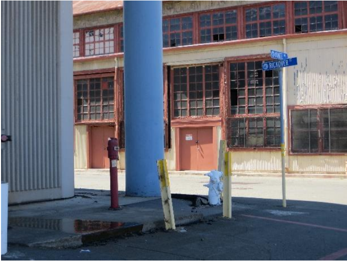
Figure E.14: Pavement damage at hydrant [NSF-GEER; GPS N38.098 W122.269; 08/24/14; 14:39]
