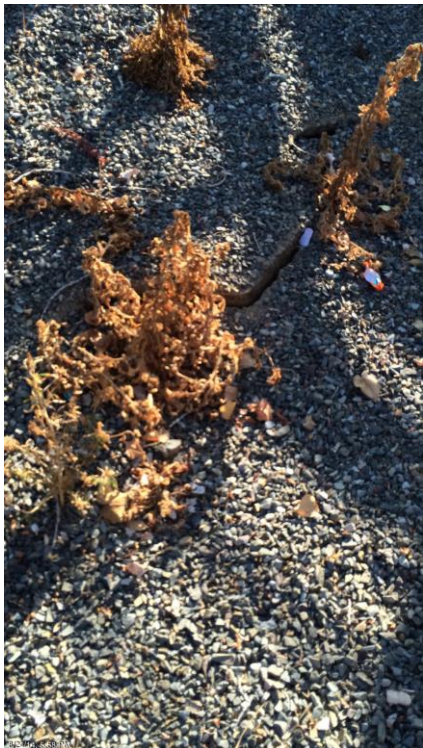
Figure E.43: Crack along sheet pile wall behind the retaining wall in the Pedestrian Bridge [NSF-GEER; N 38.3003 W -122.2881; 08/24/14 17:58]
