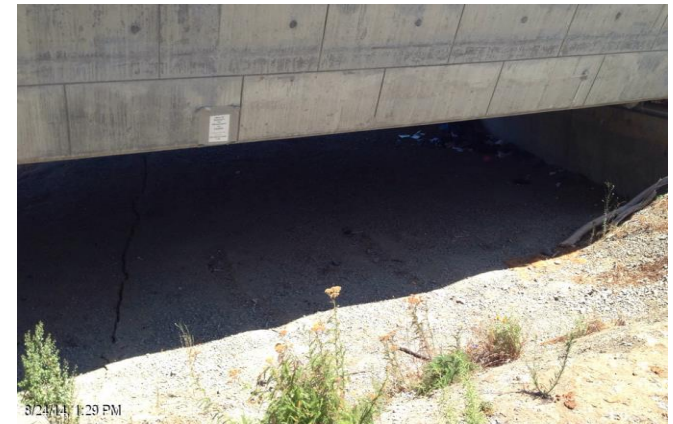
Figure E.33: Railroad Bridge. Crack observed in the interface between the South abutment foundation and the soil. [NSF-GEER; N 38.2995 W -122.2821; 08/25/14 13:28]
