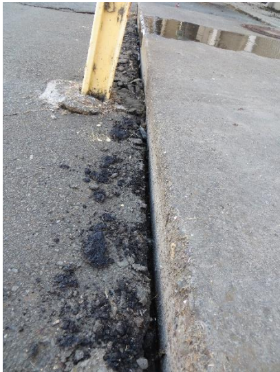
Figure E.16: Pavement damage along concrete [NSF-GEER; GPS N38.098 W122.269; 08/24/14; 14:38]
