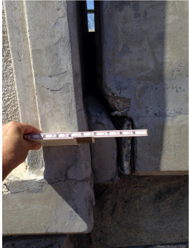
Figure E.36: Movement of the deck in 3rd St. Bridge East abutment [NSF-GEER; N 38.2981 W -122.284; 08/24/14 14:44]
