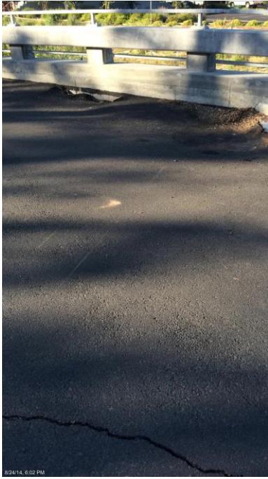
Figure E.41: Settlement of backfill near the retaining wall in the Pedestrian Bridge [NSF-GEER; N 38.3003 W -122.2881; 08/24/14 17:58]
