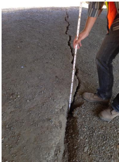
Figure E.31: Railroad Bridge. Crack observed in the interface between the North abutment foundation and the soil. [NSF-GEER; N 38.3002 W -122.282; 08/25/14 12:41]
