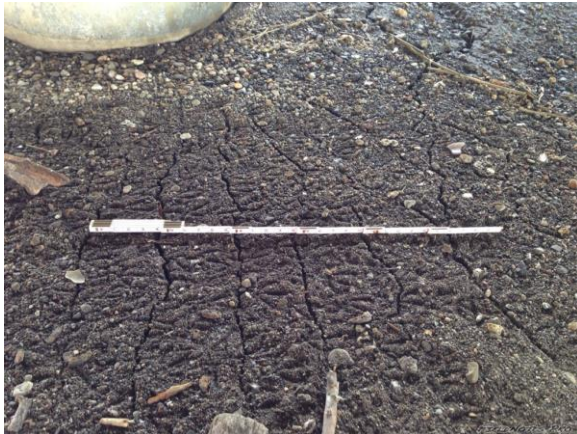
Figure E.39: Ground cracking due to liquefaction in Napa River point bar below 3 rd St. Bridge, between the two columns of the eastern pier. [NSF-GEER; N 38.2980 W -122.2840; 08/24/14 14:44]
