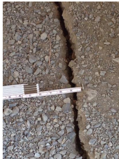
Figure E.32: Railroad Bridge. Crack observed in the interface between the South abutment foundation and the soil. [NSF-GEER; N 38.2995 W -122.2821; 08/25/14 13:28]
