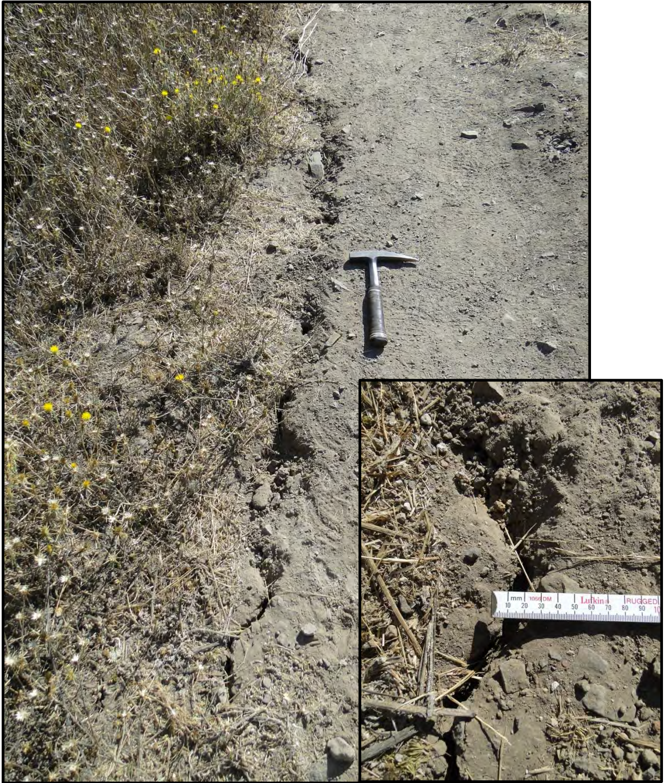
Figure F-4: Photograph of cracking on the upstream edge of the crest of Lake Marie Dam looking southeast [NSF-GEER; Napa, CA; N38.260 W 122.230; Harder, L. F.; 09/01/14]
