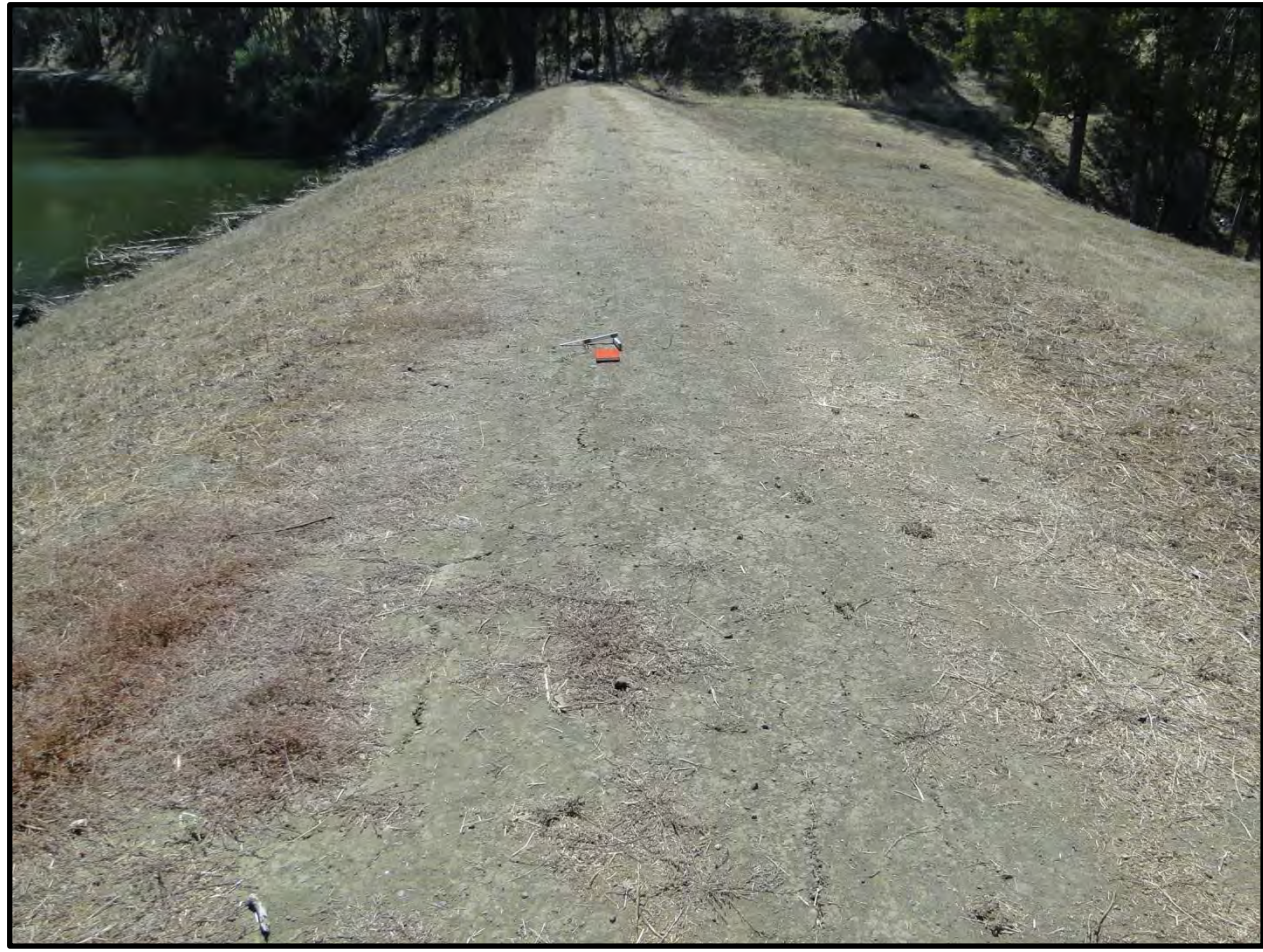
Figure F-6: Photograph of minor longitudinal cracking on the crest of Lake Chabot Dam looking southeast [NSF-GEER; Napa, CA; N38.141 W 122.241; Harder, L. F.; 08/27/14]
