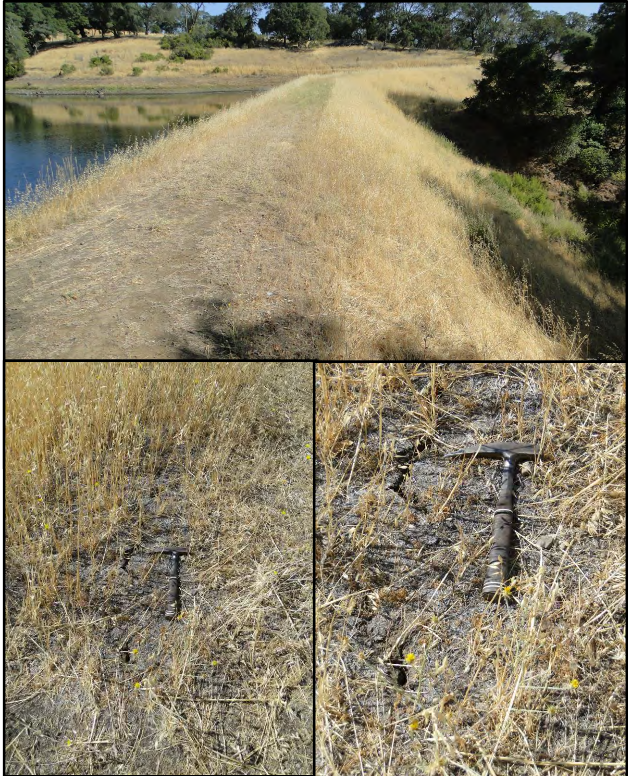
Figure F-10: Photographs of Municipal Dam and longitudinal cracks observed along the downstream edge of the crest of Municipal Dam [NSF-GEER; Napa, CA; N38.298 W 122.144; Harder, L. F.; 08/27/14]
