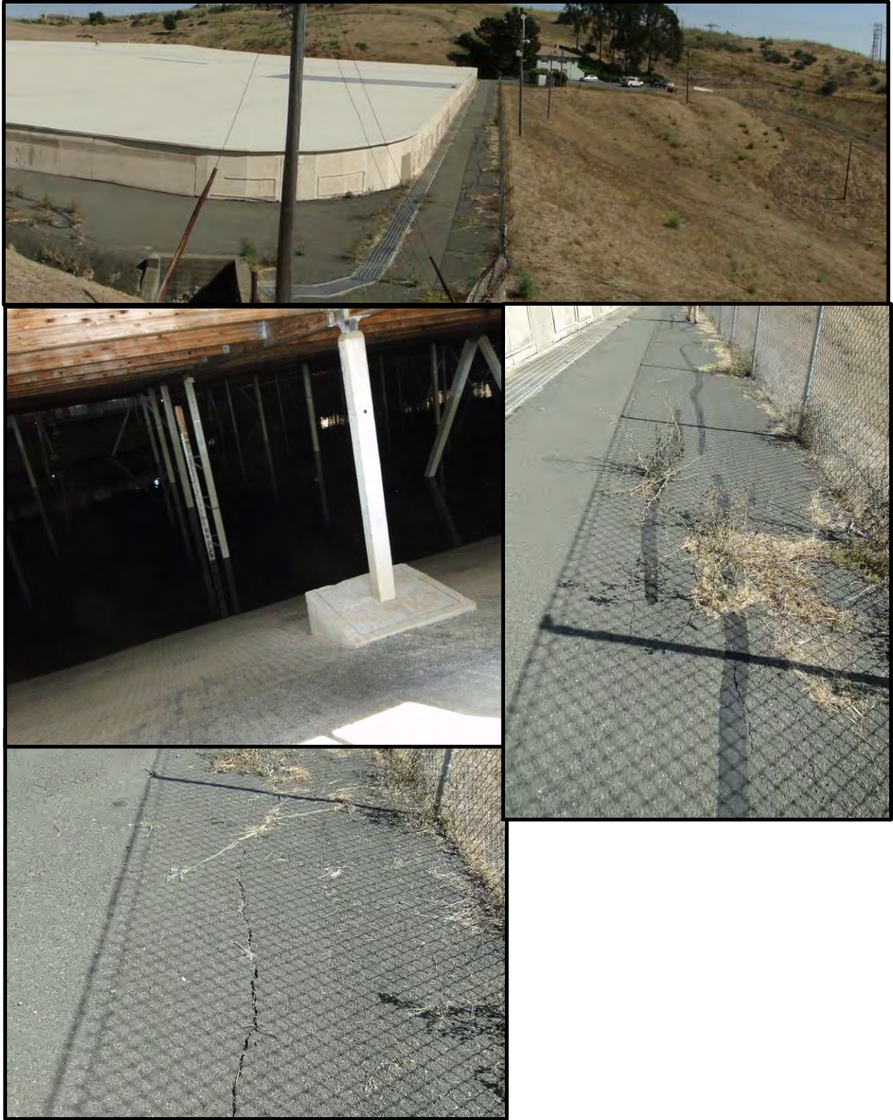
Figure F-13: Photographs of Swanzy Dam and minor longitudinal cracking [NSF-GEER; Napa, CA; N38.077 W 122.227; Harder, L. F.; 08/27/14]
