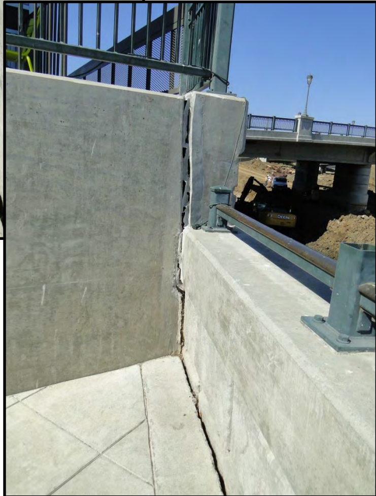
Figure F-19: Separation of concrete slab and retaining wall from Napa River floodwall along right bank of Napa River looking upstream from Third Street Bridge [NSF-GEER; Napa, CA; N38.299 W 122.285; Harder, L. F.; 09/04/14]
