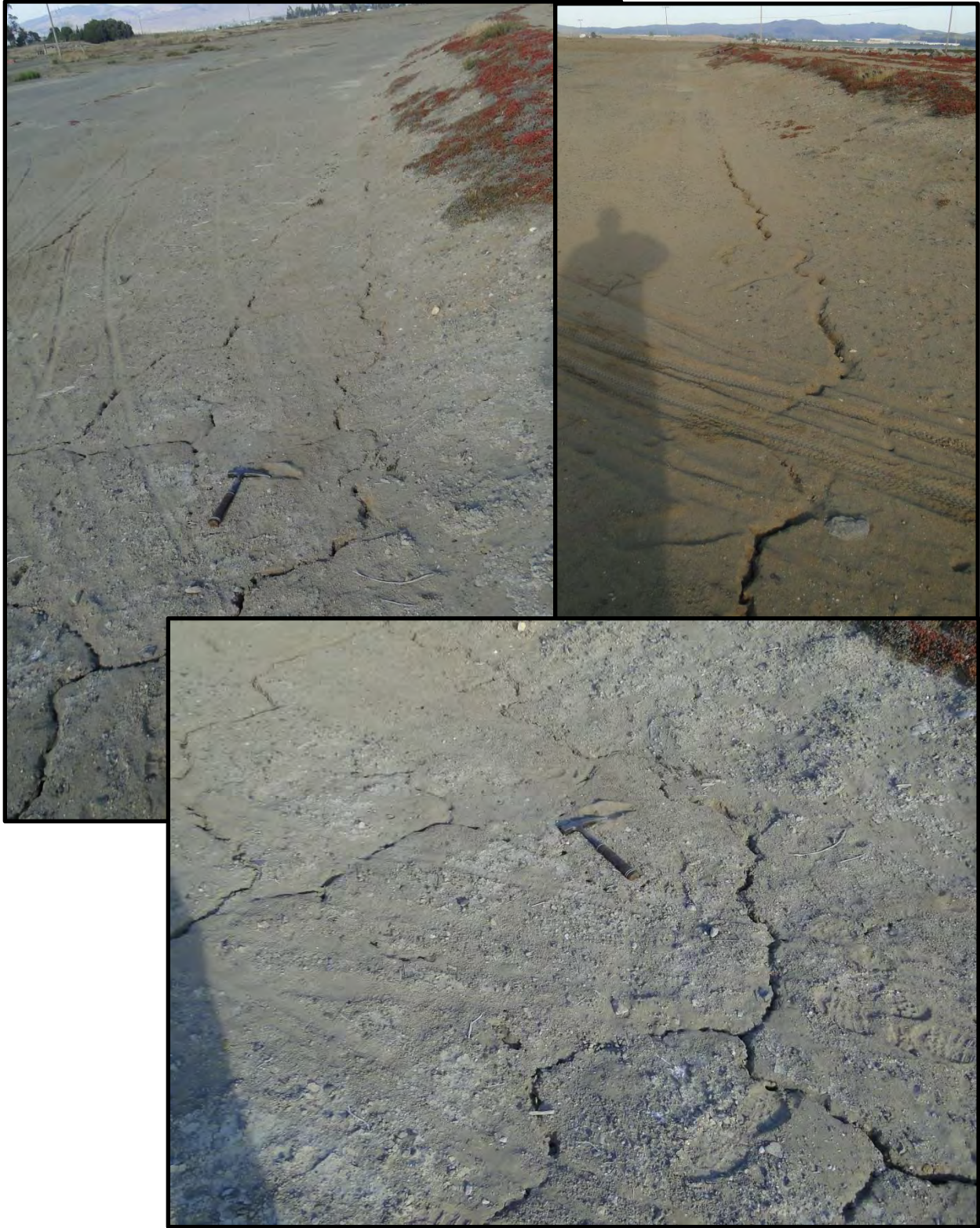
Figure F-23: Photographs of longitudinal cracking and apparent ejecta along landside toe of salt pond retaining dike on western edge of Green Island south of the epicenter [NSF-GEER; Napa, CA; N38.201 W 122.302; Harder, L. F.; 09/04/14]
