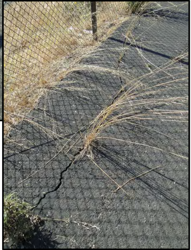
Figure F-9: Photographs of pre-existing longitudinal cracks on the crest of the maximum section of Summit Reservoir Dam [NSF-GEER; Napa, CA; N38.153 W 122.225; Harder, L. F.; 08/27/14]
