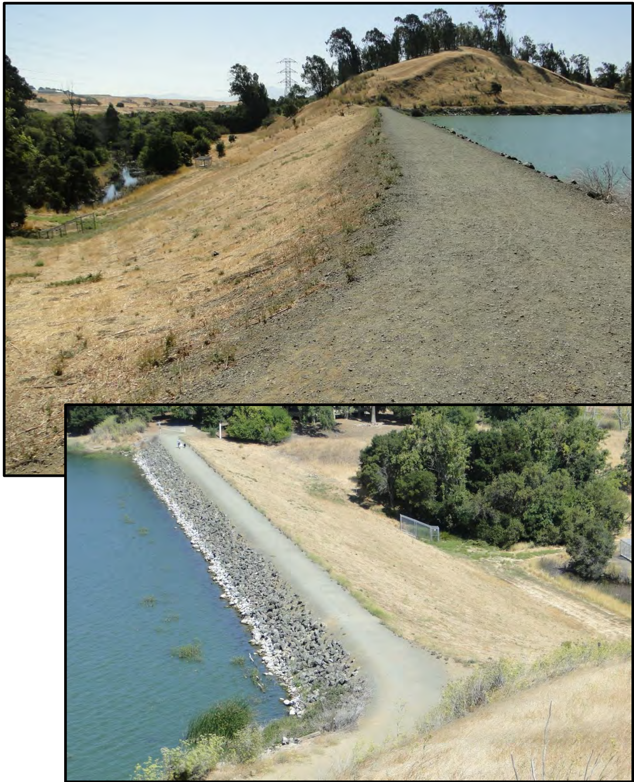
Figure F-14: Photographs of Lake Herman Dam [NSF-GEER; Napa, CA; N38.097 W 122.150; Harder, L. F.; 08/27/14]
