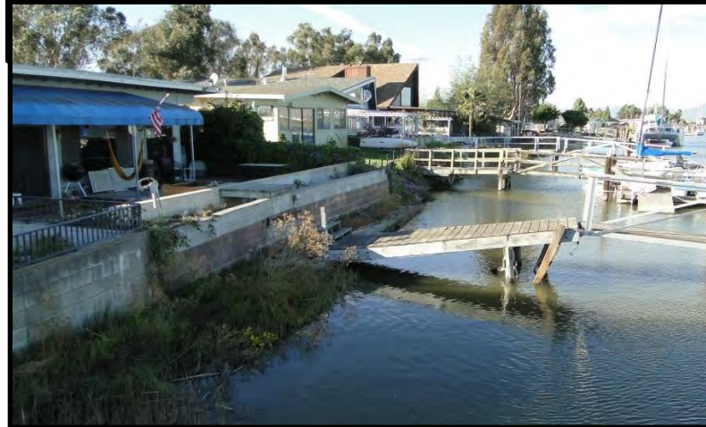
Figure F-21: Photographs of cracked asphalt pavement on Milton Road, cracked cinderblock retaining wall, and damage to waterside floodwall/boat dock on Edgerley Island south of the epicenter [NSF-GEER; Napa, CA; N38.198 W 122.316; Harder, L. F.; 09/01/14]
