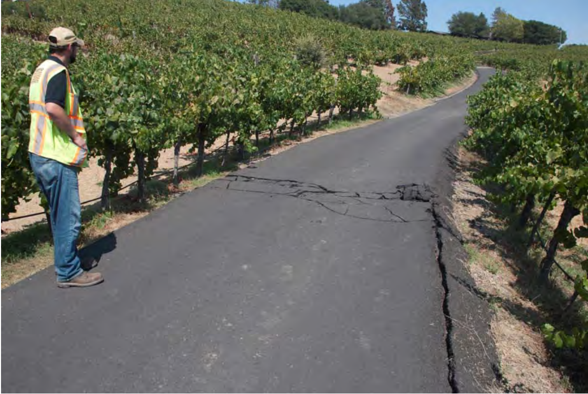
Figure 3-12. Shattering of asphalt along southern part of eastern strand on driveway near Thompson Road. Rupture was difficult to see in soil on either side of driveway, but obvious on asphalt. Right-lateral offsets were around 5 cm in this area, although difficult to measure at this location [GEER-NSF; GPS: 38.2866°, -122.3259°; 8/25/2014].
