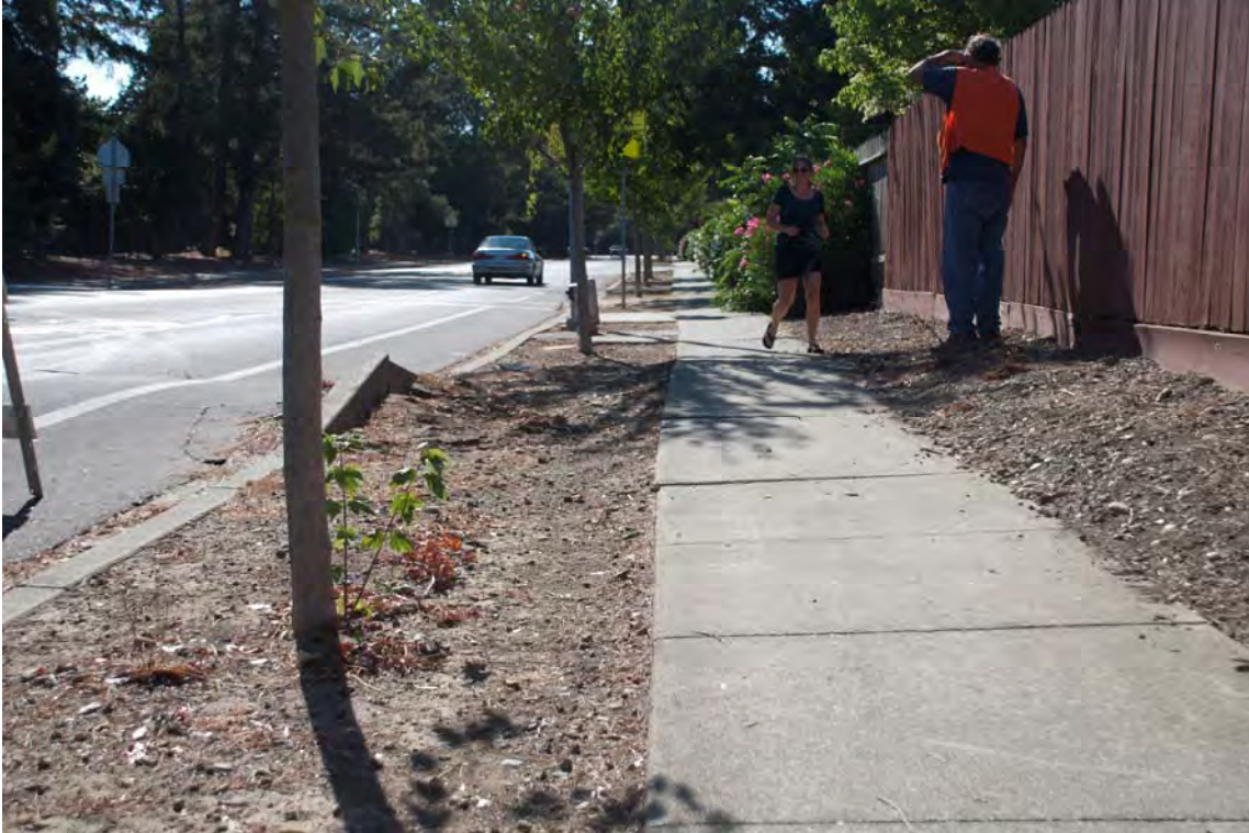
Figure 3-10. Surface rupture forming moletrack on asphalt road, tented concrete curb and displaced sidewalk in right-lateral sense on Partrick Road along eastern strand of the surface rupture. Right-lateral offset is on the order of between 5 - 10 cm. [NSF-GEER; GPS 38.3069°, -122.3374°; 08/24/2014]
