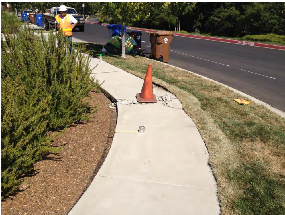
Figure 5.7: Crushed section in pavement parallel to fault with compression features in curb strip perpendicular to fault, across from creek [NSF-GEER; N 38.3055 W 122.3467; 8/28/2014 14:30]
