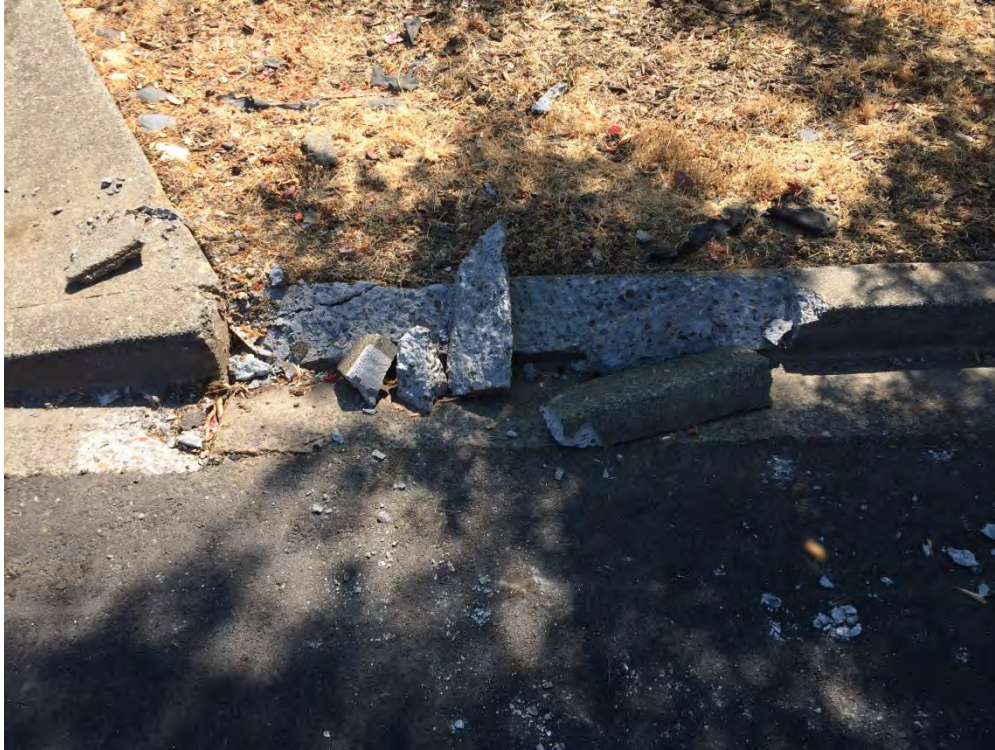
Figure 5.11: Crushed curb perpendicular to fault trace [NSF-GEER; N 38.3035 W 122.3411; 8/25/2014 14:47]
