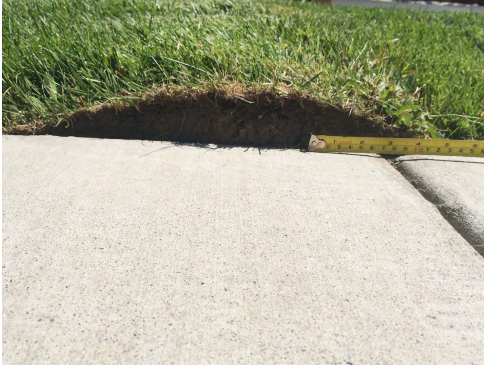
Figure 5.8: Compression feature in curb strip perpendicular to fault, across from creek [NSF-GEER; N 38.3065 W 122.3455; 8/28/2014 13:52]
