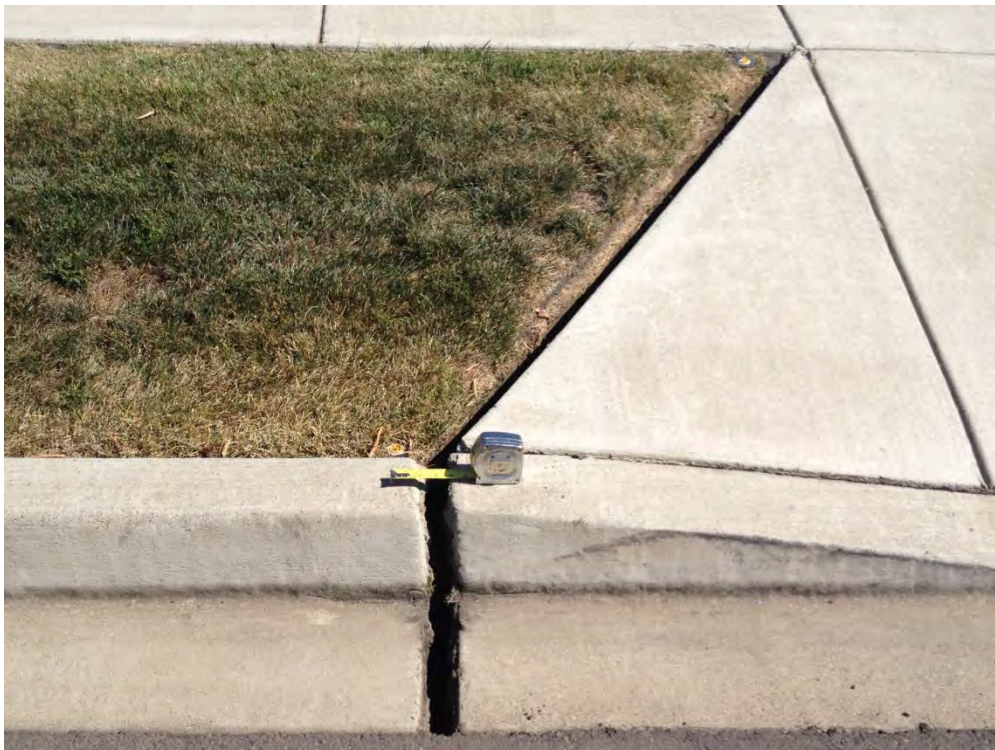
Figure 5.12: Extension crack in curb parallel to fault trace [NSF-GEER; N 38.3066 W 122.3475; 8/28/2014 15:08]
