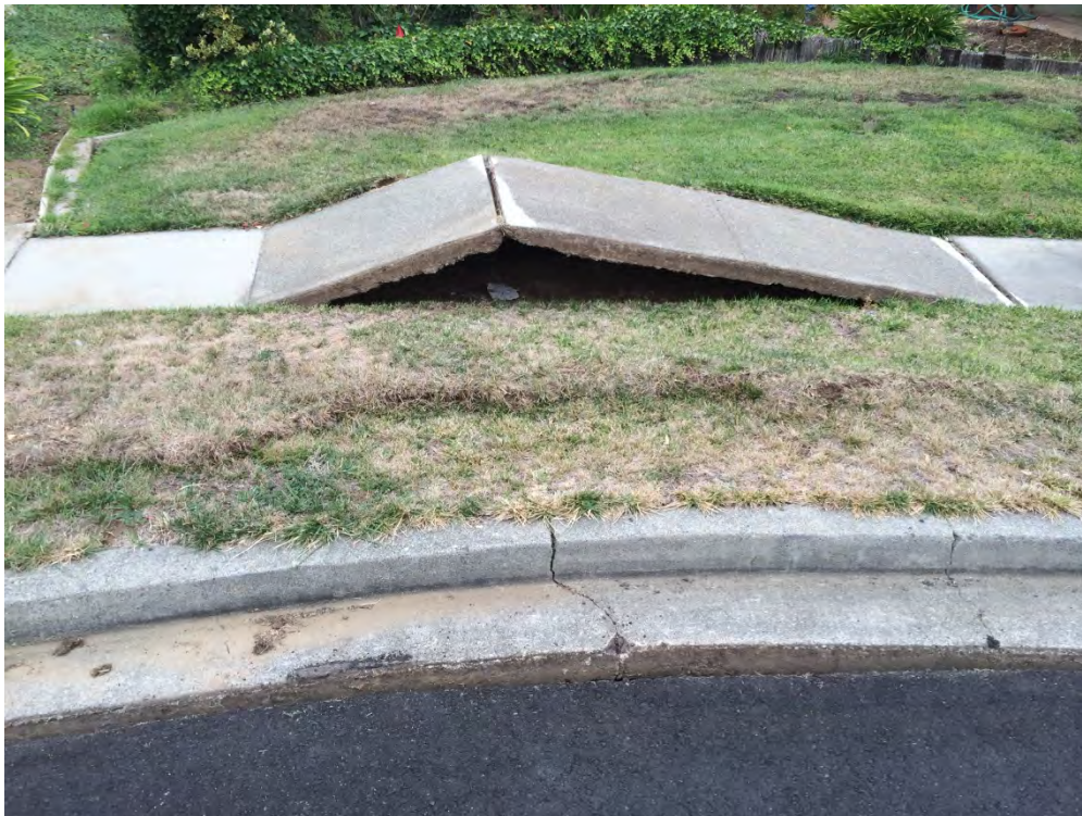
Figure 5.9: Buckled section in pavement perpendicular to fault with compression features in curb strip and lawn parallel to fault, near observed fault trace [NSF-GEER; N 38.3018 W 122.3439; 8/25/2014 10:38]
