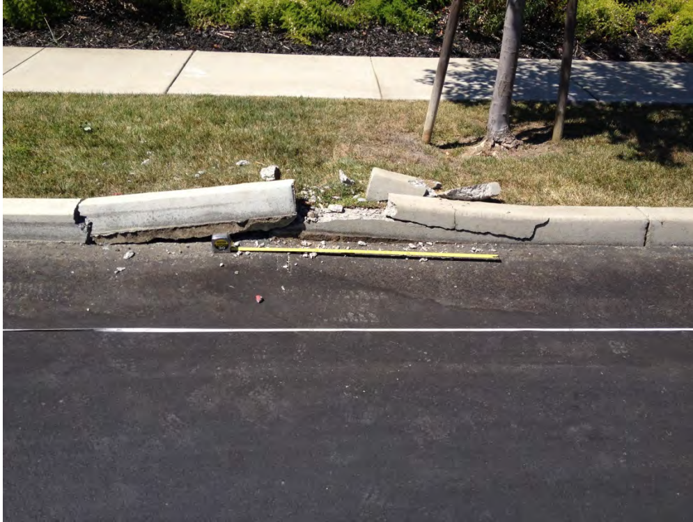
Figure 5.13: Buckled curb parallel to fault trace [NSF-GEER; N 38.3073 W 122.3443; 8/28/2014 13:41]
