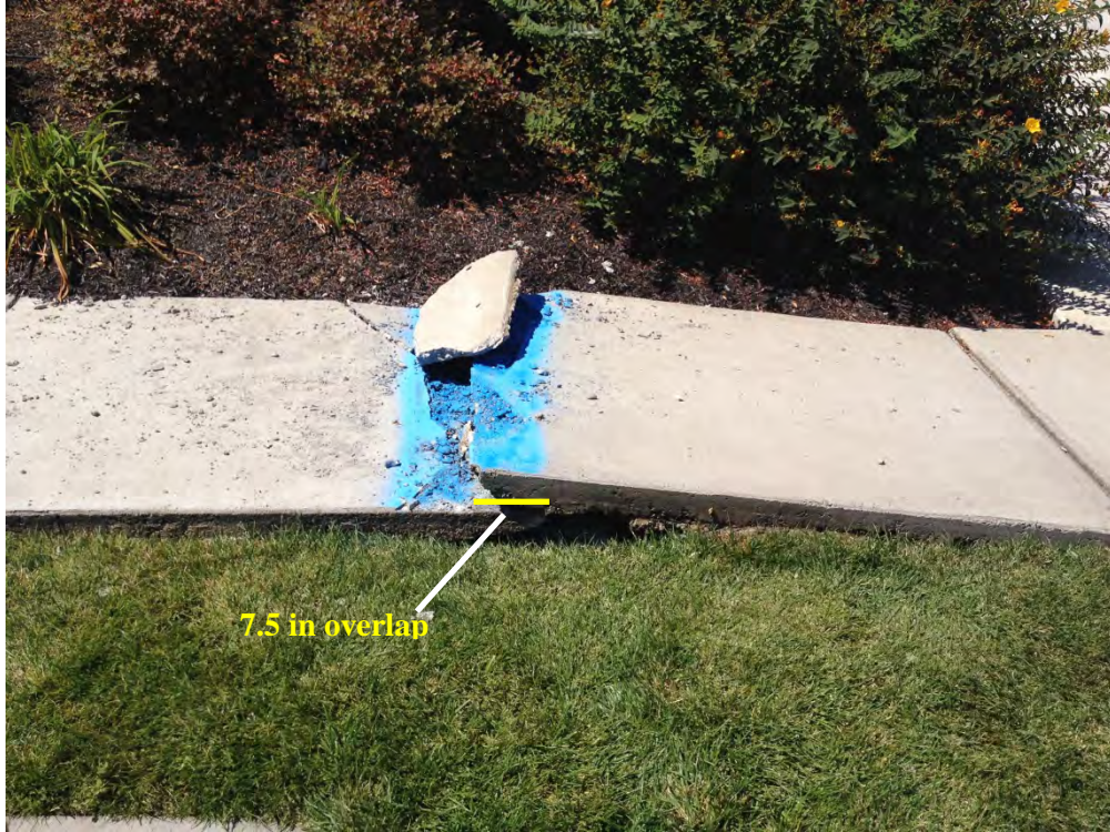
Figure 5.4: Measuring an overlapped compression zone in sidewalk pavement [NSF-GEER; N 38.3065 W 122.3454; 8/28/2014 14:00]
