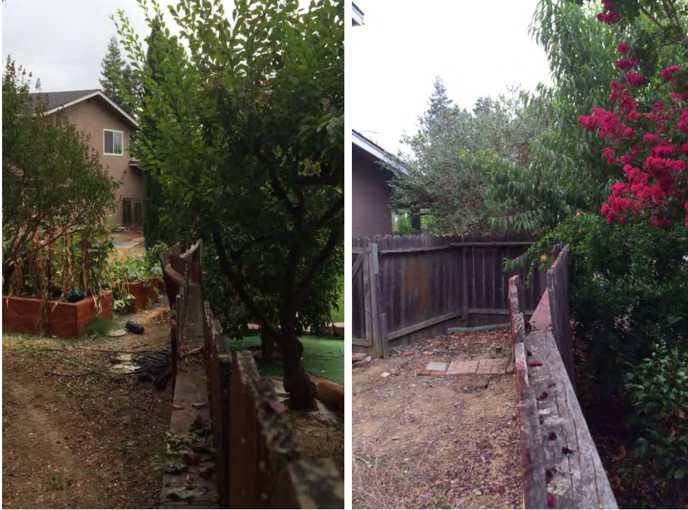
Figure 5.14: Buckled section of fence of the surveyed fence [NSF-GEER; N 38.3015 W 122.3442; 8/25/2014 09:57]
