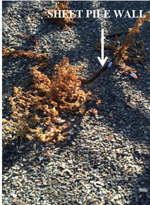
Figure 6.10: Crack along sheet pile wall behind the retaining wall in the Pedestrian Bridge [NSF-GEER; N 38.3003 W -122.2881; 08/24/14 17:58]
