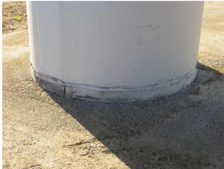
Figure 6.2: Highway 37 Bridge pier with no significant ground damage; [NSF-GEER; Mare Island, Vallejo, CA; GPS N38.122 W122.276; 08/24/14; 18:24]
