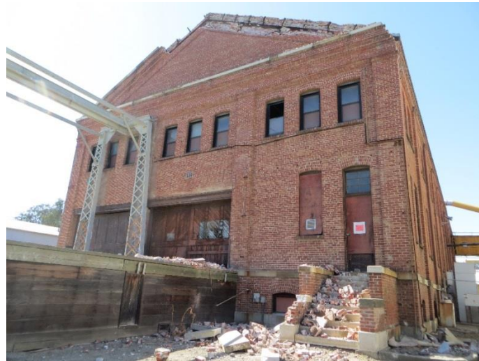
Figure 6.4: Brick facade damage; [NSF-GEER; Mare Island, Vallejo, CA; N38.095 W122.268; 08/24/14; 15:38]
