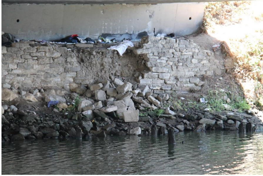
Figure 6.6: Failure of masonry retaining wall below the south abutment of Soscol Bridge [NSF-GEER; N 38.2997 W -122.2834; 08/24/14 13:09]
