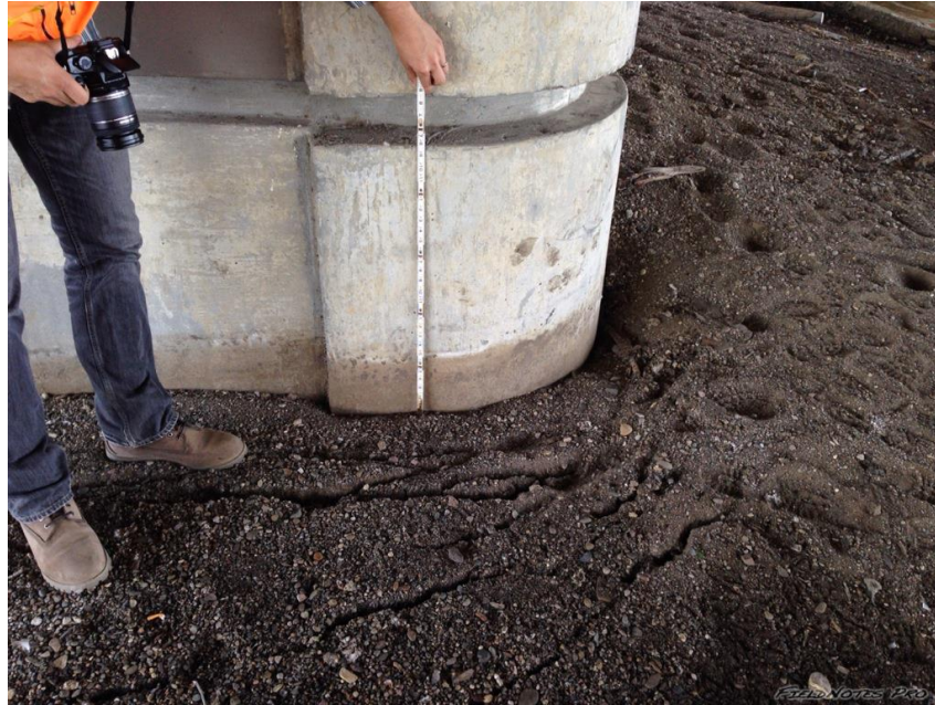
Figure 6.9: Ground cracking and settlement due to liquefaction in Napa River point bar below 3 rd St. Bridge [NSF-GEER; N 38.2980 W -122.2840; 08/24/14 14:44]
