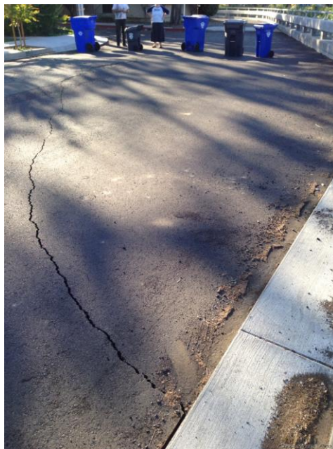
Figure 6.11: Crack in pavement behind the retaining wall in the pedestrian bridge [NSF-GEER; N 38.3003 W -122.2881; 08/24/14 17:58]
