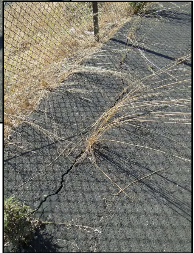
Figure 7-9: Photographs of pre-existing longitudinal cracks on the crest of the maximum section of Summit Reservoir Dam [NSF-GEER; Napa, CA; N38.153 W 122.225; Harder, L. F.; 08/27/14]
