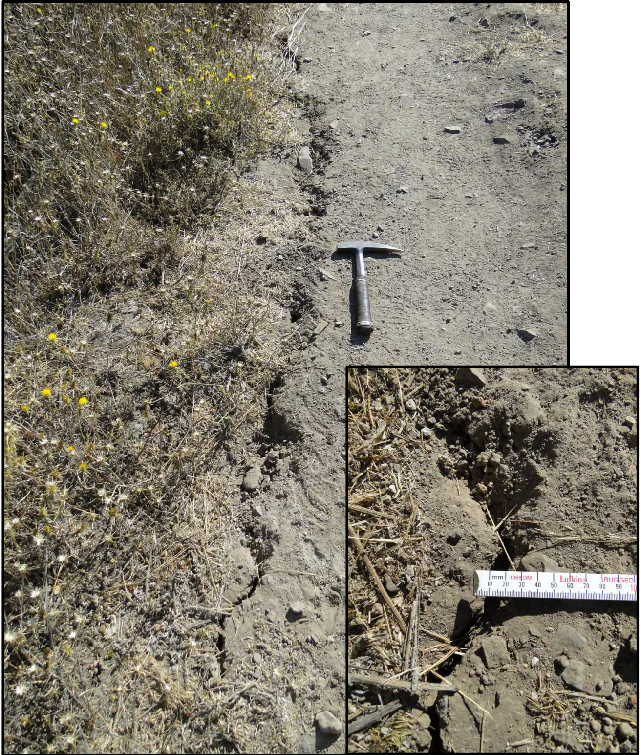
Figure 7-4: Photograph of longitudinal cracking on the upstream edge of the crest of Lake Marie Dam looking southeast [NSF-GEER; Napa, CA; N38.260 W 122.230; Harder, L. F.; 09/01/14]
