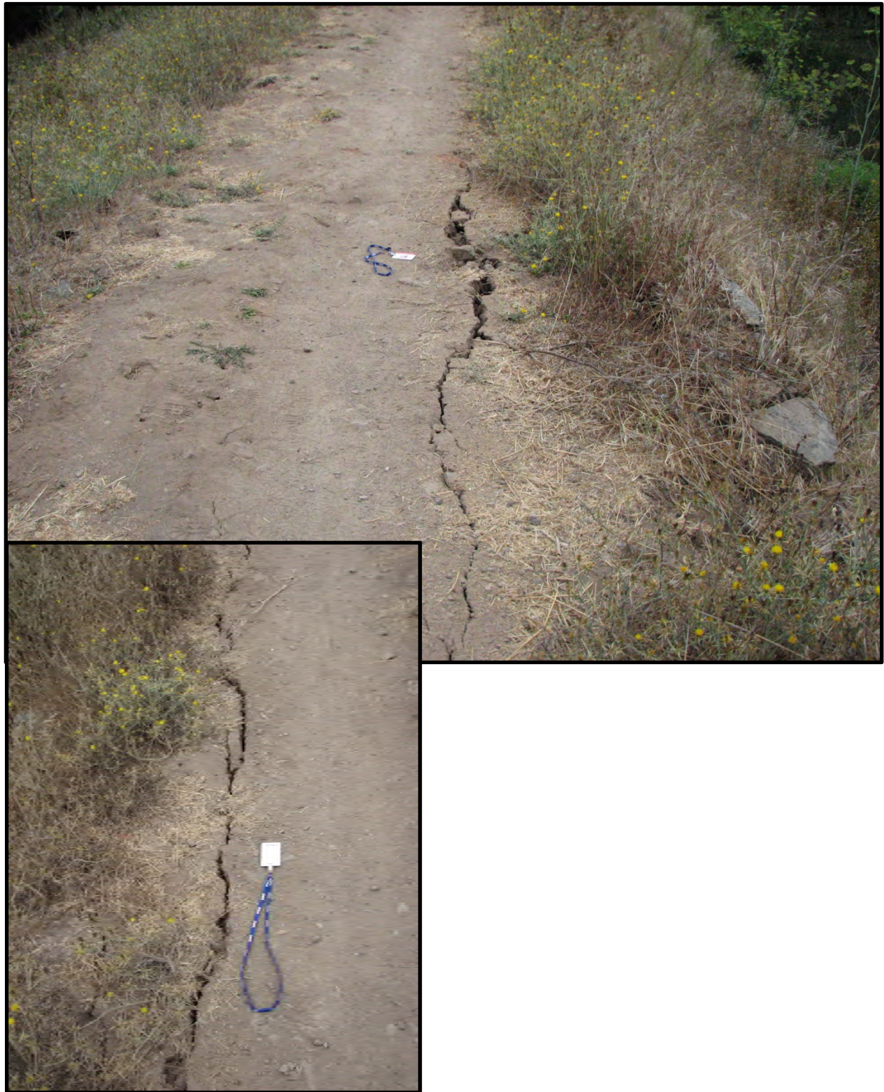
Figure 7-3: Photographs of longitudinal cracking on the upstream edge of the crest of Lake Marie Dam [Napa, CA; N38.260 W 122.230; from DSOD files; 08/24/14]
