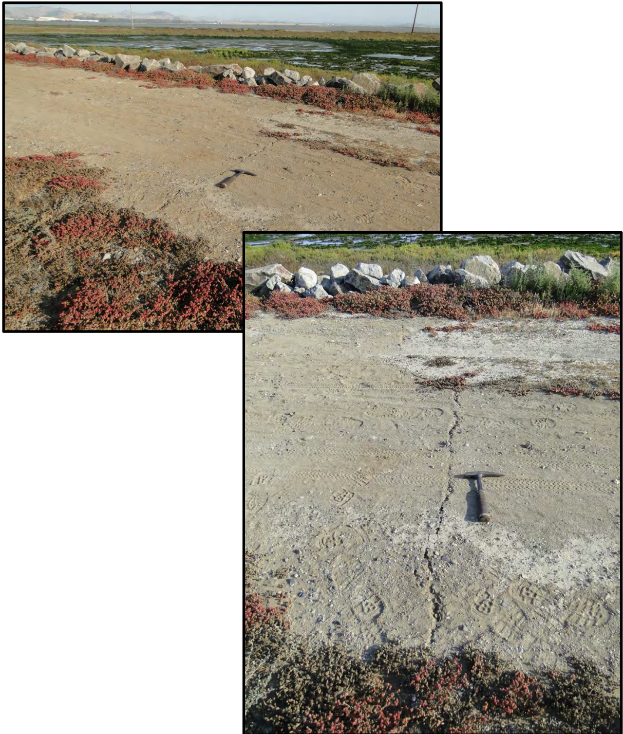
Figure 7-19: Photographs of transverse cracking on crown of salt pond retaining dike on western edge of Green Island south of the epicenter [NSF-GEER; Napa, CA; N38.201 W 122.302; Harder, L. F.; 09/04/14]
