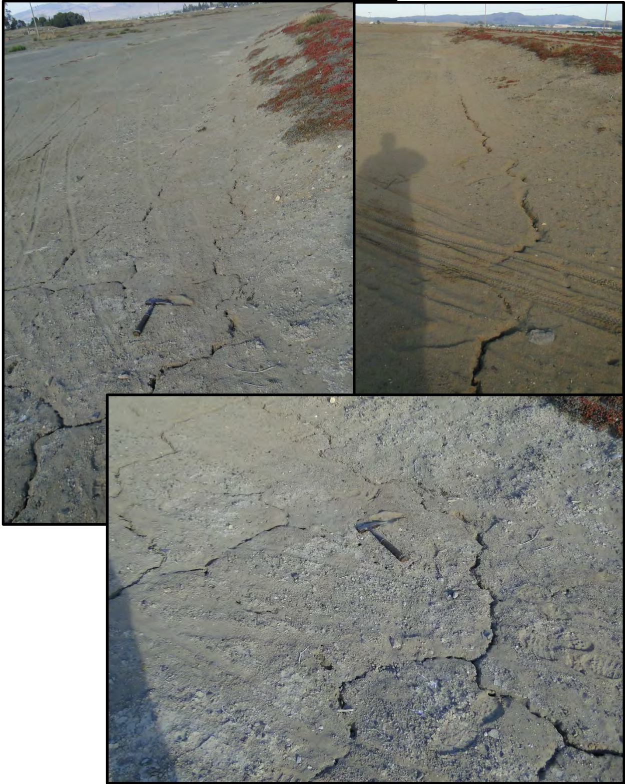
Figure 7-18: Photographs of longitudinal cracking and apparent ejecta along landside toe of salt pond retaining dike on western edge of Green Island south of the epicenter [NSF-GEER; Napa, CA; N38.201 W 122.302; Harder, L. F.; 09/04/14]
