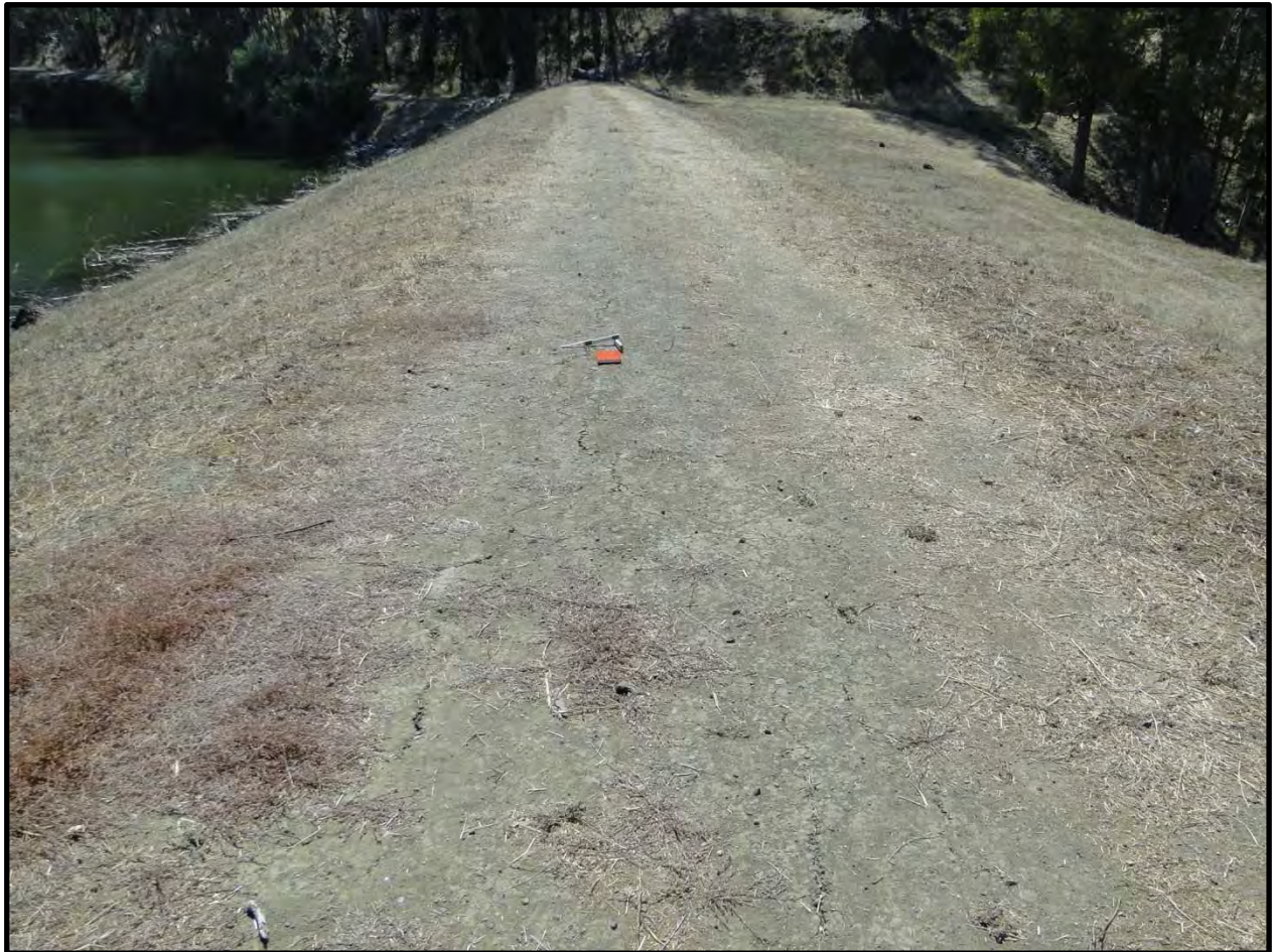
Figure 7-6: Photograph of minor longitudinal cracking on the crest of Lake Chabot Dam looking southeast [NSF-GEER; Napa, CA; N38.141 W 122.241; Harder, L. F.; 08/27/14]
