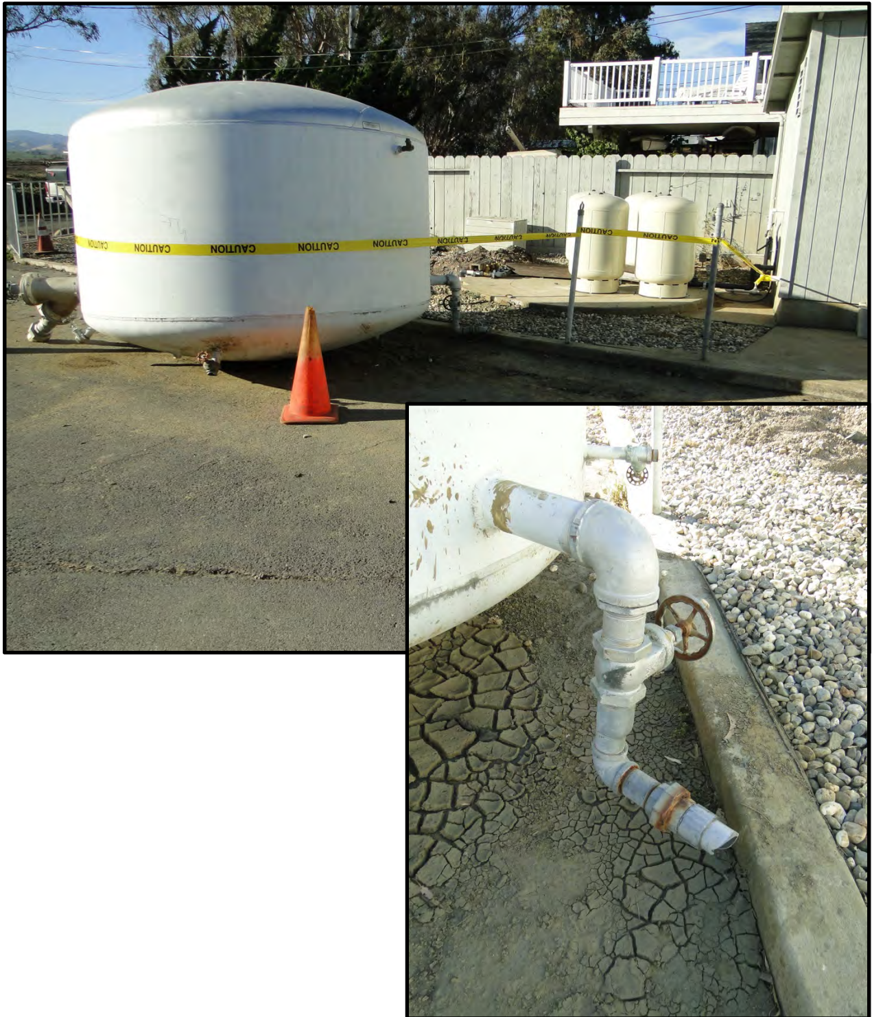
Figure 7-17: Photographs of displaced water tank moved off its concrete pad and sheared pipe connection – note replacement tanks on pad in its place - on Edgerley Island south of the epicenter [NSF-GEER; Napa, CA; N38.198 W 122.316; Harder, L. F.; 09/01/14]
