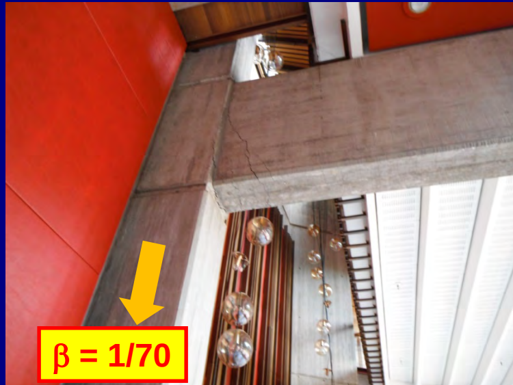
Cracking due to Differential Settlement
